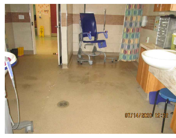
PIC. 6 EX. SHOWER AREA
