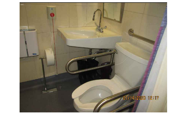
PIC. 3 EX. SINK & TOILET
