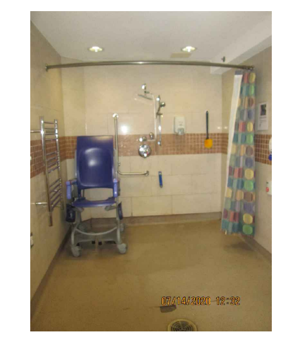
PIC. 8 EX. SHOWER AREA
