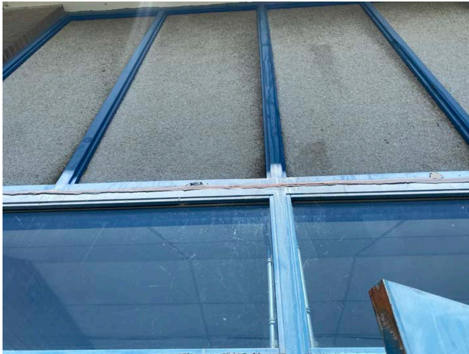
Photograph 1: View of the asbestos-containing cladding panels (cement board) above the window at Entrance 11 at the Subject Location.
