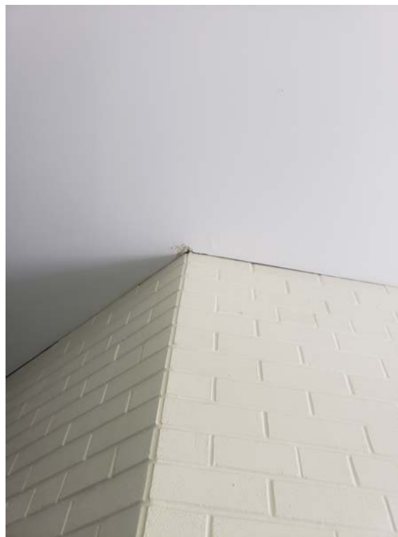
Photograph 2: View of the asbestos-containing drywall joint compound on the ceiling in the vestibule by Entrance 33 at Subject Location.
