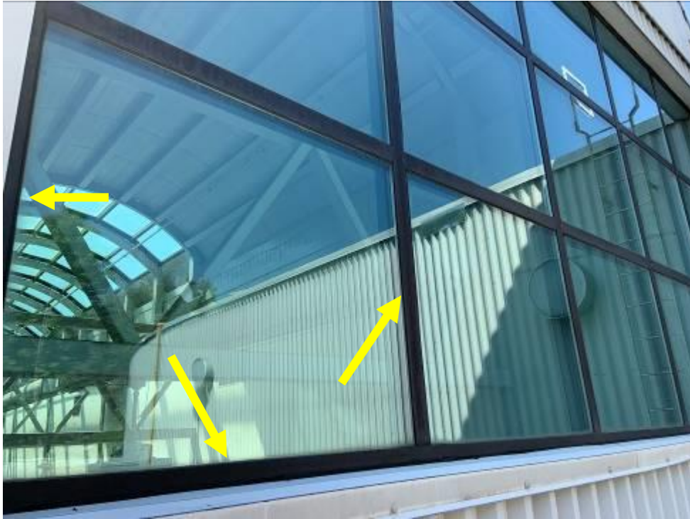
Photo 1: Asbestos-containing black putty along the joints of the interior and exterior glass and the skylight frames, in Construction Area 5.
