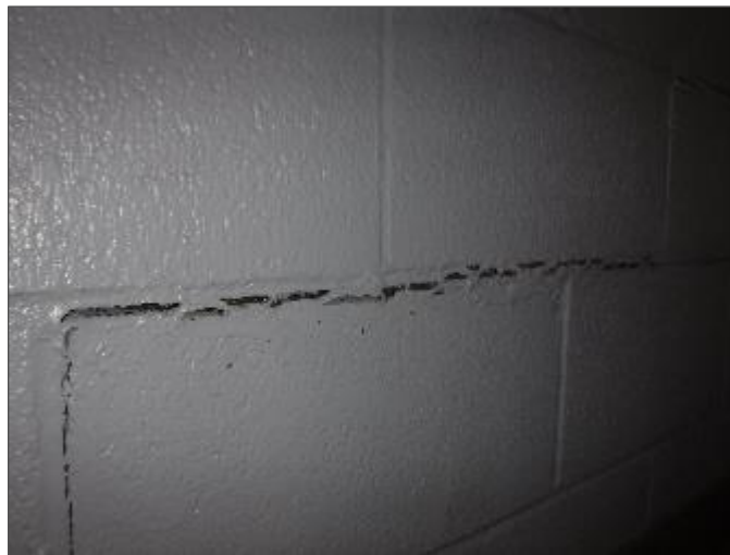
Photo 6 - Non-asbestos vermiculite is coming out of cracks in the concrete block wall.
