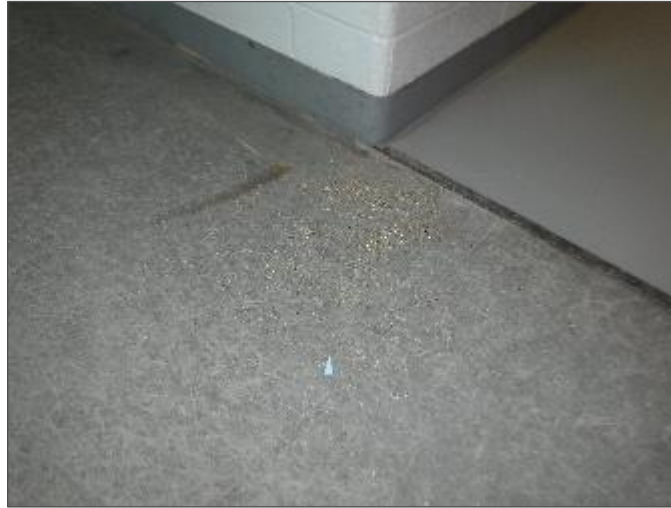
Photo 5 - Non-asbestos vermiculite in from the Hallway around the Ice Rink (Location 1-25).
