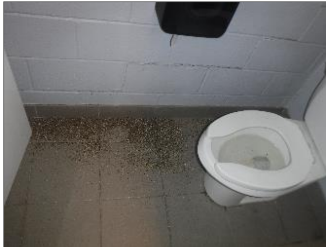
Photo 1 - Non-asbestos vermiculite in the Washroom (Location 1-22).
