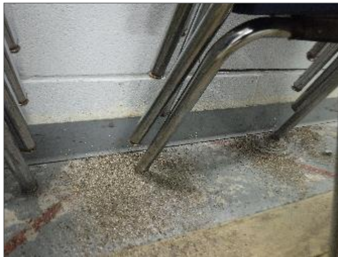
Photo 4 - Non-asbestos vermiculite in from the Hallway around the Ice Rink (Location 1-25).
