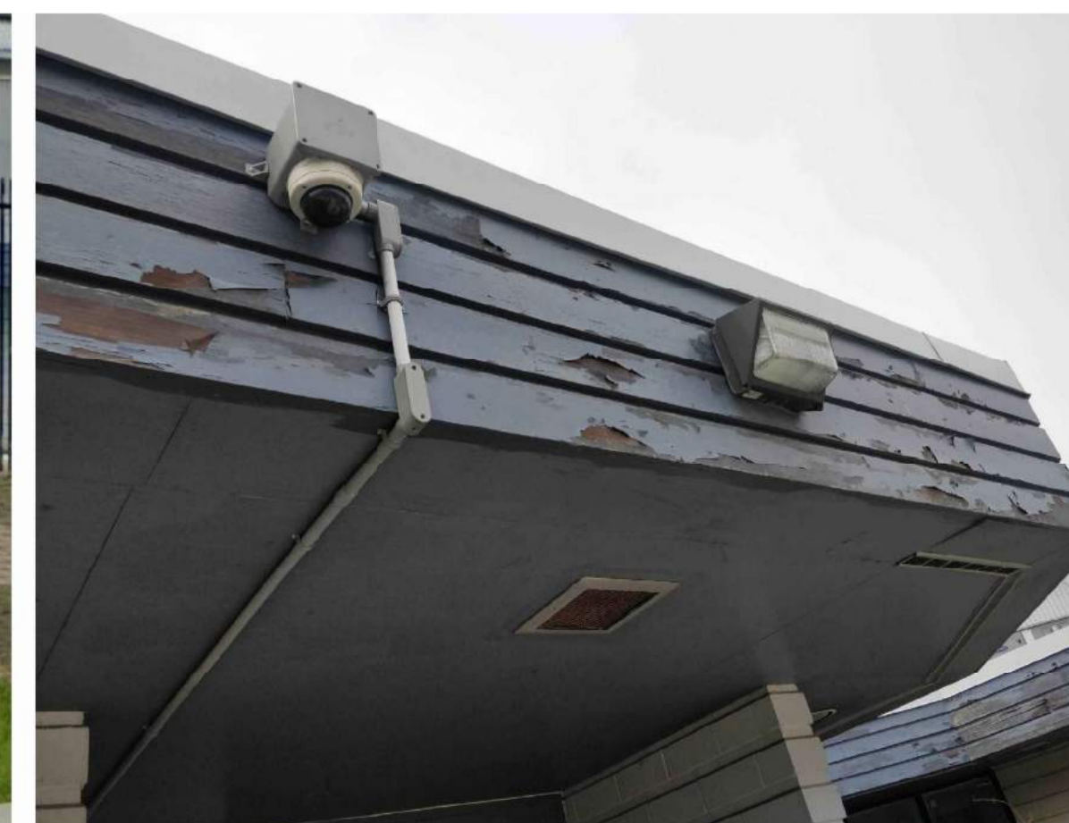
FACADE, VENT, LIGHTS & SOFFIT TO BE REPLACED
