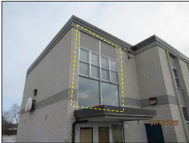
Photograph 1: Overall view of W1 window (2 total) in the stairwell landing to be replaced.
