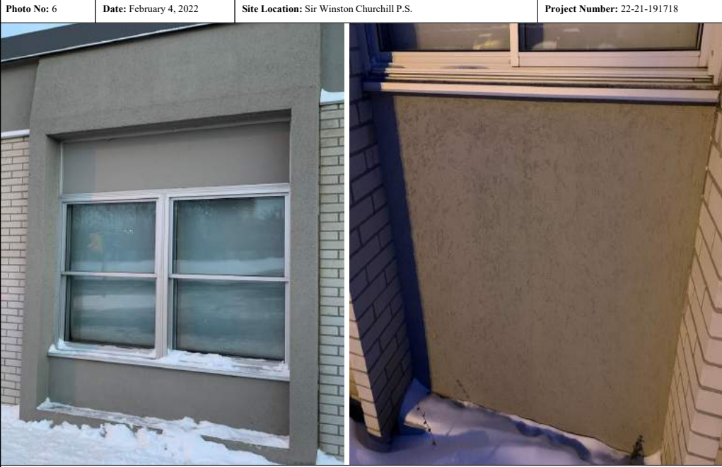
Description: Typical locations where textured/decorative plaster finishes were observed and sampled. These materials did not contain asbestos.
