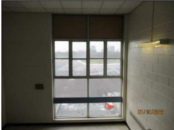
Photograph 11: At the landing adjacent to W1 Windows, remove and dispose of existing wood guard and install new engineered metal railing meeting current requirements of the OBC.
