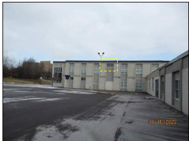
Photograph 10: Typical W10 windows (2 total) to be replaced. Glazing is to be opaque.
