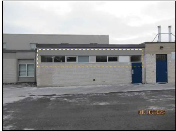
Photograph 2: Typical W2 windows (2 total) to be replaced. Glazing is to be opaque.
