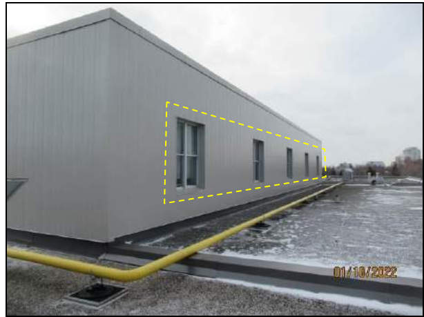
Photograph 4: Typical W4 windows (clerestory; 10 total) to be replaced. These windows are on the 2 nd storey of the building and accessed from the roof and the double height gym.
