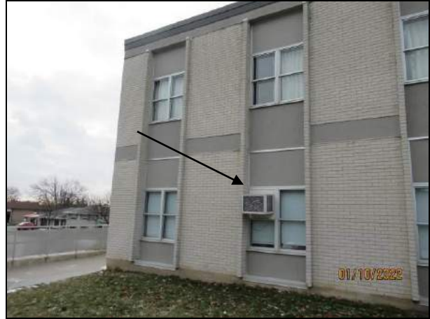
Photograph 12: AC unit for 1 st floor Window W5 on the east elevation to be removed, temporarily stored, and reinstated following installation of new W5 window assemblies. New bracket is to be provided for the AC unit.
