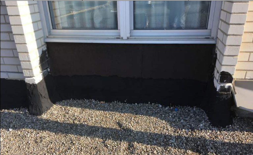
Description: Typical location where black mastics and brown sealants were observed in the December 2019 Report. These materials did not contain asbestos.
