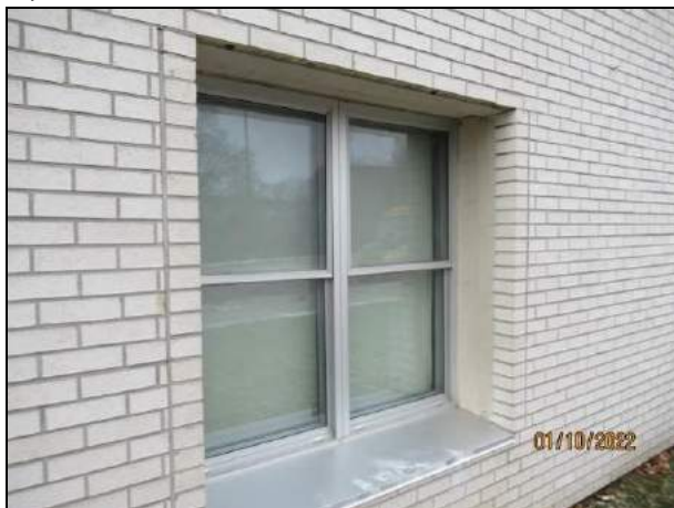
Photograph 9: One (1) W9 window on the 1 st floor, east elevation to be replaced. New aluminum trim is to be provided at the jambs and head to cover the painted portion of the wall.
