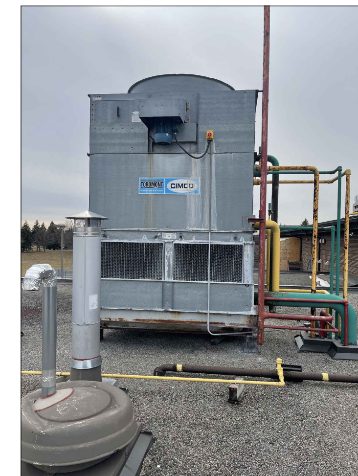
PHOTO#1: EXISTING ROOF TOP EVAPORATIVE CONDENSER, TO BE REMOVED AND REPLACED.
