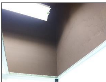
Brown paint on drywall containing low levels of lead
