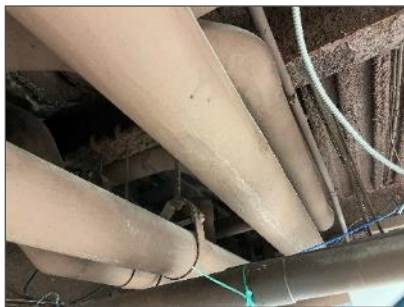
Asbestos-containing parging cement present on pipe elbows
