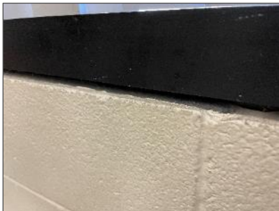
Asbestos-containing cream paint on masonry block
