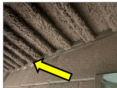
Non-asbestos firestopping present at pipe and conduit penetrations
