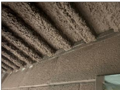
Asbestos-containing sprayed fireproofing present in metal deck and structural steel
