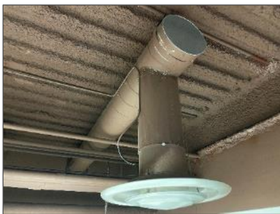
Asbestos-containing sprayed fireproofing present in metal deck and structural steel
