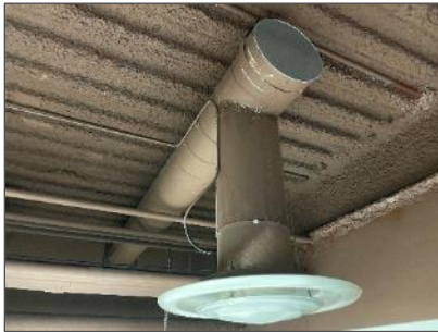
Duct work with asbestos-containing sprayed fireproofing overspray
