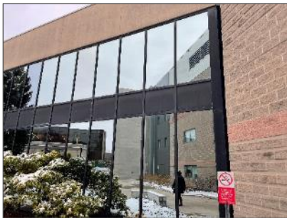
Non-PCB black butyl sealant on exterior windowpanes
