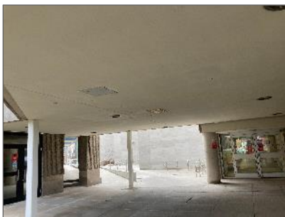
Non-asbestos brown mastic associated with fibreglass insulation present above drywall soffit
