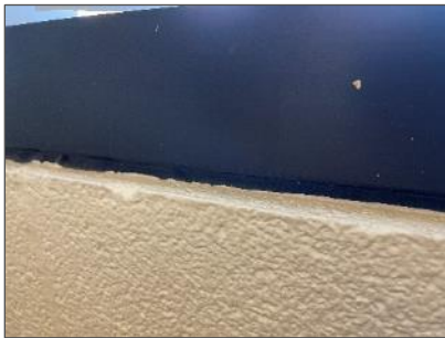
Non-PCB caulking on window frames
