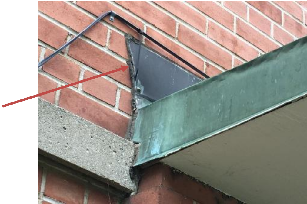
Photo 1: Non-Friable exterior white (weathered) caulking was confirmed to contain 2% Chrysotile Asbestos (DST Sample ID A-150-02A-C). The material was observed on the south entrance canopy.
