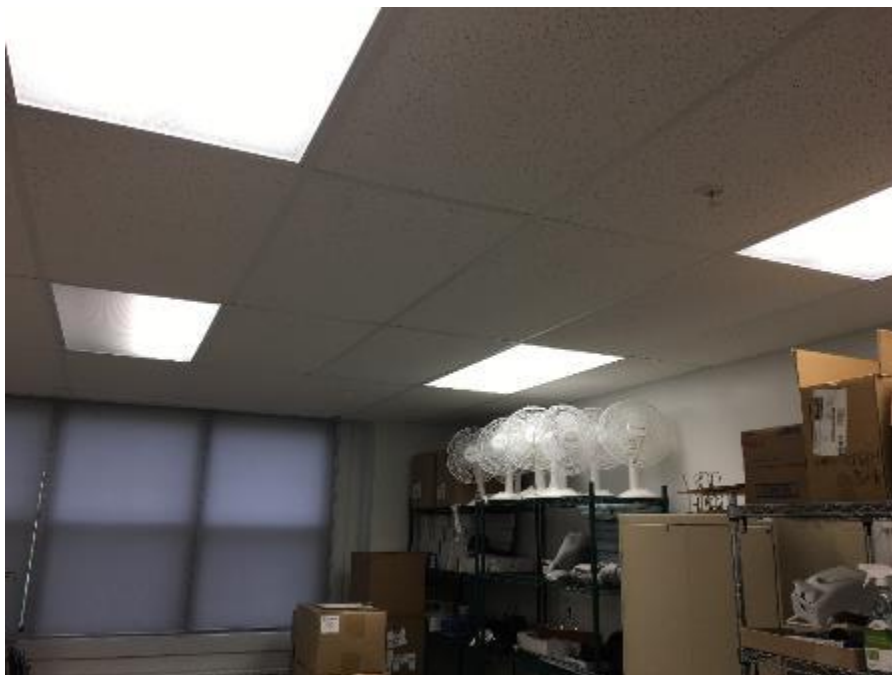
Photo 6: 2' x 4' Acoustic Ceiling Tile, pinhole and fissures confirmed to not contain asbestos (recent manufacture date stamp).
