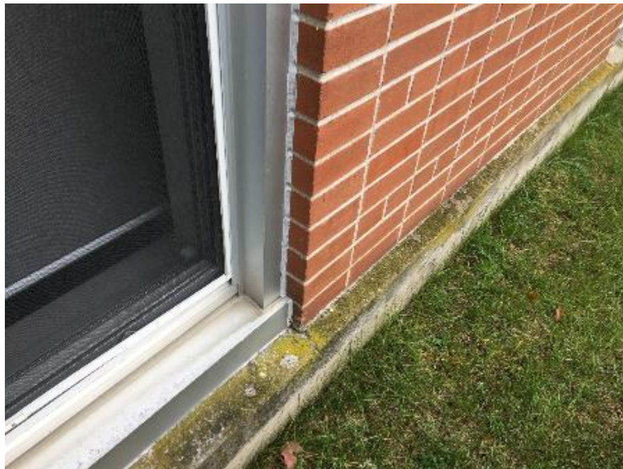
Photo 2: Non-Friable exterior grey window caulking was confirmed to contain 10% Chrysotile Asbestos (DST Sample ID A-150-03A-C).
