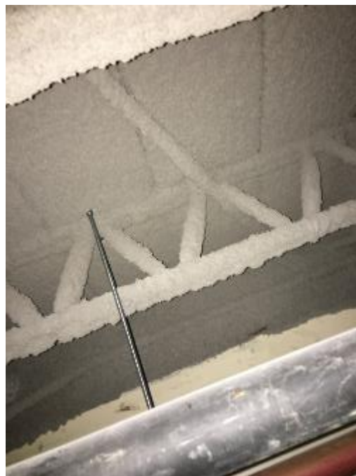
Photo 4: Fireproofing, observed in Corridor 138, was confirmed to not contain asbestos (DST Sample ID A-150-05A-C).
