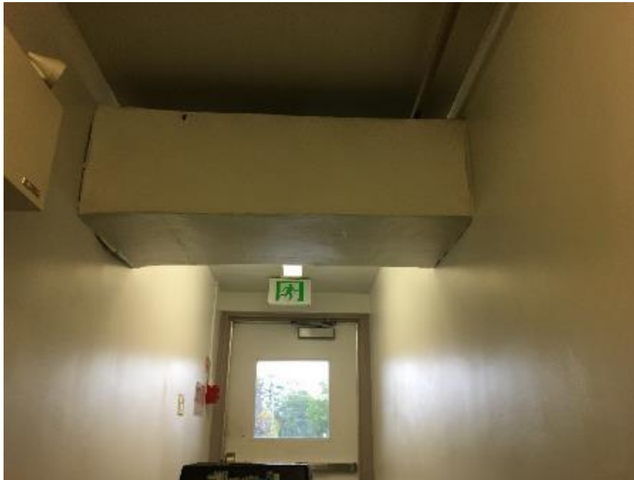
Photo 5: Friable paring cement within canvased duct seams confirmed to contain 60% Chrysotile asbestos, sampled in Corridor 140 (Maple Sample ID 12233-S-06A).
