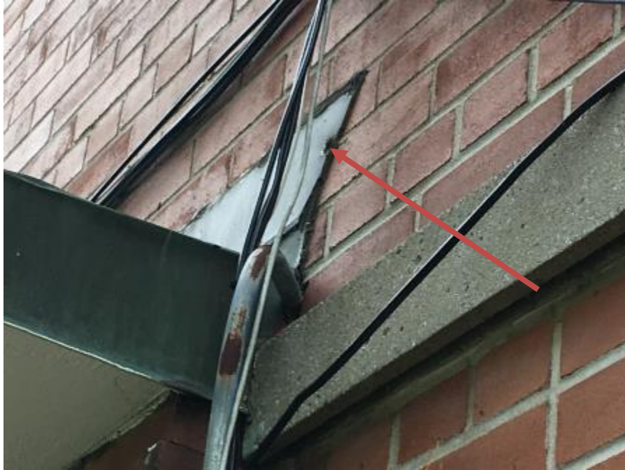
Photo 3: Exterior brown caulking was confirmed to not contain asbestos (DST Sample ID A-150-04A-C).
