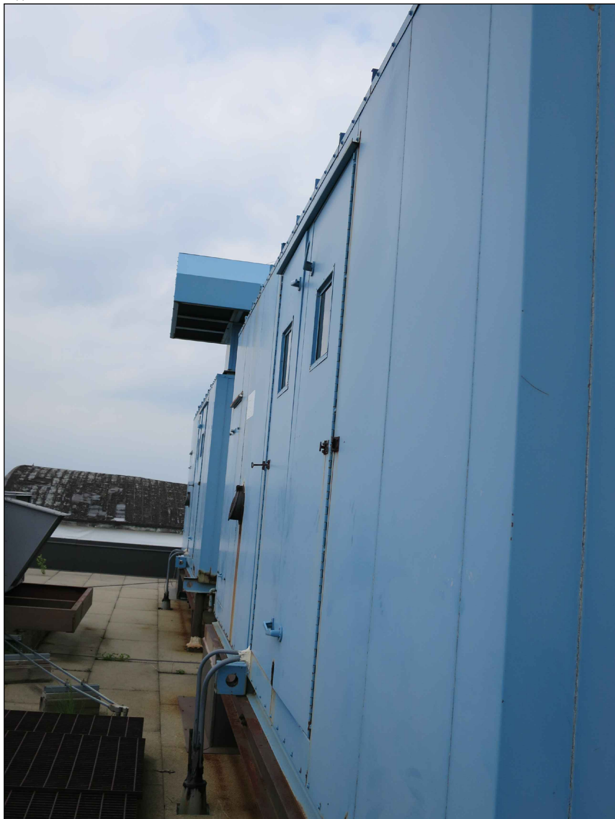
EXISTING ELECTRICAL ROOF PENETRATION
