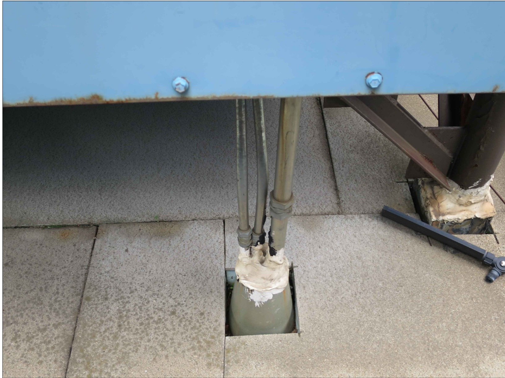
EXISTING ELECTRICAL ROOF PENETRATION
