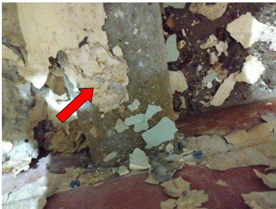
Photograph 5: View of the damaged (peeling and flaking) lead-containing multiple layer (green/off-white) paint on the wall in the basement sprinkler room at the Subject Location.
