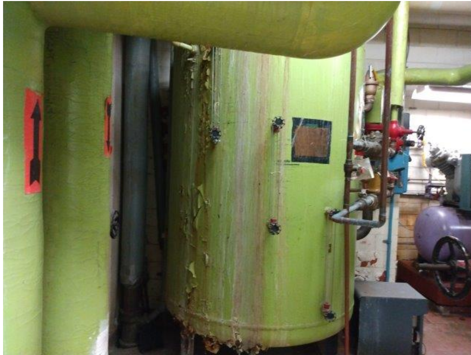
Photograph 7: View of the damaged (peeling and flaking) lead-containing light green paint on the mechanical systems insulation and on the tank in the boiler room 18 in the basement at the Subject Location.
