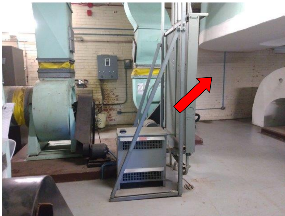
Photograph 1: View of the damaged (peeling and flaking) lead-containing light yellow paint on the brick wall in the west penthouse at the Subject Location.
