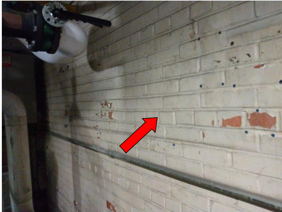
Photograph 3: View of the damaged (peeling and flaking) lead-containing light yellow paint on the brick wall in the east penthouse at the Subject Location.
