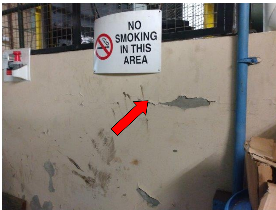
Photograph 2: View of the damaged (peeling) lead-containing light yellow paint on the concrete wall in the east penthouse at the Subject Location.
