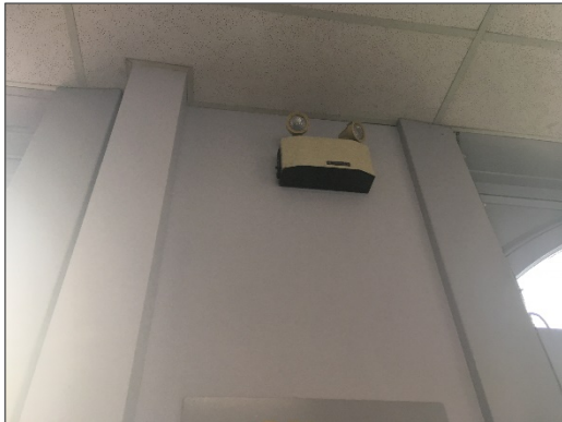
Lead-acid batteries within emergency lighting
