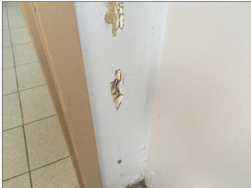
Visible mould growth around the door frame in the Women's Washroom, Location 3
