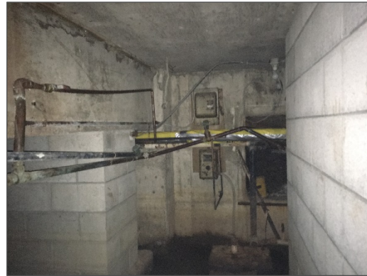
Presumed asbestos-containing pipe insulation within the crawlspace
