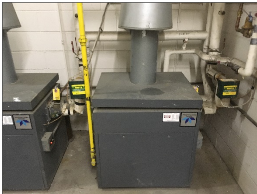
Furnace externally uninsulated
