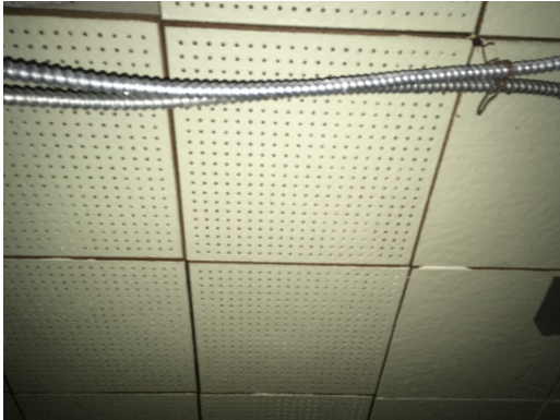
Non-asbestos grey textured plaster ceiling finish behind the 12"x12" order pinhole (wood fibre) ceiling tiles within the VIA OTS, Location 10
