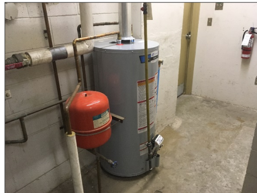
Hot water tank externally uninsulated
