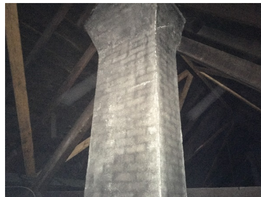
Non-asbestos plaster present on the chimney within the Attic, Location 15
