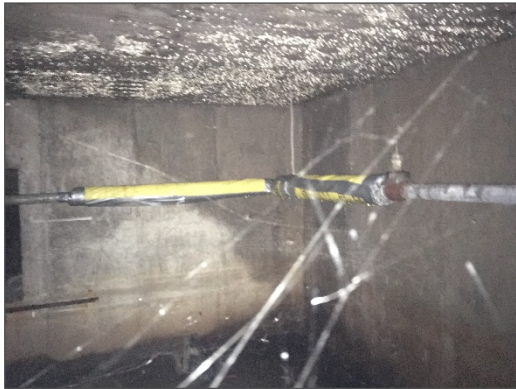
Presumed asbestos-containing pipe insulation within the crawlspace
