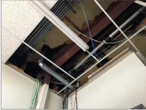
Photo 7 - Damaged hardboard ceiling in the baggage/server room
