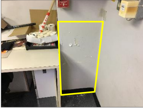
Photo 1 - Wet drywall in the ticket booth office.
