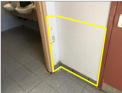
Photo 5 - Area of mould and water impacted drywall in the women's washroom
