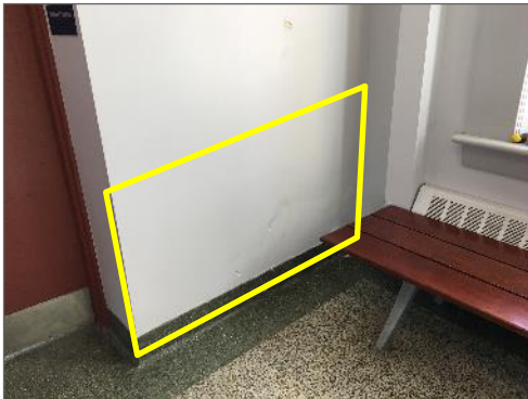
Photo 9 - Wet drywall in the waiting area adjacent to women's washroom
