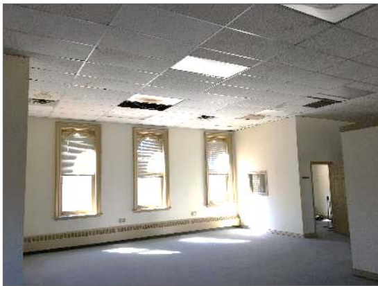
Photo 13 - Missing and water stained ceiling tiles in the open area
