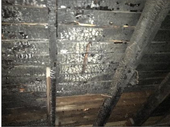
Photo 11 - Charred roof in attic
