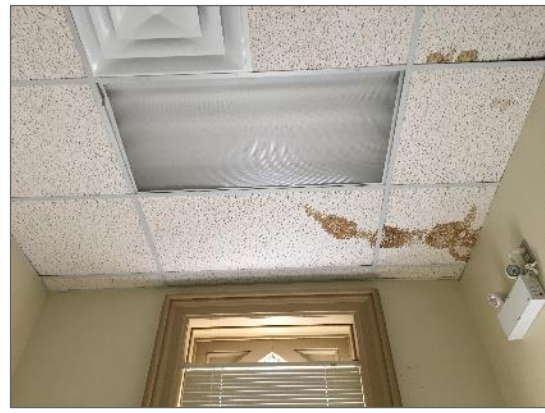
Photo 14 - Water stained ceiling tiles in the lunchroom
