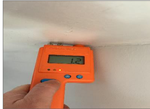
Photo 10 - Moisture reading of wet drywall in waiting area adjacent to the women's washroom
