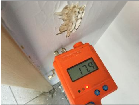
Photo 3 - Moisture meter confirms wet drywall adjacent to janitor's closet in the women's washroom
