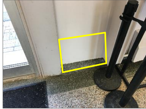
Photo 2 - Wet drywall adjacent to the north entrance
