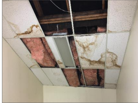
Photo 12 - Missing and water damaged ceiling tiles and insulation in the west stairwell
