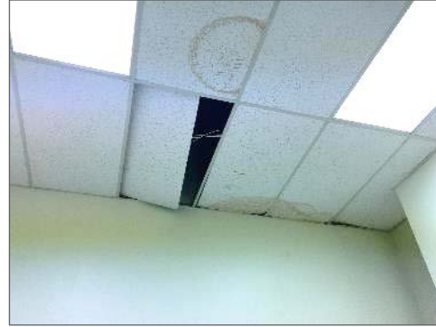
Photo 8 - Water damaged ceiling tile in the VIA train operations (location 12)
