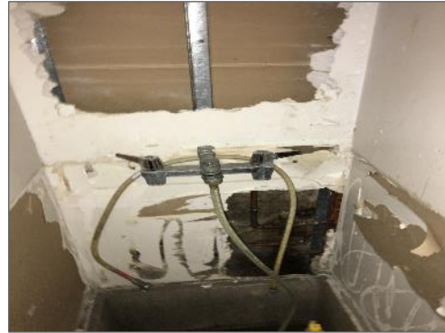
Photo 4 - Mould impacted drywall in the janitor's closet
