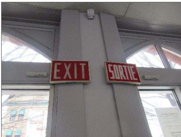
View of typical exit signage and emergency lighting noted throughout the Site Building.
