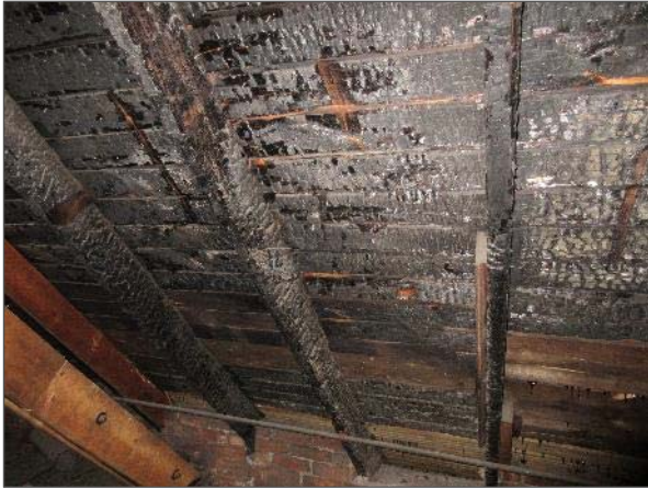
View of charred and damaged wood trusses and decking noted throughout the west attic spaces.
