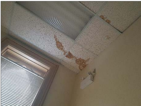
View of typical water staining noted throughout the second floor area of the Site Building.
