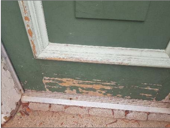
View of typical peeling paint and deterioration noted at the wood doors.
