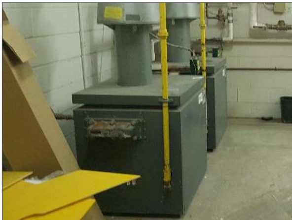
View of the two heating boilers noted serving the Site Building.
