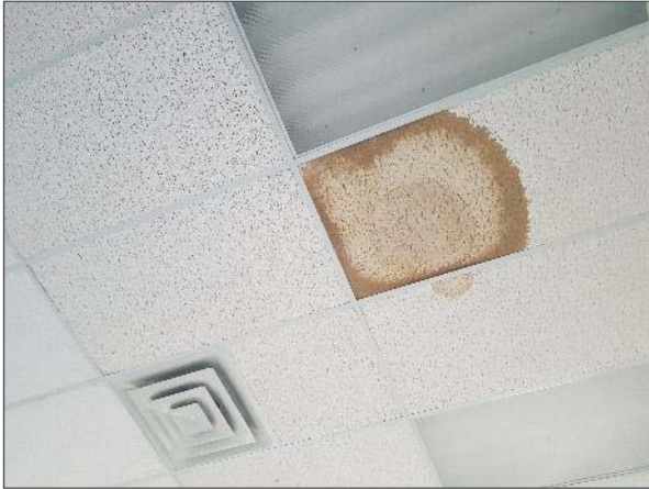
View of stained ceiling tiles noted throughout the second floor spaces of the Site Building.
