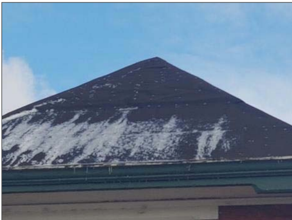
View of the west portion of the roof system which has reportedly been temporarily covered due to leaks.
