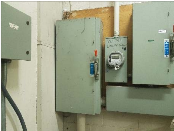
View of the main electrical disconnect switch noted serving the Site Building.
