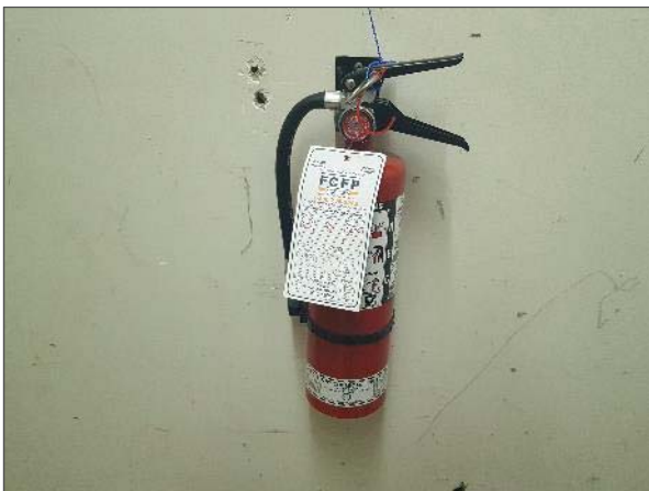
View of a typical stand-alone chemical fire extinguisher noted serving the Site Building.
