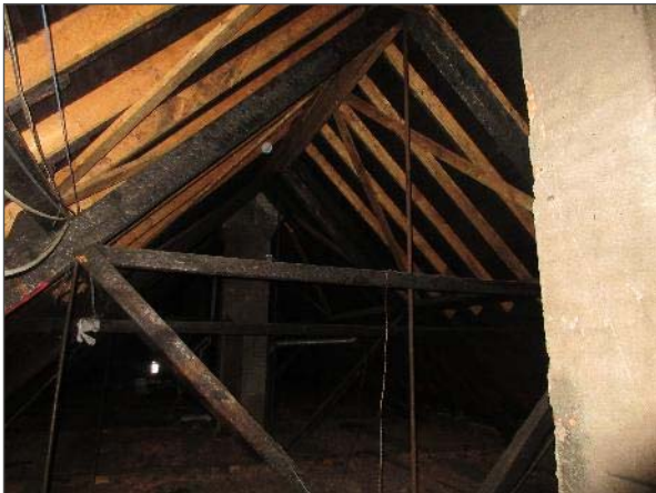
View of the attic space on the west portion of the Site Building.
