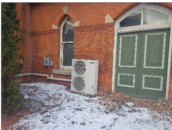
View of a heat pump unit noted serving the Site Building.
