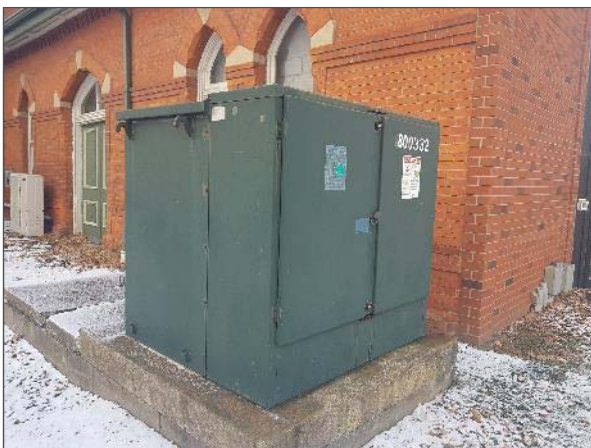
View of the pad mounted transformer noted serving the Site.
