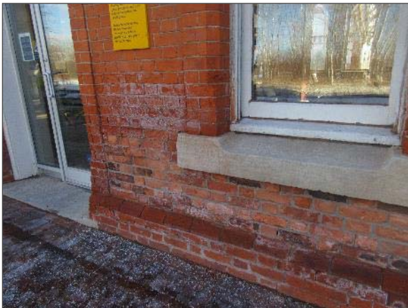
View of typical efflorescence noted at the lower portion of the brick masonry walls on all elevations.
