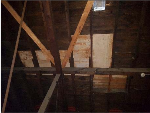
View of patch work within the attic of the west portion of the Site Building.
