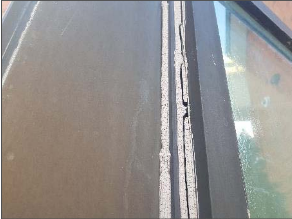
View of a typical failed perimeter window sealant at the east curtain wall system.
