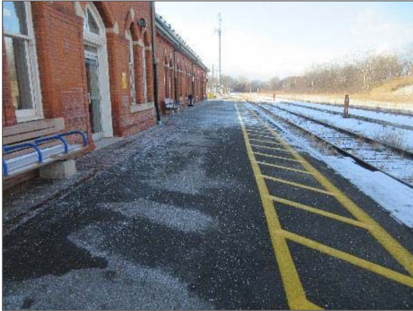
View of the asphalt pavements on the north train platform area of the Site Building.
