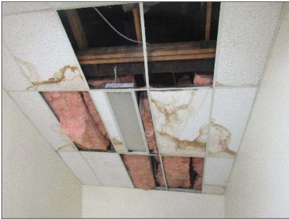
View of stained ceiling tiles and active roof leaks noted within the central stairwell of the Site Building.
