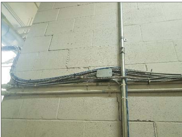
View of step cracking noted within a demising wall of the mechanical area.
