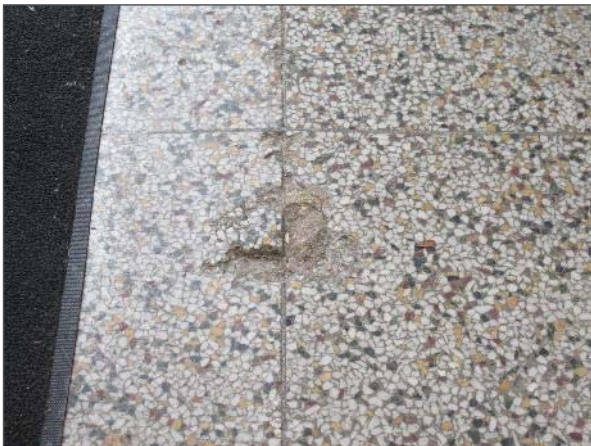
View of damaged terrazzo flooring noted within the lobby area of the Site Building.
