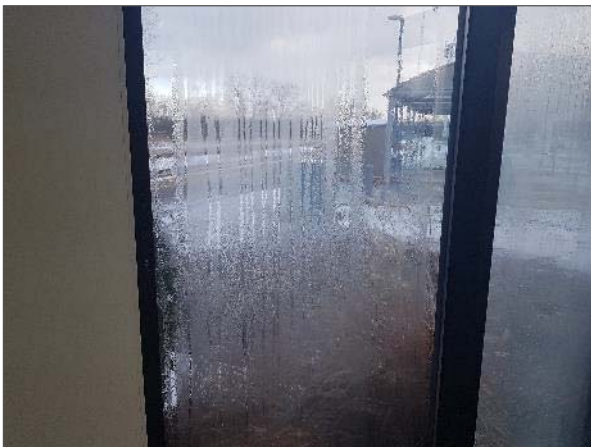
View of the failed IG curtain wall system at the east elevation.
