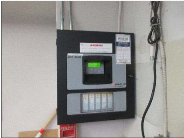
View of the fire alarm panel noted serving the Site Building.
