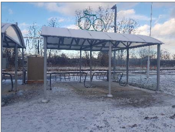
View of the cast-in-place concrete pads and shelter serving the waiting area/bike area adjacent to the east elevation of the Site Building.
