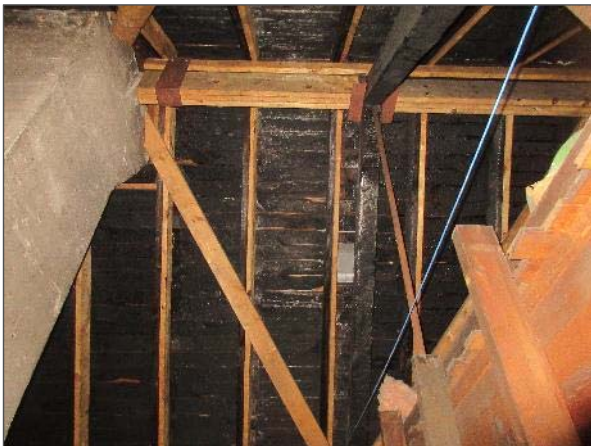
View of charred and damaged wood trusses and decking noted throughout the west attic spaces.
