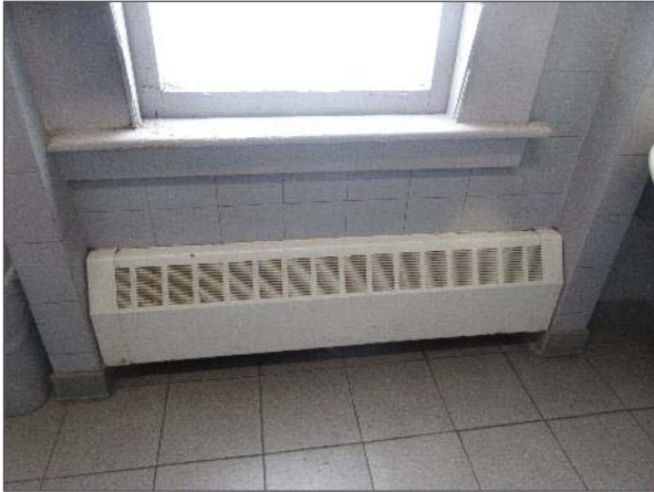
View of a typical hydronic baseboard noted throughout the Site Building.
