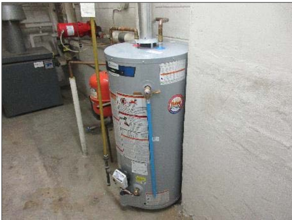
View of the DHW unit noted serving the Site Building.
