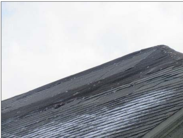
View of the roof on the north portion of the asphalt roof system which has also reportedly been temporarily patched.
