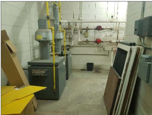
View of the finishes within the mechanical area.
