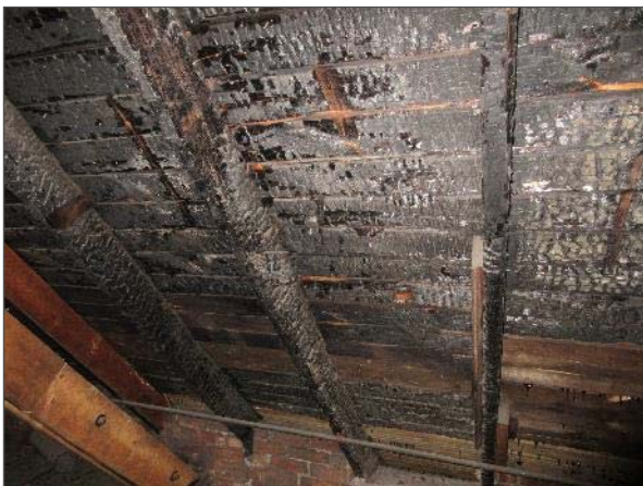
View of fire damage noted within the attic of the west portion of the Site Building.
