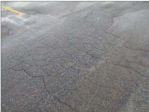
View of alligator cracking noted within the asphalt pavements of the Site.
