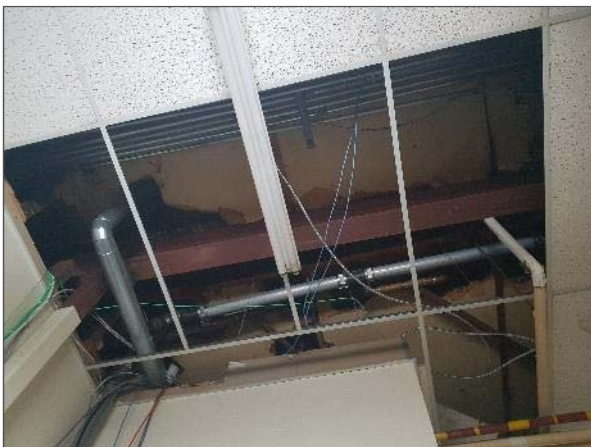
View of an area of steel beams and columns which appear to be retrofitted on the main floor level of the Site Building
