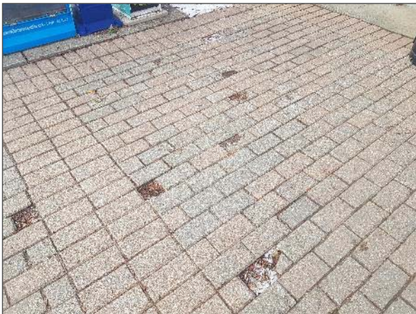
View of missing/damaged stone pavers noted on the south portion of the Site.
