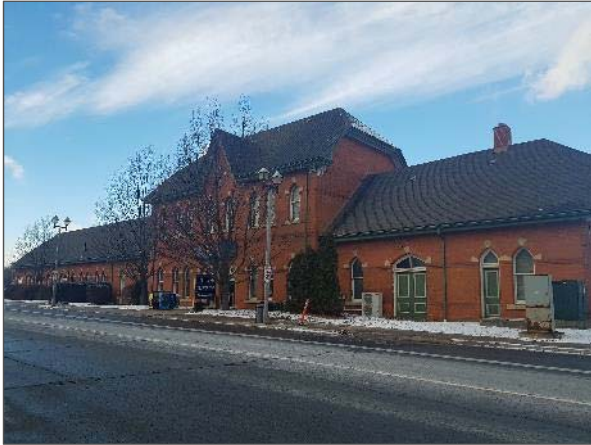
General view of the south portion of the asphalt shingled roof systems.
