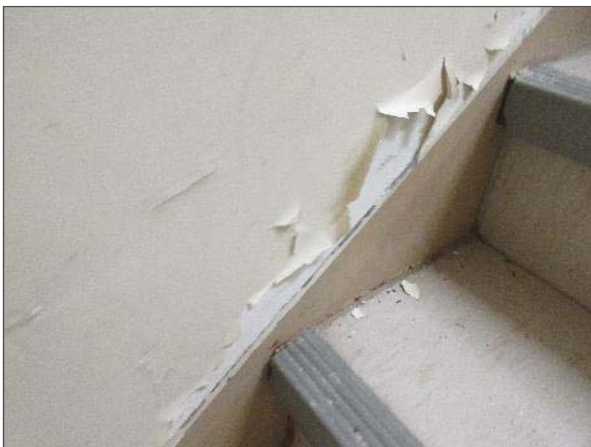
View of peeling paint noted within the central stairwell of the Site Building.
