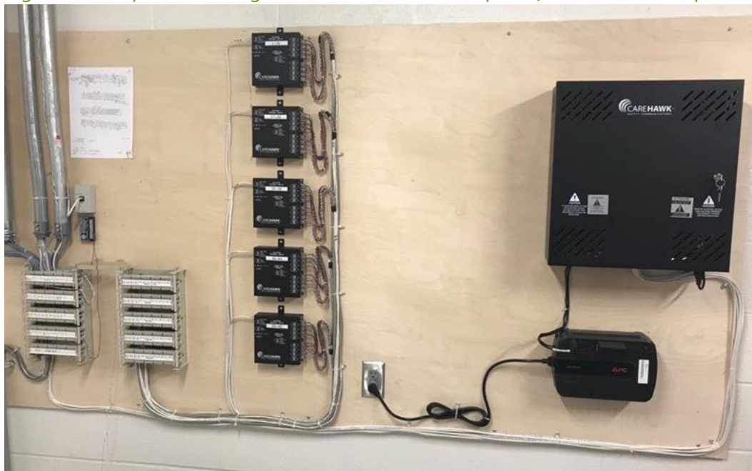
Figure 1: PA system cabling and termination to BIX panel, with service loops and neat cabling
