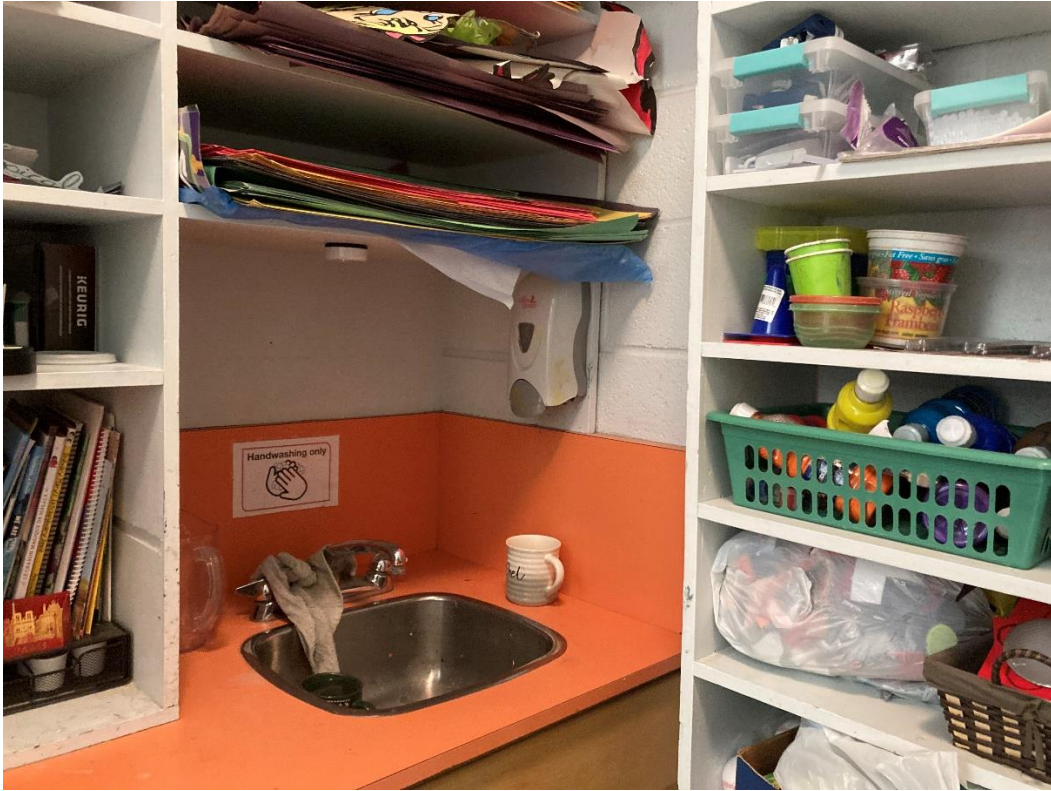
S0171 (Confirmed Asbestos), Sink mastic on the underside of the sink in Location #: 260
