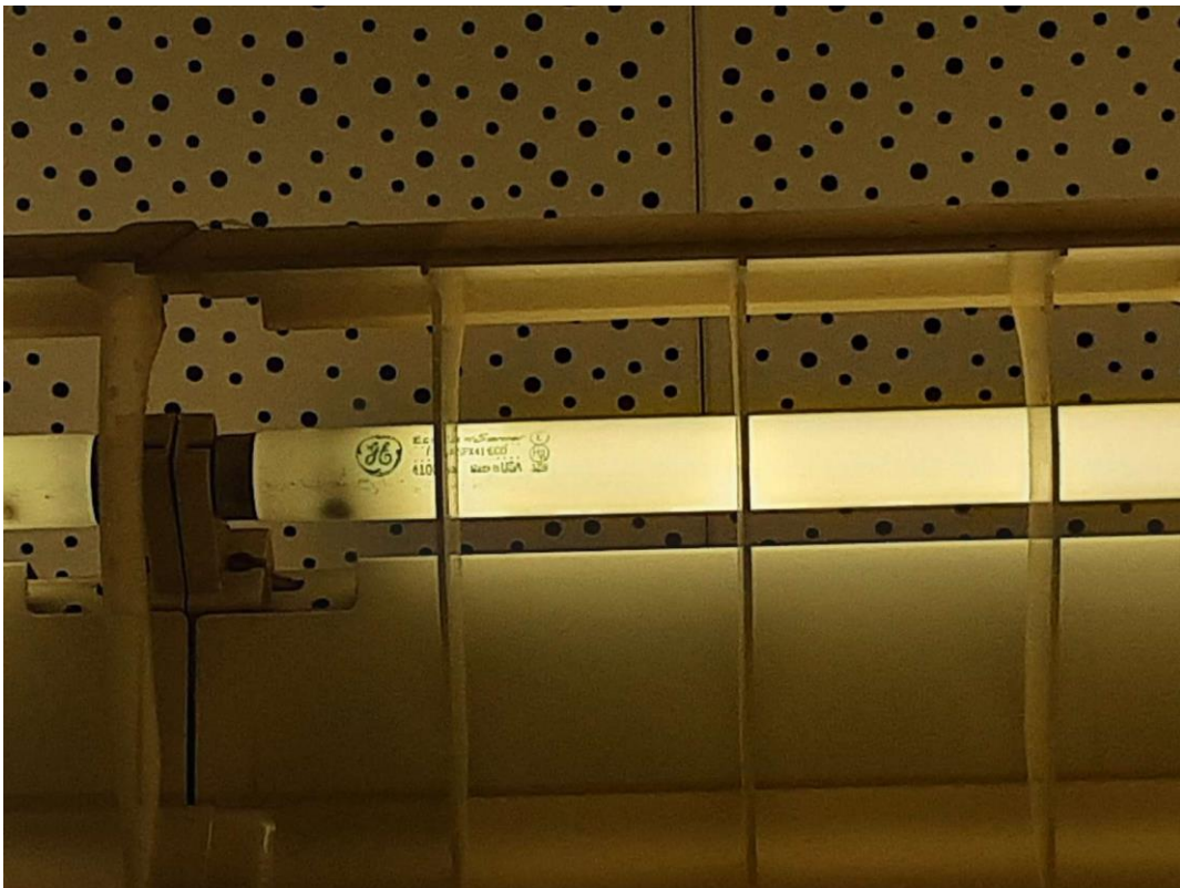
Mercury, V9000(Yes), Mercury containing light fixtures in Location #: 259
