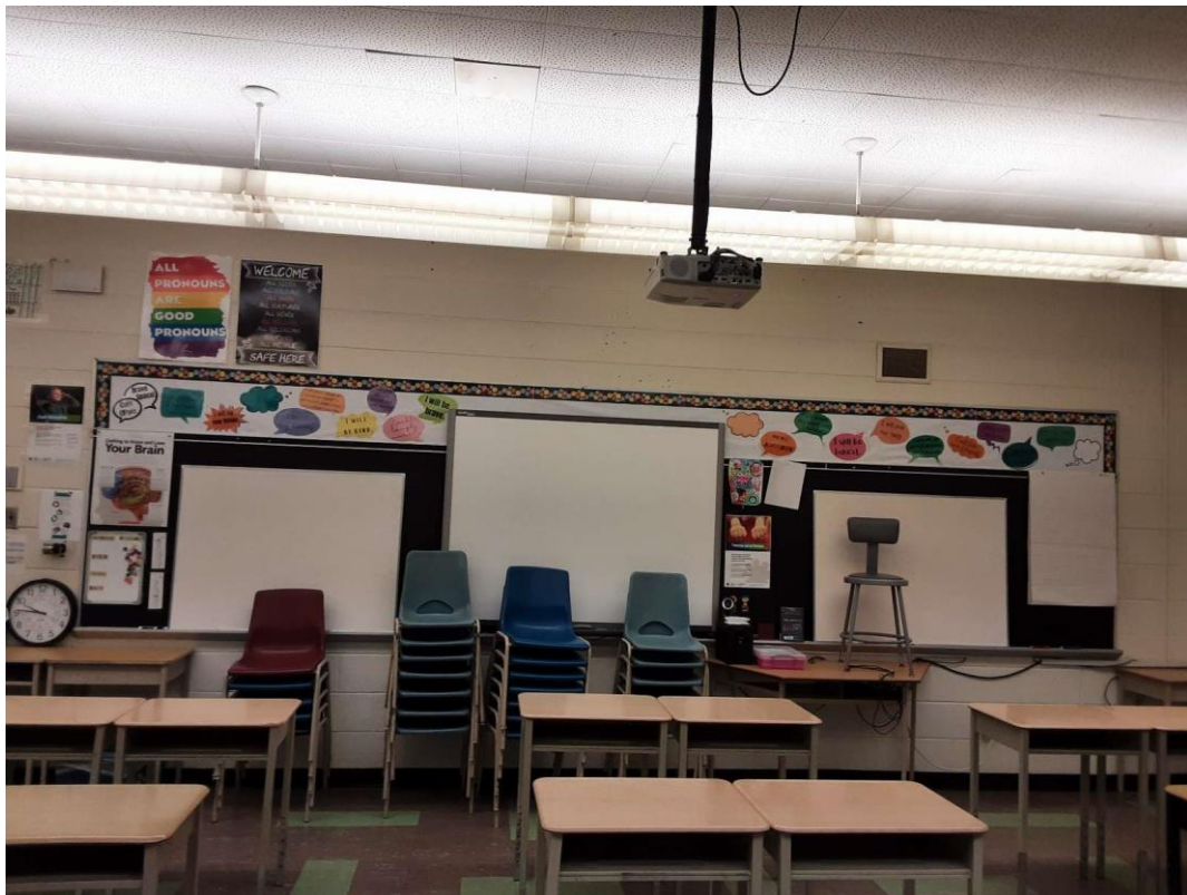
V9500 (Presumed Asbestos), Mastic behind chalkboard and corkboard in Location #: 257
