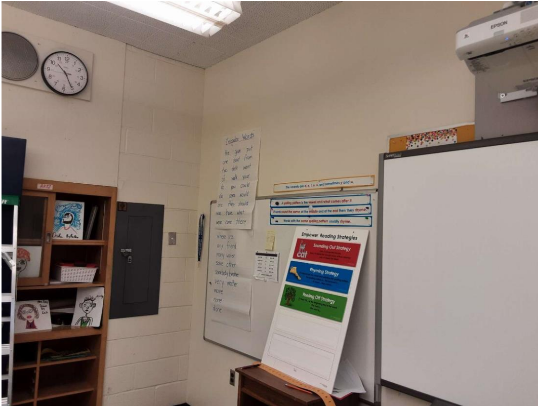
L0037(Lead, Low), White paint on drywall in Location #: 262
