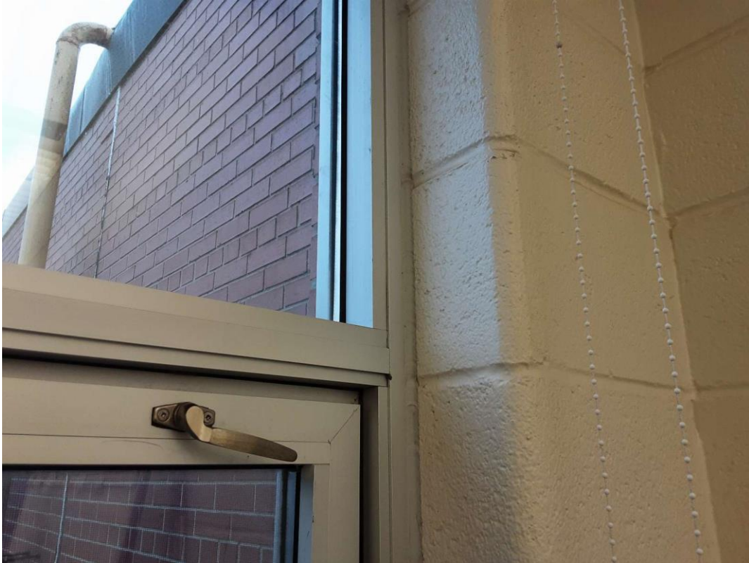
PCB, P0008(No), Grey caulking near windows in Location #: 262
