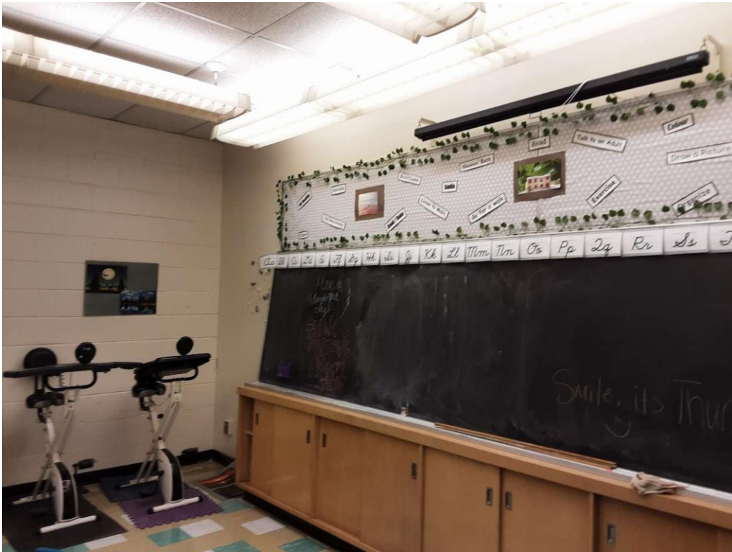
S0158C (Confirmed Asbestos), Drywall and joint compound on wall of Location #: 261
