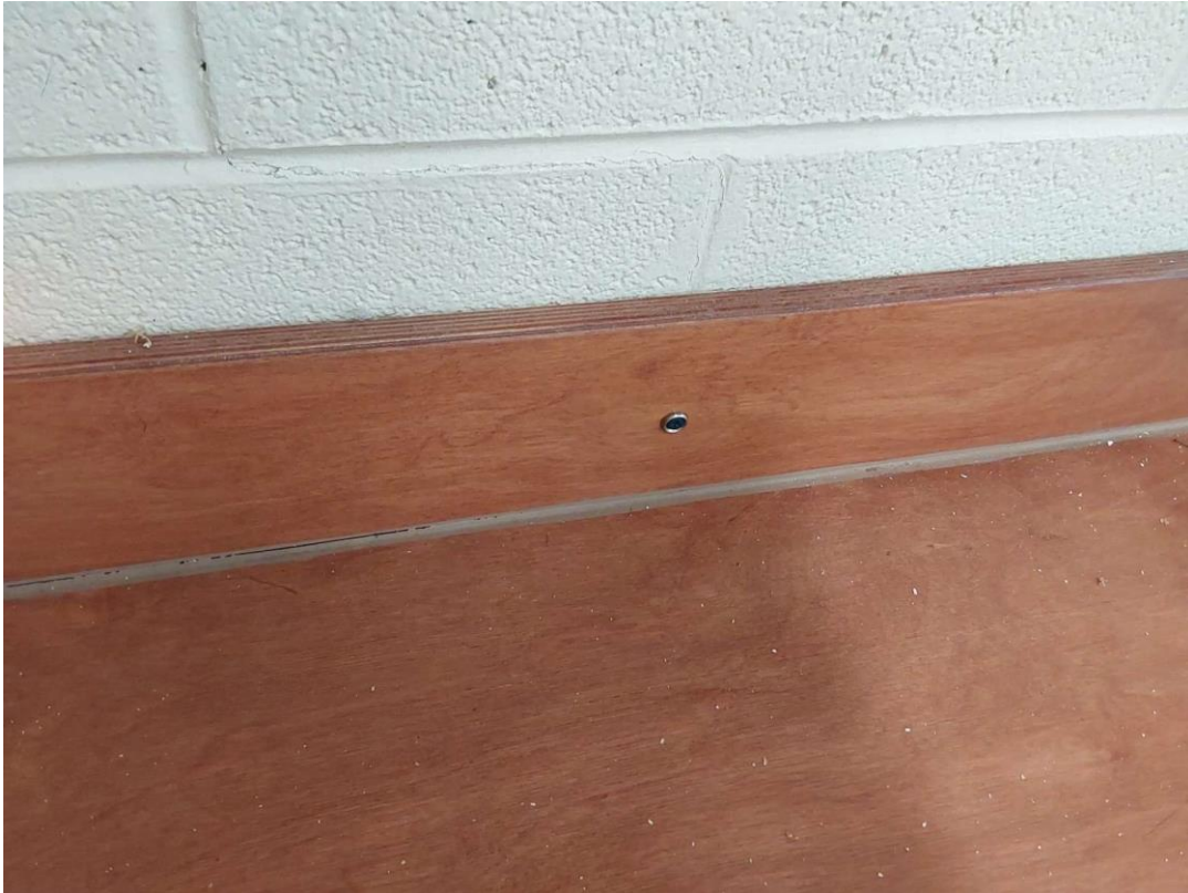
PCB, P0001(No), CAULKING, Grey caulking on wood bench, CLASSROOM (Location #: 13)
