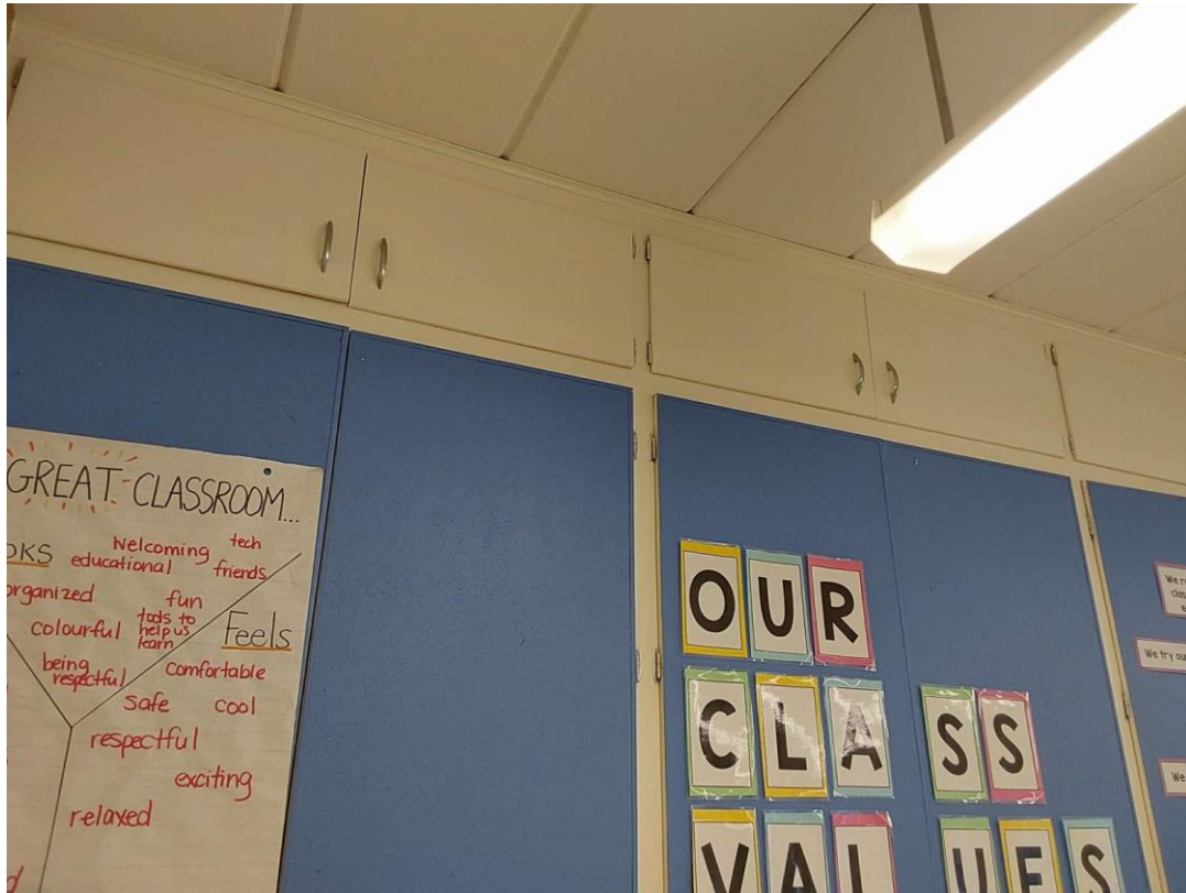
L0003(Lead, None), White on wood, Wall, CLASSROOM (Location #: 13)
