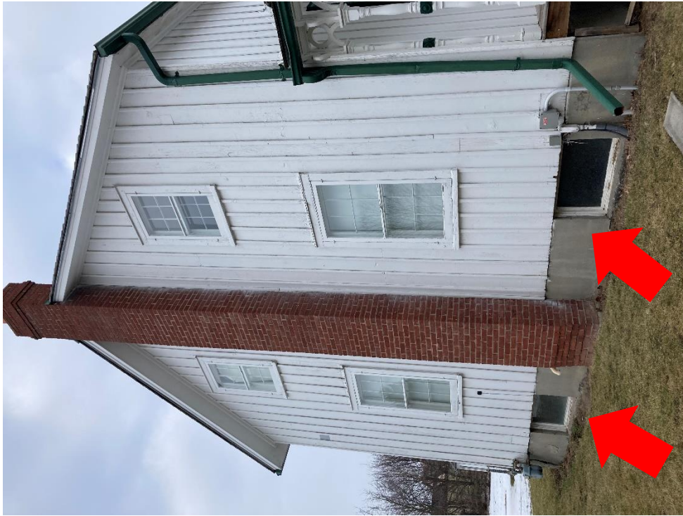
5. South face, reglaze the top four (4) windows and replace the bottom two (2) windows
