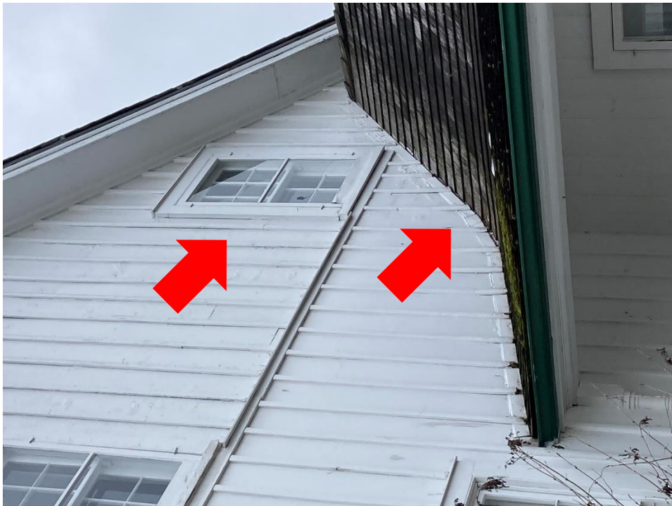
6. Replace one (1) window and repair existing window frame on north wall. Localized batten repair above the roof on north wall.
