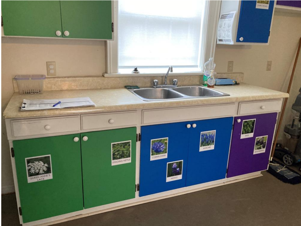
7. Existing kitchen countertop, sink and faucet to be replaced
