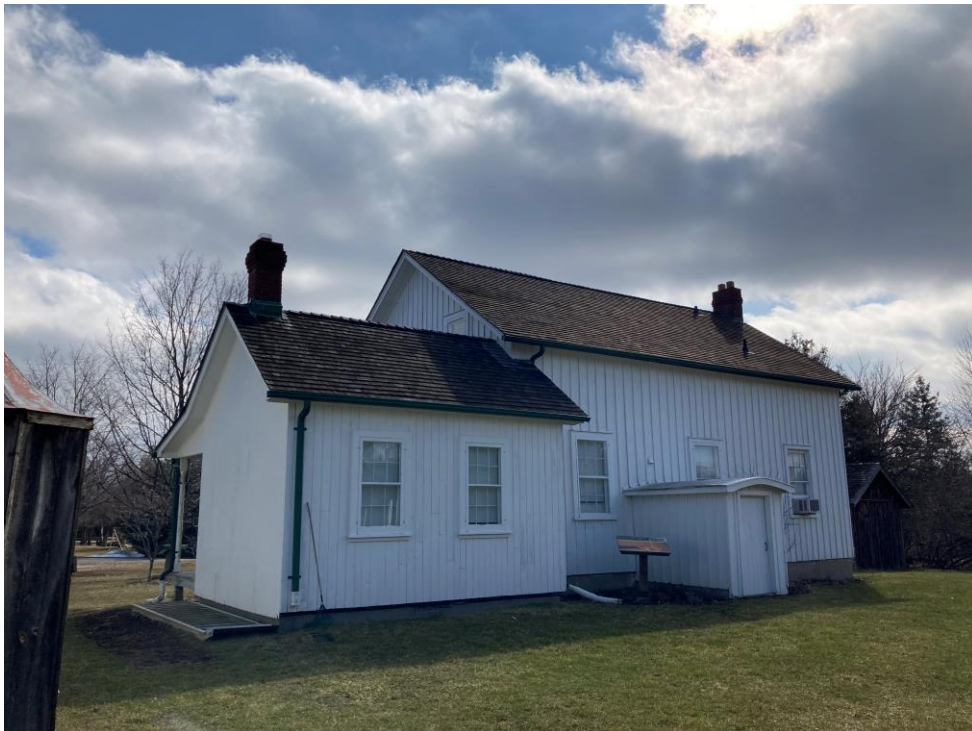
4. West face, reglaze and repair the window frames of all five (5) windows
