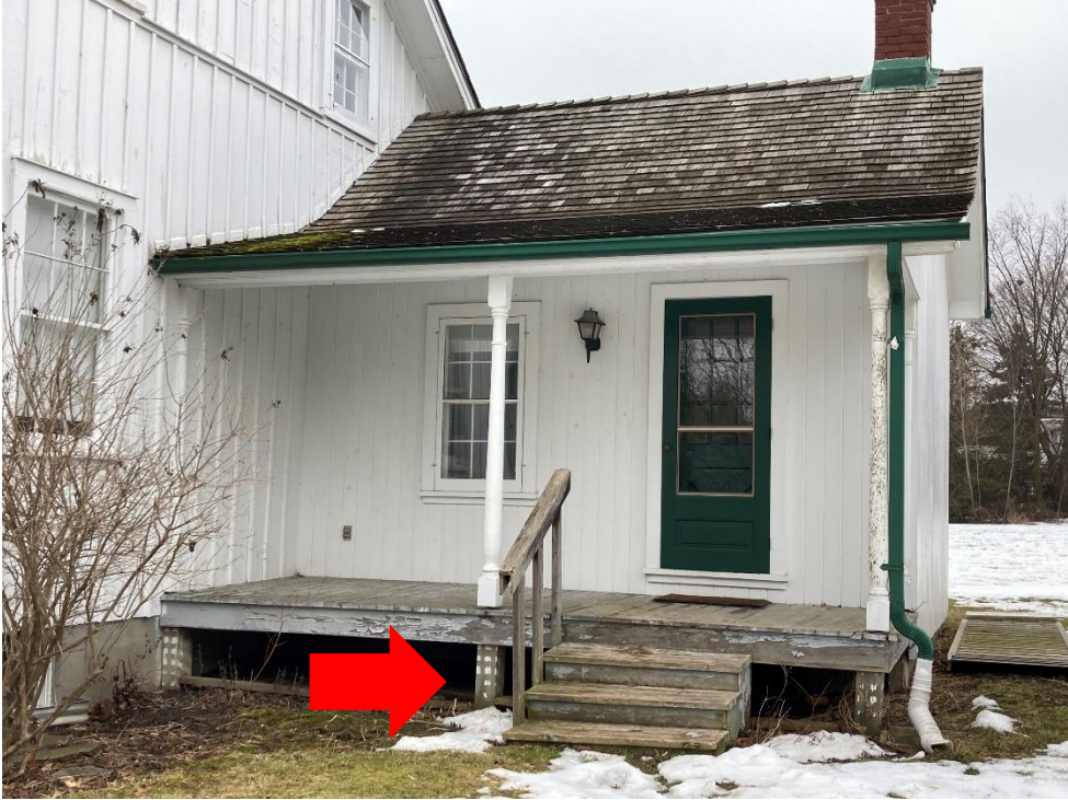
2. East face – north side, existing stair to be replaced with new double railing wood stair
