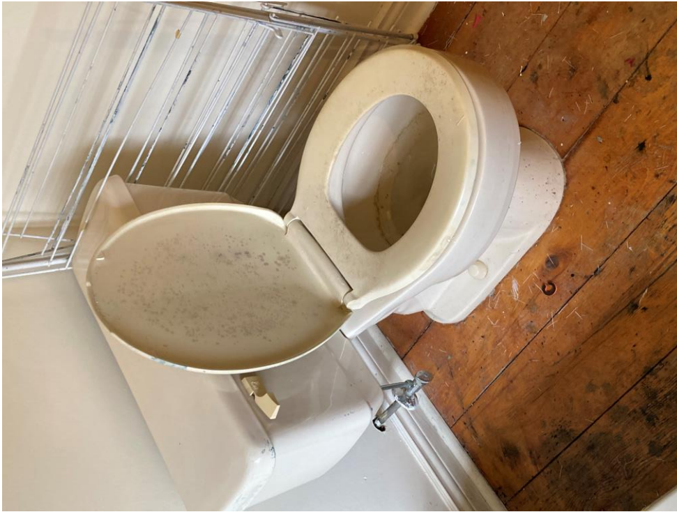
11. Existing toilet in the upstairs washroom to be removed with opening sealed
