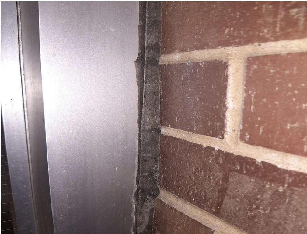
Photograph No. 8 – Exterior dark gray sealant at main entrance doors contains asbestos.
