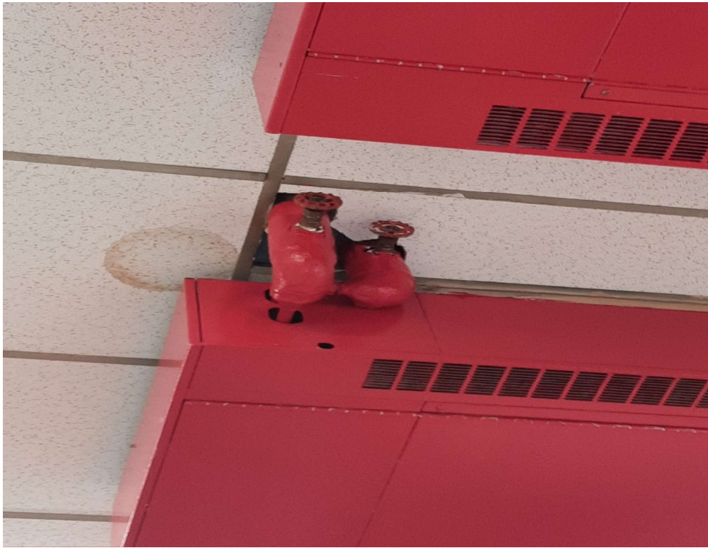
Photograph No. 1 – Suspect asbestos-containing pipe fittings at ceiling level in room 2044. The ceiling was too high to be safely sampled. Additional fittings are assumed present above the ceiling tiles.
