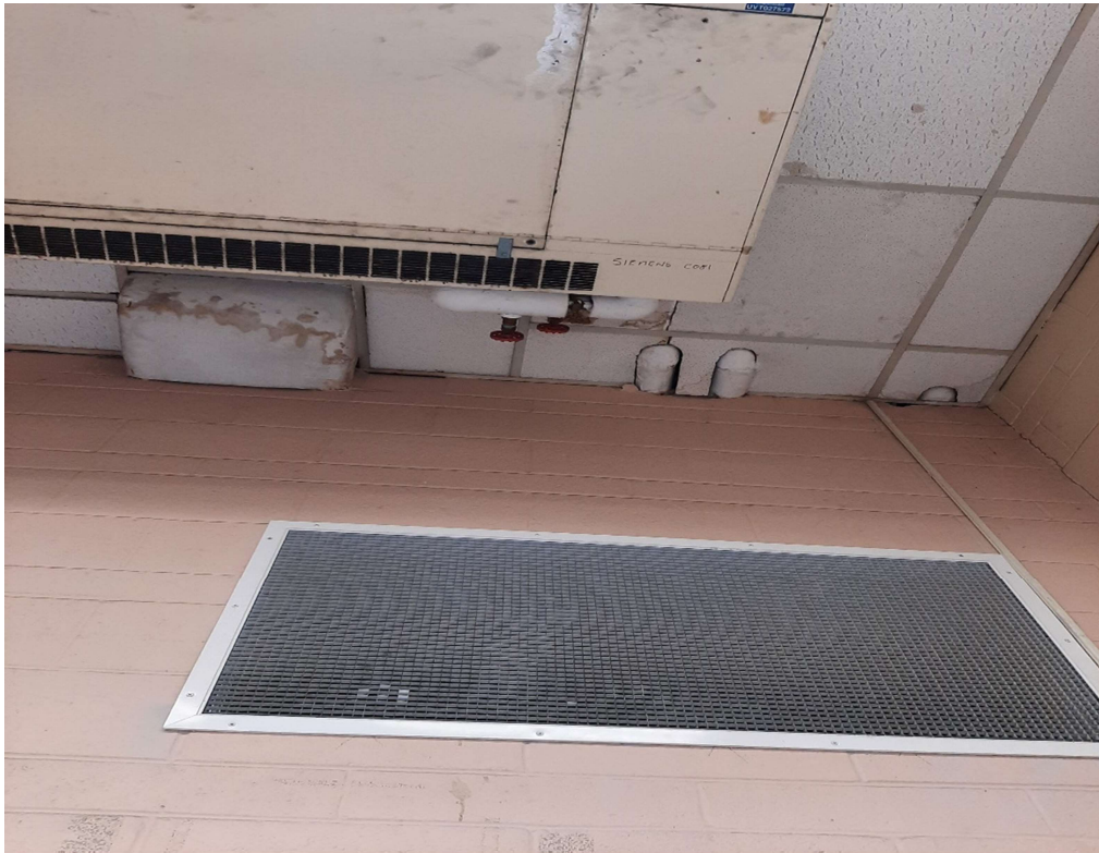
Photograph No. 5 – Suspect asbestos pipe fittings at ceiling level in room 2041. Additional fittings are assumed present above the ceiling tiles.
