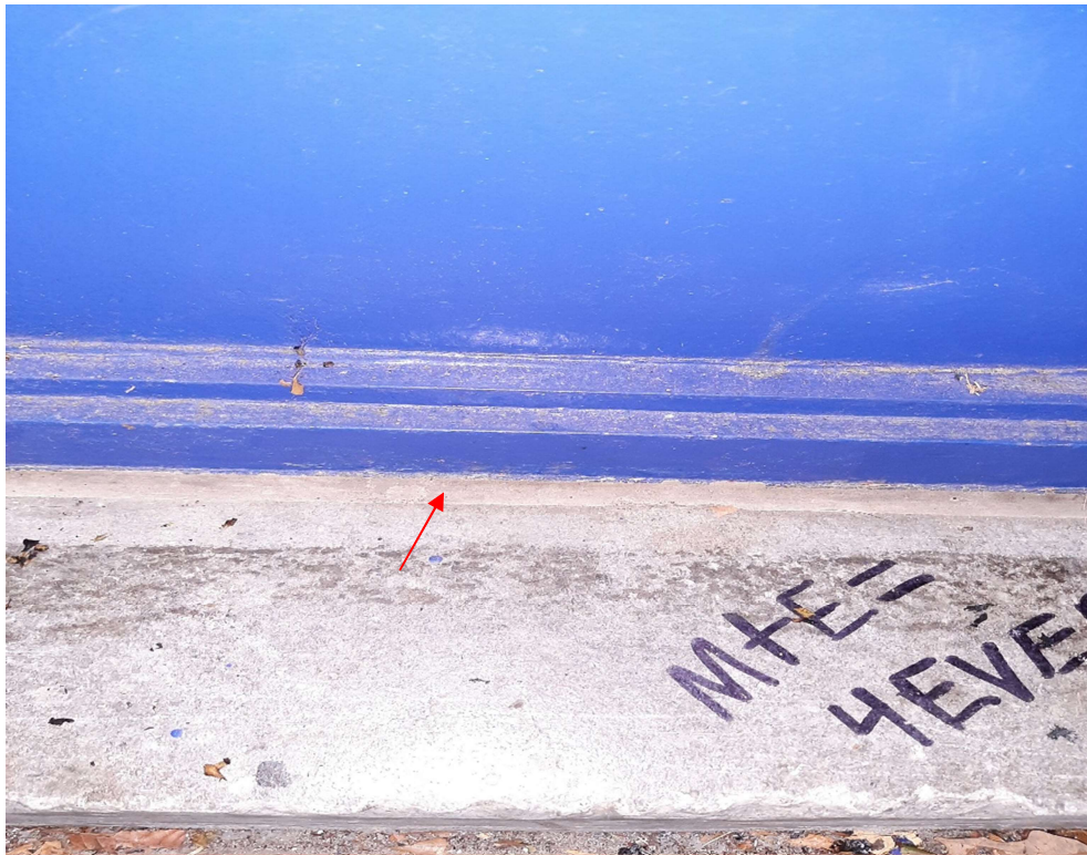
Photograph No. 6 – Gray exterior sealant around exterior doors and panels contains PCBs.
