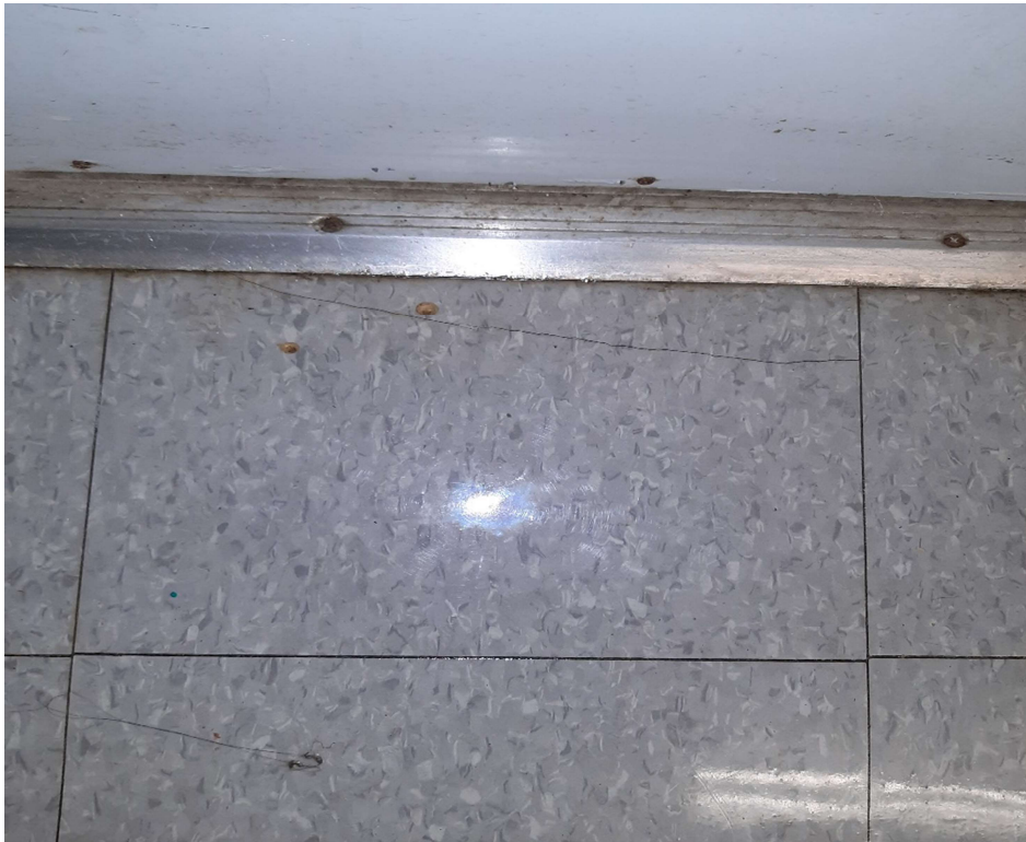
Photograph No. 4 – Black mastic under 12"x12" gray fleck pattern vinyl floor tiles in classroom 123 contains asbestos.
