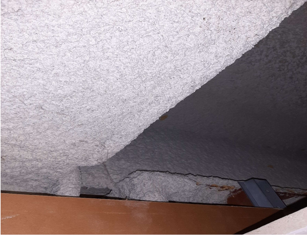
Photograph No. 7 – Fireproofing present within ceiling cavities throughout contains asbestos.
