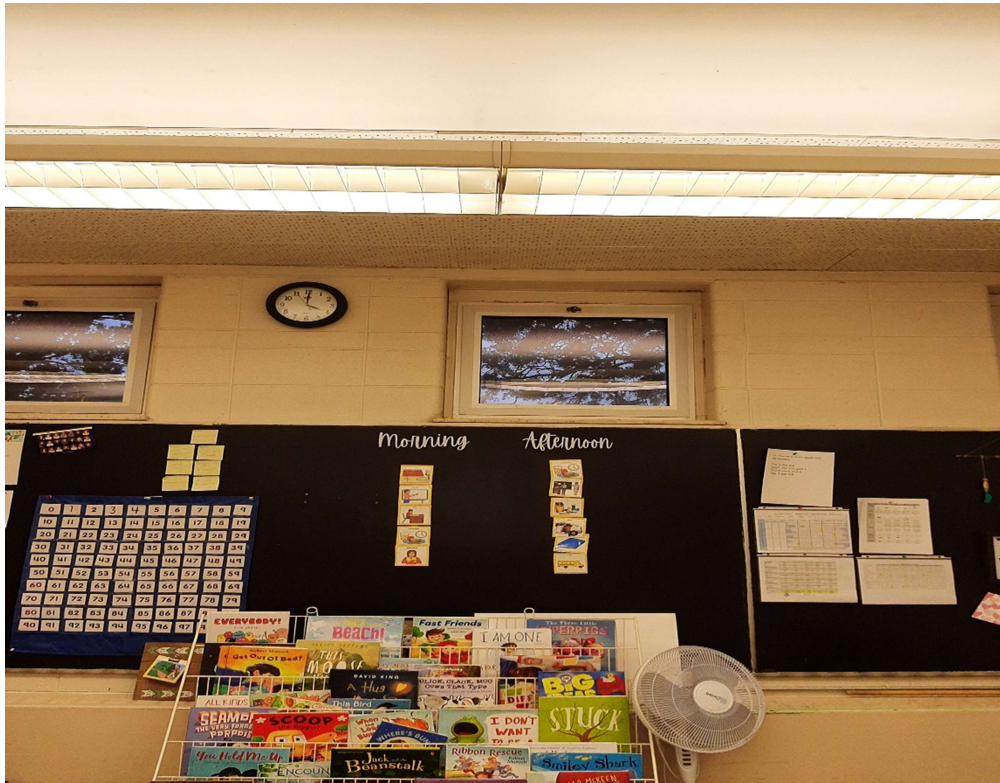
Photograph No. 5 – Drywall joint compound on the ceiling in classroom 123 contains asbestos.
