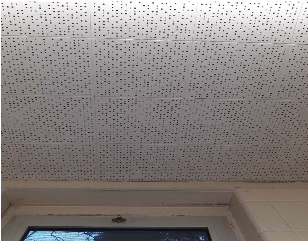
Photograph No. 2 – 1’x1’ pinhole pattern ceiling tiles in classroom 123 are non-asbestos, however suspect asbestos containing mastic may be concealed underneath.
