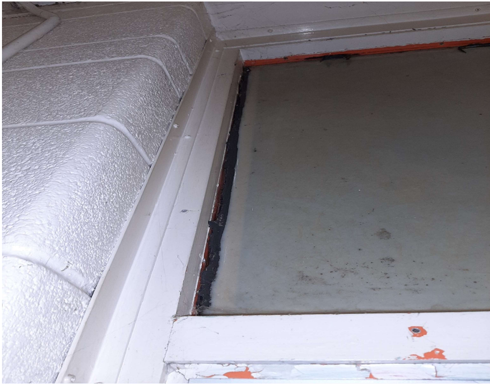
Photograph No. 3 – Black sealant on the door inside classroom 123 contains asbestos.
