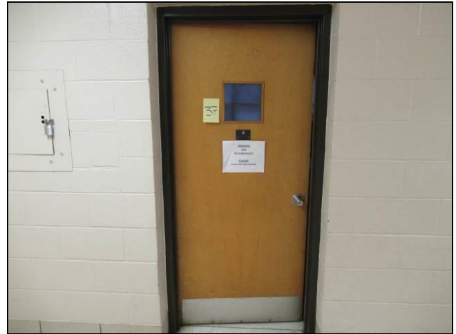
Photograph 2: Typical classroom door to be replaced.
