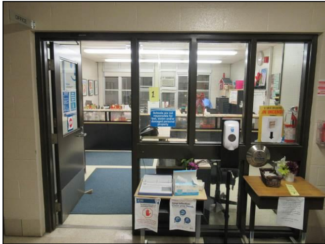
Photograph 1: General Office door and frame to be replaced.
