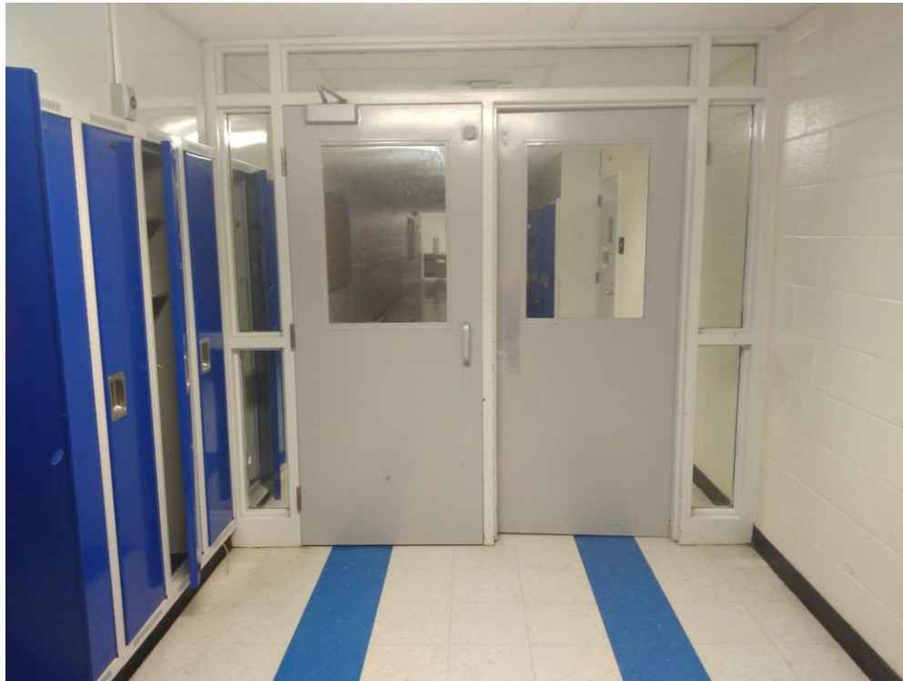
Photograph 9: Existing elevation for double door slab and frame replacement for door No. 66.
