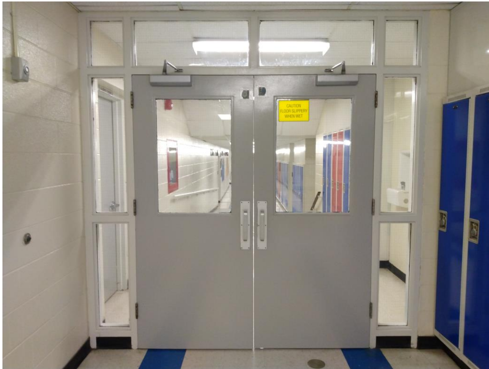
Photograph 7: Existing elevation for double door slab and frame replacement for door No. 30.
