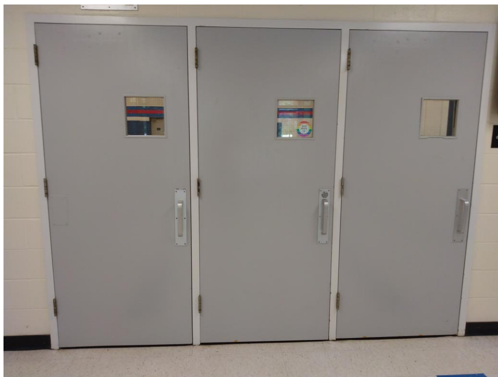
Photograph 4: Existing elevation for triple door slabs and frame replacement for door No. 5.
