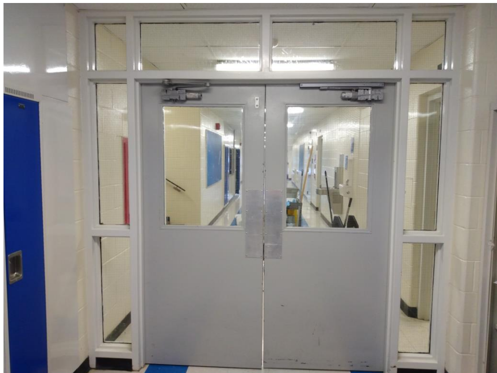
Photograph 8: Existing elevation for double door slab and frame replacement for door No. 40.
