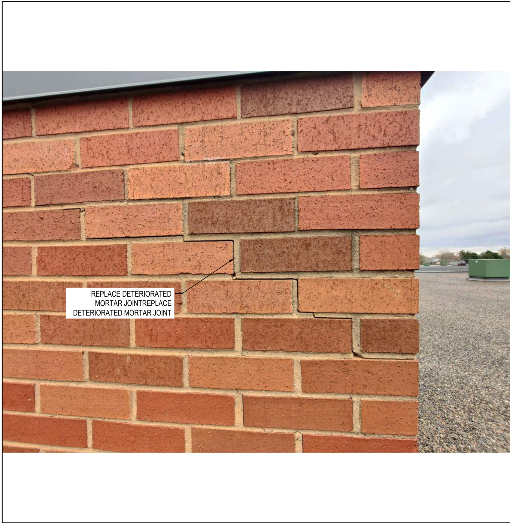
2 DETERIORATED MORTAR JOINT R600
