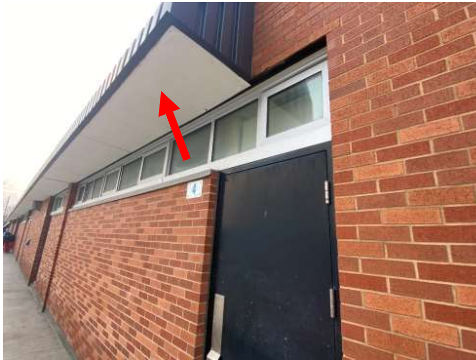
Photo 1 – View of asbestos-containing Transite board on the exterior soffit.
