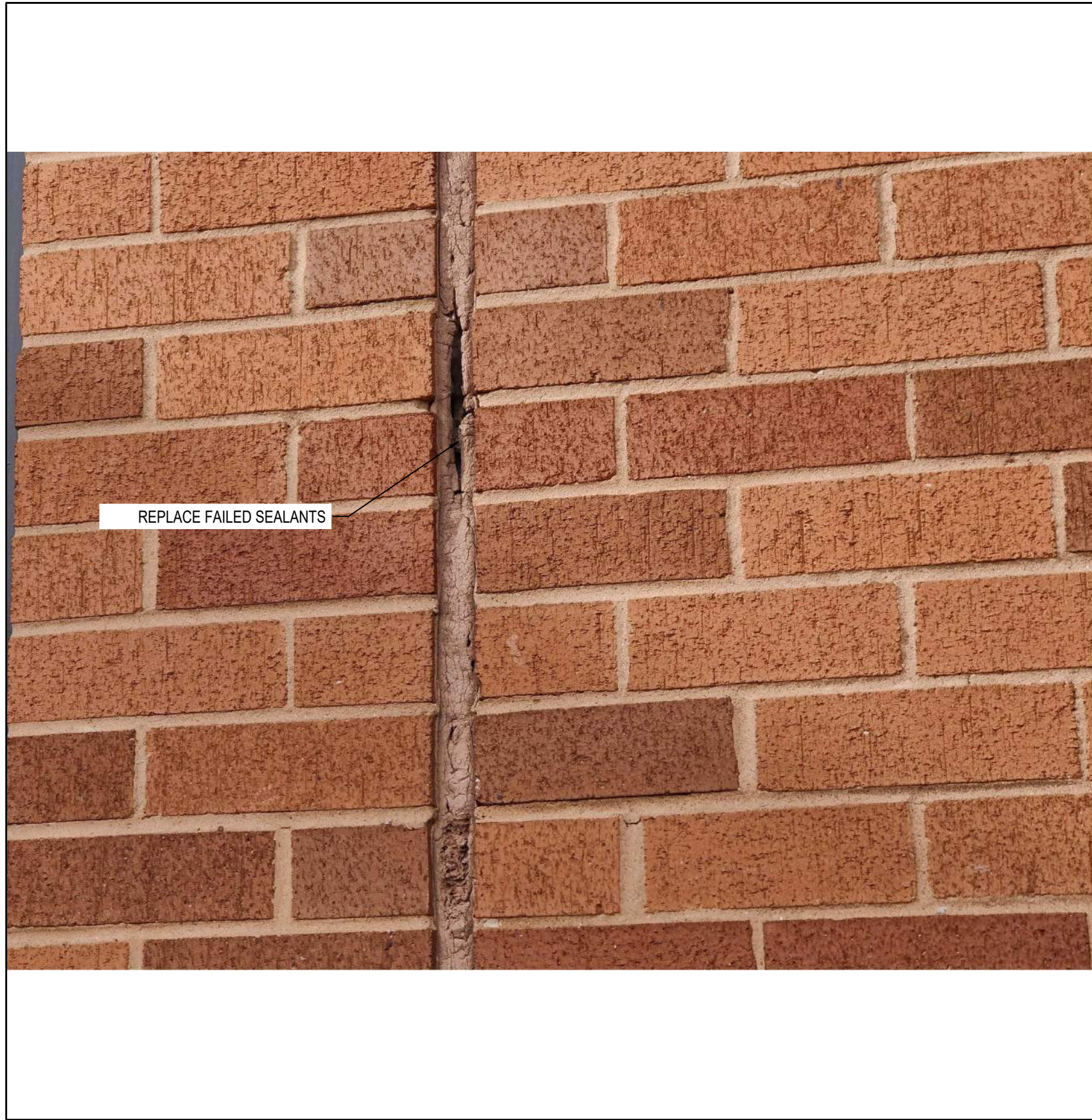
3 FAILED SEALANT JOINT R600
