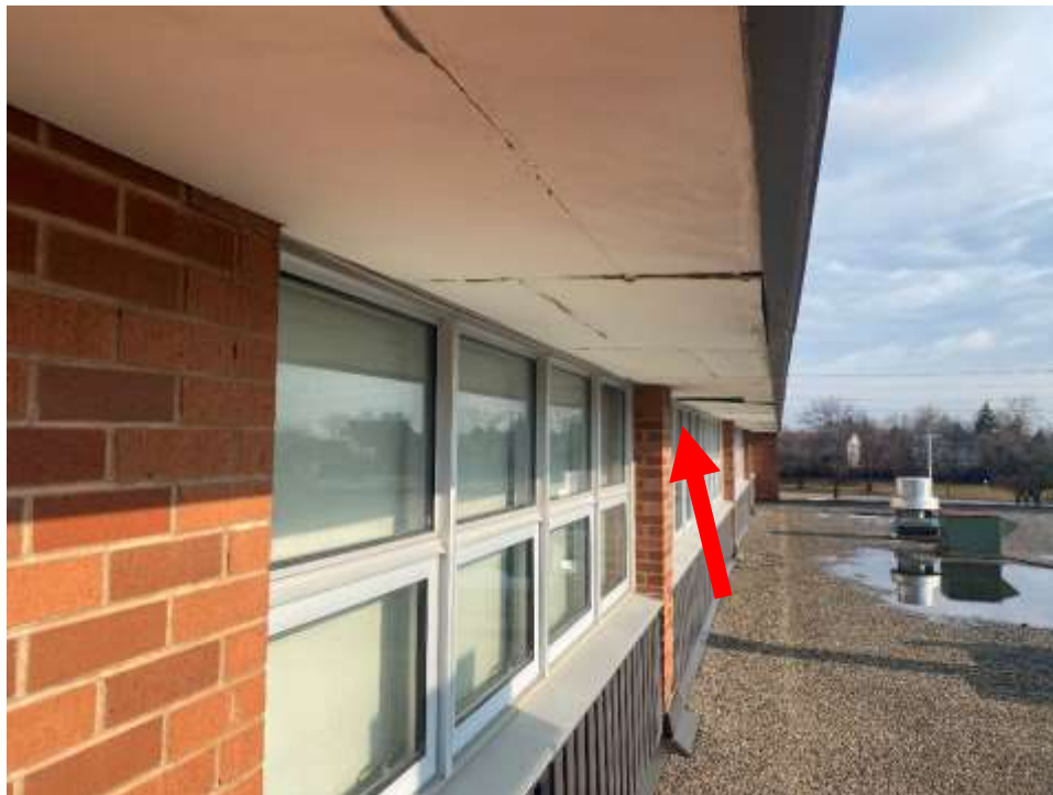
Photo 2 – Another view of asbestos-containing Transite board on the exterior soffit.
