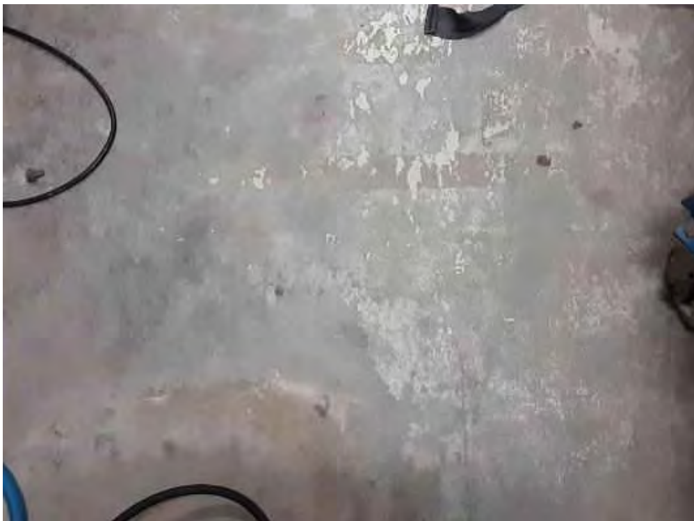
V0000 (None), Floor, All, Concrete (poured), Equipment Room 2 (Location #: 20)
