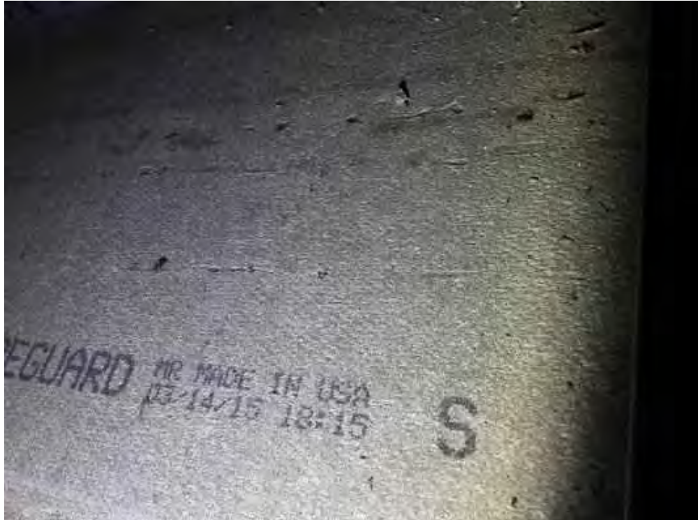
V0000 (None), Ceiling, All, Ceiling Tiles (lay-in), Corridor (Location #: 27) Water staining observed, date stamp -03/14/15
