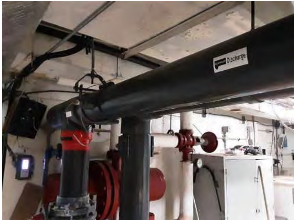
V0000 (None), Piping, Polyvinyl chloride (PVC), Filter Room (Location #: 2) Inlet, discharge, vacuum, skimmer, waste
