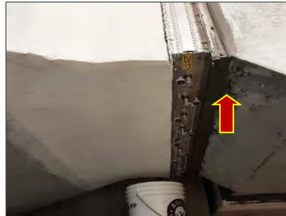
Photo 7: Non-asbestos grey duct mastic present in the Mechanical Room and Stairwell (Loc. 21).
