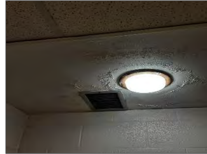
Photo 15: Non-asbestos plaster in the Men's Washroom (Loc. 22).
