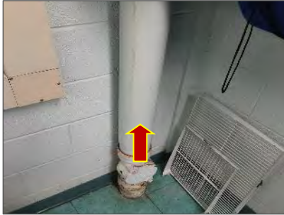
Photo 18: Presumed asbestos cement pipe (Transite) present in the Phys. Ed. Room (Loc. 24).
