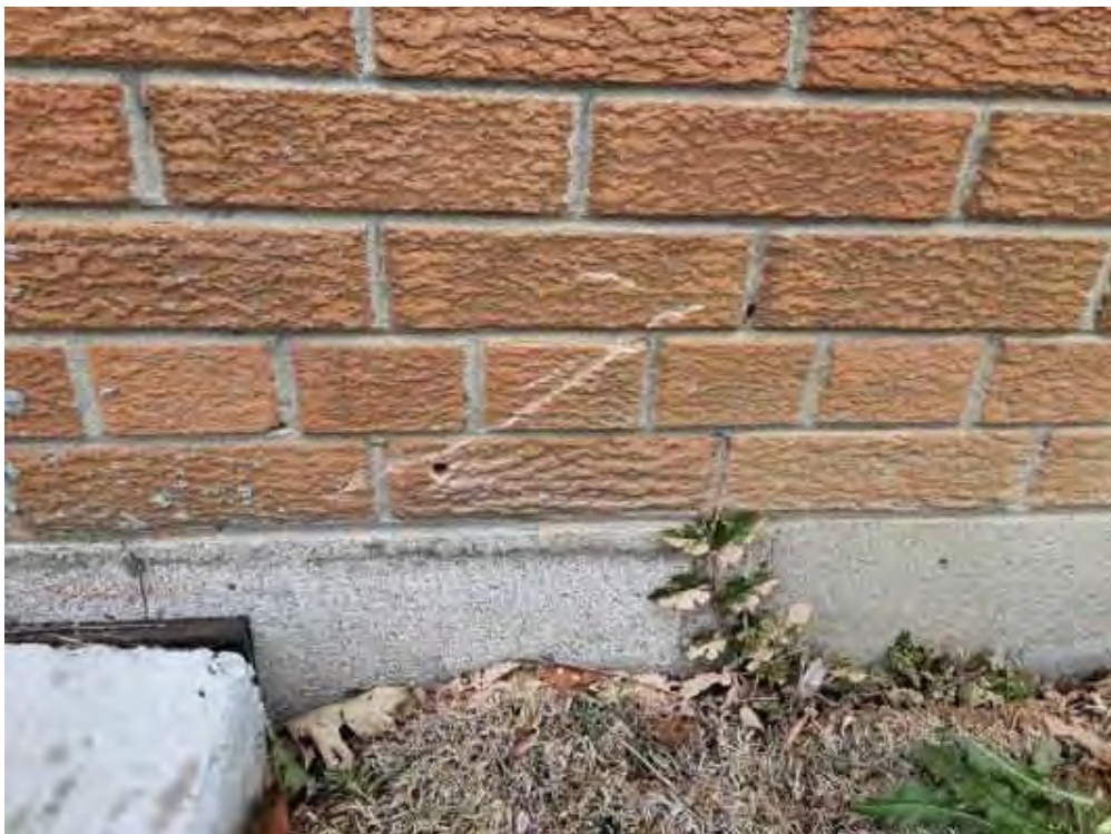
V0000 (None), Wall, Vermiculite, Exterior (Location #: 14) 5 Drill holes, no vermiculite, N wall, NE wall, S wall, SW wall, brick wall
