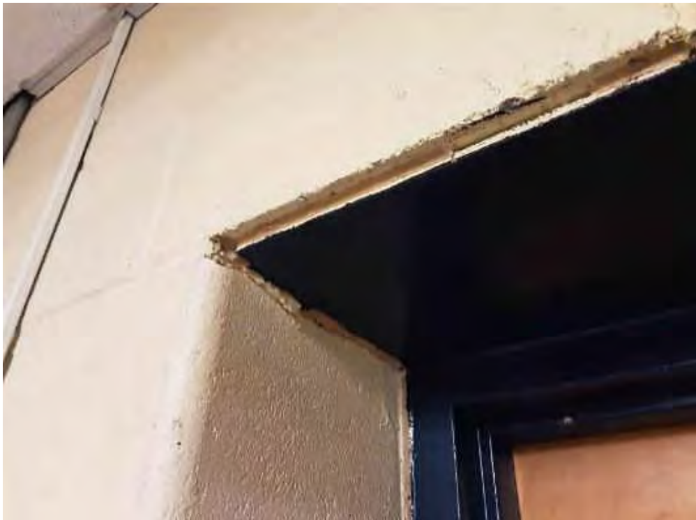
S0029A (Confirmed Asbestos), Wall, Door, Caulking, Gym Storage (Location #: 25) Between wall and door frame
