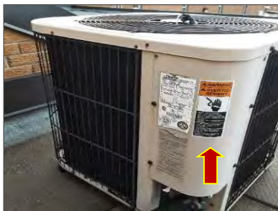
Photo 10: Uninsulated compressor present in the Lower Roof (Loc.17).
