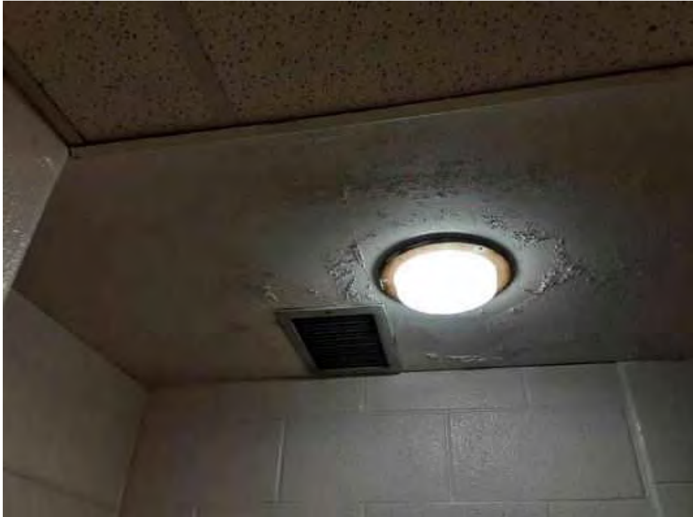
V0018 (None), Ceiling, Plaster, Men's Washroom (Location #: 22) Same as men's change room
