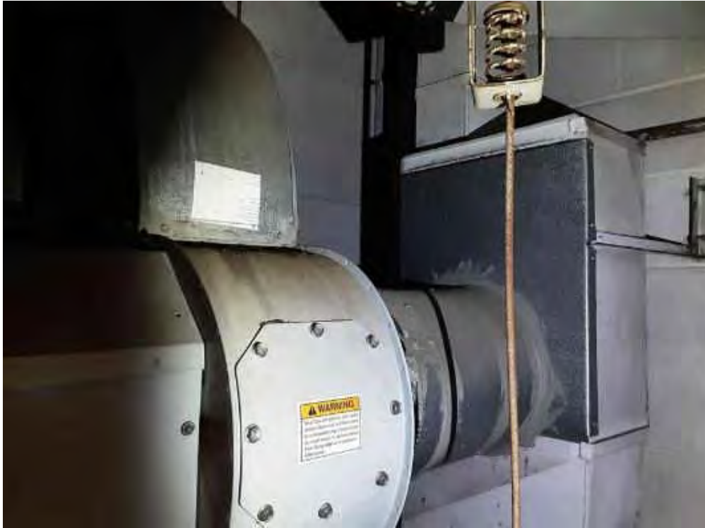
V0000 (None), Mechanical Equipment, Fan Unit, Not Insulated, Mechanical Room And Stairwell (Location #: 21)
