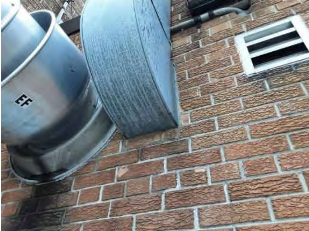
V0015 (None), Duct, Caulking, Exterior (Location #: 14) Lightgrey, S wall
