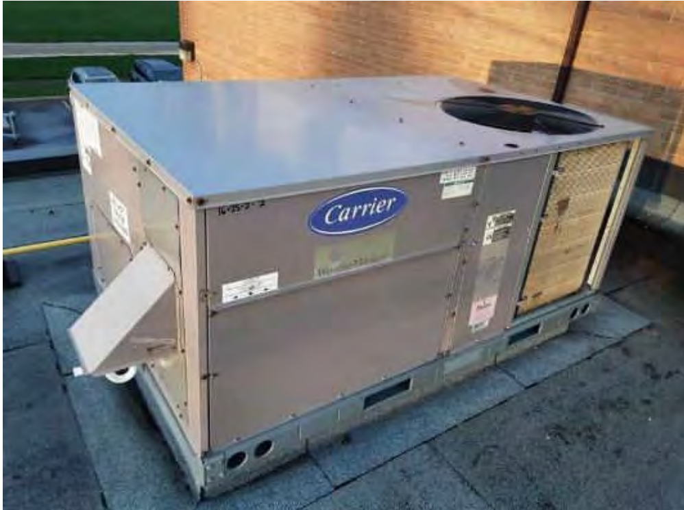
V0000 (None), Mechanical Equipment, Air Handling Unit, Not Insulated, Lower Roof (Location #: 17)
