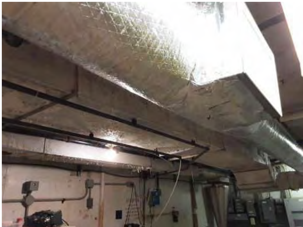
V0000 (None), Duct, All, Fibreglass, Filter Room (Location #: 2)
