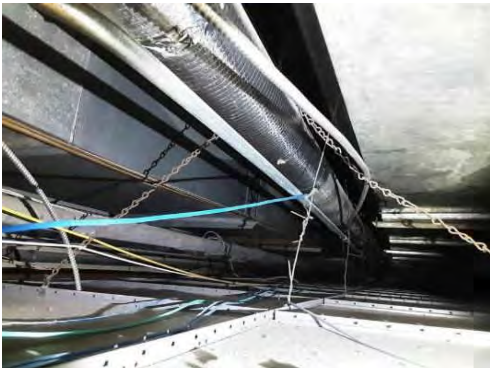
V0000 (None), Duct, All, Not Insulated, Corridor (Location #: 27)
