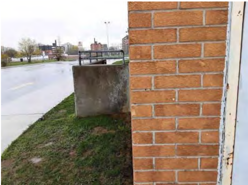
S0012B (Confirmed Asbestos), Wall, Mortar, Exterior (Location #: 14) Brick
