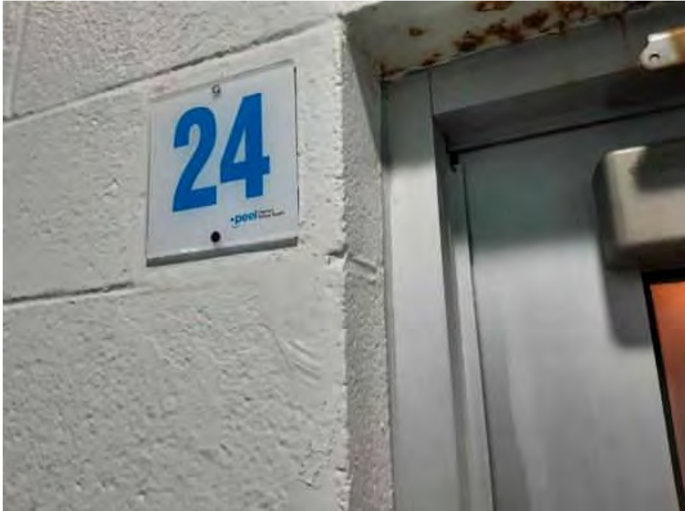
V0013 (Confirmed Asbestos), Other, Door, Caulking, In door Pool (Location #: 13) Grey, S wall, between wall and door frame
