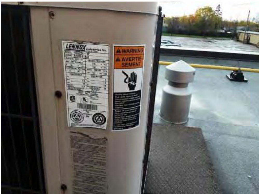
V0000 (None), Mechanical Equipment, Compressor, Not Insulated, Lower Roof (Location #: 17) Fan unit
