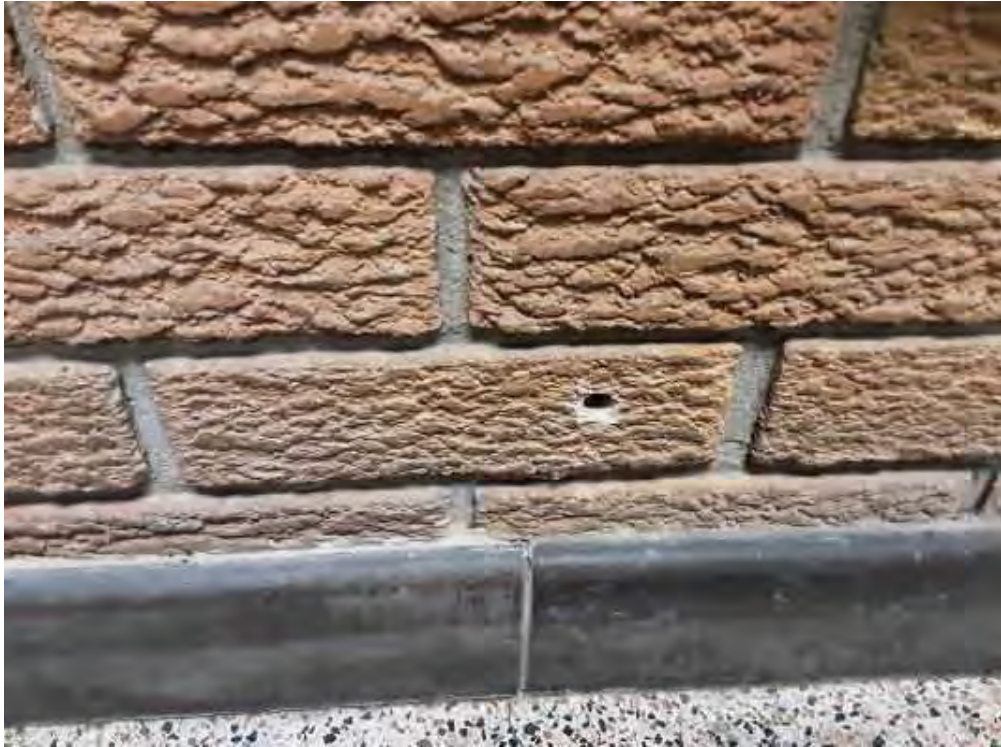
V0000 (None), Wall, Base, Vermiculite, Lobby (Location #: 7) 1 drill hole, no vermiculite, NW wall beside stairwell, brick
