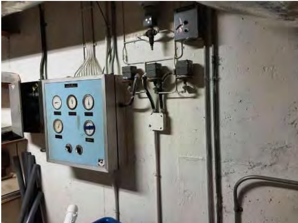
V0000 (None), Other, Electrical Panel, Not Insulated, Fan Room (Location #: 1)
