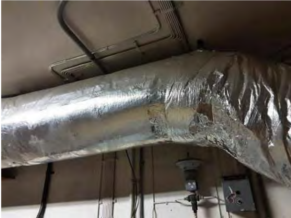
V0000 (None), Duct, All, Fibreglass, Fan Room (Location #: 1)
