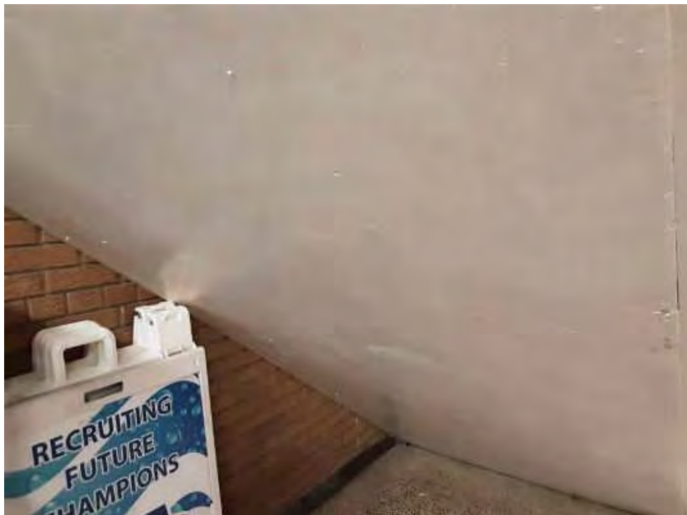
S0008A (Confirmed Asbestos), Other, Stairs, Drywall Compound, Lobby (Location #: 7) Underneath the stairwell
