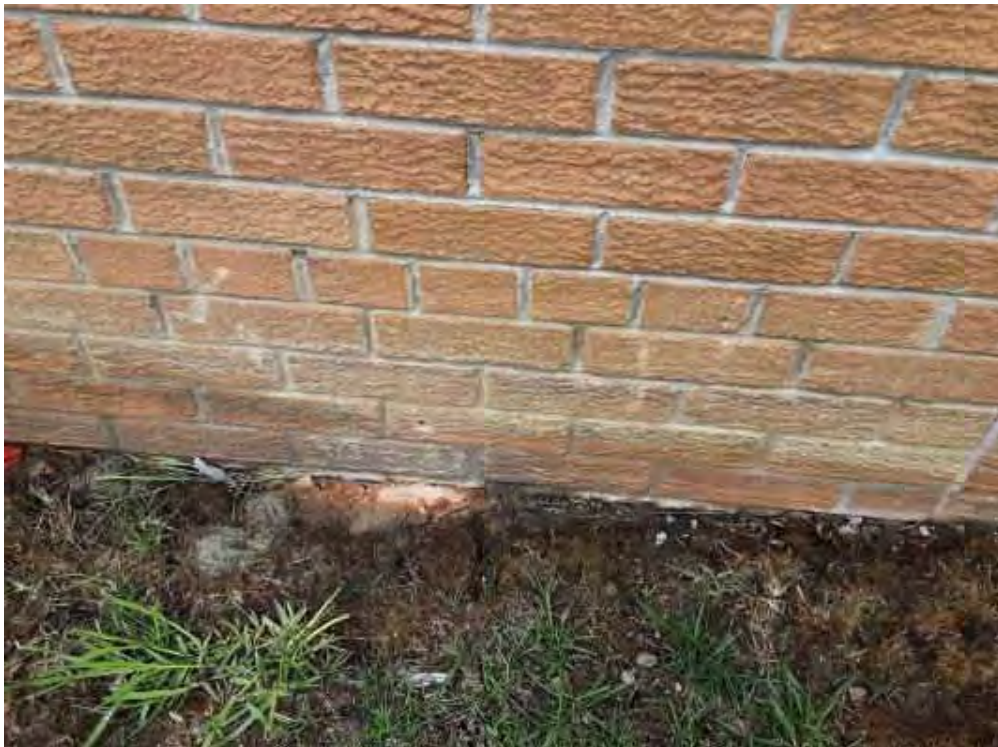
V0000 (None), Wall, Vermiculite, Exterior (Location #: 14) 5 Drill holes, no vermiculite, N wall, NE wall, S wall, SW wall, brick wall
