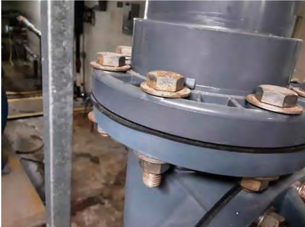
V0000 (None), Mechanical Equipment, Rubber, Filter Room (Location #: 2)
