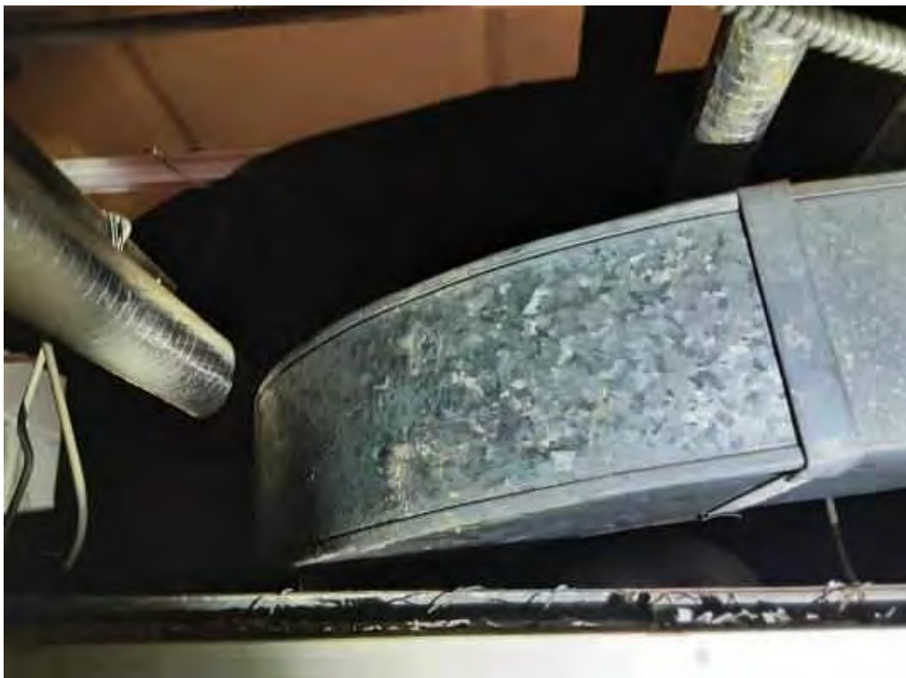
V0000 (None), Duct, All, Not Insulated, Men's Washroom (Location #: 22)
