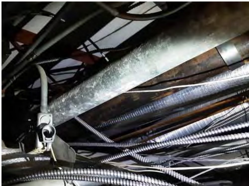
V0000 (None), Duct, All, Not Insulated, Hallway (Location #: 28)
