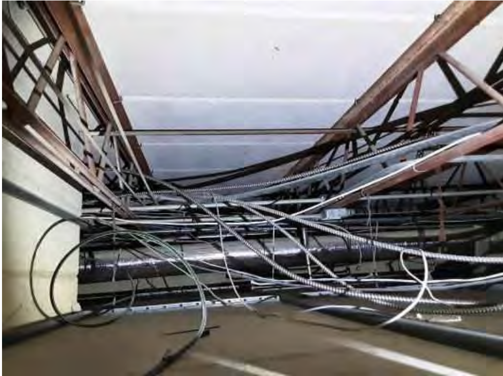
V0000 (None), Piping, Fibreglass, Gym Storage (Location #: 25)
