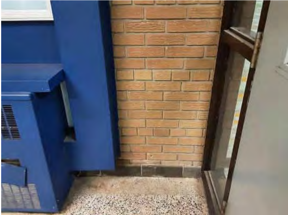
V0000 (None), Wall, Base, Vermiculite, Entrance Vestibule (Location #: 6) 1 drill hole, no vermiculite, NE wall, brick wall
