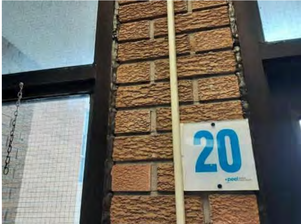
S0016A (Confirmed Asbestos), Other, Door, Caulking, Entrance Vestibule (Location #: 6) Black, between wall and door frame
