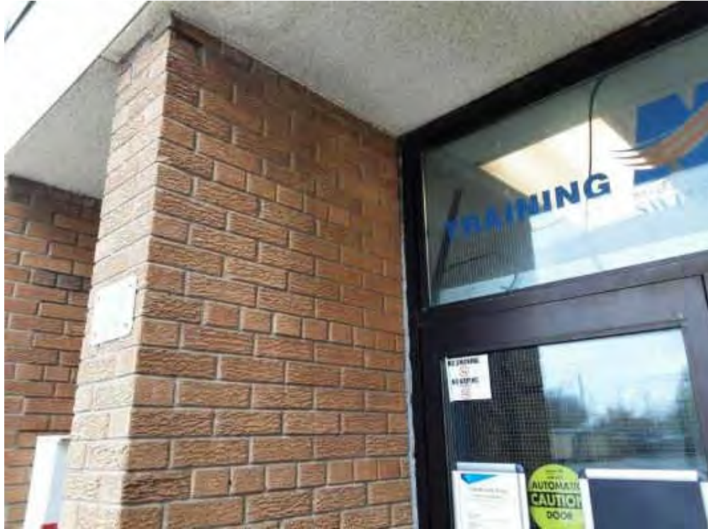
V0013 (Confirmed Asbestos), Other, Door, Caulking, Exterior (Location #: 14) Grey, N wall, main entrance
