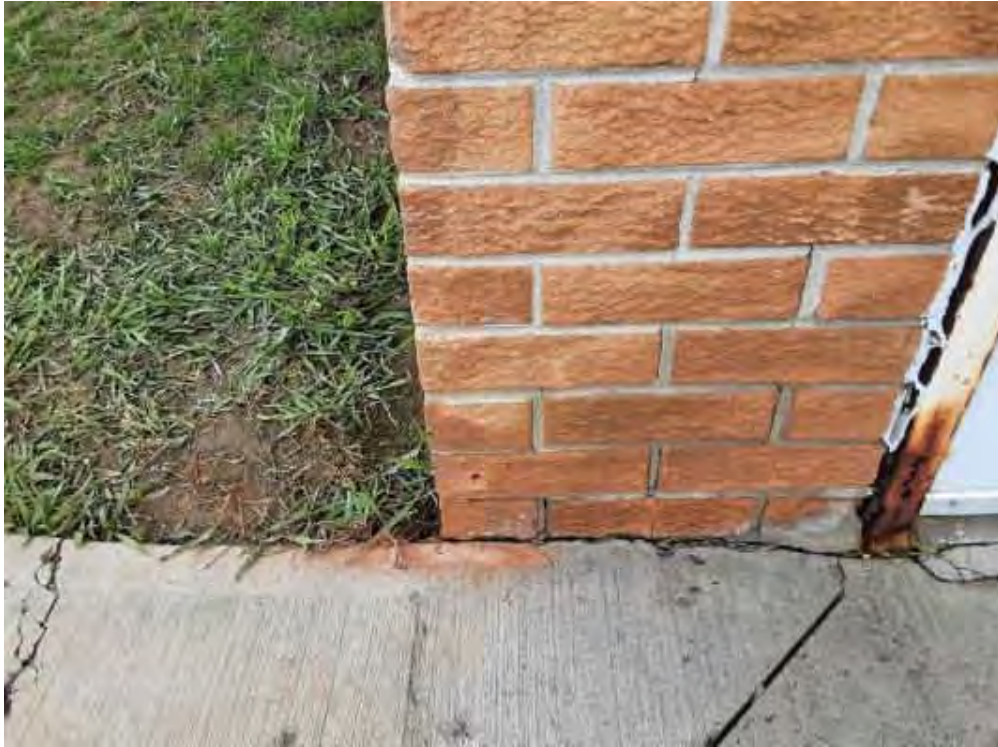
V0000 (None), Wall, Vermiculite, Exterior (Location #: 14) 5 Drill holes, no vermiculite, N wall, NE wall, S wall, SW wall, brick wall
