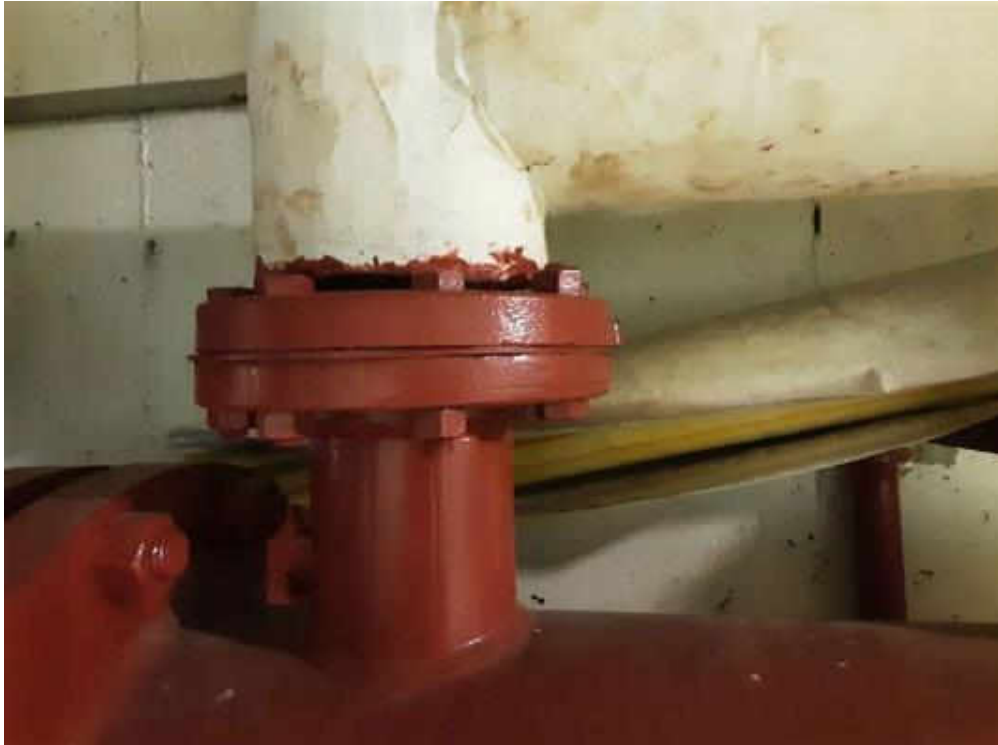
V9500 (Presumed Asbestos), Mechanical Equipment, Gasket, Filter Room (Location #: 2)
