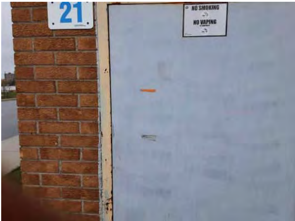
S0013A (Confirmed Asbestos), Other, Door, Caulking, Exterior (Location #: 14) Grey
