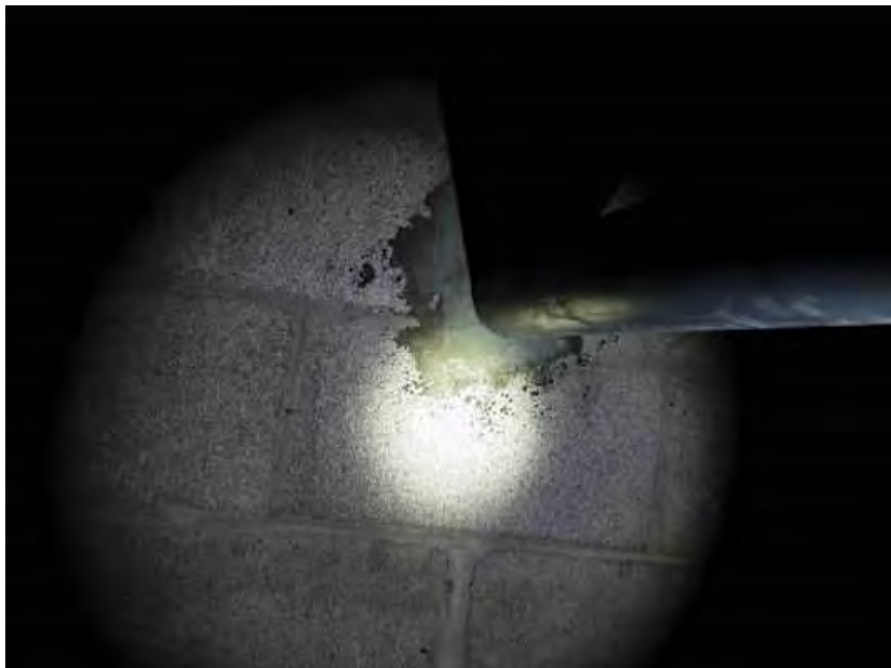
S0002C (None), Wall, Fire Stop, Cement Product, Tunnel Area (Location #: 3)
