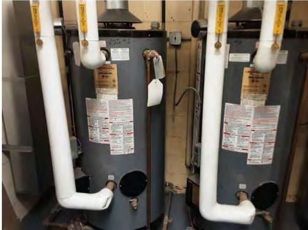
V0000 (None), Piping, Fibreglass, Custodian (Location #: 29)
