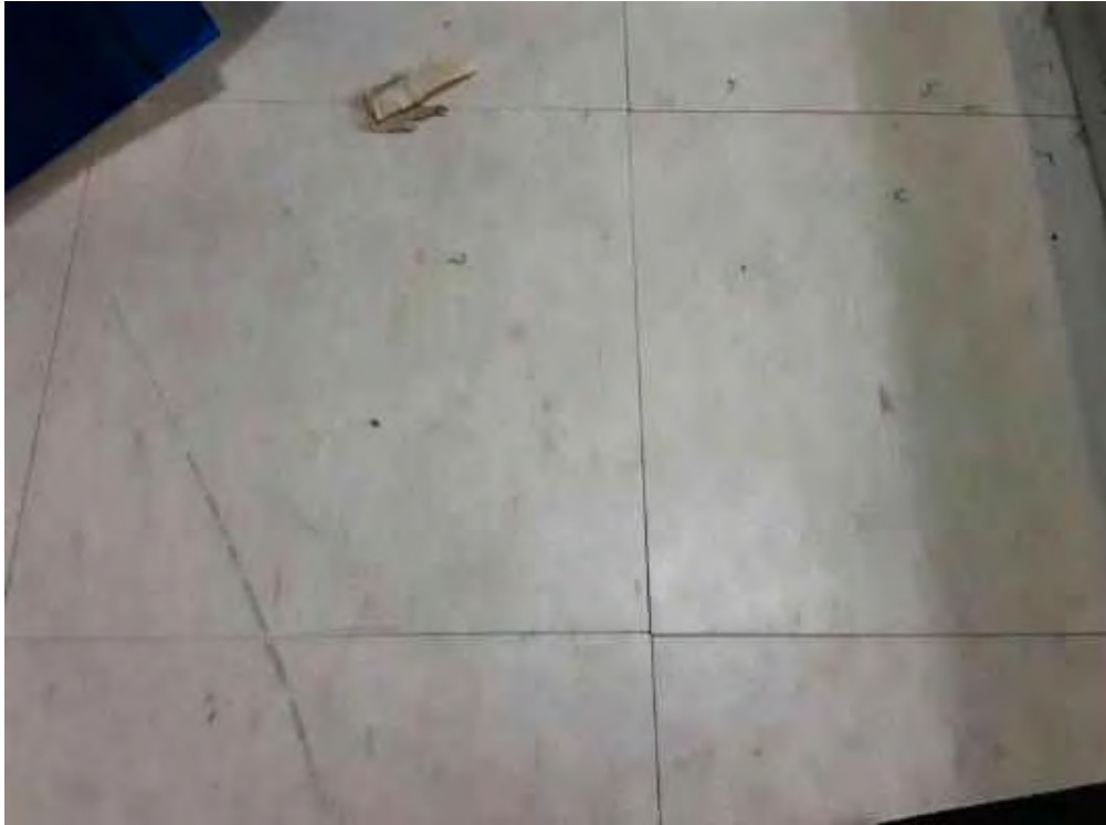
S0005A (None), Floor, All, Vinyl Floor Tile and Mastic, East Stairwell (Location #: 5)
