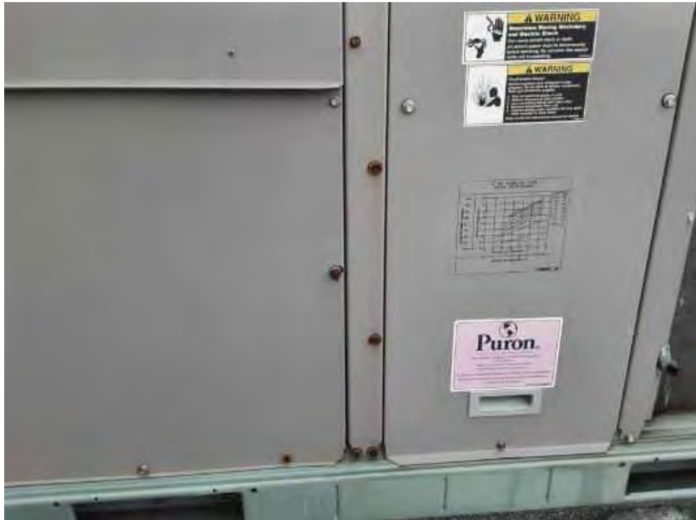
V0000 (None), Mechanical Equipment, Air Handling Unit, Not Insulated, Lower Roof (Location #: 17)
