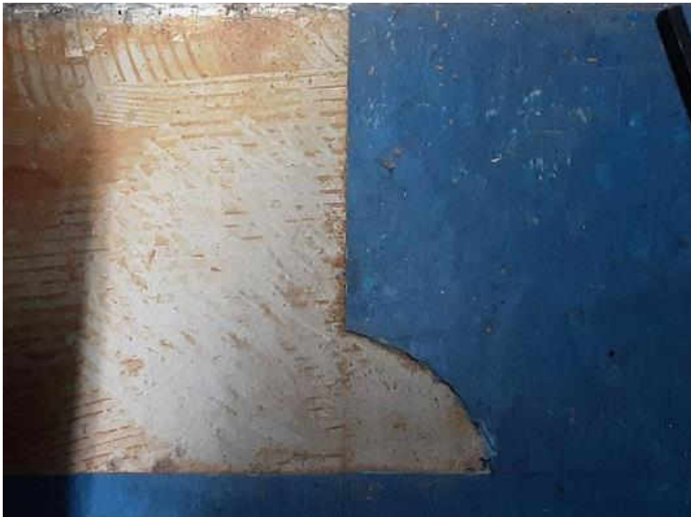
S0020B (None), Floor, Vinyl Floor Tile and Mastic, Equipment Storage (Location #: 16) Yellow mastic
