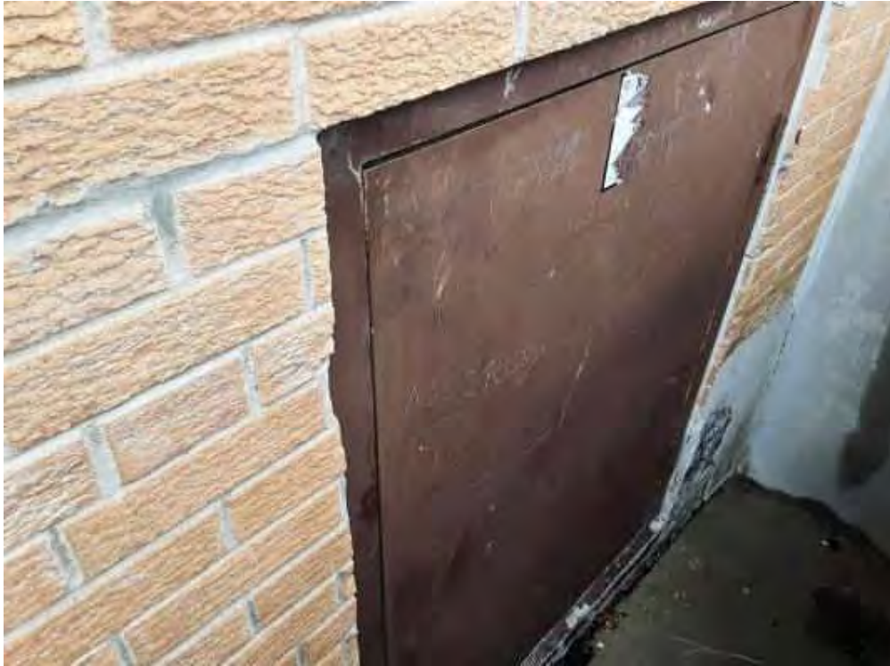
S0013B (Confirmed Asbestos), Other, Door, Caulking, Exterior (Location #: 14) Grey, back door NE wall
