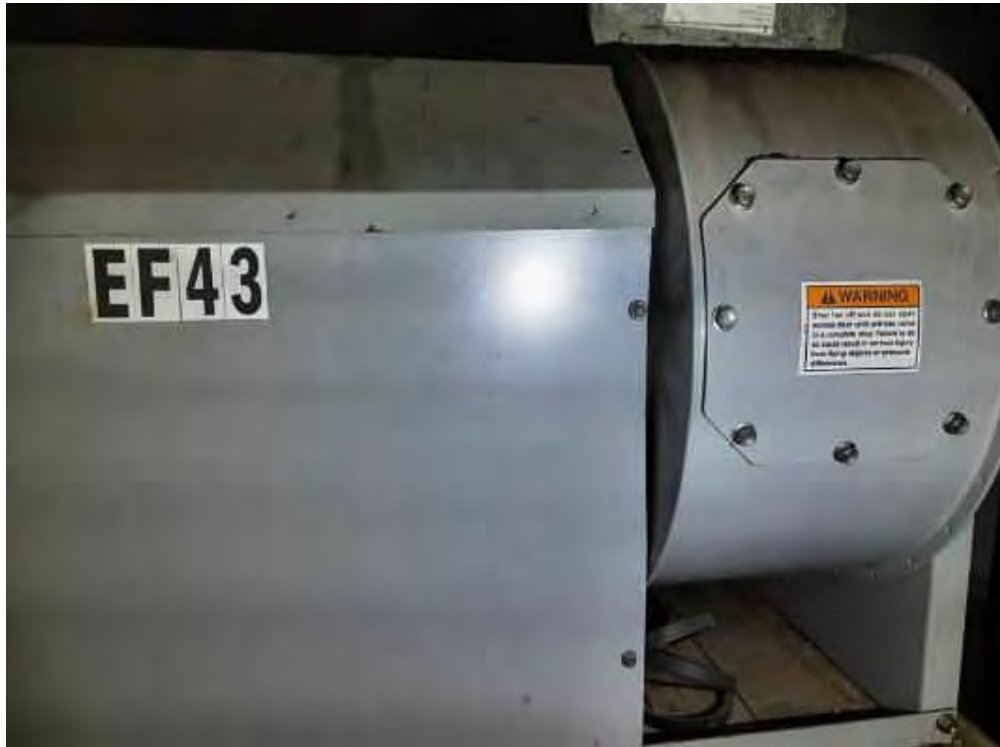
V0000 (None), Mechanical Equipment, Fan Unit, Not Insulated, Mechanical Room And Stairwell (Location #: 21)
