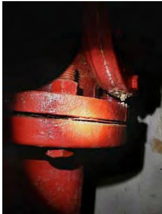
V9500 (Presumed Asbestos), Mechanical Equipment, Gasket, Filter Room (Location #: 2)
