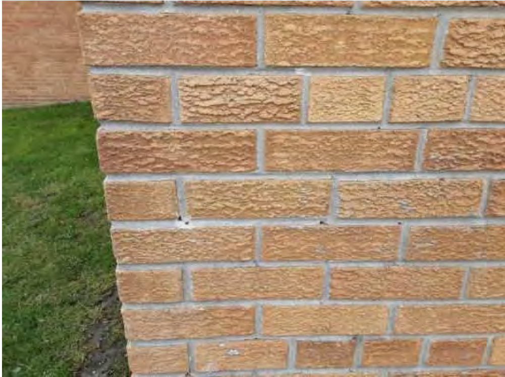
S0012A (Confirmed Asbestos), Wall, Mortar, Exterior (Location #: 14) Brick
