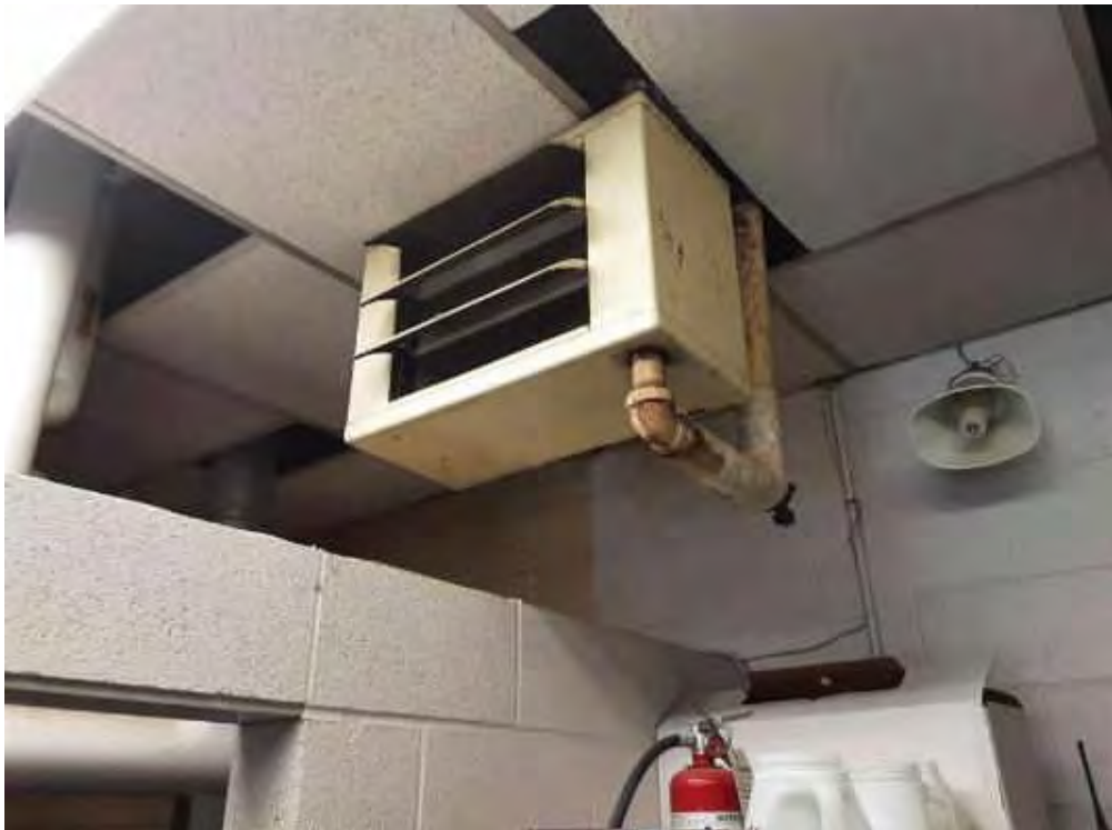
V0000 (None), Mechanical Equipment, Fan Unit, Not Insulated, Custodian (Location #: 29)
