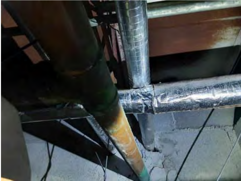
V0000 (Non e), Piping, Not Insulated, Men's Washroom (Location # 22)
