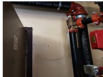
Photo 17: Asbestos-containing drywall joint compound on wall finishes present in the Custodian (Loc. 29).
