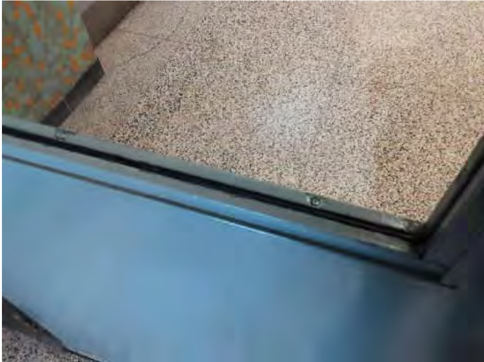
S0017A (None), Other, Door, Caulking, Entrance Vestibule (Location #: 6) Black, between door frame and glass
