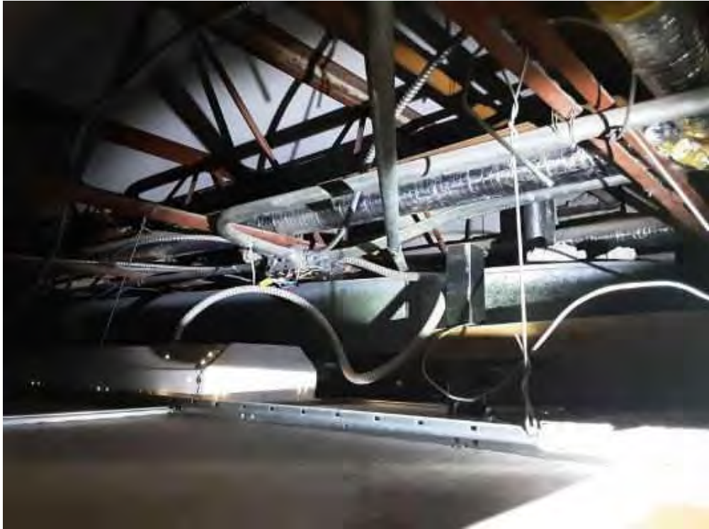
V0000 (None), Duct, All, Not Insulated, Men's Washroom (Location #: 10)
