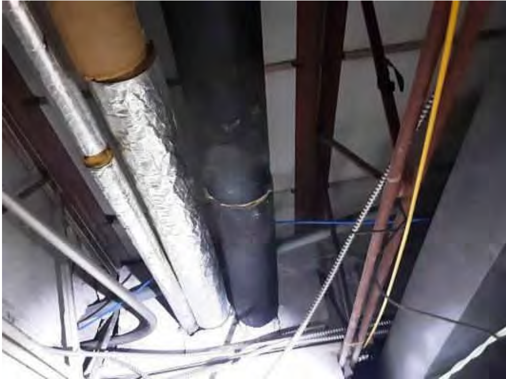
V0000 (None), Piping, Fibreglass, Supervisor Office (Location #: 15)
