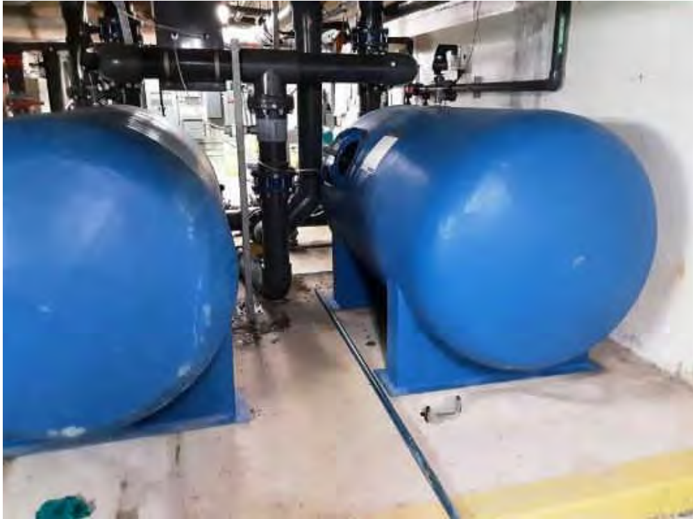
V0000 (None), Mechanical Equipment, Filters, Not Insulated, Filter Room (Location #: 2)
