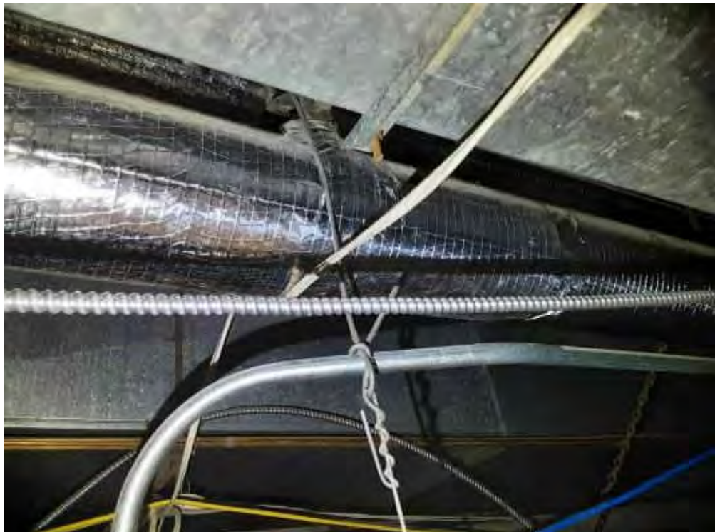
V0000 (None), Piping, Fibreglass, Corridor (Location #: 27)
