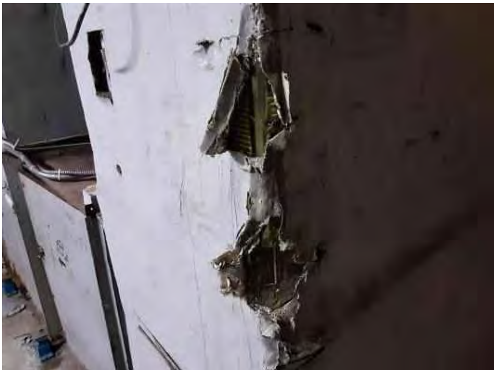
V0000 (None), Mechanical Equipment, Air Handling Unit, Fibreglass, Fan Room (Location #: 1)
