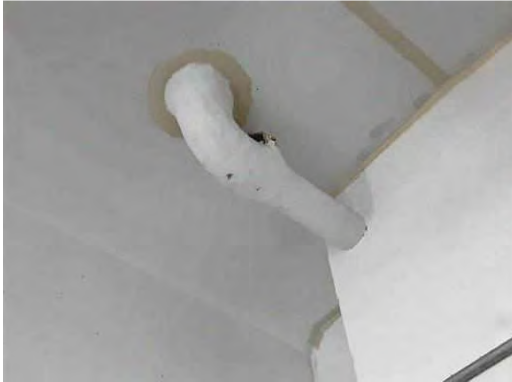
S0026A (Confirmed Asbestos), Piping, Parging Cement, Balcony (Location #: 4)
