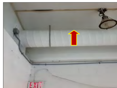
Photo 6: Uninsulated duct present in the Filter Room (Loc. 2).
