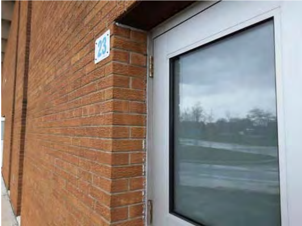
V0013 (Confirmed Asbestos), Other, Door, Caulking, Exterior (Location #: 14) Grey, S wall
