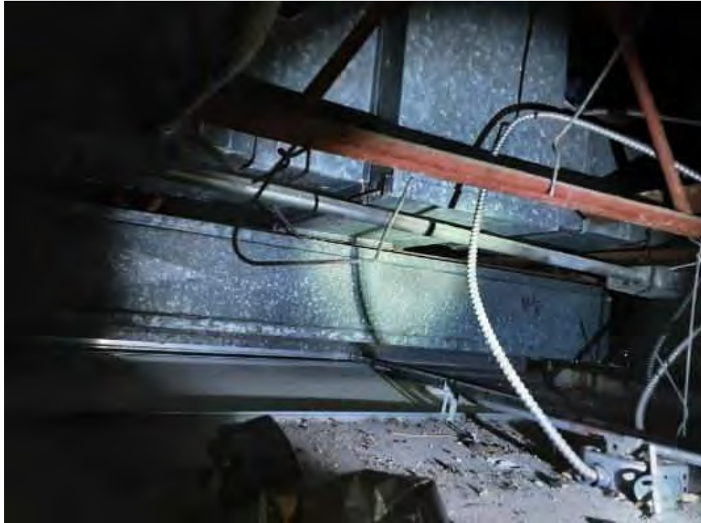
V0000 (None), Duct, All, Not Insulated, Women's Change Room (Location #: 12)
