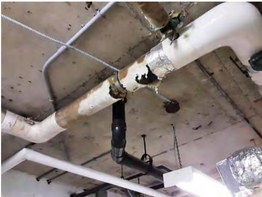
V0000 (None), Piping, All, Fibreglass, Filter Room (Location #: 2)
