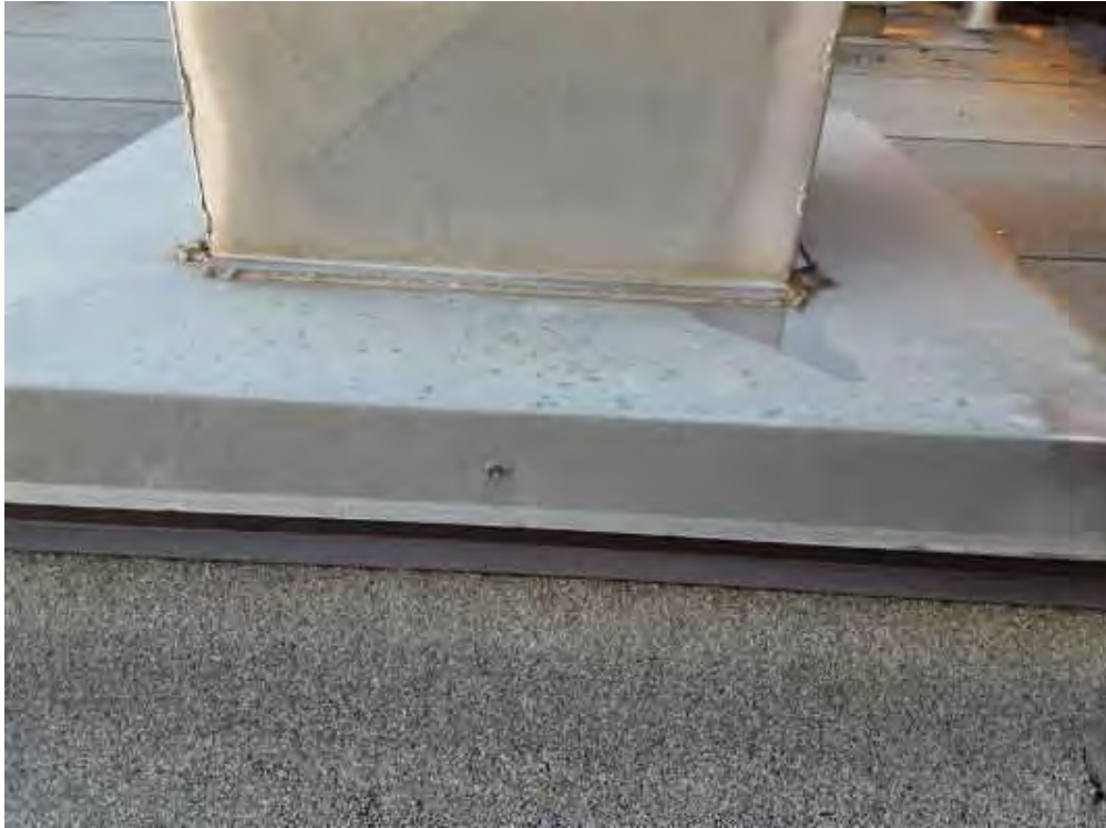
V0000 (None), Duct, Exhaust, Not Insulated, Lower Roof (Location #: 17)
