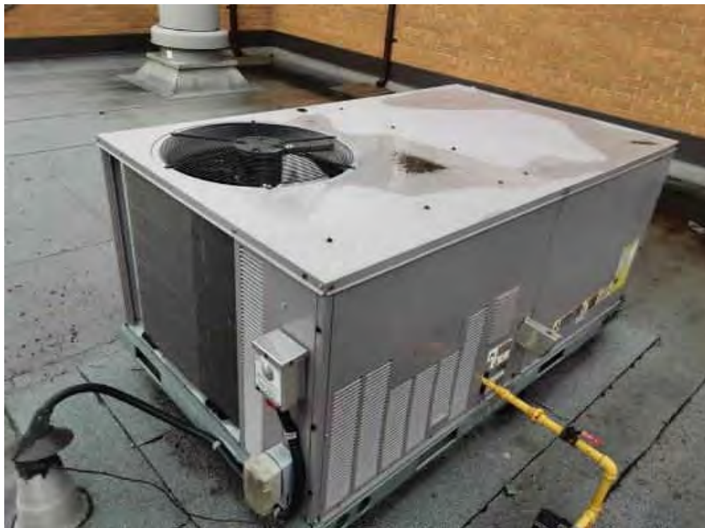
V0000 (None), Mechanical Equipment, Air Handling Unit, Not Insulated, Lower Roof (Location #: 17)
