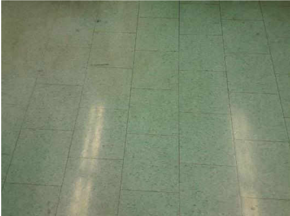
S0030A (None), Floor, All, Vinyl Floor Tile and Mastic, Phys. Ed. Room (Location #: 24) Red mastic
