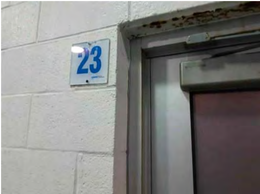
V0013 (Confirmed Asbestos), Other, Door, Caulking, In door Pool (Location #: 13) Grey, S wall, between wall and door frame
