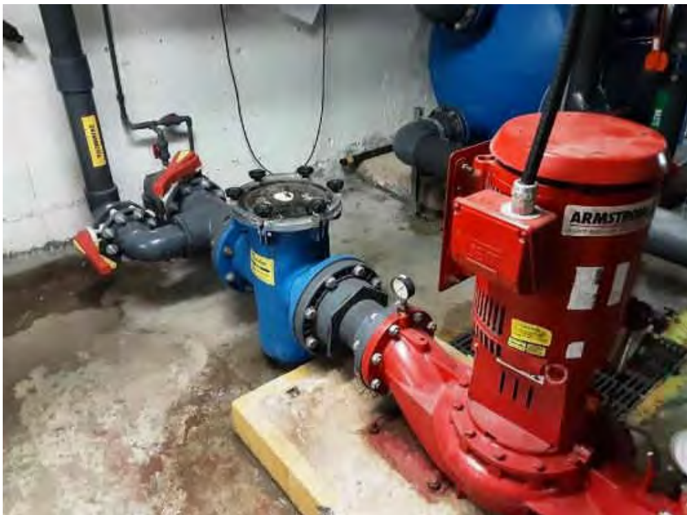
V0000 (None), Mechanical Equipment, Pump, Not Insulated, Filter Room (Location #: 2)
