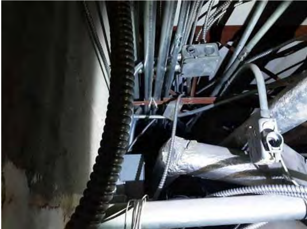
V0000 (None), Piping, Fibreglass, Hallway (Location #: 28)
