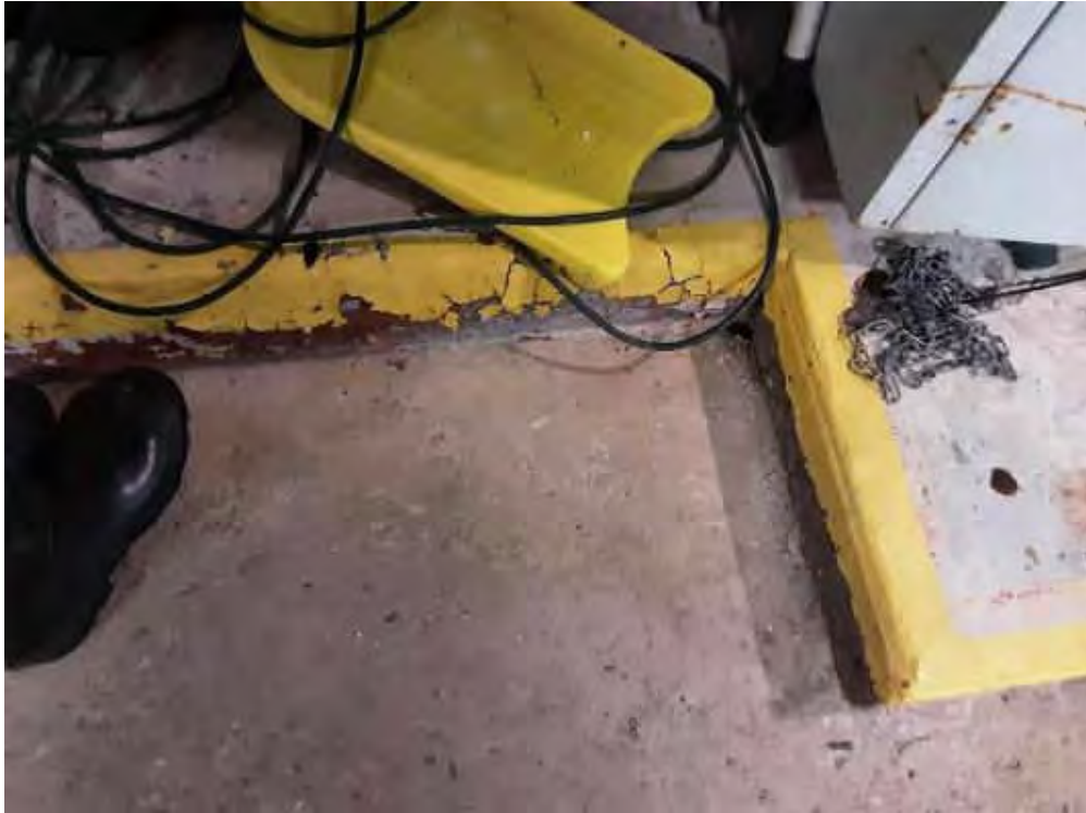
Concrete (poured), Yellow, L0006(Lead (High)), Filter Room (Location #: 2)
