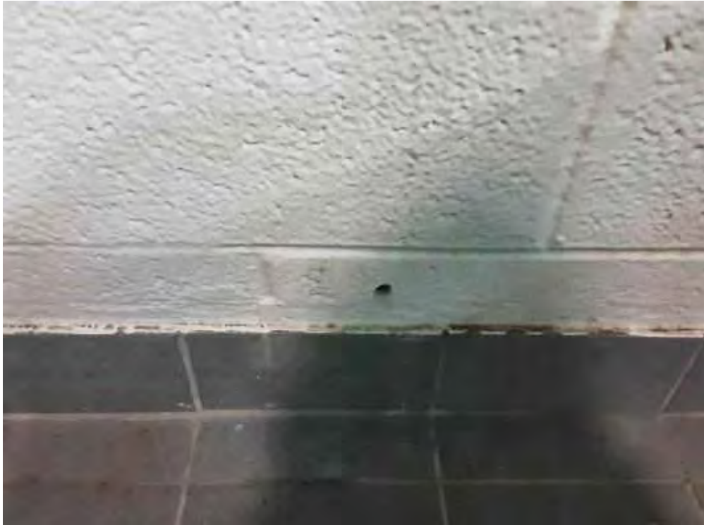
V0000 (None), Wall, Vermiculite/concrete block walls, In do or Pool (Location #: 13) 4 Drill holes, no vermiculite, N wall, E wall, W wall, S wall
