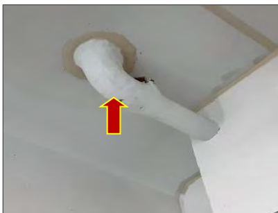
Photo 3: Asbestos containing parging cement insulated pipe present in the Balcony (Loc.4).
