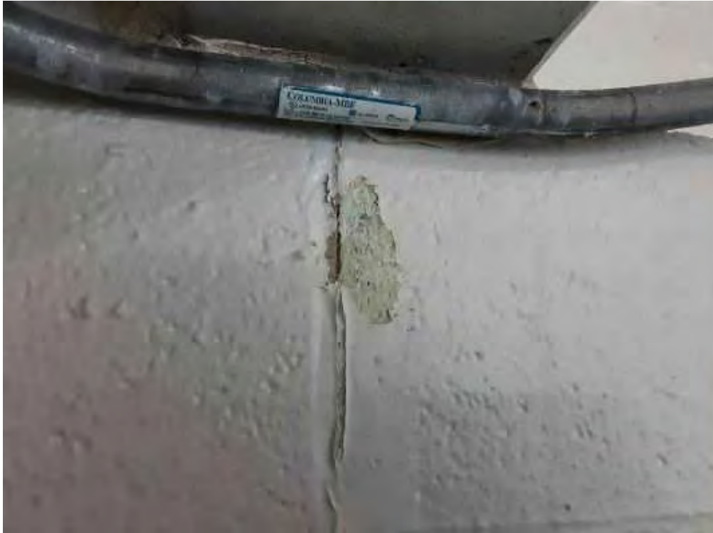
Masonry, Green, L0010(Lead (High)), Balcony (Location #: 4)
