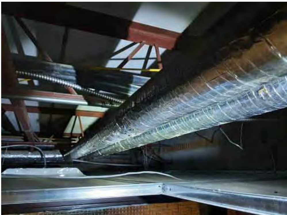
V0000 (None), Piping, All, Fibreglass, Entrance Vestibule (Location #: 6)
