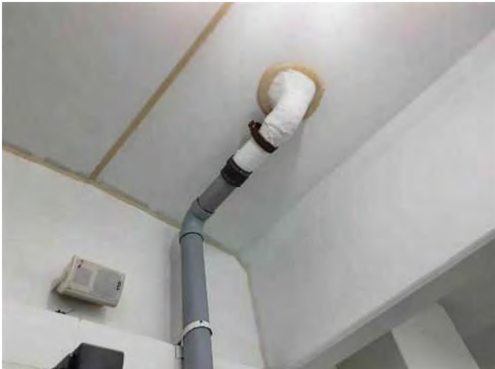
V0000 (None), Piping, Rain Water Leader, Polyvinyl chloride (PVC), Balcony (Location #: 4)
