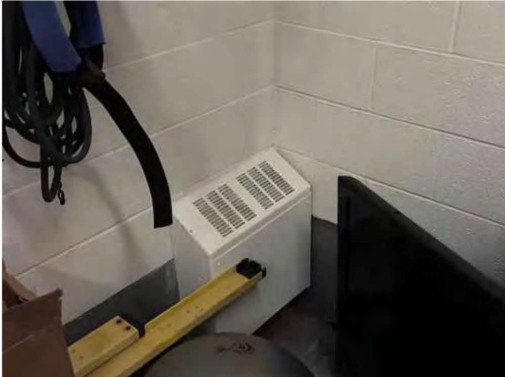
V0000 (None), Mechanical Equipment, Unit Heater, Not Insulated, Equipment Room 2 (Location #: 20)
