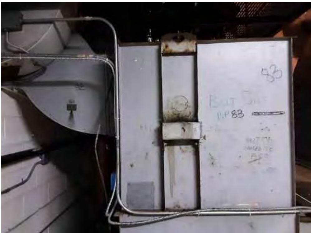
V0000 (No ne), Mechanical Equipment, Air Handling Unit, Not Insulated, Fan Room (Location #: 1)
