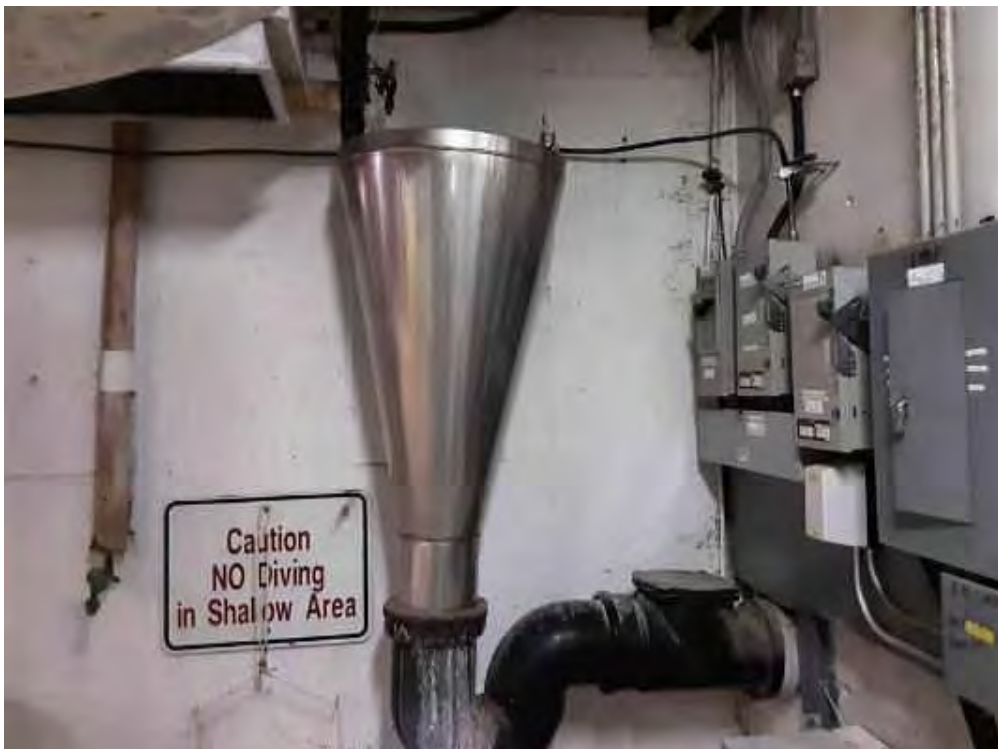
V0000 (None), Piping, Not Insulated, Filter Room (Location #: 2)
