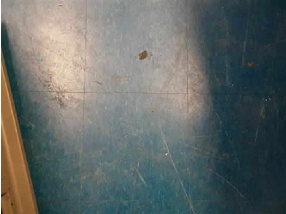
S0020A (None), Floor, Vinyl Floor Tile and Mastic, Equipment Storage (Location #: 16) Yellow mastic
