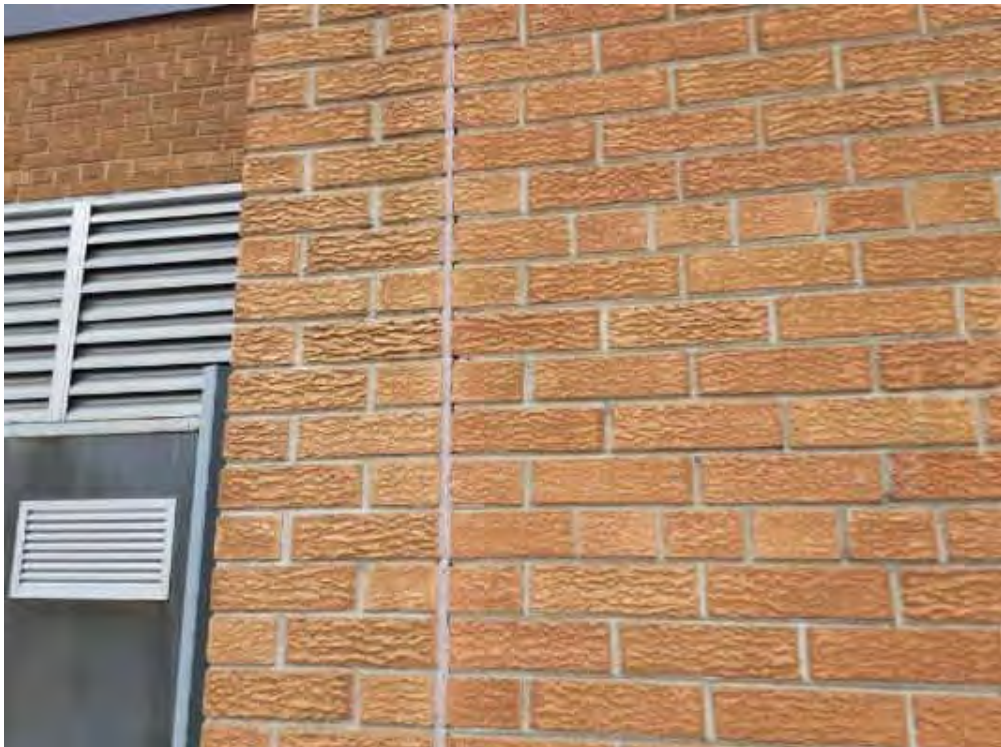
S0011C (None), Wall, Expansion Joint, Caulking, Exterior (Location #: 14) Light red, S wall
