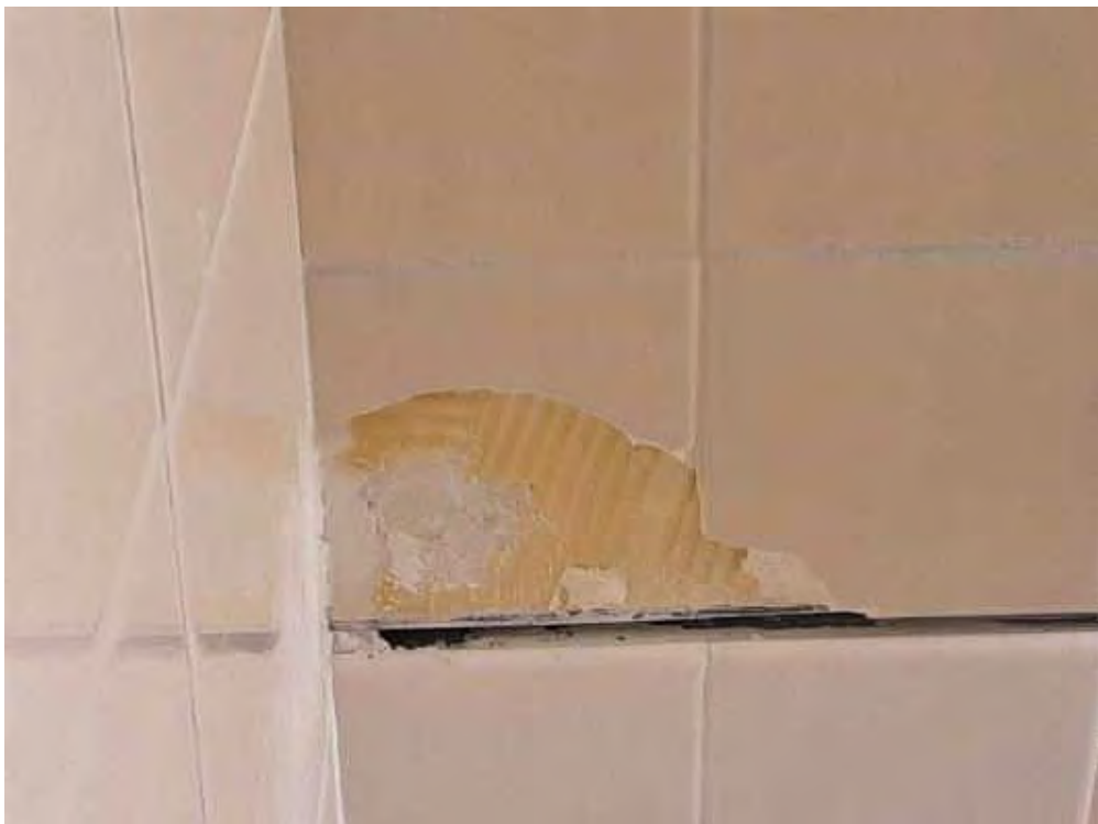
S0018A (None), Ceiling, Mastic, Men's Change Room (Location #: 9) Multiple layers of plaster underneath
