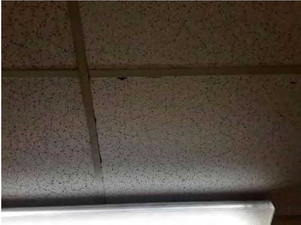
S0031A (None), Ceiling, All, Ceiling Tiles (lay-in), Corridor (Location #: 27) Water staining observed
