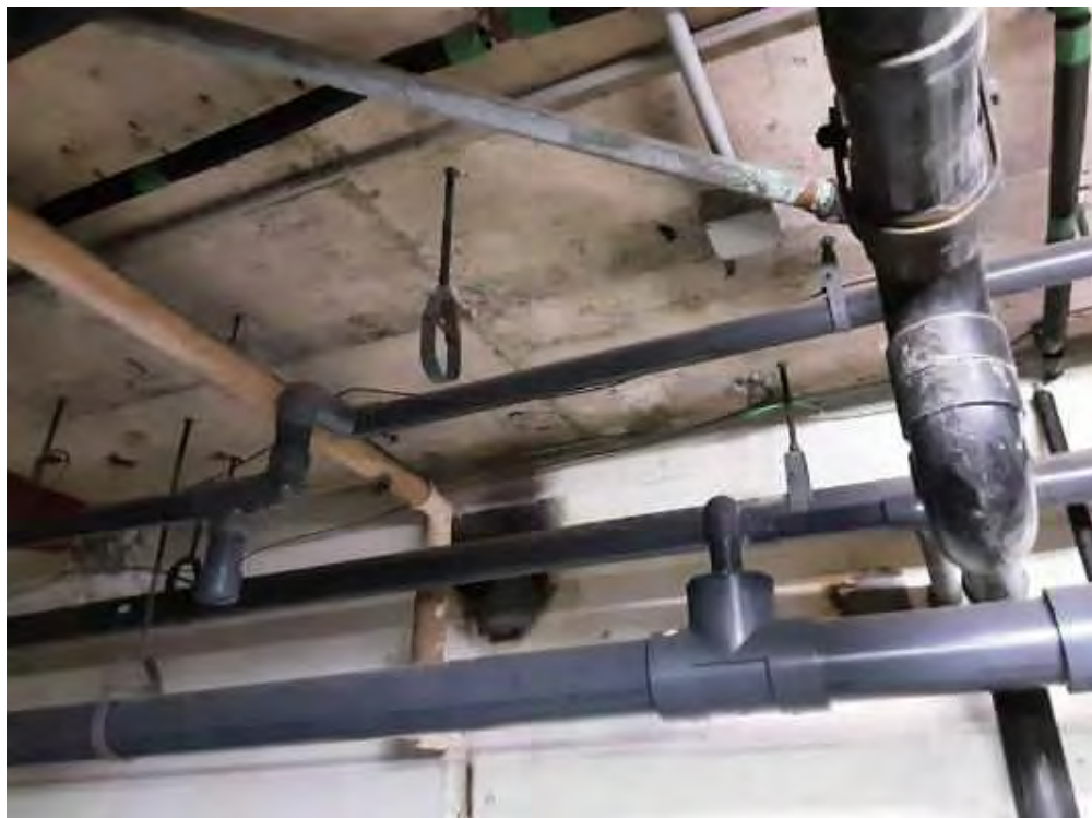
V0000 (None), Piping, Polyvinyl chloride (PVC), Filter Room (Location #: 2) Inlet, discharge, vacuum, skimmer, waste
