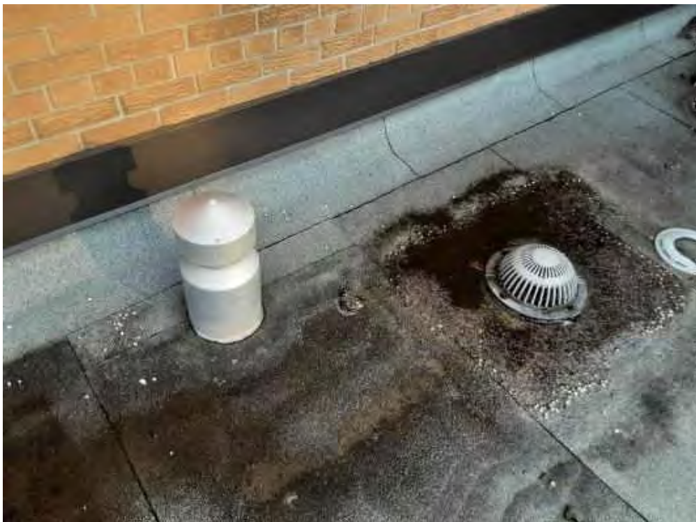
V0000 (None), Mechanical Equipment, Roof Hopper (Drain), Not Insulated, Lower Roof (Location #: 17)
