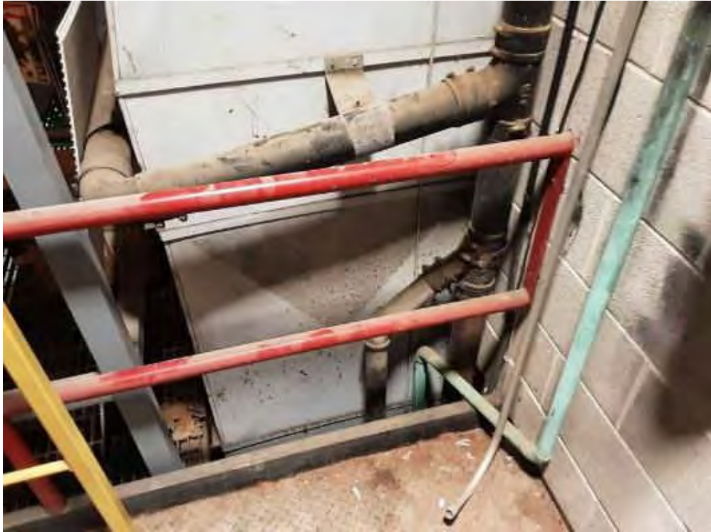
Metal, Red, V0003(Lead (High)), Mechanical Room And Stairwell (Location #: 21)
