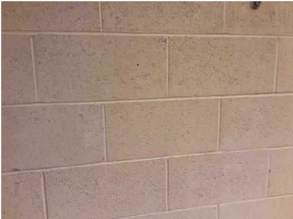
S0028A (Con firmed Asbestos), Wall, Mortar, Gym Storage (Location #: 25) Block wall
