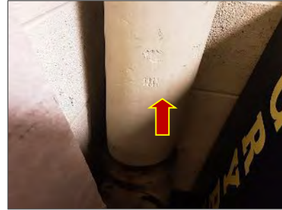
Photo 19: Presumed asbestos cement pipe (Transite) present in the Gym storage (Loc. 25).
