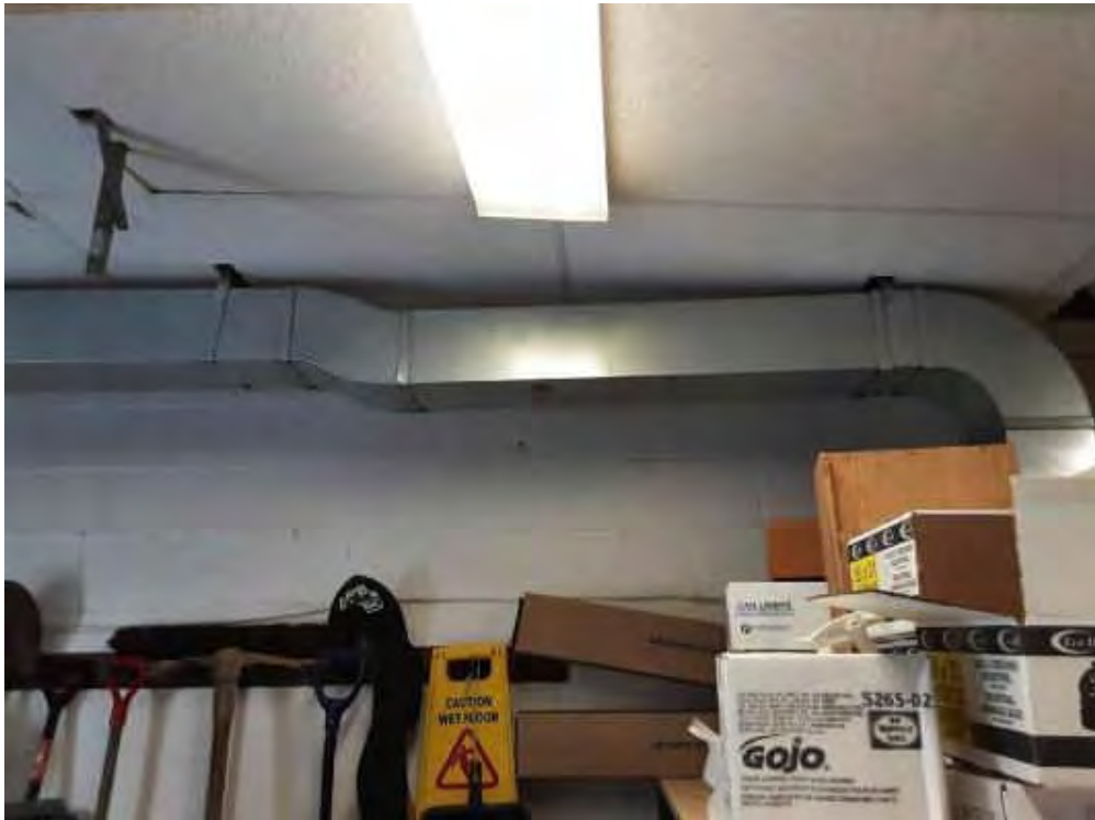
V0000 (None), Duct, All, Not Insulated, Custodian (Location #: 29)
