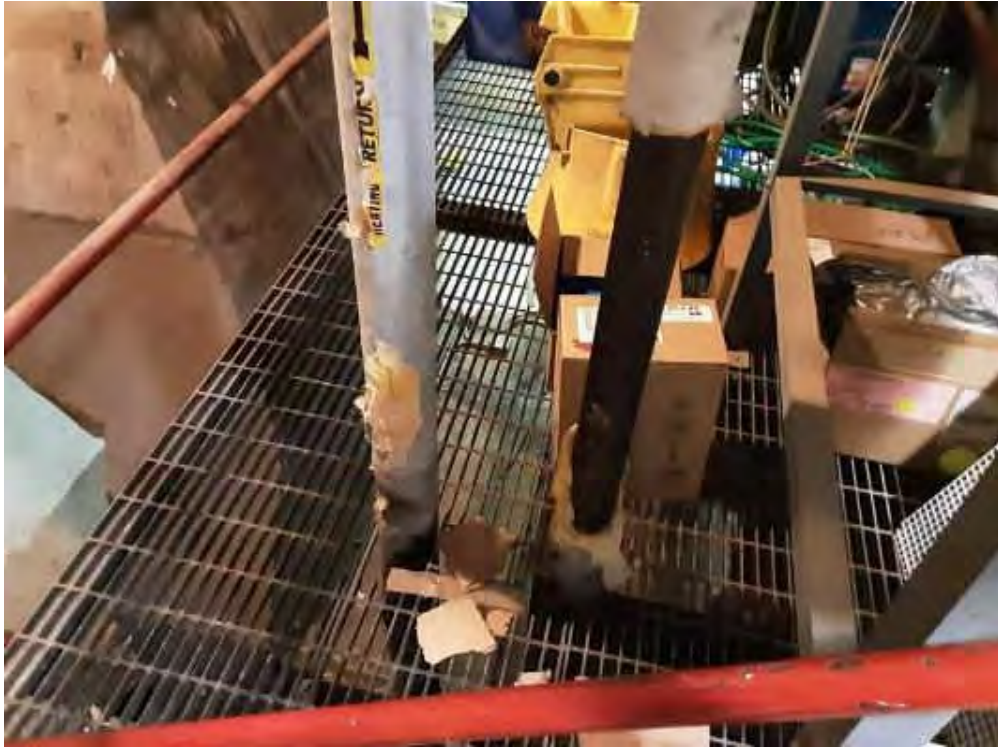
V0000 (None), Piping, All, Fibreglass, Mechanical Room And Stairwell (Location #: 21)
