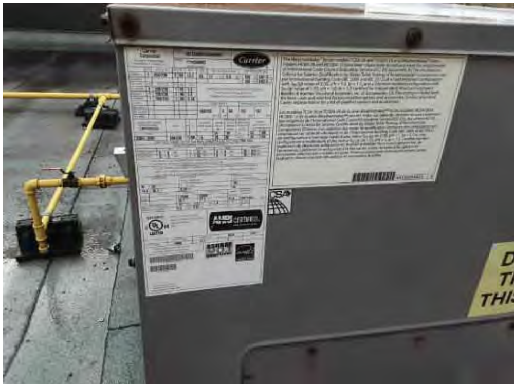
V0000 (None), Mechanical Equipment, Air Handling Unit, Not Insulated, Lower Roof (Location #: 17)
