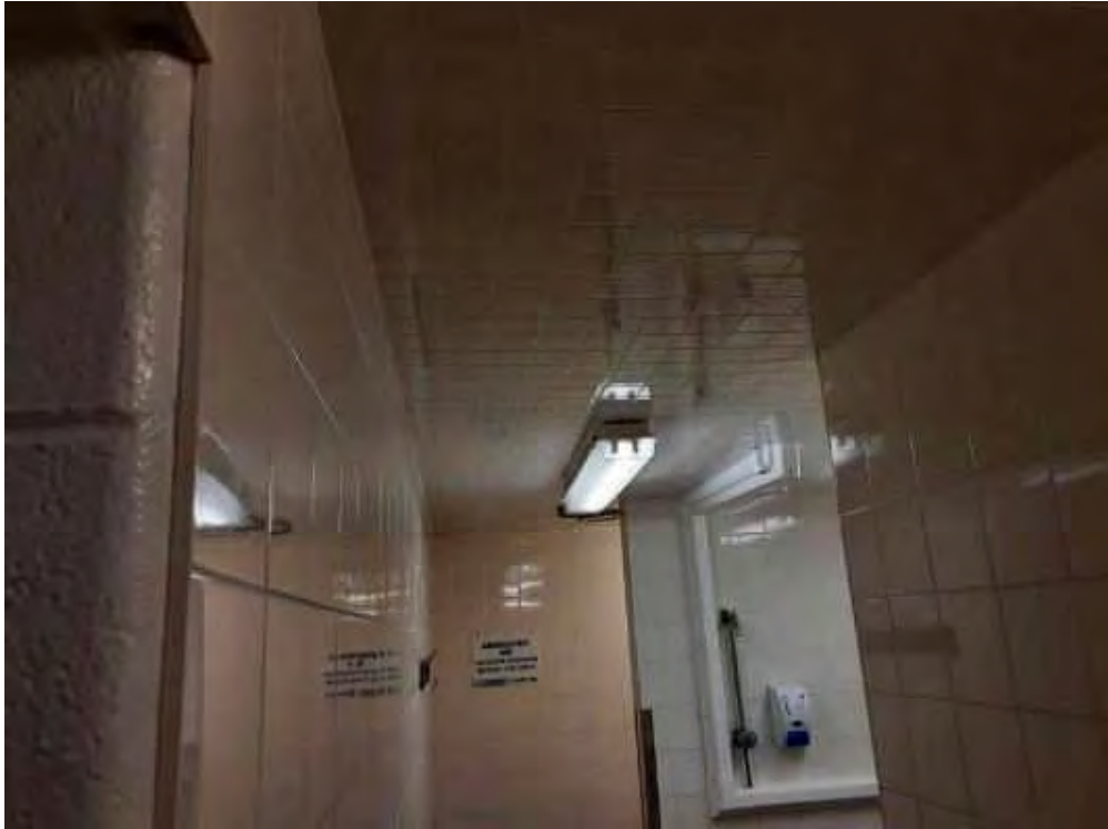
S0018B (None), Ceiling, Mastic, Men's Change Room (Location #: 9) Multiple layers of plaster underneath
