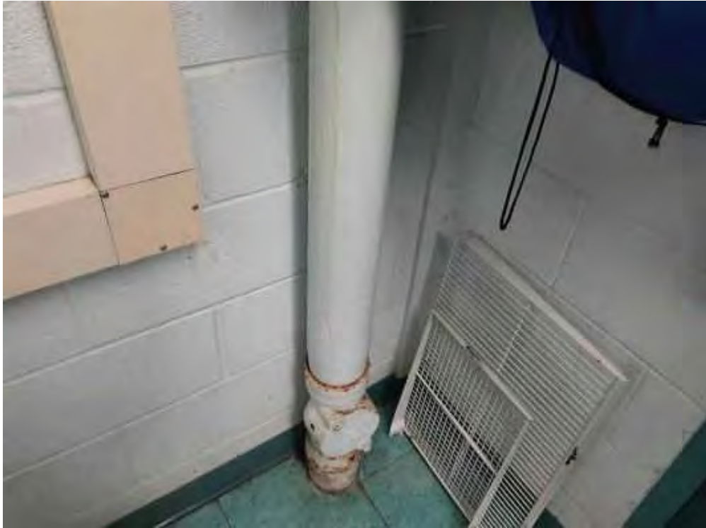
V9000 (Confirmed Asbestos), Piping, All, Cement Product, Phys. Ed. Room (Location #: 24) Transit3
