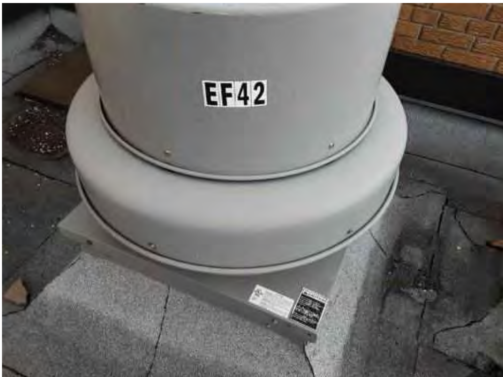
V0000 (None), Mechanical Equipment, Fan Unit, Not Insulated, Lower Roof (Location #: 17) Ventilator
