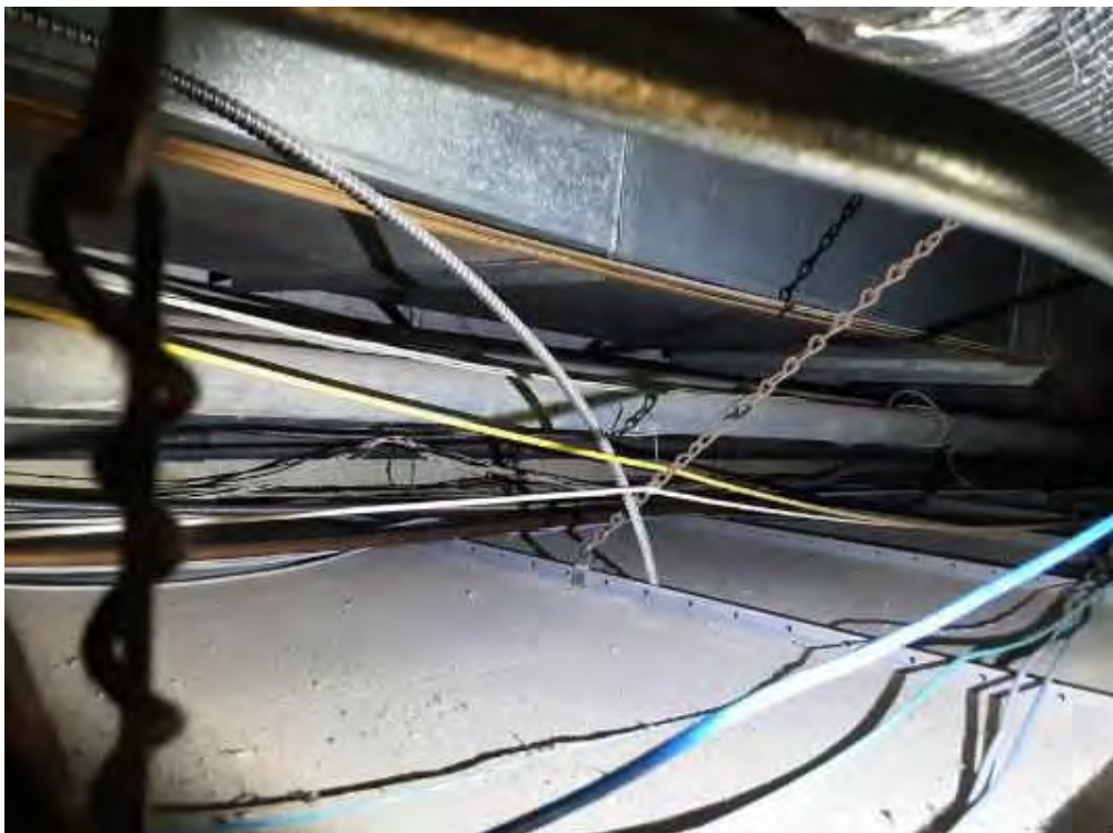
V0000 (None), Piping, All, Not Insulated, Corridor (Location #: 27)
