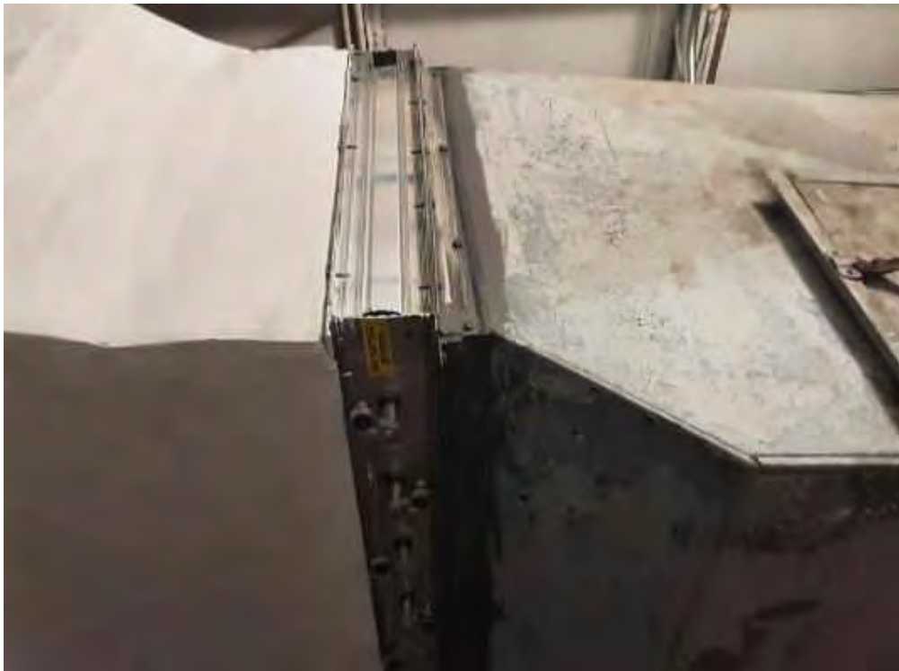
S0023A (None), Duct, Mastic, Mechanical Room And Stairwell (Location #: 21) Grey, 4 connectors
