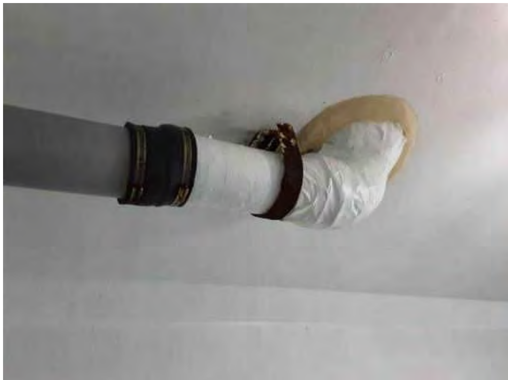
S0026B (Confirmed Asbestos), Piping, Parging Cement, Balcony (Location #: 4)
