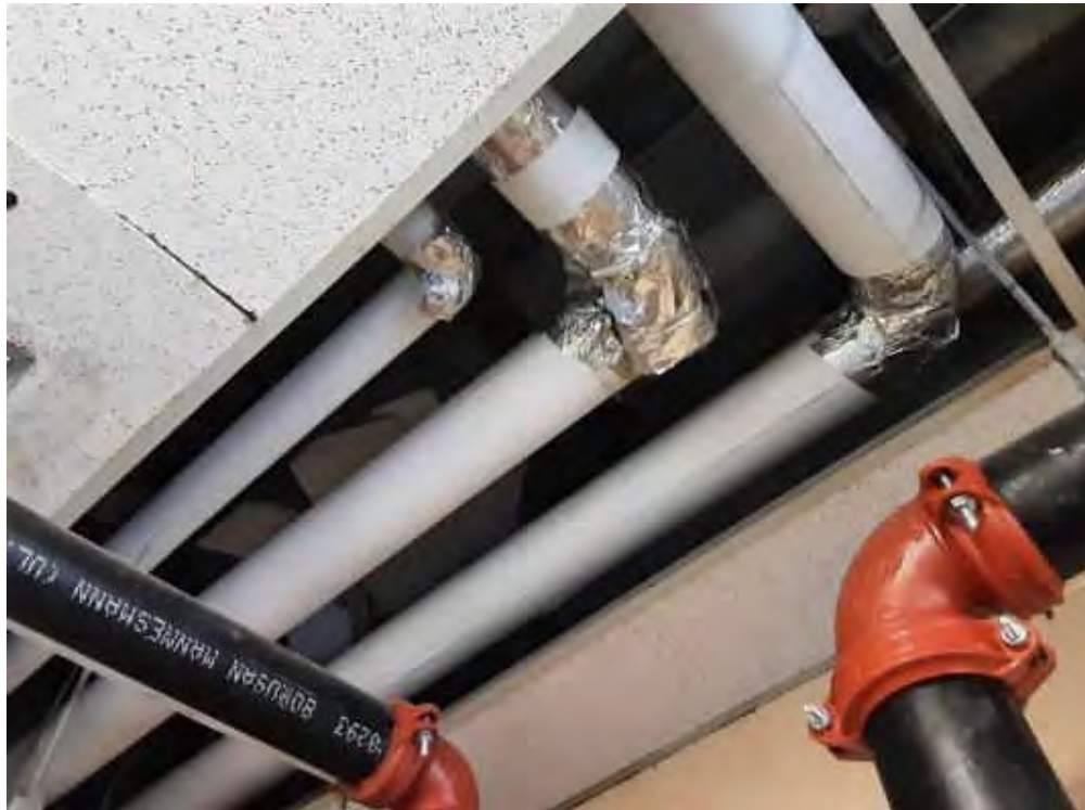
V0000 (None), Piping, Fibreglass, Custodian (Location #: 29)
