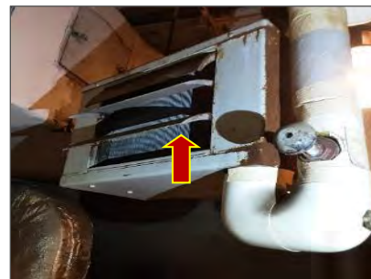
Photo 11: Uninsulated fan unit present in the Mechanical Room and Stairwell (Loc. 21).
