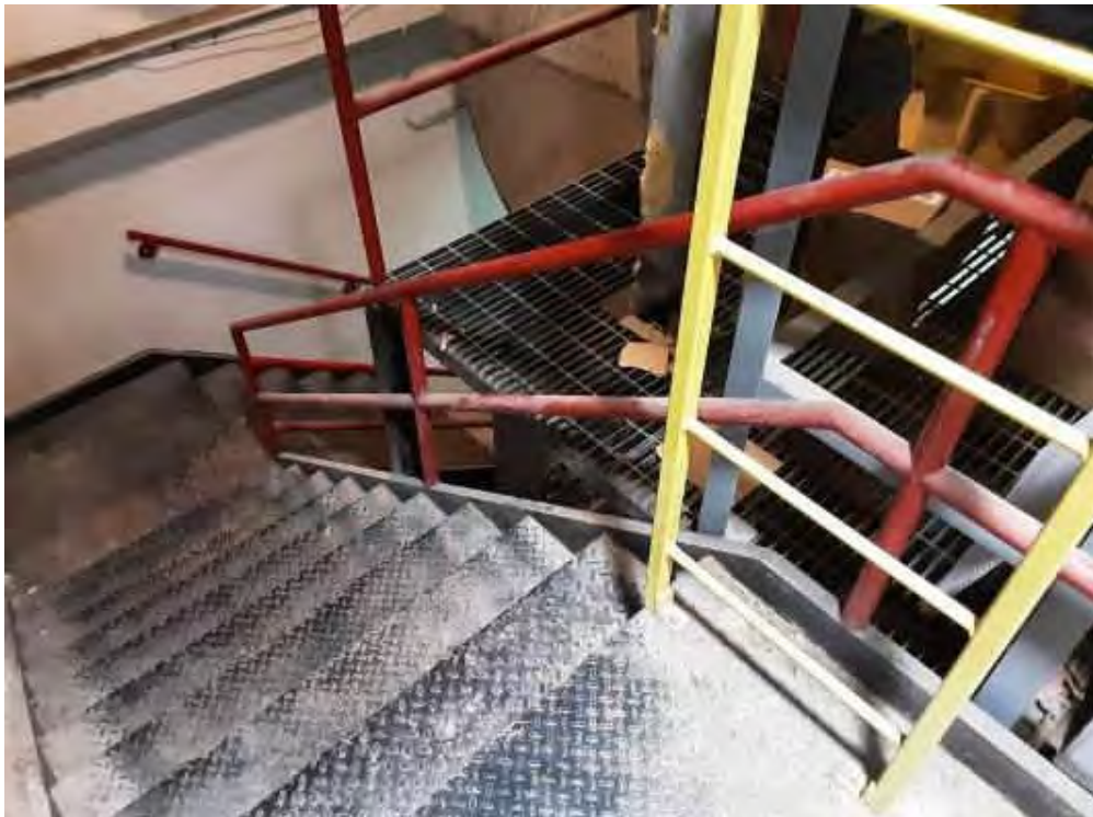
Metal, Yellow, V0006(Lead (High)), Mechanical Room And Stairwell (Location #: 21)
