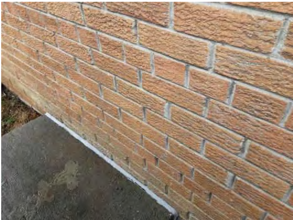
S0013C (Confirmed Asbestos), Wall, Expansion Joint, Caulking, Exterior (Location #: 14) Grey, NE wall
