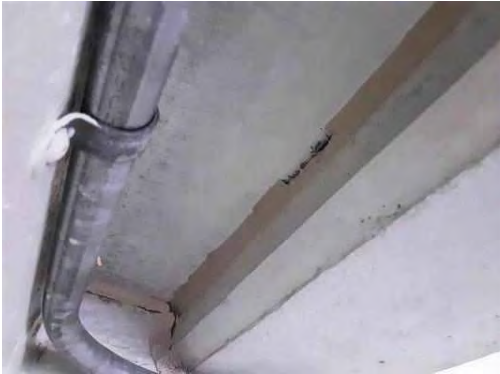
S0004A (None), Wall, Expansion Joint, Caulking, Balcony (Location #: 4) Off white, some underneath beige caulking
