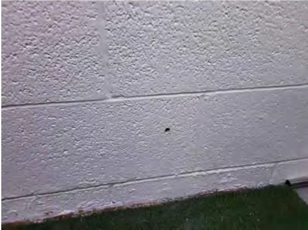
V0000 (None), Wall, Vermiculite/concrete block walls, Balcony (Location #: 4) 2 Drill holes, no vermiculite
