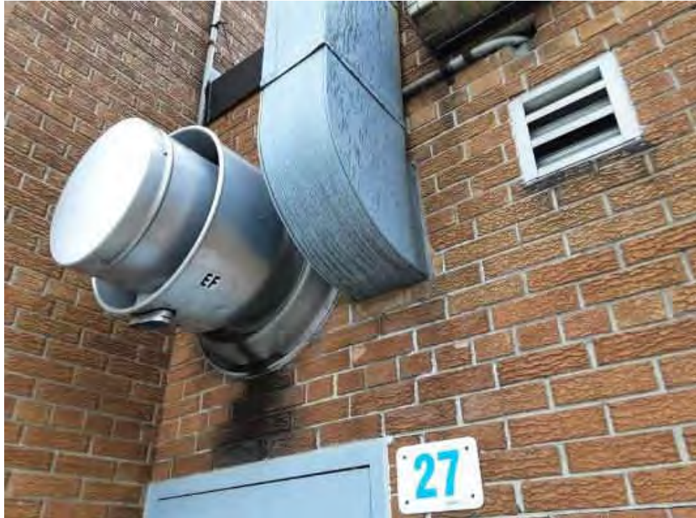
V0000 (None), Duct, Not Insulated, Exterior (Location #: 14)
