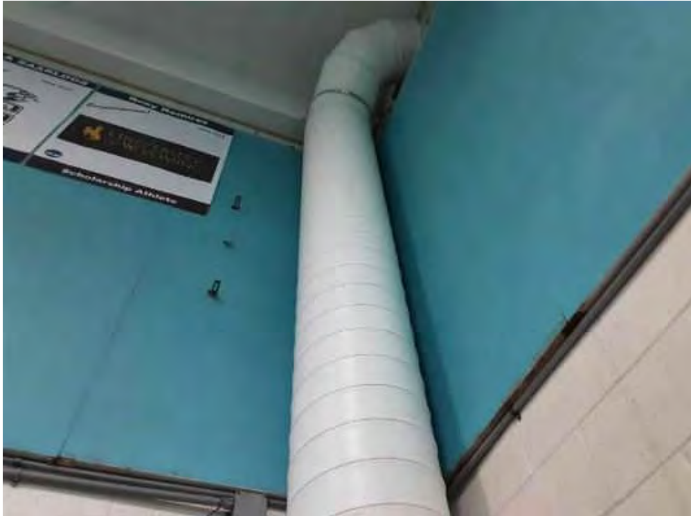
V0000 (None), Duct, All, Not Insulated, Indoor Pool (Location #: 13)
