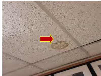
Photo 24: View of water-stained acoustic ceiling tiles present in the Corridor (Loc. 27).
