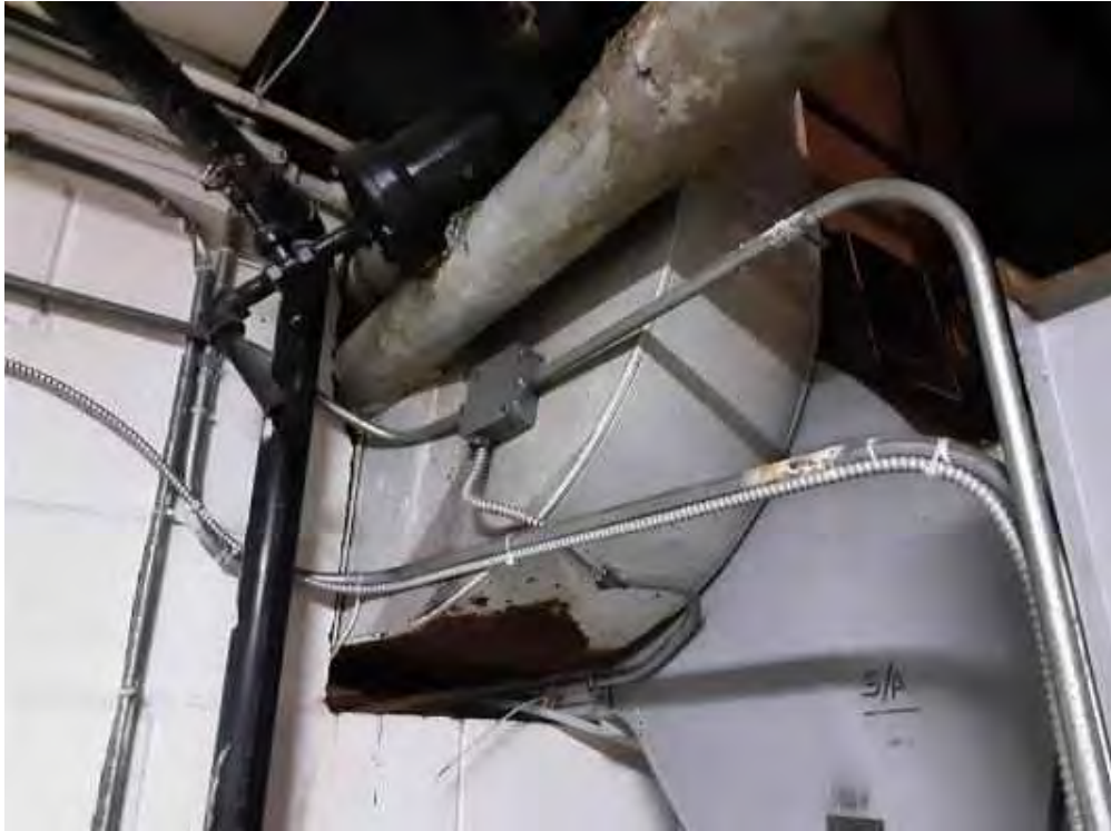
V0000 (None), Duct, All, Not Insulated, Fan Room (Location #: 1)
