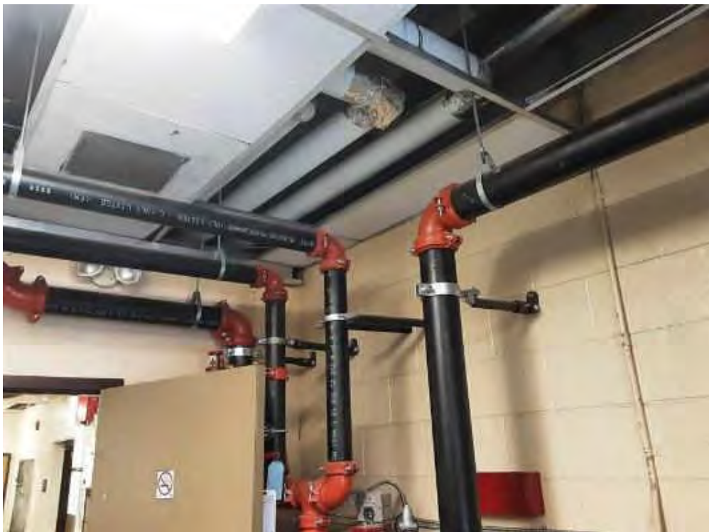
V0000 (None), Piping, All, Not Insulated, Custodian (Location #: 29)
