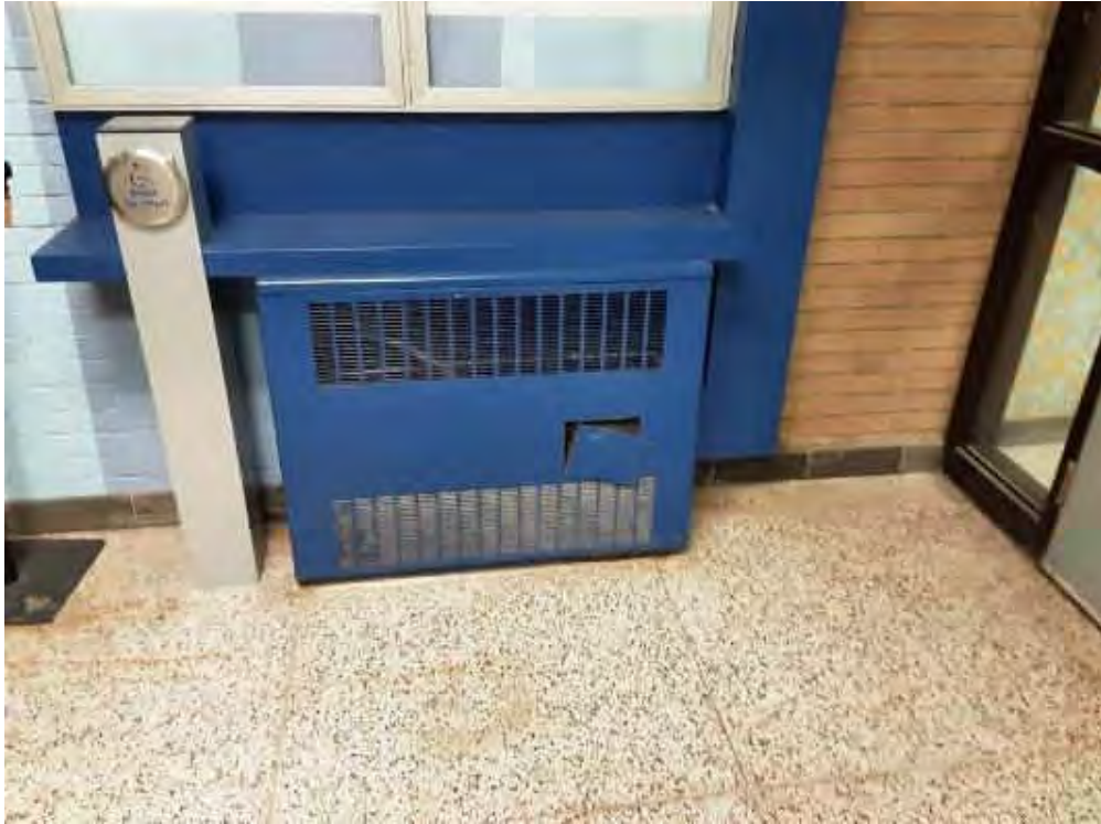
V0000 (None), Mechanical Equipment, Unit Heater, Not Insulated, Entrance Vestibule (Location #: 6)
