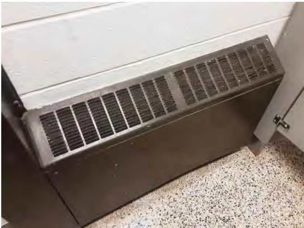
V0000 (None), Mechanical Equipment, Unit Heater, Not Insulated, Men's Washroom (Location #: 10)
