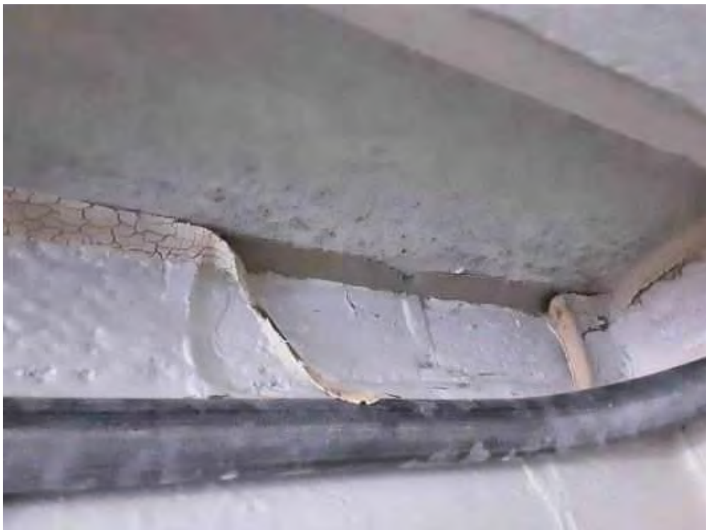
S0004C (None), Wall, Expansion Joint, Caulking, Balcony (Location #: 4) Off white, underneath beige caulking
