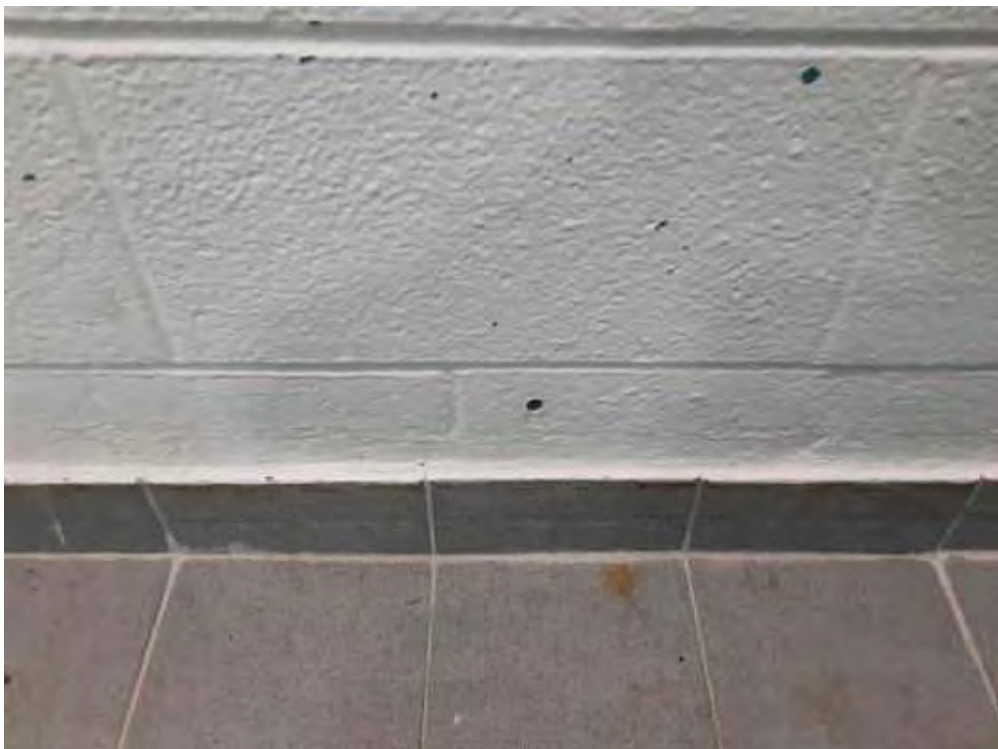
V0000 (None), Wall, Vermiculite/concrete block walls, In do or Pool (Location #: 13) 4 Drill holes, no vermiculite, N wall, E wall, W wall, S wall
