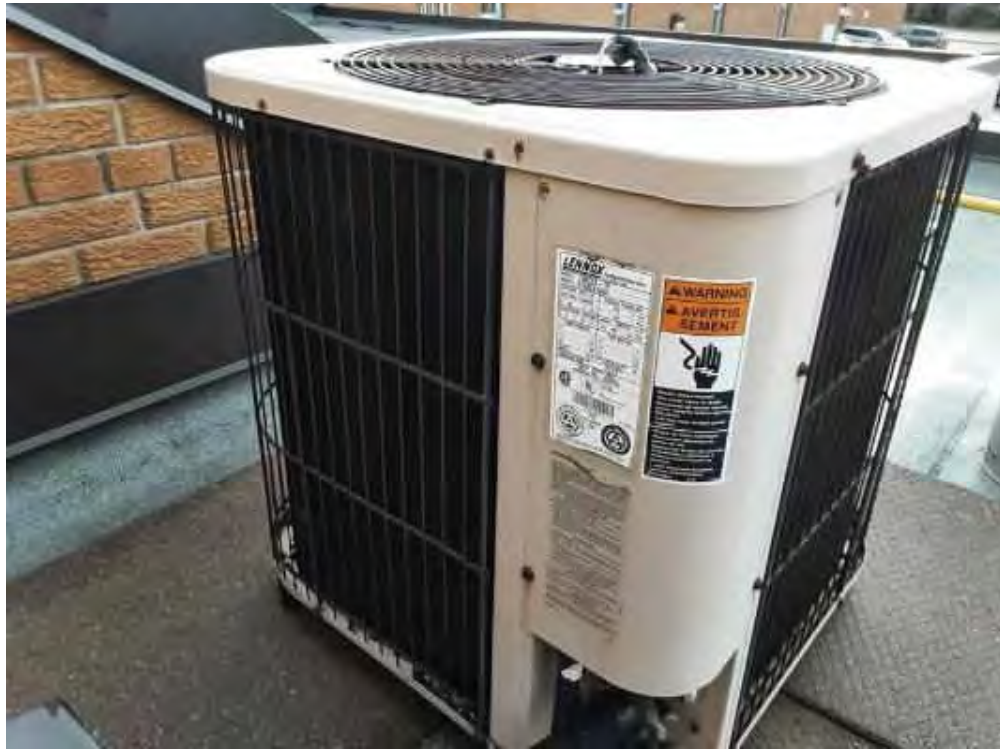
V0000 (None), Mechanical Equipment, Compressor, Not Insulated, Lower Roof (Location # 17) Fan unit
