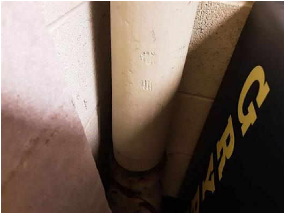
V9000 (Confirmed Asbestos), Piping, Rain Water Leader, Cement Product, Gym Storage (Location #: 25) Transite
