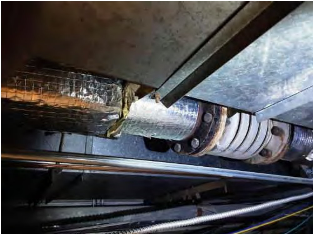
V0000 (None), Piping, Fibreglass, Corridor (Location #: 27)
