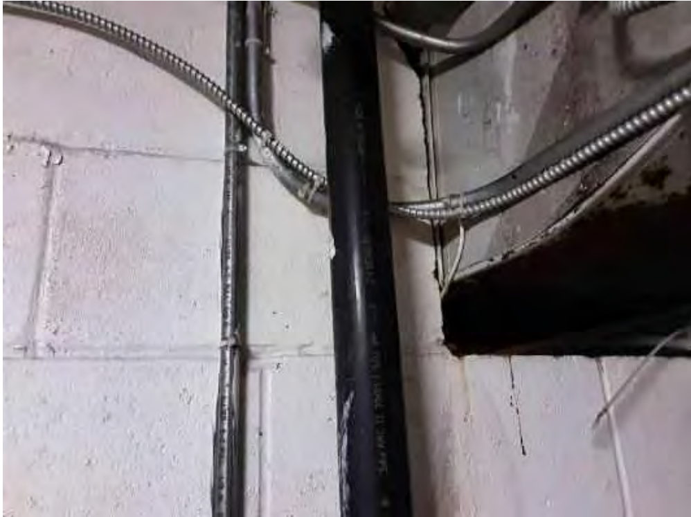
V0000 (None), Piping, Not Insulated, Fan Room (Location #: 1)
