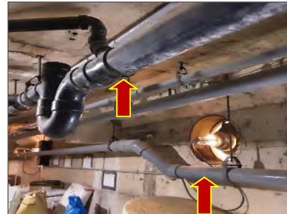
Photo 2: Uninsulated piping present in the Tunnel Area (Loc. 3).
