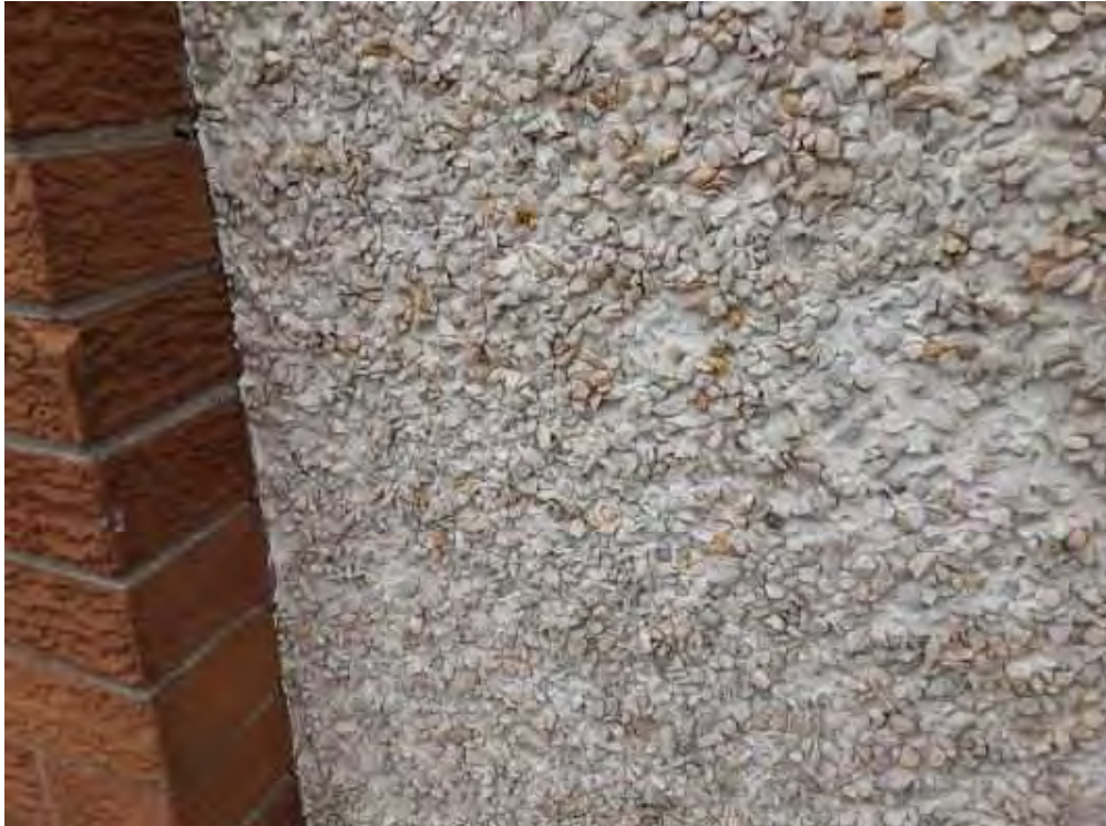
S0014B (None), Wall, Unidentified Material, Exterior (Location #: 14) Gravel stuck on top of coat
