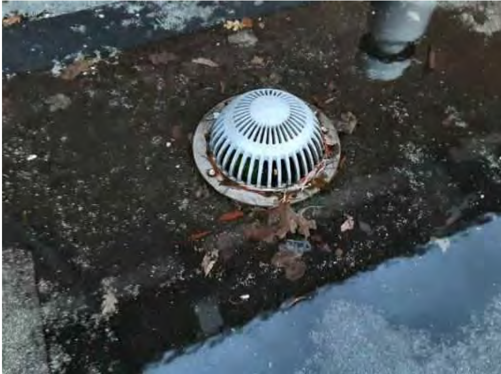
V0000 (None), Mechanical Equipment, Roof Hopper (Drain), Not Insulated, Lower Roof (Location #: 17)
