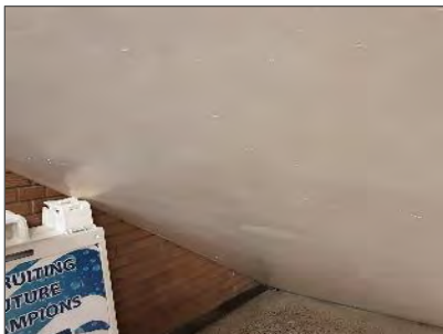
Photo 16: Asbestos-containing drywall joint compound underneath the stairwell present in the Lobby (Loc. 7).
