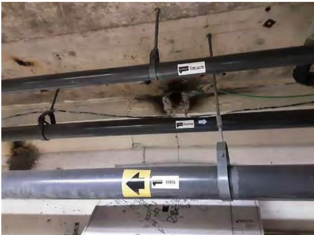
V0000 (None), Piping, Polyvinyl chloride (PVC), Filter Room (Location #: 2) Inlet, discharge, vacuum, skimmer, waste
