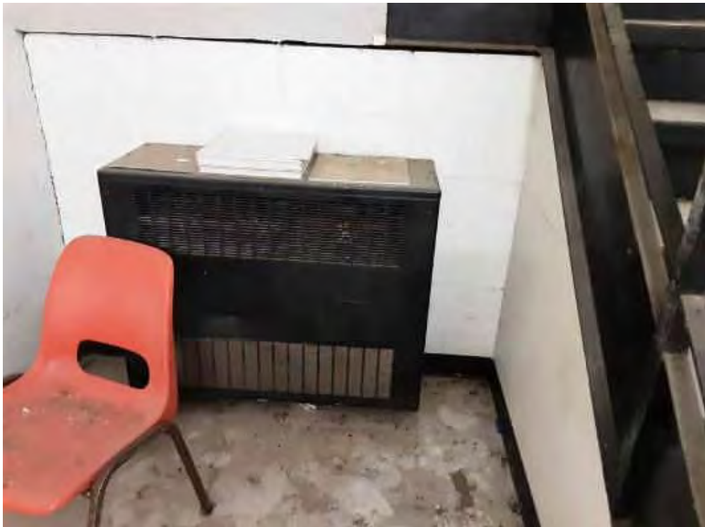
V0000 (None), Mechanical Equipment, Unit Heater, Not Insulated, East Stairwell (Location #: 5) At the exit level
