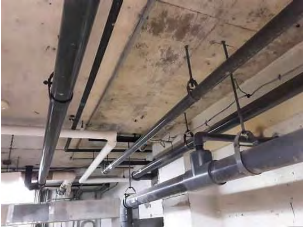
V0000 (None), Piping, Polyvinyl chloride (PVC), Filter Room (Location #: 2) Inlet, discharge, vacuum, skimmer, waste
