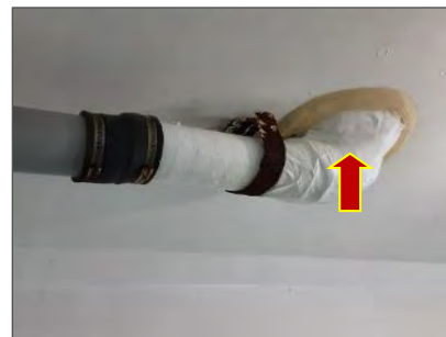
Photo 4: Asbestos containing parging cement insulated pipe present in the Balcony (Loc.4).
