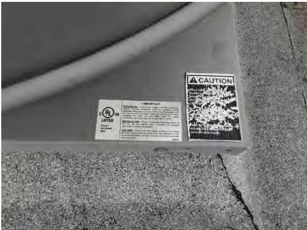
V0000 (None), Mechanical Equipment, Fan Unit, Not Insulated, Lower Roof (Location #: 17) Ventilator
