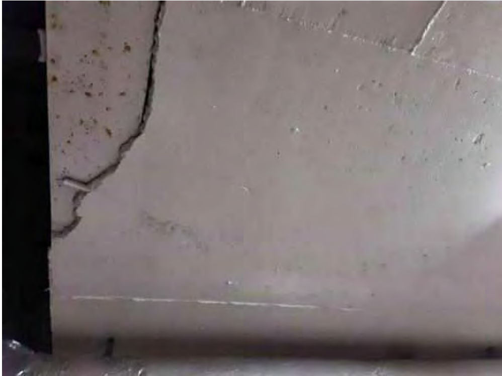
V0000 (None), Structure, All, Concrete (poured), Fan Room (Location #: 1)
