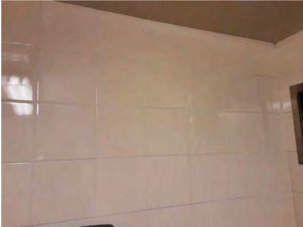
S0010A (None), Wall, Mastic, Men's Change Room (Location #: 9) Light green, ceramic tiles are covered over Block wall
