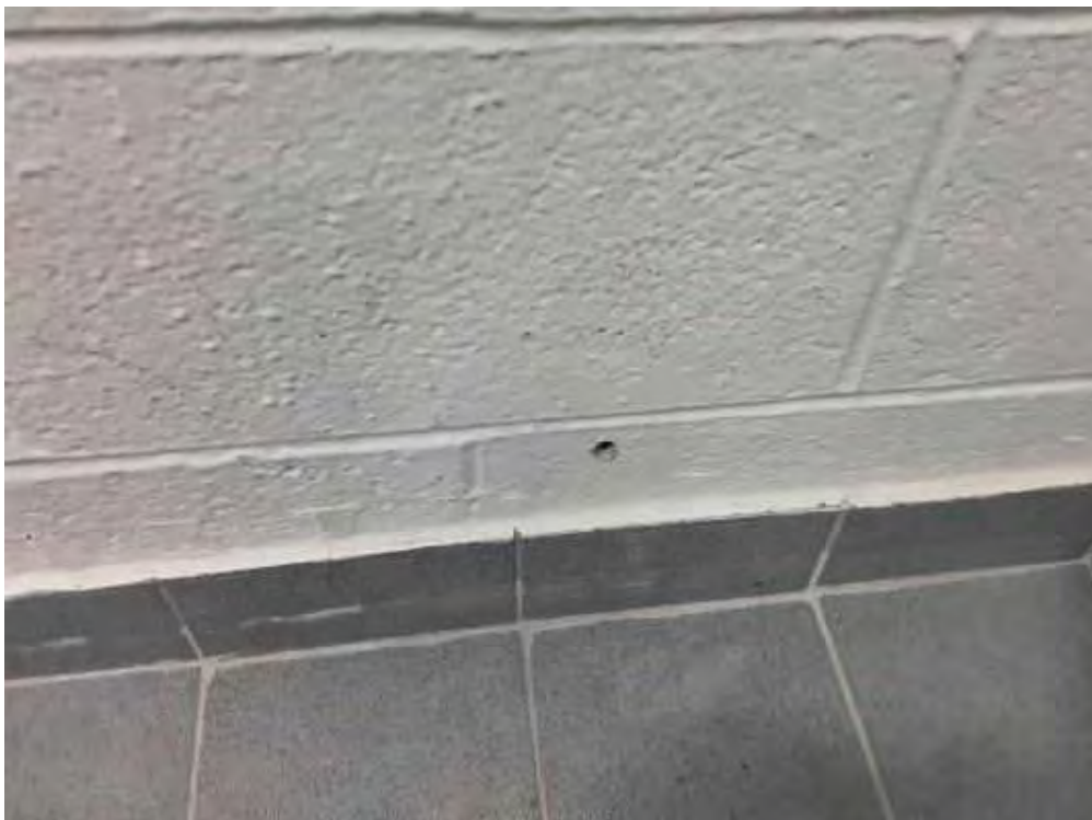
V0000 (None), Wall, Vermiculite/concrete block walls, In do or Pool (Location #: 13) 4 Drill holes, no vermiculite, N wall, E wall, W wall, S wall
