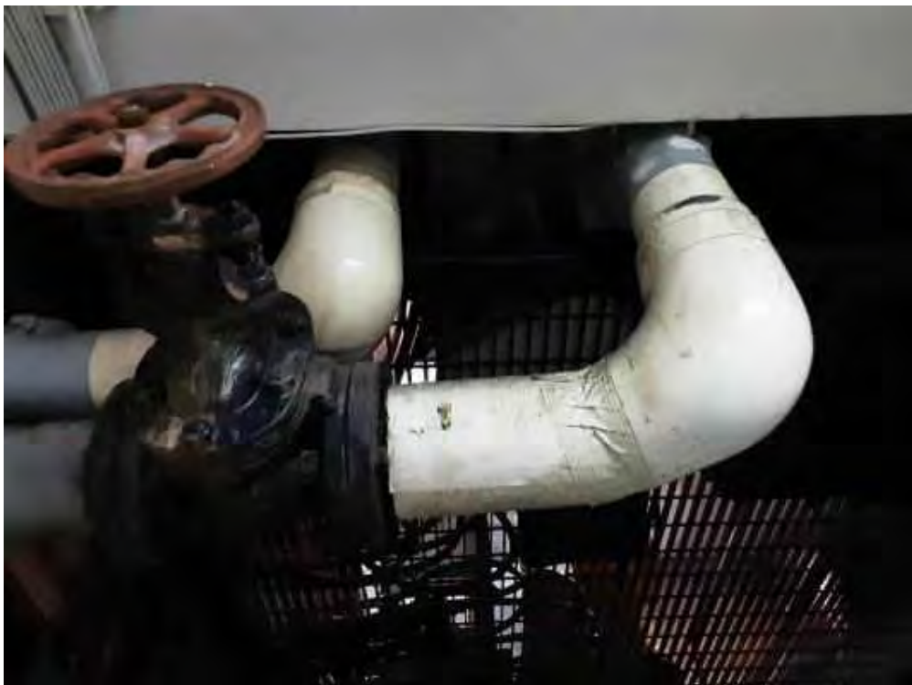
V0000 (None), Piping, All, Fibreglass, Fan Room (Location #: 1)
