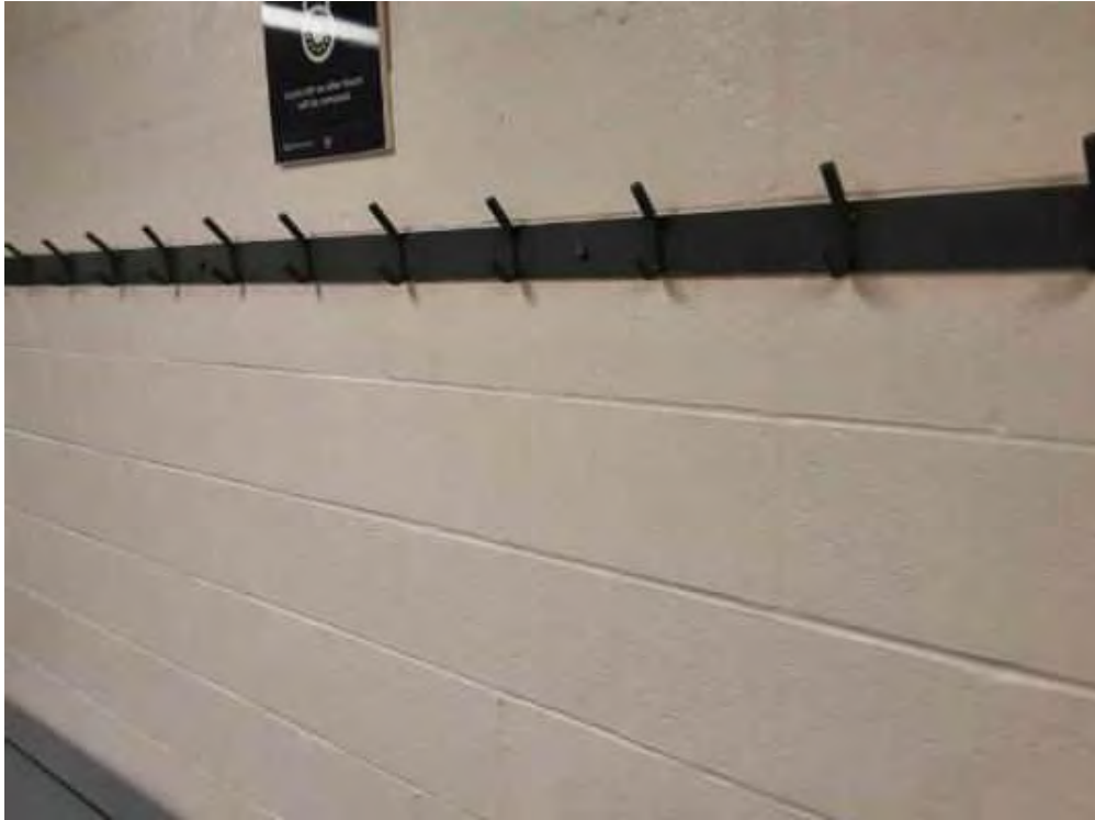
Masonry, Light beige, L0013(Lead (Low)), Men's Change Room (Location #: 9)
