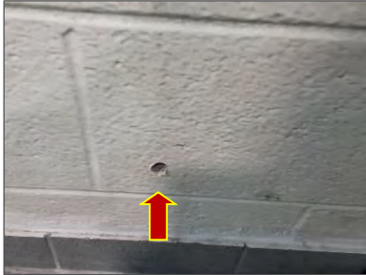
Photo 12: Vermiculite drill hole made on block wall present in Indoor Pool (Loc. 13).
