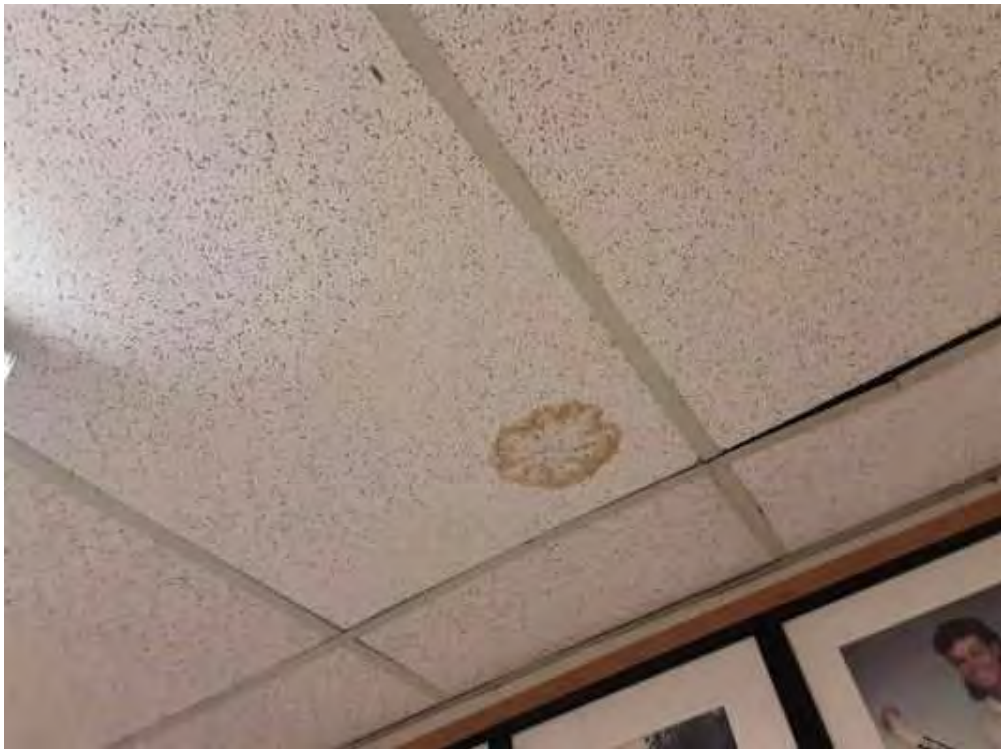
S0031A (None), Ceiling, All, Ceiling Tiles (lay-in), Corridor (Location #: 27) Water staining observed
