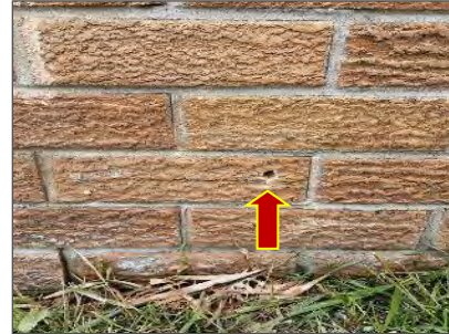
Photo 13: Vermiculite drill hole made on brick wall present in Exterior (Loc. 14).
