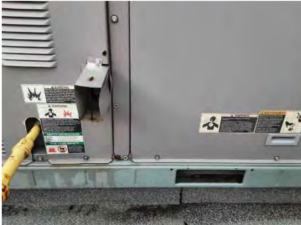
V0000 (None), Mechanical Equipment, Air Handling Unit, Not Insulated, Lower Roof (Location #: 17)
