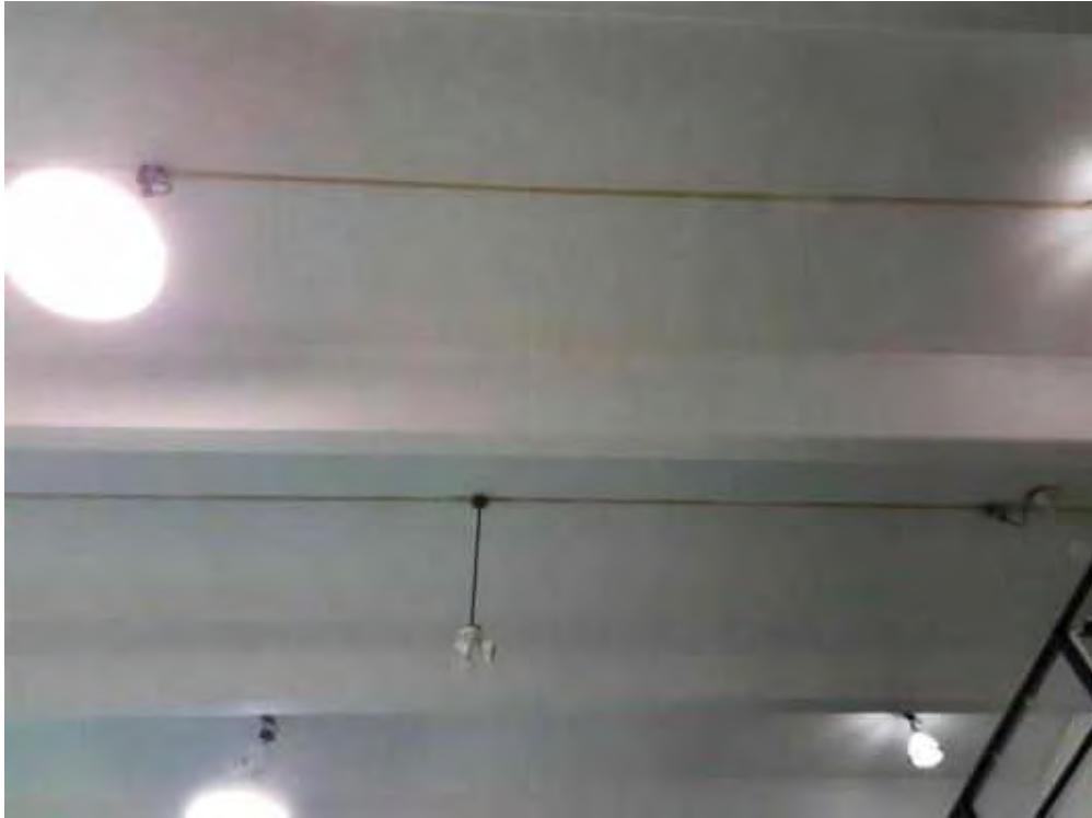
V0003 (None), Structure, Expansion Joint, Caulking, Indoor Pool (Location #: 13) Beige
