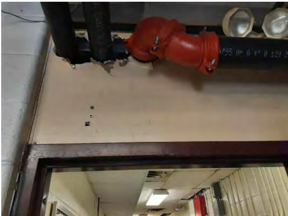
S0008C (Confirmed Asbestos), Wall, Drywall and joint compound, Custodian (Location #: 29)
