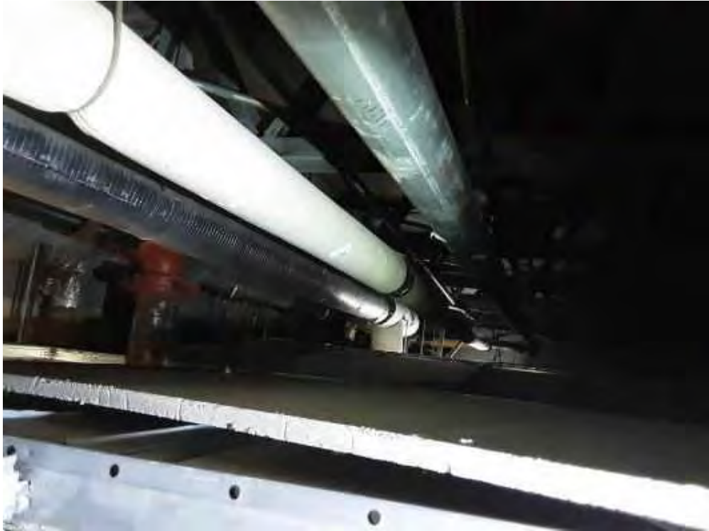
V0000 (None), Piping, Fibreglass, Custodian (Location #: 29)
