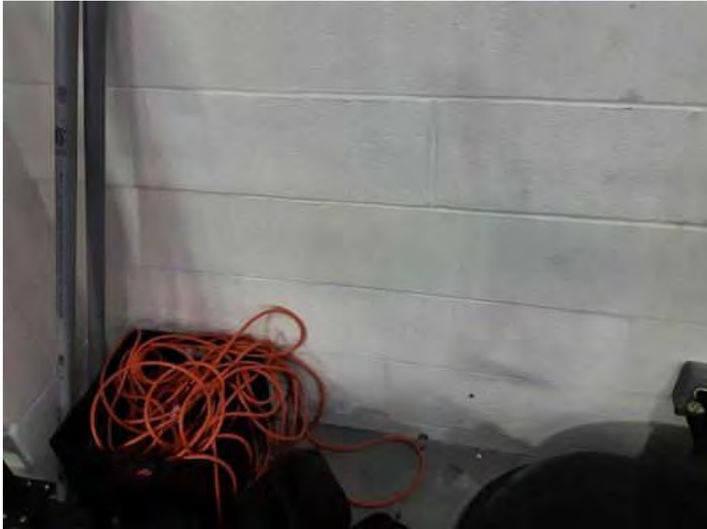
V0000 (Non e), Wall, Vermiculite/concrete block walls, Balcony (Location #: 4) 2 Drill holes, no vermiculite
