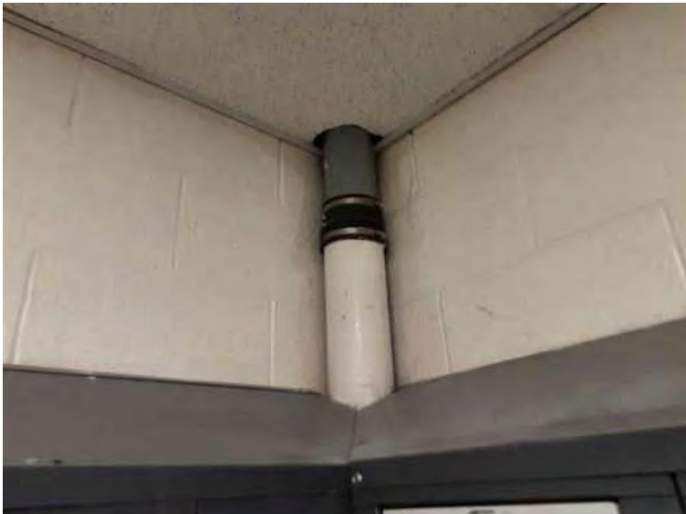
V0000 (None), Piping, Rain Water Leader, Polyvinyl chloride (PVC), Men's Change Room (Location #: 9)
