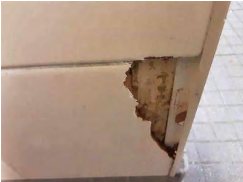
S0010B (None), Wall, Mastic, Men's Change Room (Location #: 9) Light green
