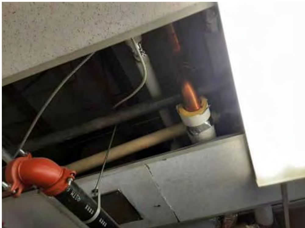
V0000 (None), Piping, Fibreglass, Custodian (Location #: 29)
