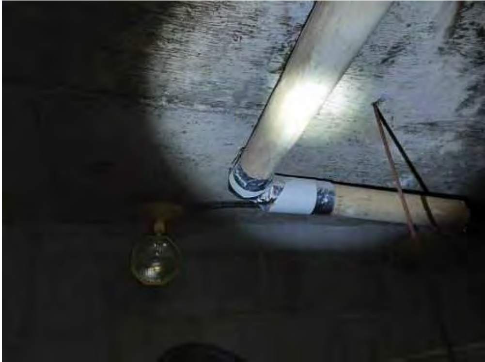
V0000 (None), Piping, All, Fibreglass, Tunnel Area (Location #: 3)
