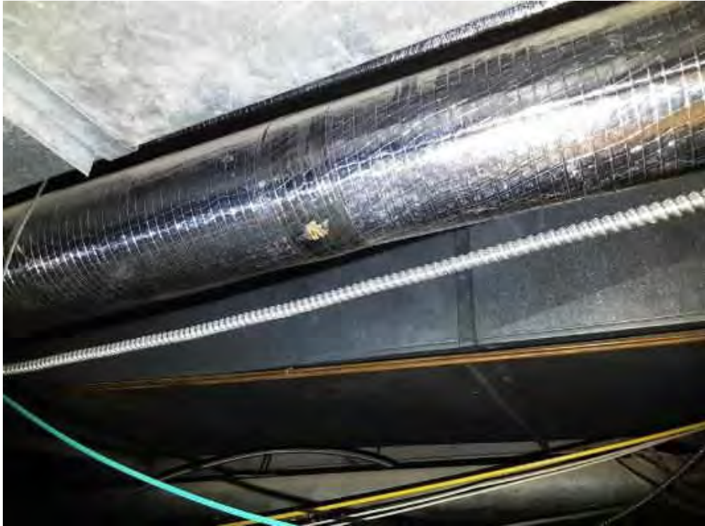
V0000 (None), Piping, Fibreglass, Corridor (Location #: 27)
