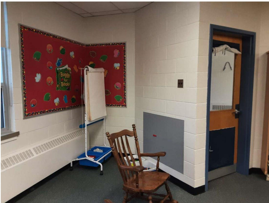
S0029C (None), White paint on block wall in the Library (Location #: 37)
