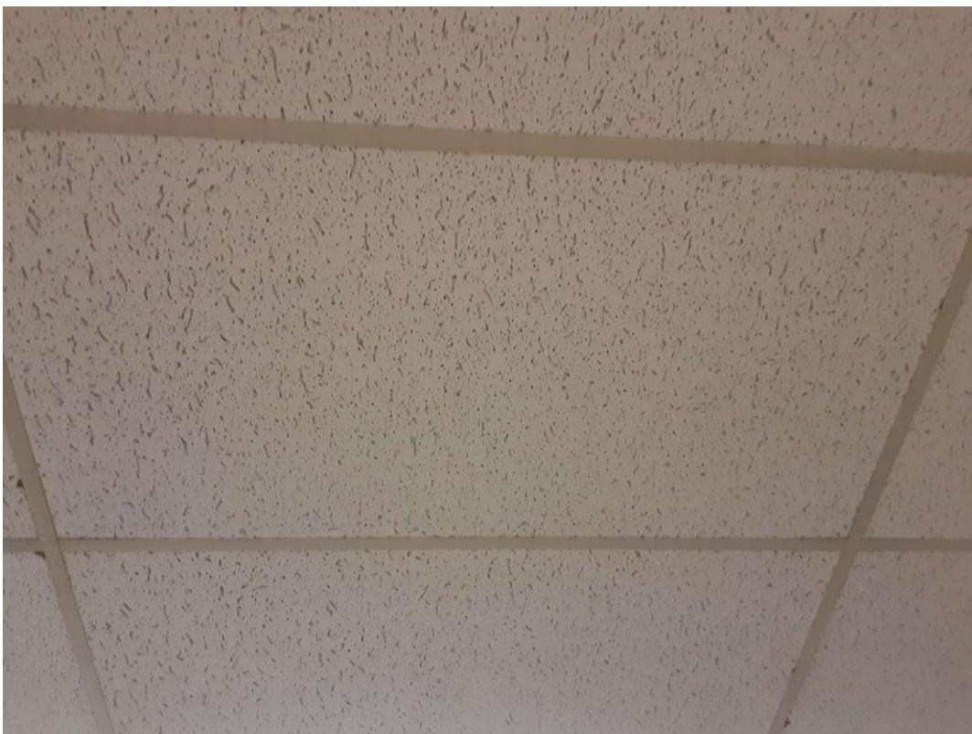
V0000 (None), 2ft by 4ft pinhole and fissure Ceiling Tiles (lay-in) in the Library (Location #: 37) Date code 3183B
