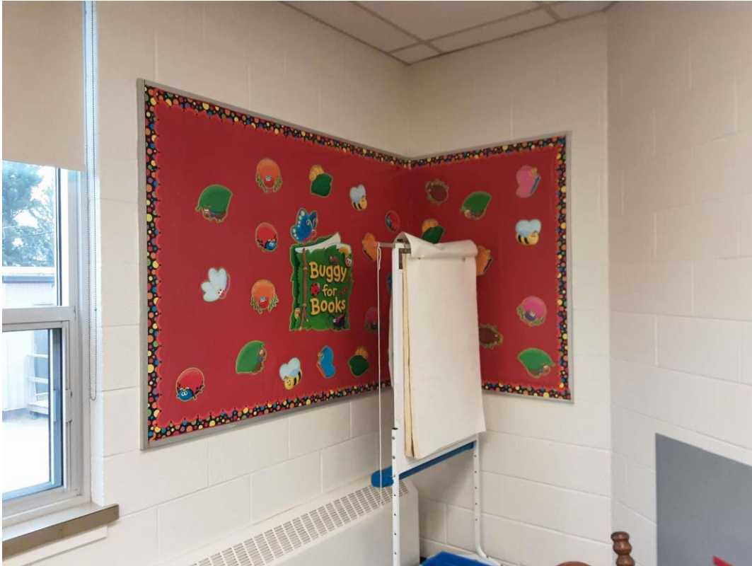
V9500 (Presumed Asbestos), Mastic behind corkboard in the Library (Location #: 37)
