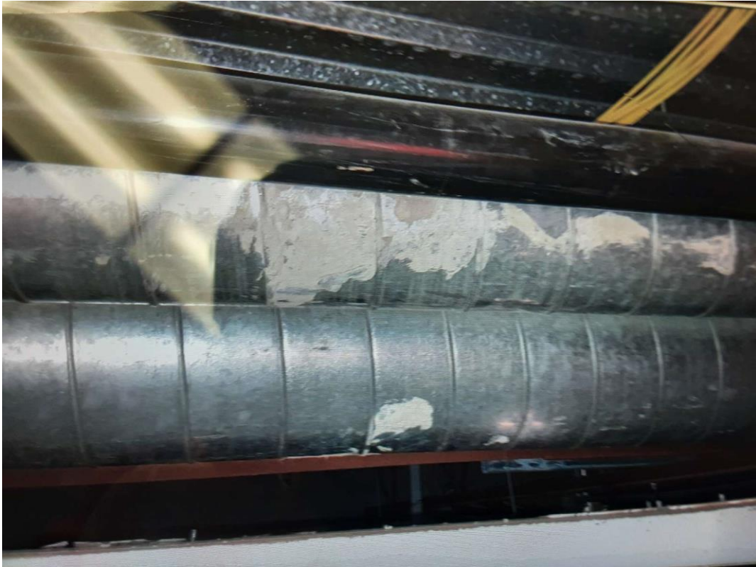
S0033C (None), Cementitious product on ducts in the Library (Location #: 37)
