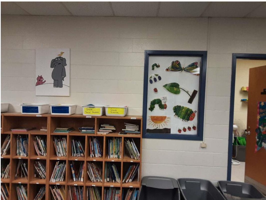
L0001(Lead, High), White paint on block wall in the Library (Location #: 37)
