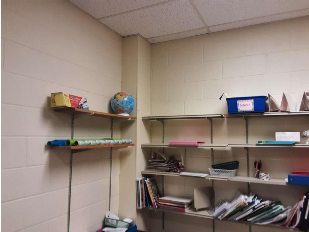
S0030C (None), Beige paint on block wall in the Work Room (Location #: 38)
