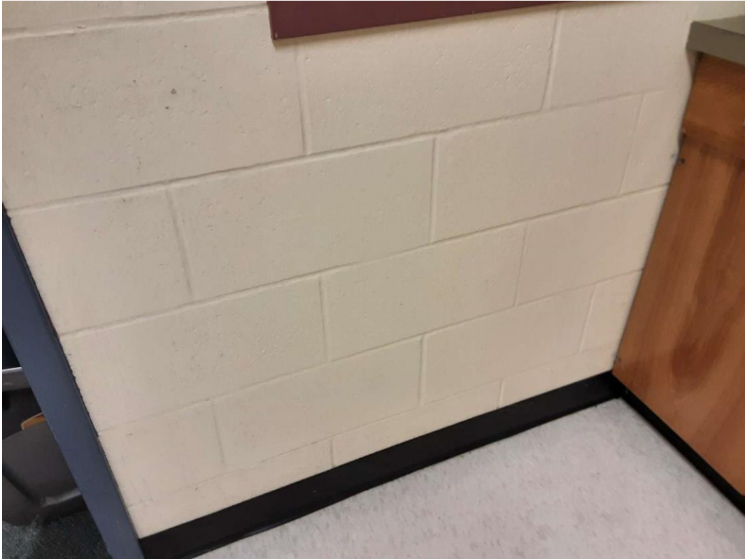
L0002(Lead, High), Beige paint on block wall in the Work Room (Location #: 38)
