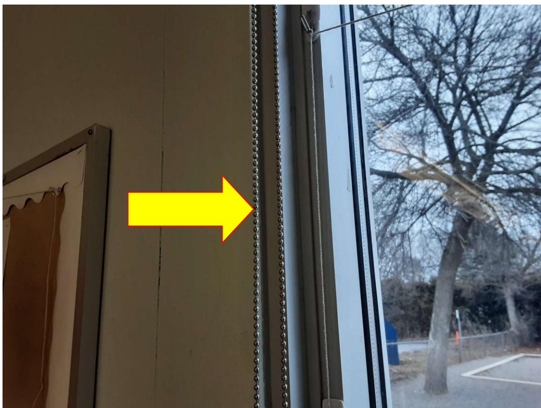
S0036C (None), Grey caulking around windows in Location #: 7
