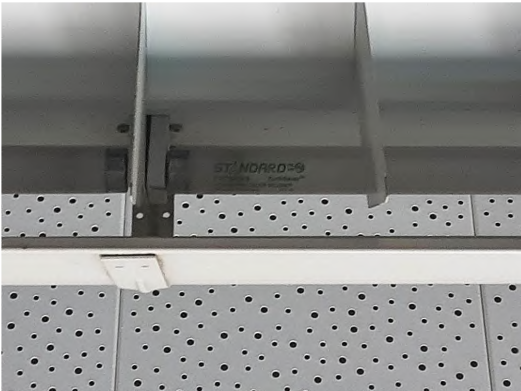
Mercury, V9000(Yes), Light Fixture in the Classroom (Location #: 105)
