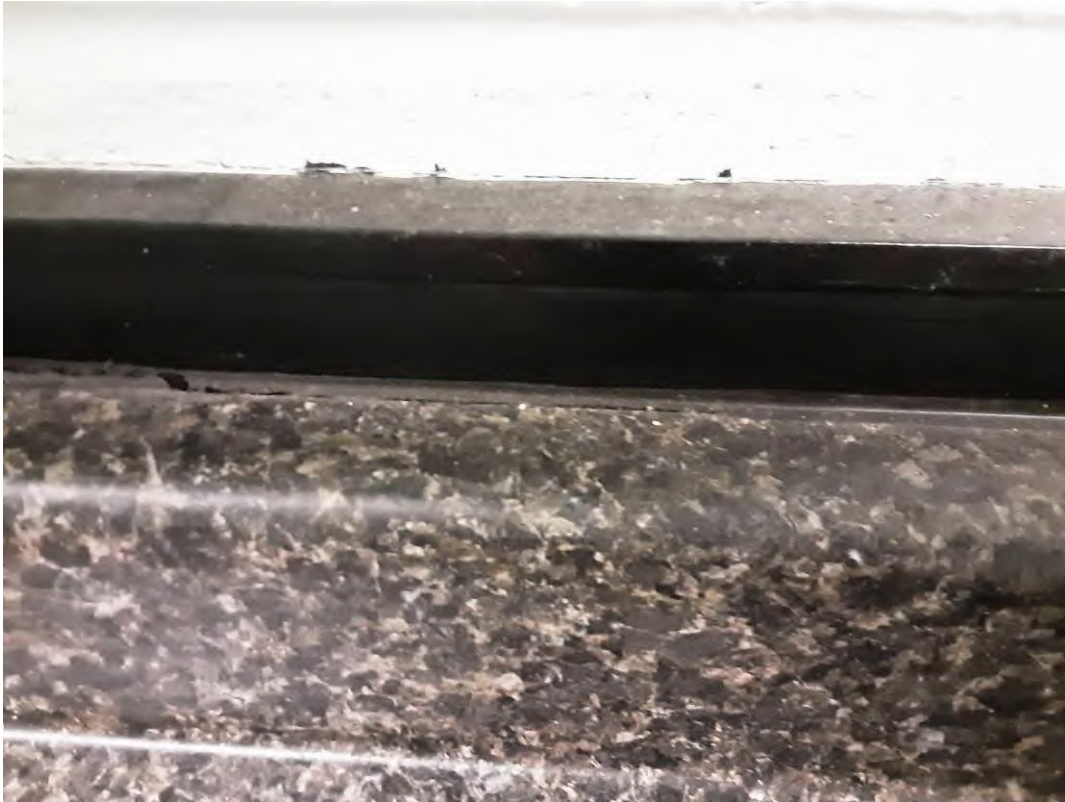
S0052C (None), Black caulking in the Prep Room (Location #: 21)
