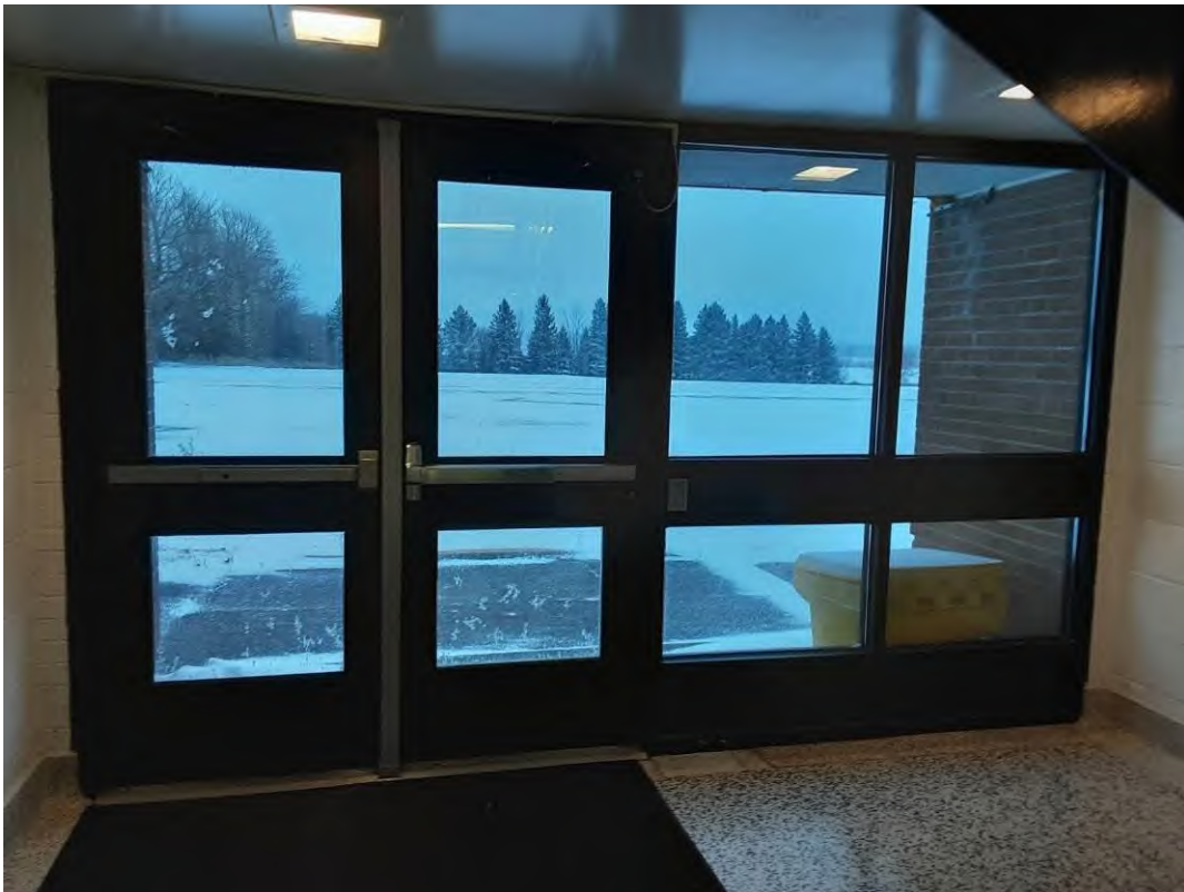
V9500(Presumed Lead), Black paint on doors and frames in the Stairs (Location #: 90)
