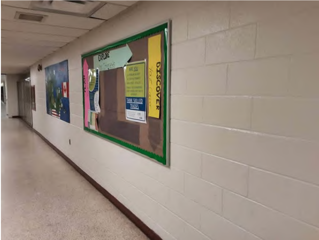
V0015(Lead, Low), White paint on masonry walls in the Corridor (Location #: 125)
