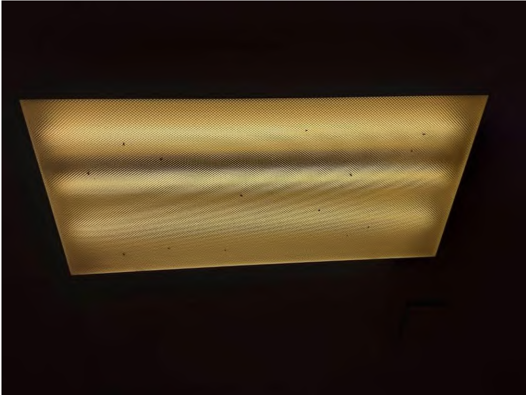
Mercury, V9000(Yes), Light Fixtures in the Classroom (Location #: 22)
