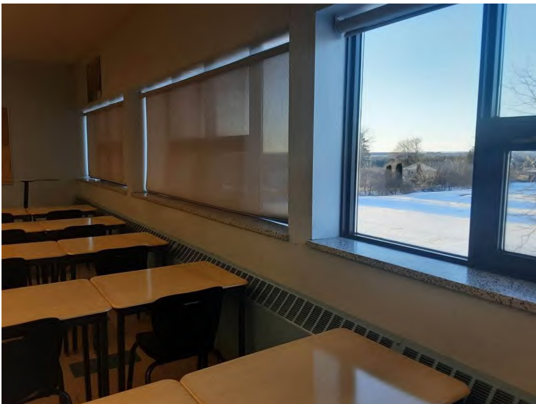
V9500 (Presumed Asbestos), Terrazzo window sills in Classroom (Location #: 105)
