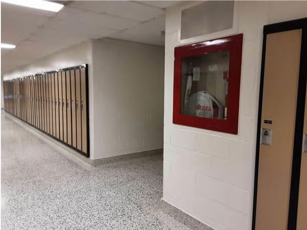
S0049F (None), White paint on block wall in the Corridor (Location #: 89)
