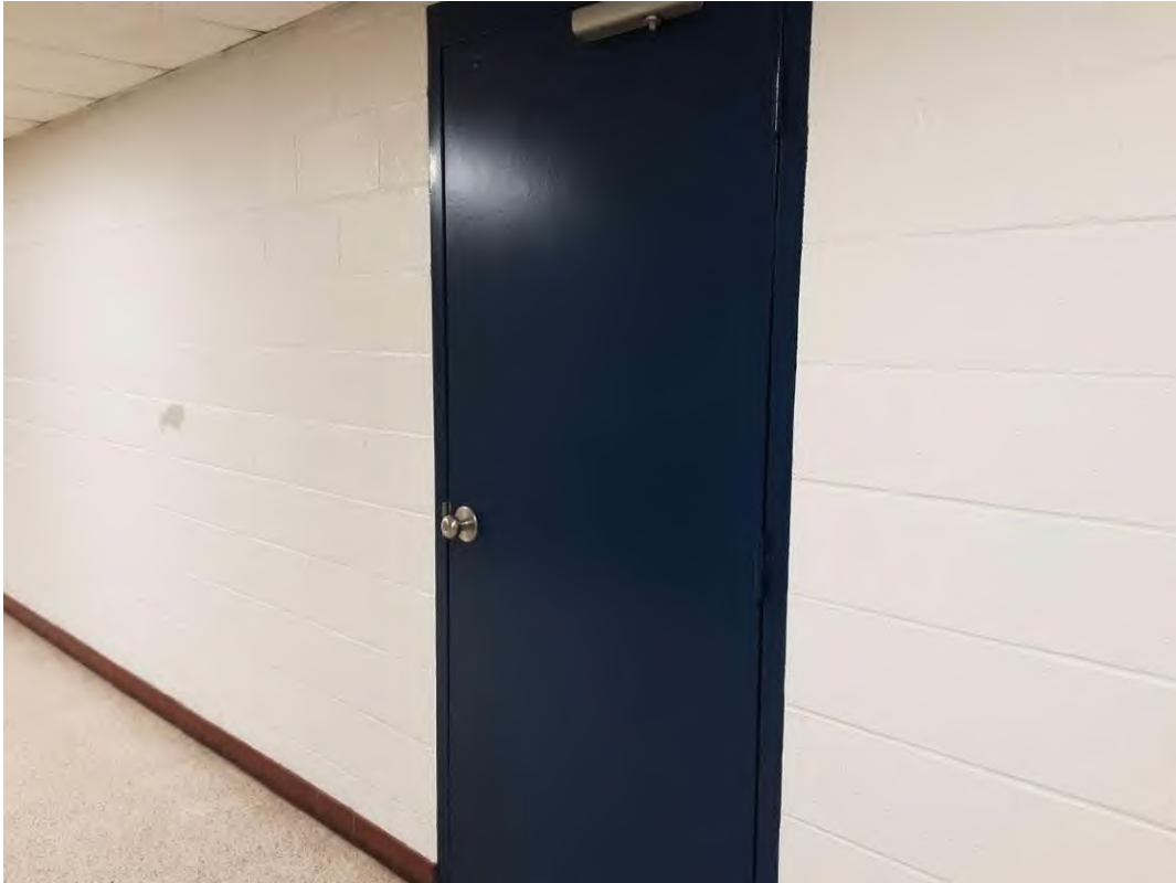
V0013(Lead, Low), Blue paint on doors and door frames in the Corridor (Location #: 125)
