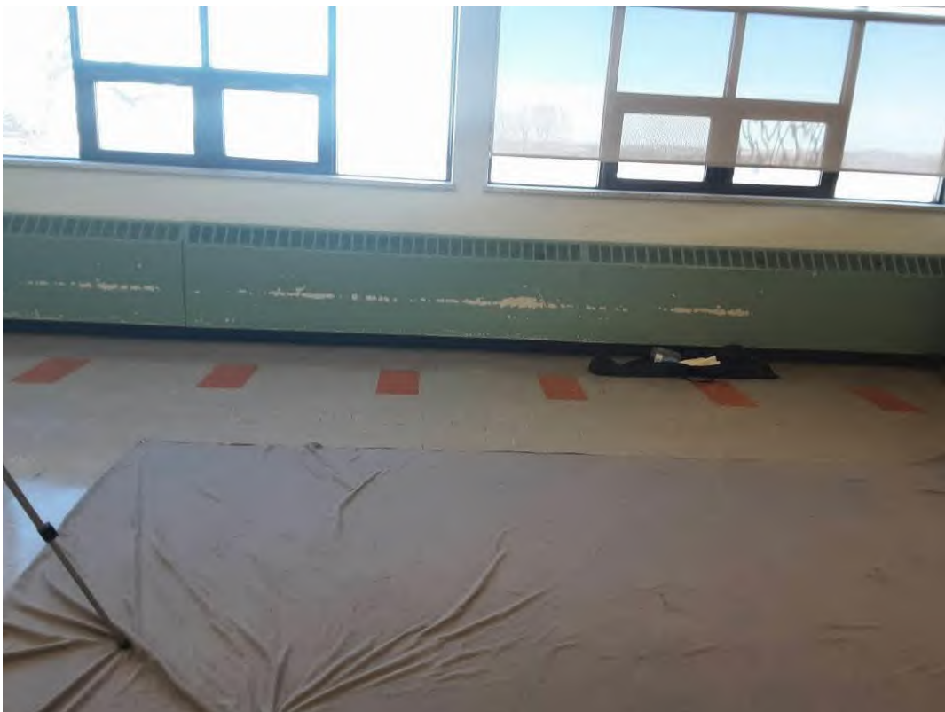
V0016(Lead, High), Green paint on radiators in the Classroom (Location #: 106)
