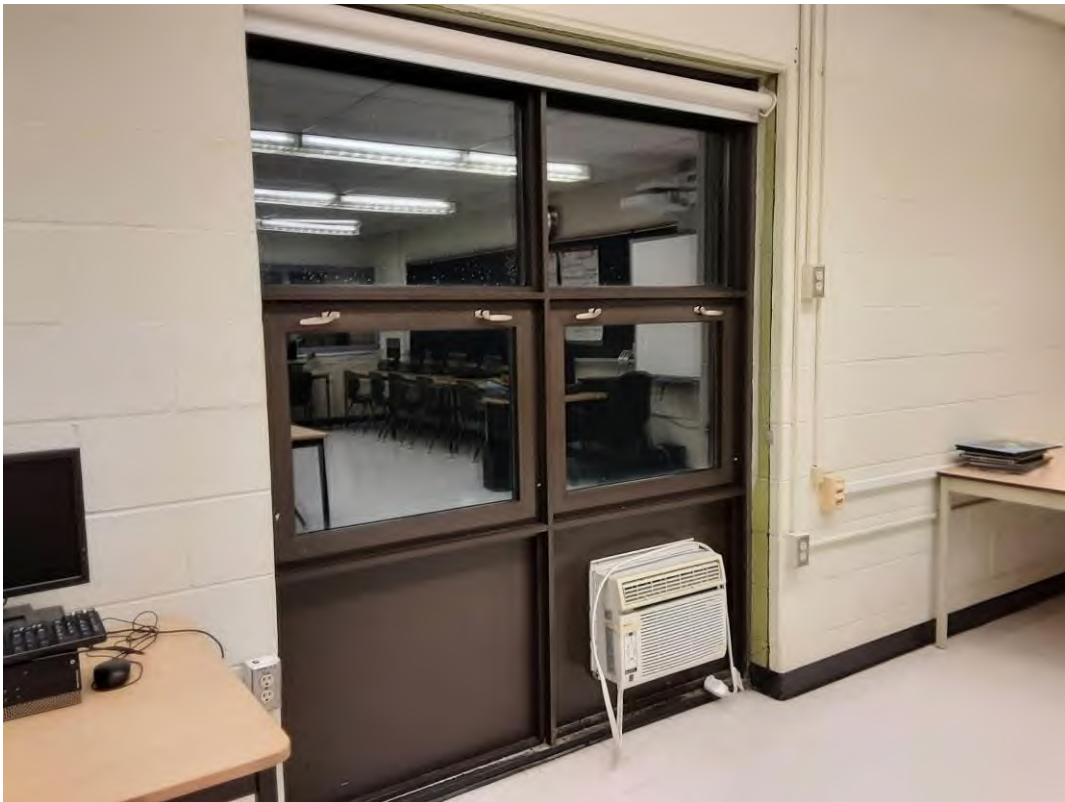
V9500(Presumed Lead), Black paint on windows frame in the Classroom (Location #: 100)
