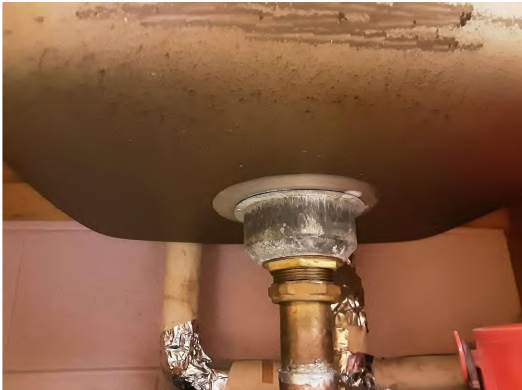
S0056C (Confirmed Asbestos), Sink mastic in the Study/Storage (Location #: 101)
