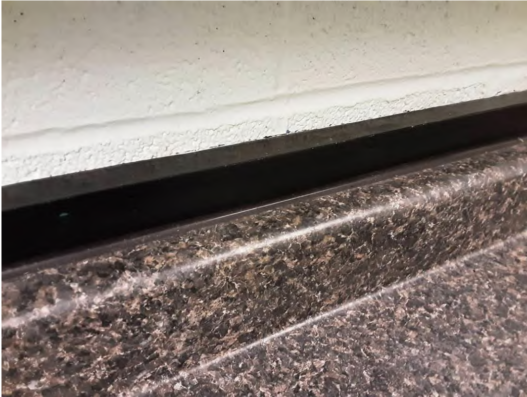
PCB, P0001(No), Black caulking in the Prep Room (Location #: 21)
