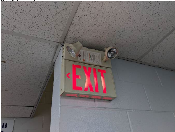
Presumed lead-containing batteries in emergency fixtures
