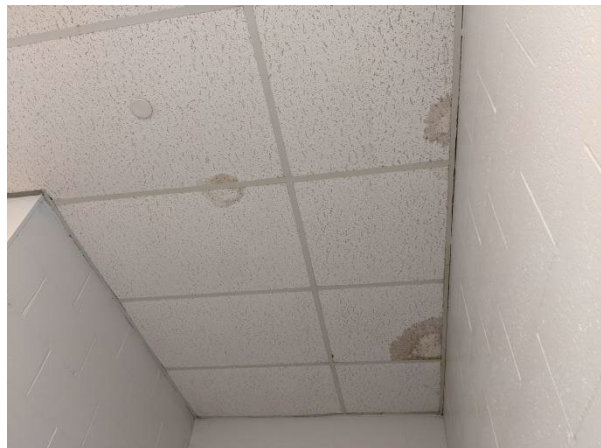
Water-stained ceiling tiles, Stairwell/Vestibule
