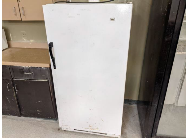
Presumed ODS-containing refrigeration units
