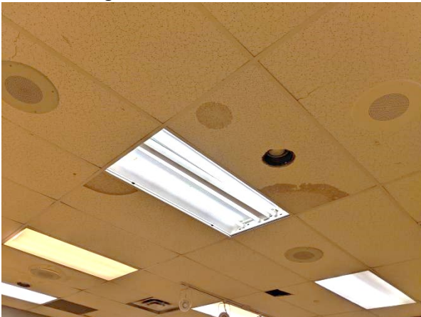
Water-stained ceiling tiles, Second Floor Multipurpose Room
