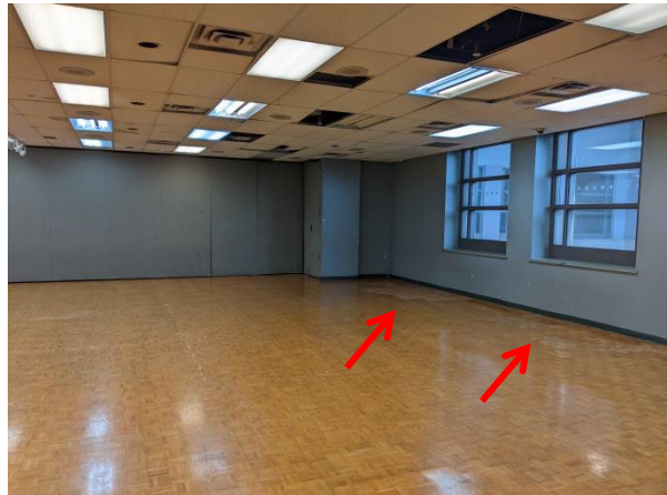
Water-damaged floor, Second Floor Multipurpose Room
