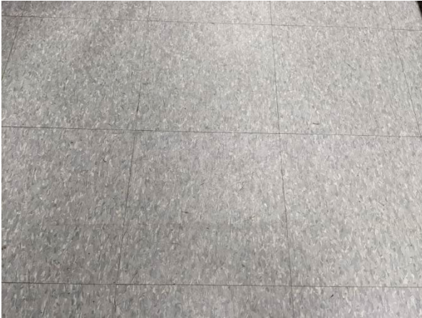
Samples 6A-C: non-asbestos dark grey flecked 12"x12" vinyl floor tile and mastic, Ground Floor Servery
