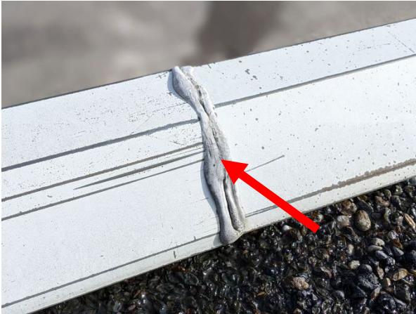
Samples 18A-C: asbestos-containing white caulking, roof flashing, East and West Roofs
