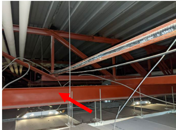
Presumed lead-containing coatings on steel supports
