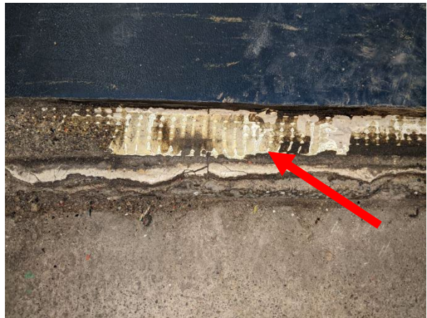
Samples 5A-C: non-asbestos concealed 12"x12" vinyl floor tile and mastic; Administration Office
