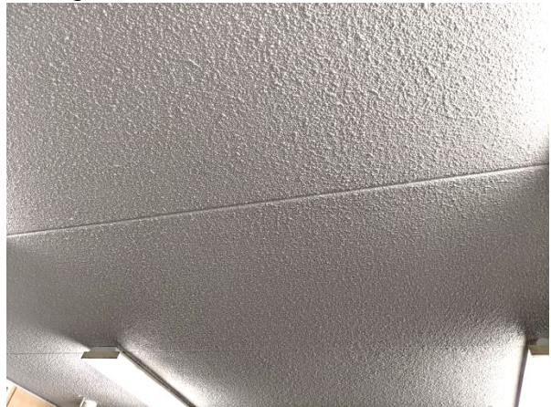
Samples 9A-E: non-asbestos ceiling texture coat, Ground Floor Main Corridor
