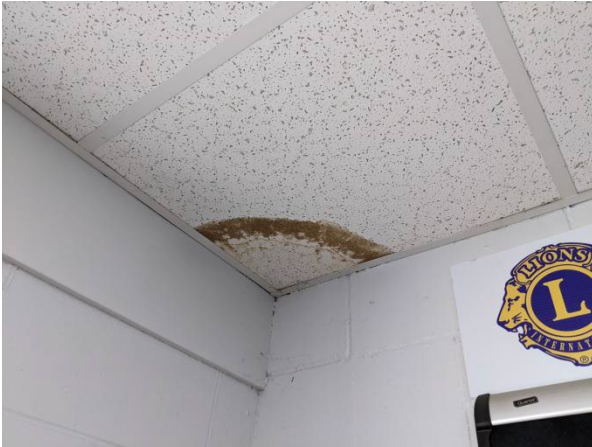
Water-stained ceiling tiles, Administration Office
