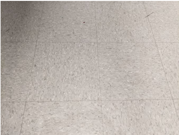
Samples 2A-C: non-asbestos grey flecked 12"x12" vinyl floor tile and mastic, Second Floor Servery, Second Floor Corridor, and OPP Office
