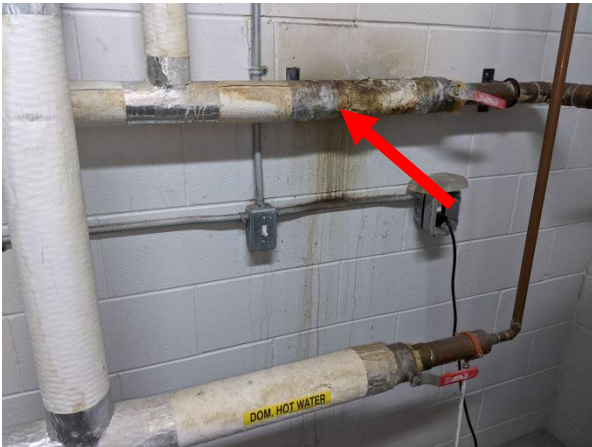
Water-stained pipe insulation, Arena Mechanical Room
