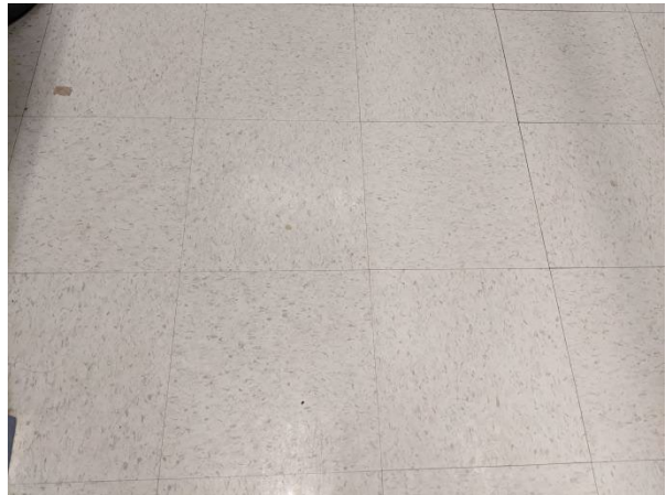
Samples 3A-C: non-asbestos white flecked 12"x12" vinyl floor tile and mastic; Second Floor Washrooms
