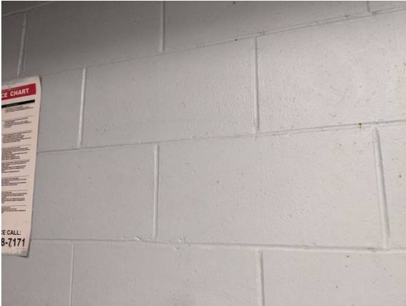
Sample LP4: non-lead light blue paint, Ground Floor Servery
