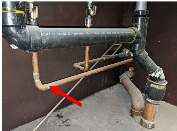
Presumed lead-containing solder in copper pipes
