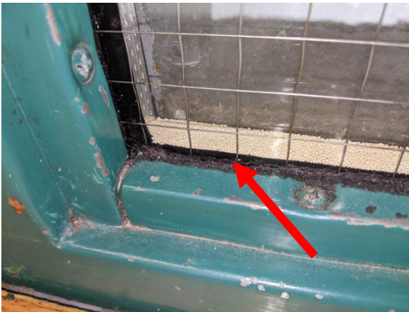
Samples 14A-C: asbestos-containing black interior window glazing, Second Floor Multipurpose Room, OPP Office, Ground Floor Hall, 1977 build
