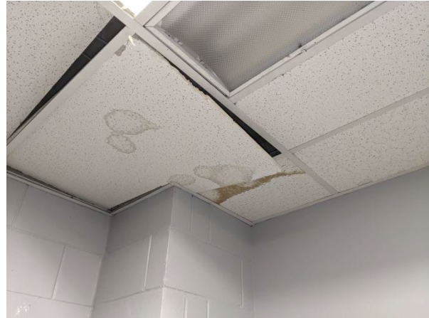
Water-stained ceiling tiles, OPP Office
