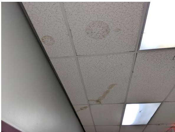
Water-stained ceiling tiles, Second Floor Corridor
