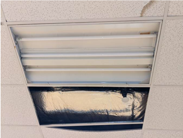
Presumed mercury and PCBs associated with fluorescent light fixtures, interior
