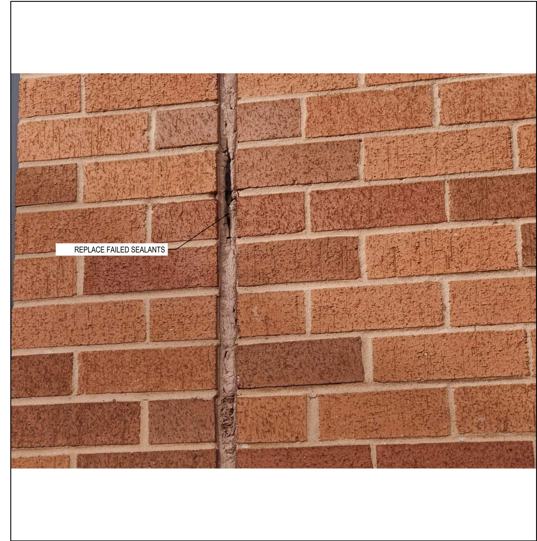
3 FAILED SEALANT JOINT R600
