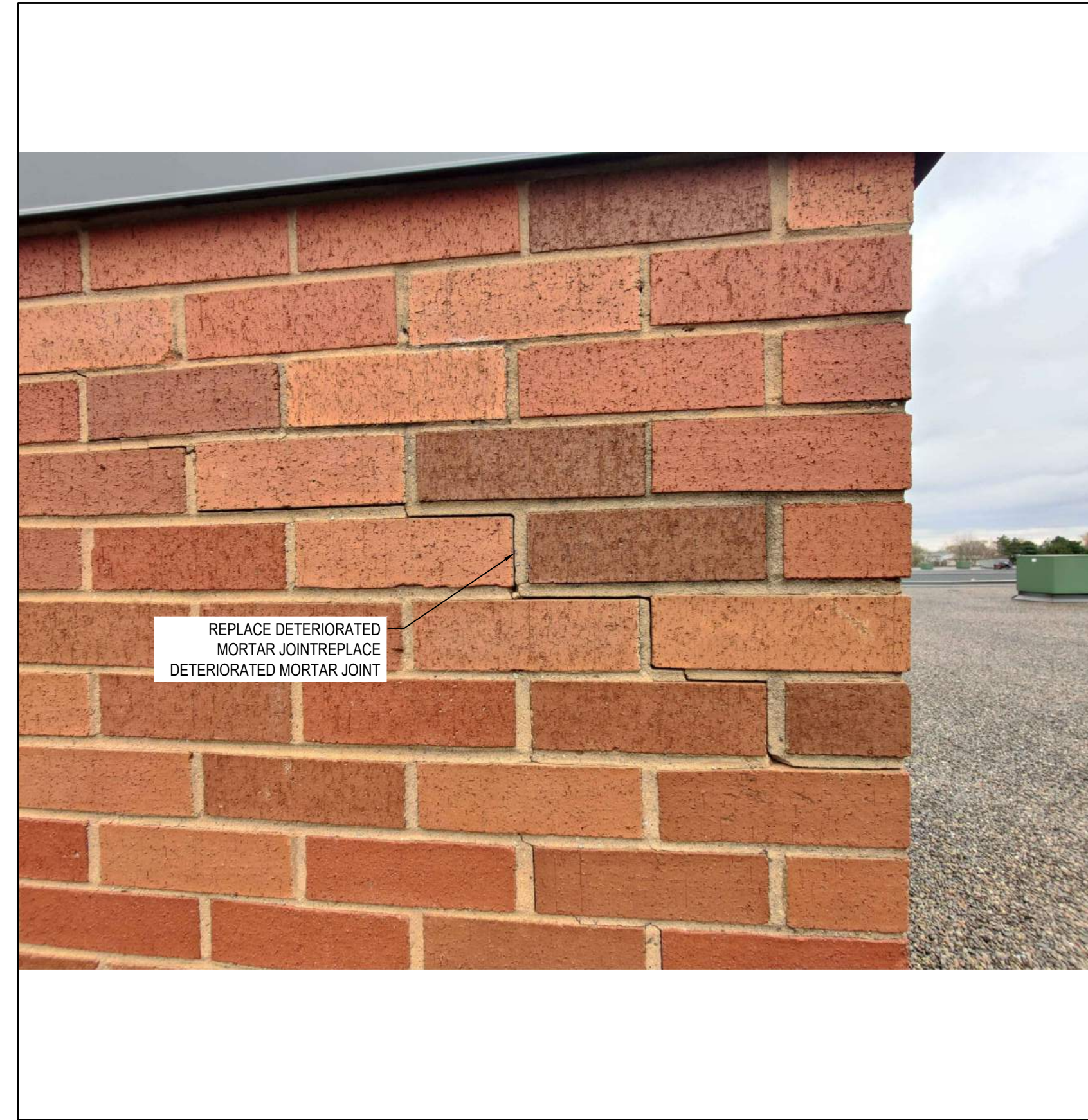
2 DETERIORATED MORTAR JOINT R600
