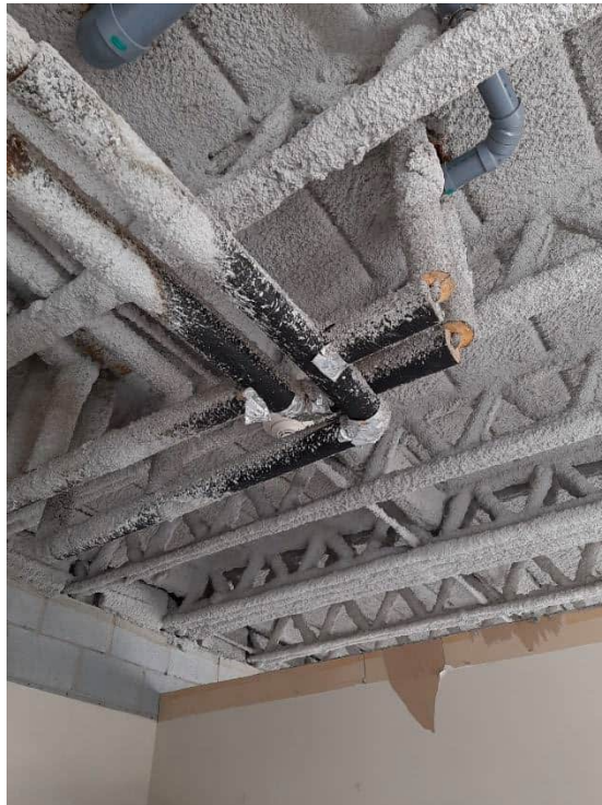
Photograph No. 28 – 125 Delhi Street – 2nd Floor Shell Space – June 27, 2023. Spray applied fireproofing on deck and open web steel joists confirmed as non-asbestos-containing (S08A, B, C). Spray-applied fireproofing on Level 1 (Elevator Lobby) also confirmed as non-asbestos-containing.
