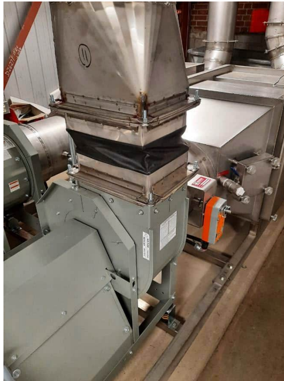
Photograph No. 14– 115 Delhi Street – Level 4 Mechanical Room September 23, 2023. Inspected duct expansion joints were confirmed as Neoprene or rubberized fabric.
