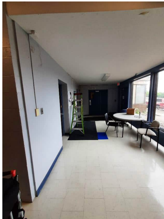
Photograph No. 4 – 73 Delhi Street – Ground Floor Lobby, June 26, 2023. One of several locations where non-asbestos vinyl floor tiles had asbestos containing mastics. Additional sampling should be conducted at other locations prior to disturbance or removal.
