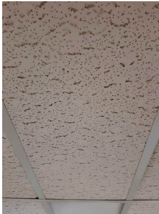
Photograph No. 2 – 73 Delhi Street – 4 th Floor Administrative Offices, June 26, 2023 – One of four types of 2’x4’ and 2’x2’ ceiling tiles found within the building. All tested ceiling tiles returned negative for asbestos content at or above 0.5% asbestos content and are not classified as asbestos-containing.
