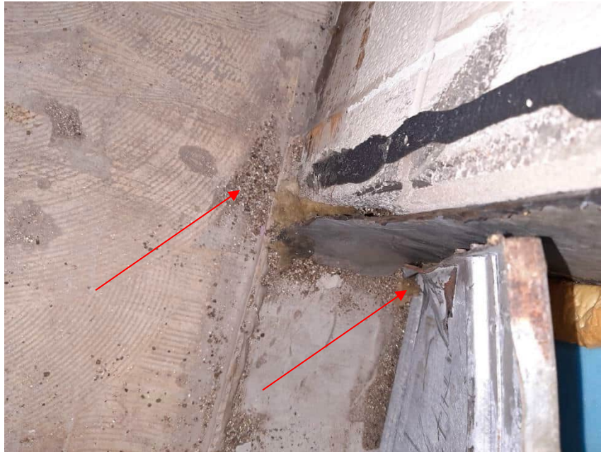
Photograph No. 28 – 125 Delhi Street – 2nd Floor Shell Space – June 27, 2023. Vermiculite loose-fill insulation in block wall behind register confirmed to be contaminated with asbestos (S10A - 1% Tremolite). All exterior walls should be treated with caution due to the presence of vermiculite. Debris found at a register “blank” on the south wall west of the lobby corridor.
