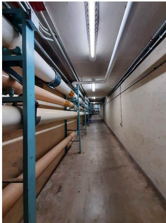
Photograph No. 6 – 73 Delhi Street – Ground Floor Steam Tunnel, June 26, 2023. Inspected steam, hot water and chilled water pipes were visually confirmed as fiberglass with canvas or PVC cladding. No asbestos-containing pipe or fitting insulation was confirmed.
