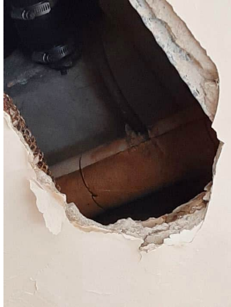
Photograph No. 5 – 73 Delhi Street – Ground Floor Security Office Storage Closet, June 26, 2023. One of several locations where asbestos pipe insulation was discovered above solid plaster ceilings. It is likely that additional asbestos-containing pipe and fitting insulation will be found above such surfaces including plumbing risers and wall cavities. Care should be taken when accessing solid ceiling and wall spaces due to the possibility of asbestos debris. Sample analysis confirmed the plaster as non-asbestos containing (S19B).
