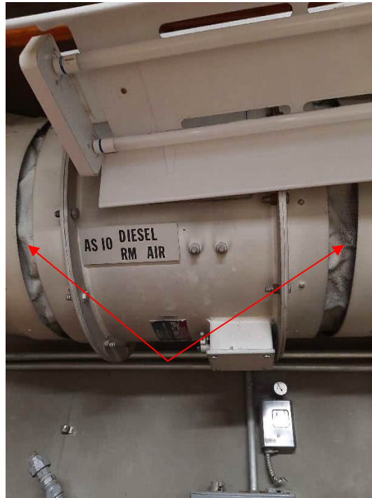
Photograph No. 21 – 115 Delhi Street – Level 1 Diesel Generator Room - September 23, 2023. Suspect asbestos containing duct expansion joints on a diesel generator exhaust fan.
