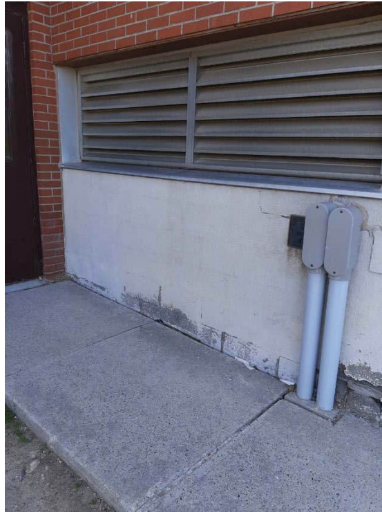
Photograph No.32 – 125 Delhi Street – Exterior – June 27, 2023. Cement parging on concrete block confirmed as non-asbestos-containing (S13A, B, C).
