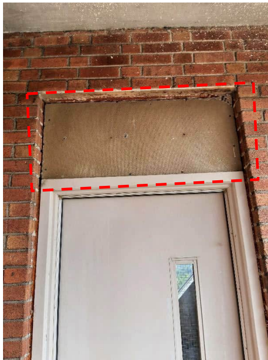
Photograph No. 17 – 115 Delhi Street – Level 4 Exterior Balcony, September 23, 2023. Suspect asbestos-containing cement panel over doorway to Stairwell C.
