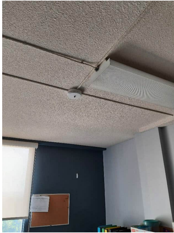
Photograph No. 3 – 73 Delhi Street – 1 st Floor Print/Staff Room, June 26, 2023 – Textured “paint” on concrete slab ceilings reported non-detect for asbestos content above the laboratory detection limit of 0.5% and are not classified as asbestos-containing (S12A, B, C).
