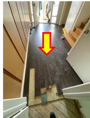
Asbestos-containing VFT concealed under wood flooring, Location 4.
