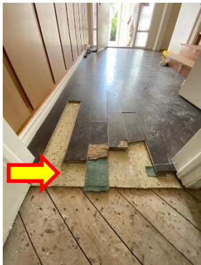
Asbestos-containing VFT concealed under wood flooring, Location 4.
