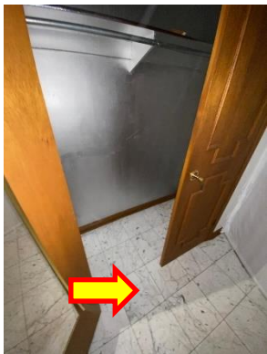
Ceramic floor tile and concealed asbestos-containing levelling compound to be abated, Location 8.
