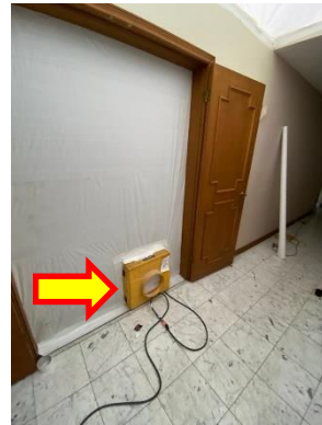
View of one D air unit exhausting air out of the enclosure, Location 8.
