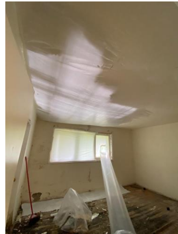
View of inside enclosure.
