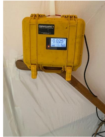
Sufficient negative air pressure displayed on manometer.
