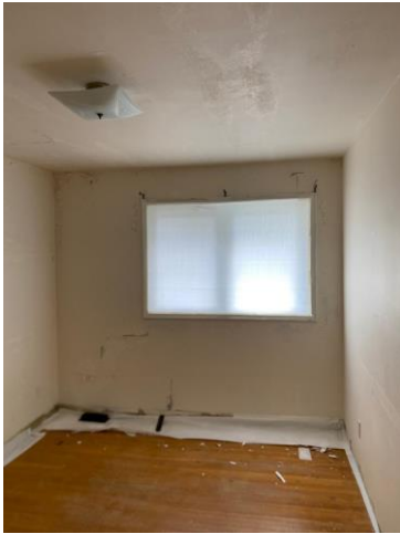
View of inside enclosure.
