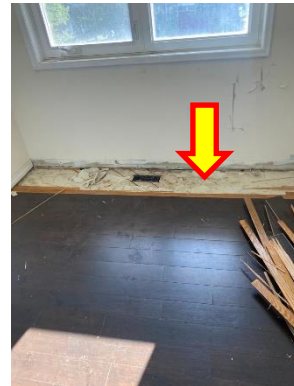
Asbestos-containing white paper insulation found under original hardwood flooring to be abated, Bedroom, 2 nd Floor, Location 14.
