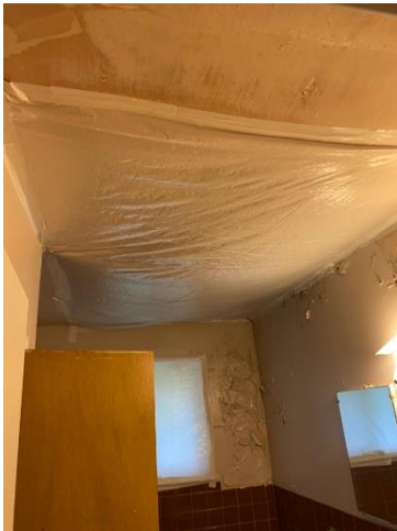
View of inside enclosure.
