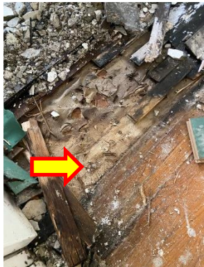
Asbestos-containing white paper insulation under original hardwood flooring to be abated, Bedroom, 2 nd Floor, Location 13
