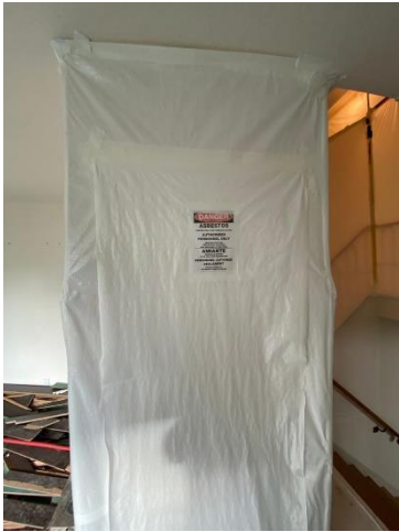
Asbestos warning sign posted on the entrance to the enclosure
