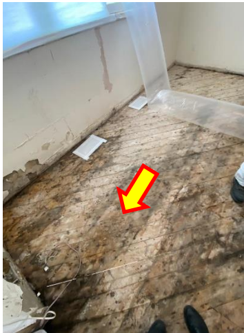
Visible mould growth was observed on plywood floor, Bedroom, Location 13.
