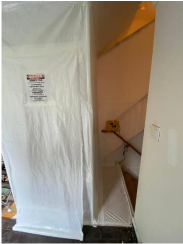
Asbestos warning sign posted on the entrance to the enclosure and manometer.
