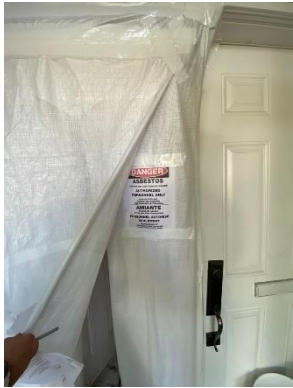
Enclosure entrance with posted asbestos warning sign, Location 8.
