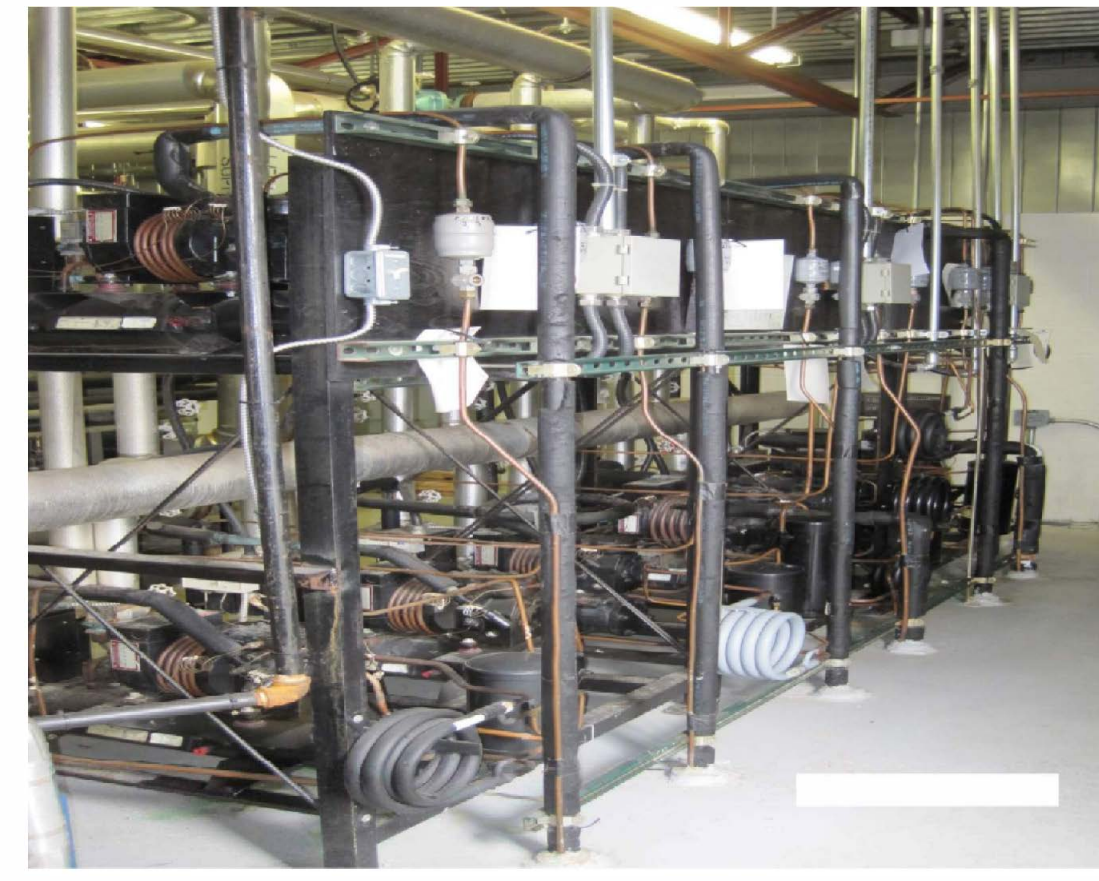
PHOTO 2: EXISTING COMPRESSOR/CONDENSING UNITS ON RACK (REFER TO DRAWING 404 FOR SYSTEM LOCATION)
