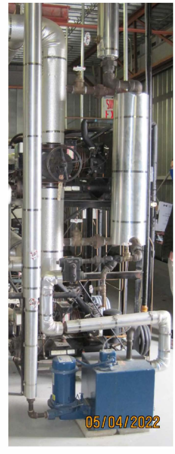
PHOTO 3: EXISTING STEAM-WATER REHEAT SYSTEM FOR CONDENSING WATER (REFER TO DRAWING 404 FOR SYSTEM LOCATION)
