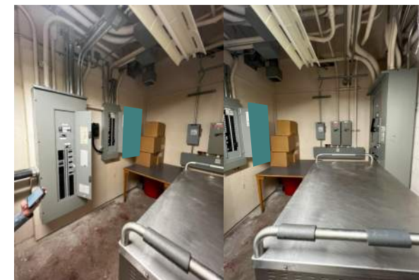
ELECTRICAL ROOM - B-65
