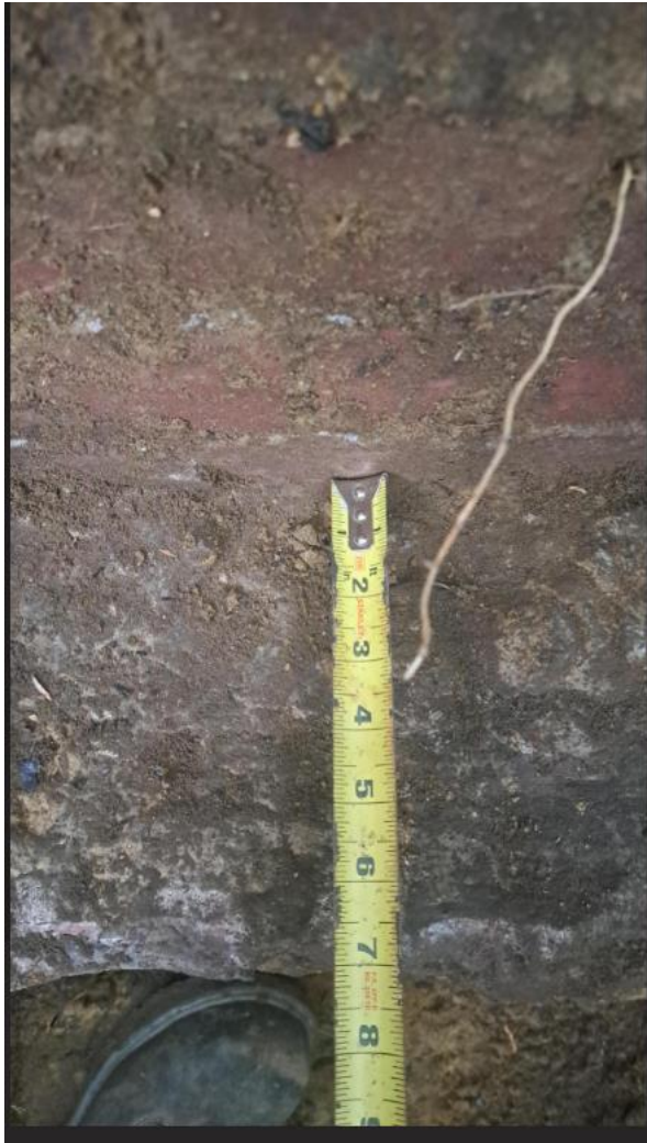
Photo 4: Projection of the stone footing along east wall of the testpit (175 mm)
