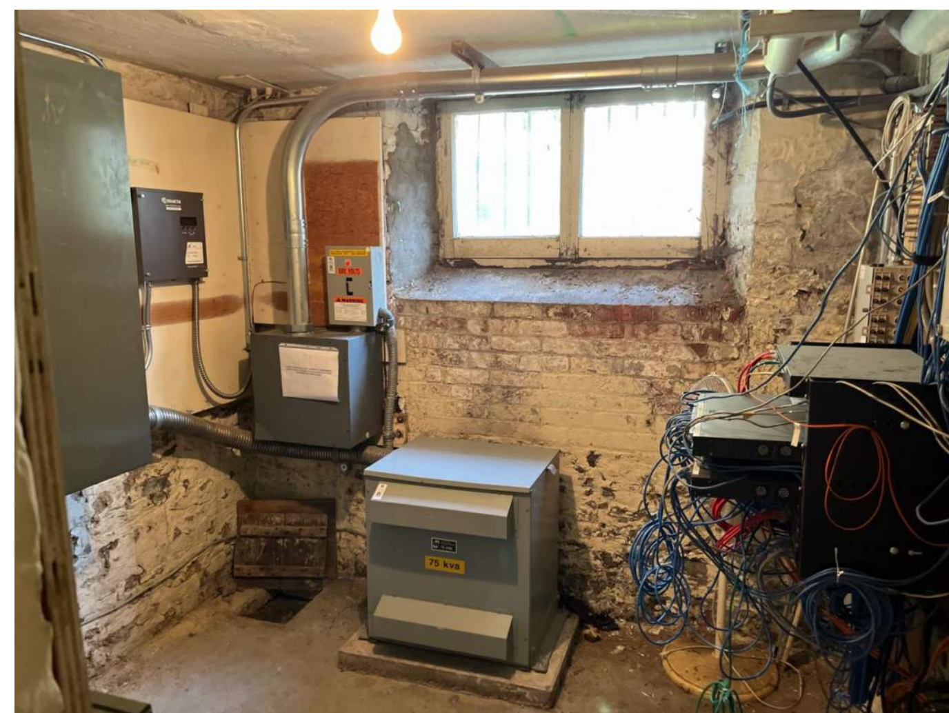
5 ELECTRICAL ROOM - NORTH WALL SCALE:N.T.S.
