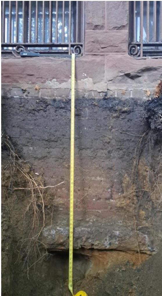
Photo 2: Below grade portion of the west exterior wall of the building / east wall of the test pit, showing top of the footing (looking East)
