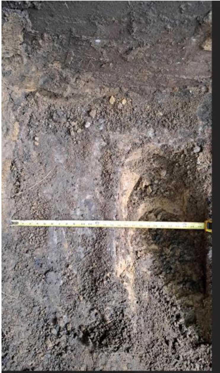
Photo 6: Projection of the stone footing along north wall of the test pit (360 mm)
