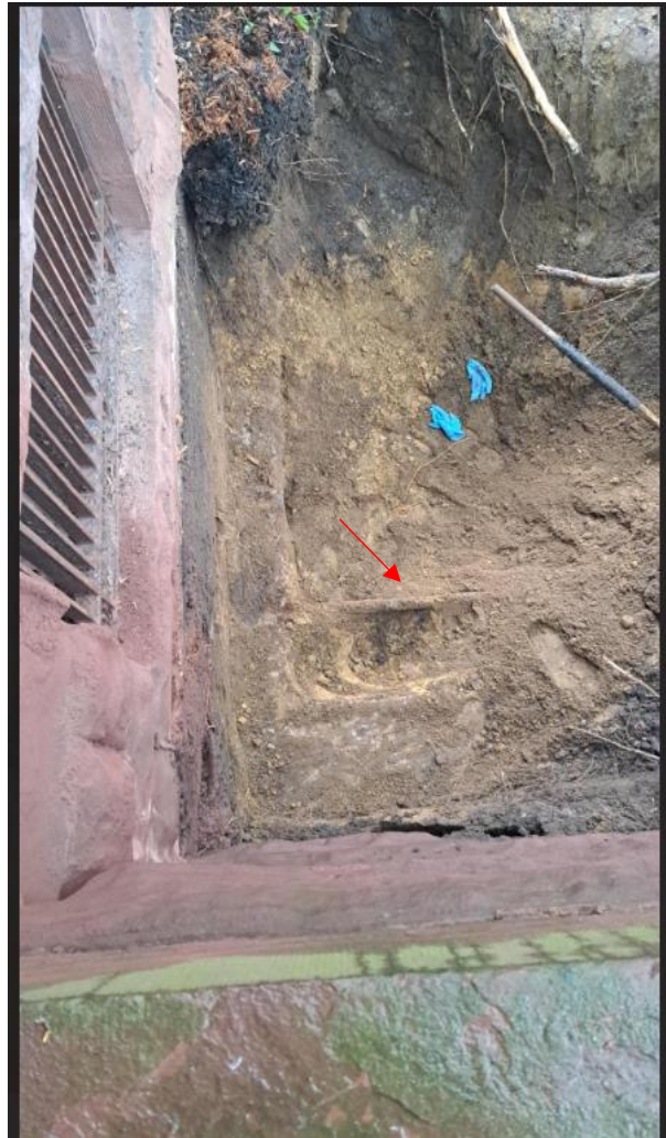
Photo 5: Top view below grade, looking down inside test pit, red arrow pointing to buried metal pipe
