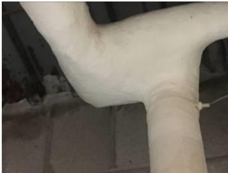
Basement Piping Elbows and Piping T Joints Canvas Wrapped Applied White, Cementitious Insulations Not Asbestos Containing
