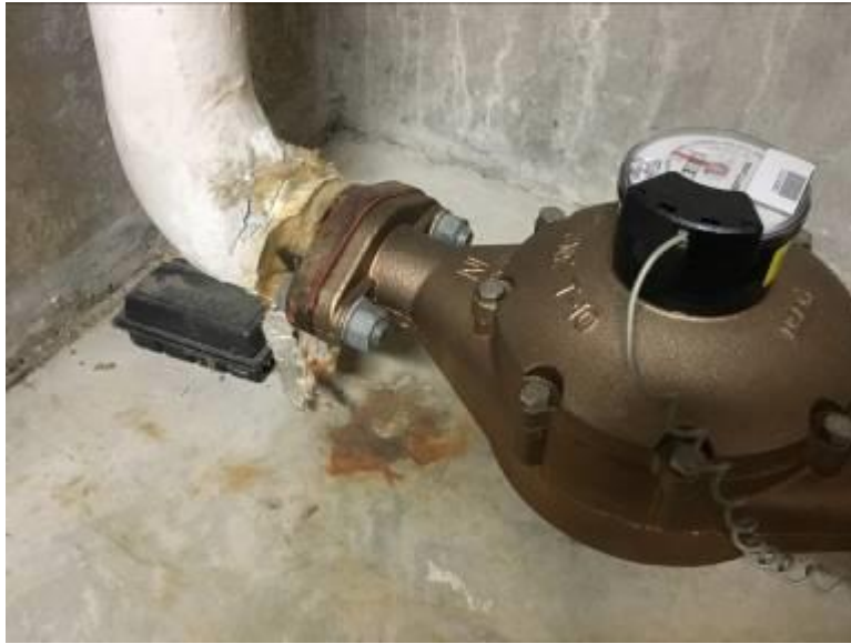
Basement Water Meter Piping Elbows and Piping T Joints Canvas Wrapped Applied White, Cementitious Insulations Not Asbestos Containing
