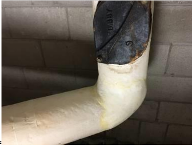
Basement Piping Elbows and Piping T Joints Canvas Wrapped Applied White, Cementitious Insulations Not Asbestos Containing
