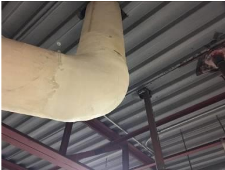
Apparatus Bay - Piping Elbows and Piping T Joints Canvas Wrapped Applied White, Cementitious Insulations Not Asbestos Containing
