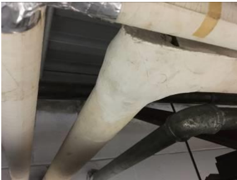
Basement Piping Elbows and Piping T Joints Canvas Wrapped Applied White, Cementitious Insulations Not Asbestos Containing
