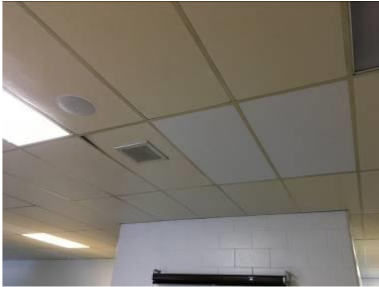
Main Floor Kitchen/Lounge/Sleeping Areas - T-Bar 2'X3' Ceiling Tiles White with Fibrous Glass Material Not Asbestos Containing
