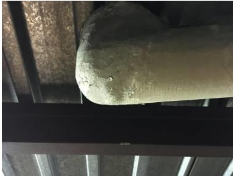
Basement Piping Elbows and Piping T Joints Canvas Wrapped Applied White, Cementitious Insulations Not Asbestos Containing
