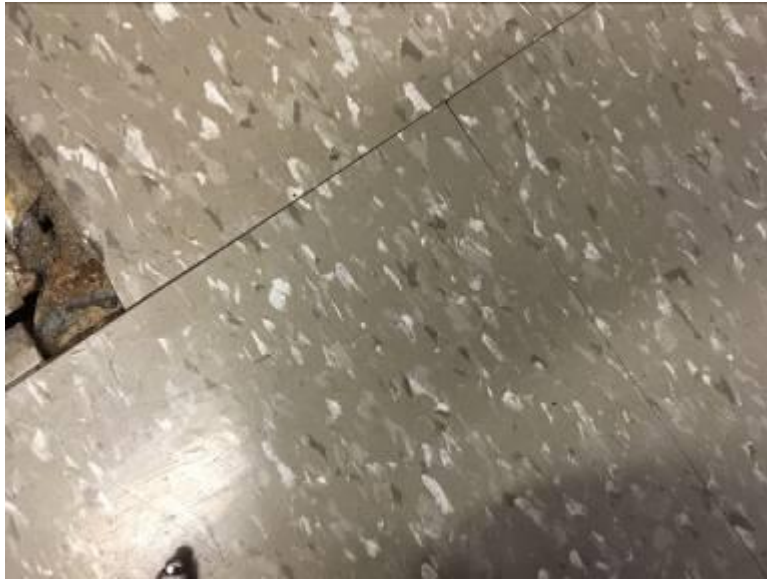
Main Floor Kitchen/Lounge/Sleeping Areas – 12” x 12” Vinyl Floor Tiles Beige White Flecked and Black Mastic Material Not Asbestos Containing
