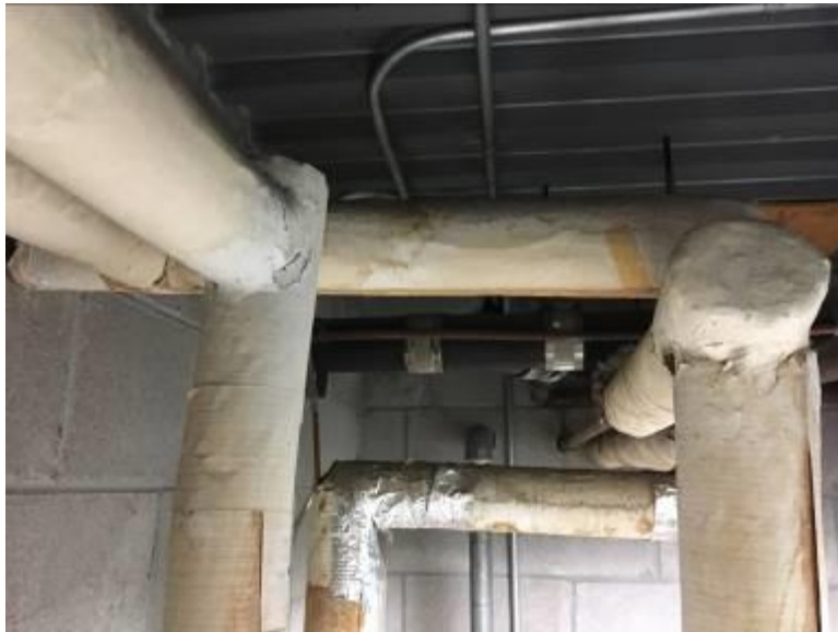
Basement Mechanical Room Piping Elbows and Piping T Joints Canvas Wrapped Applied White, Cementitious Insulations Not Asbestos Containing
