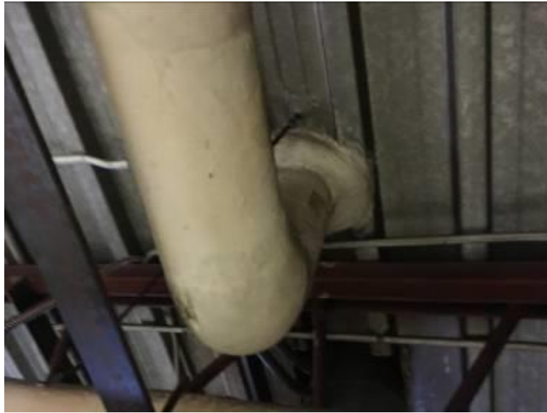
Apparatus Bay - Piping Elbows and Piping T Joints Canvas Wrapped Applied White, Cementitious Insulations Not Asbestos Containing
