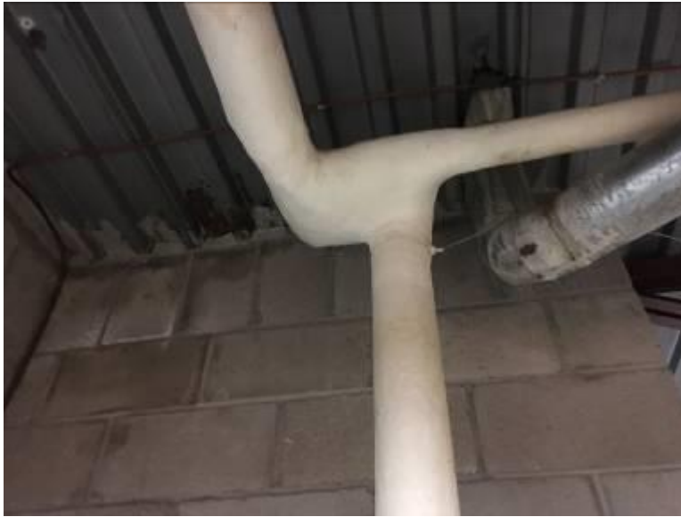
Basement Piping Elbows and Piping T Joints Canvas Wrapped Applied White, Cementitious Insulations Not Asbestos Containing
