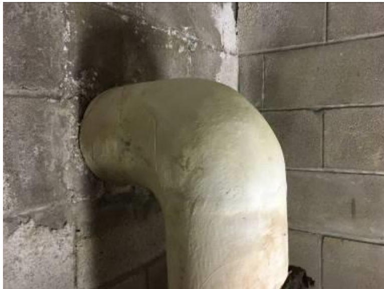
Basement Piping Elbows and Piping T Joints Canvas Wrapped Applied White, Cementitious Insulations Not Asbestos Containing
