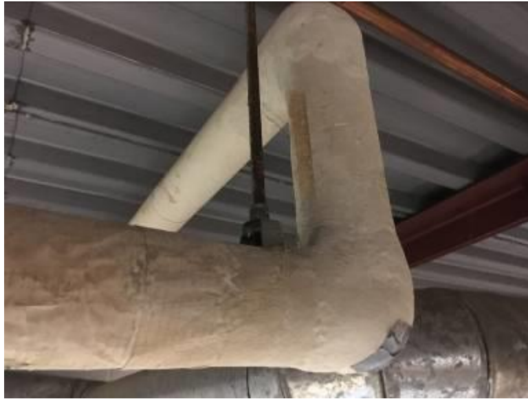
Basement - Piping Elbows and Piping T Joints Canvas Wrapped Applied White, Cementitious Insulations Not Asbestos Containing
