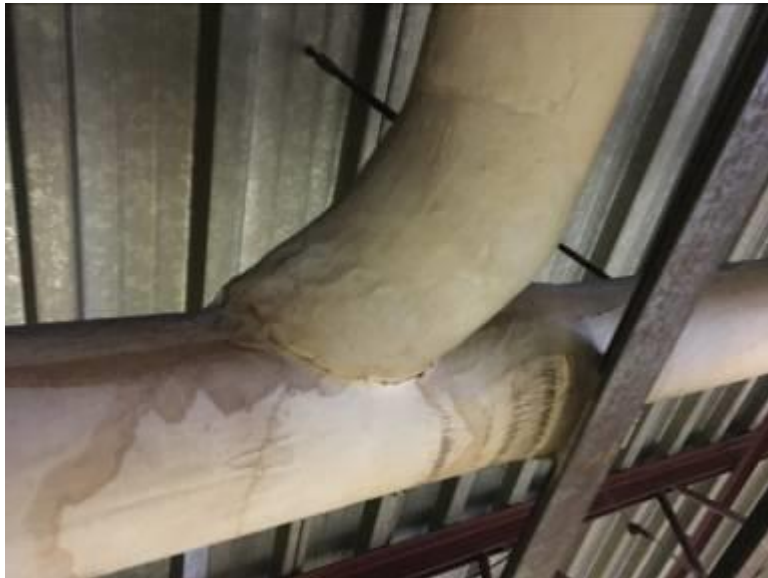
Basement Piping Elbows and Piping T Joints Canvas Wrapped Applied White, Cementitious Insulations Not Asbestos Containing
