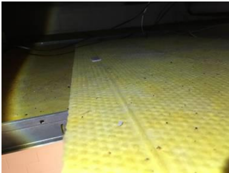
Main Floor Kitchen/Lounge/Sleeping Areas - T-Bar 2'X3' Ceiling Tiles White with Fibrous Glass Material Not Asbestos Containing
