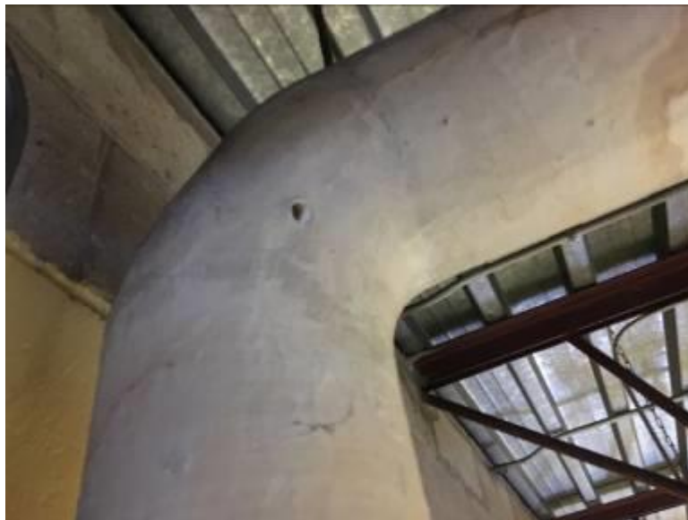
Apparatus Bay - Piping Elbows and Piping T Joints Canvas Wrapped Applied White, Cementitious Insulations Not Asbestos Containing
