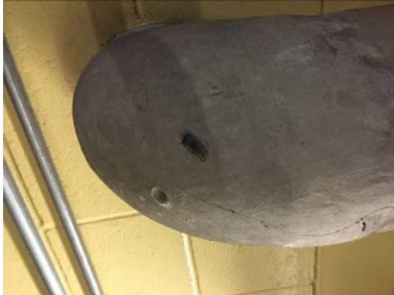
Apparatus Bay - Piping Elbows and Piping T Joints Canvas Wrapped Applied White, Cementitious Insulations Not Asbestos Containing
