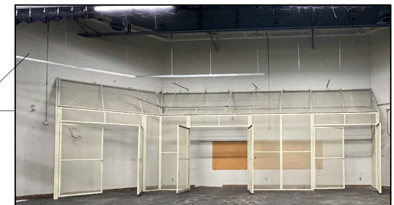
EXISTING CAGE TO REMAIN. H:21.98 ft. EXISTING BAR ABOVE THE CAGE. H:14.44 ft.
