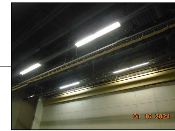
REPLACE THE EXISTING LIGHTING FIXTURES WITH THE NEW LED LIGHT FIXTURES. REFER TO ITEM 5.1 IN SCHEDULE.
