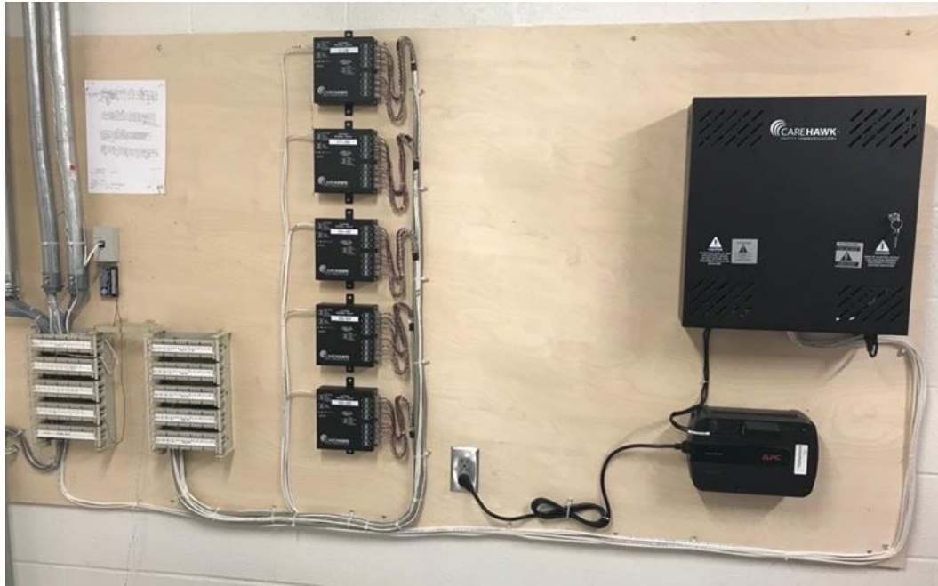
Figure 1: PA system cabling and termination to BIX panel, with service loops and neat cabling
