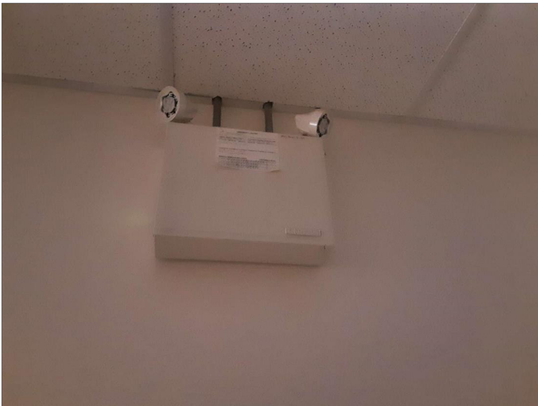
Pb Products, V9000(Yes), BATTERIES IN EMER. LIGHTS, Corridor (Location #: 34)
