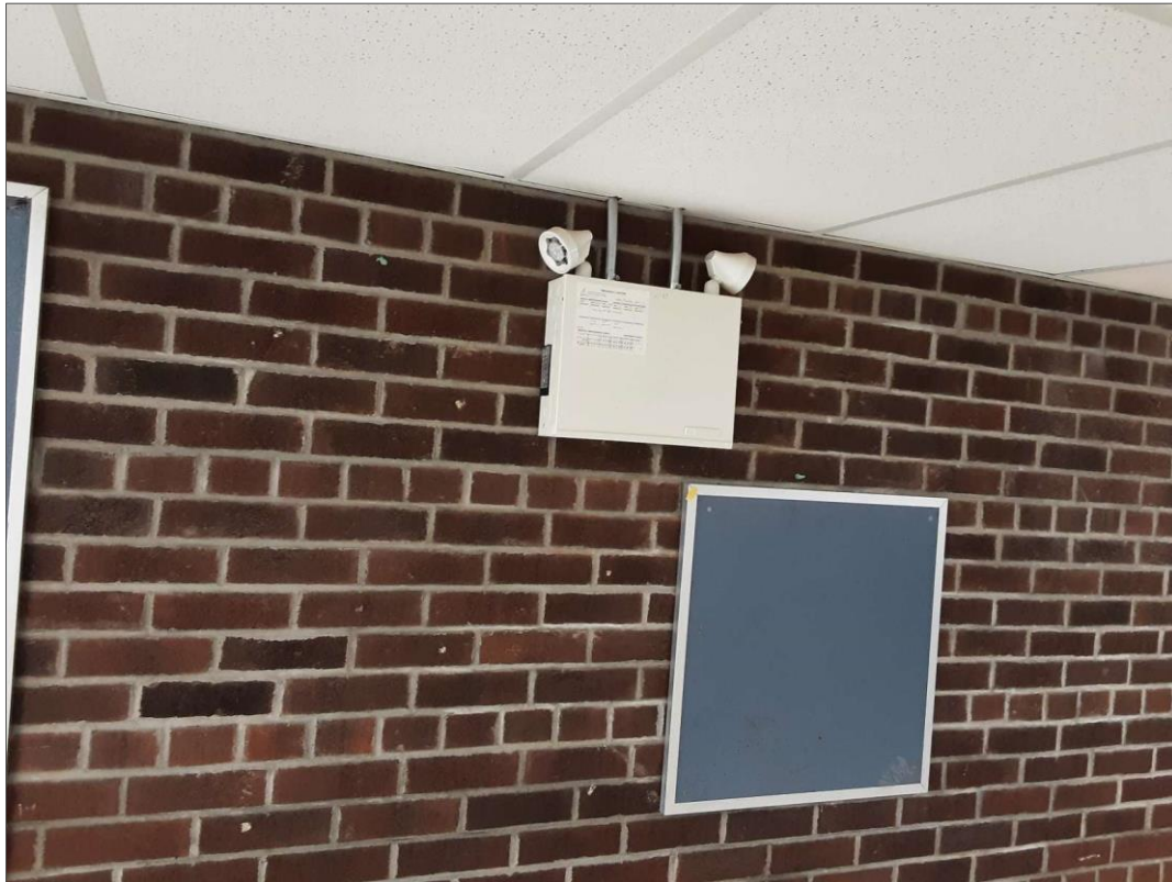
Pb Products, V9000(Yes), BATTERIES IN EMER. LIGHTS, Corridor (Location #: 47)
