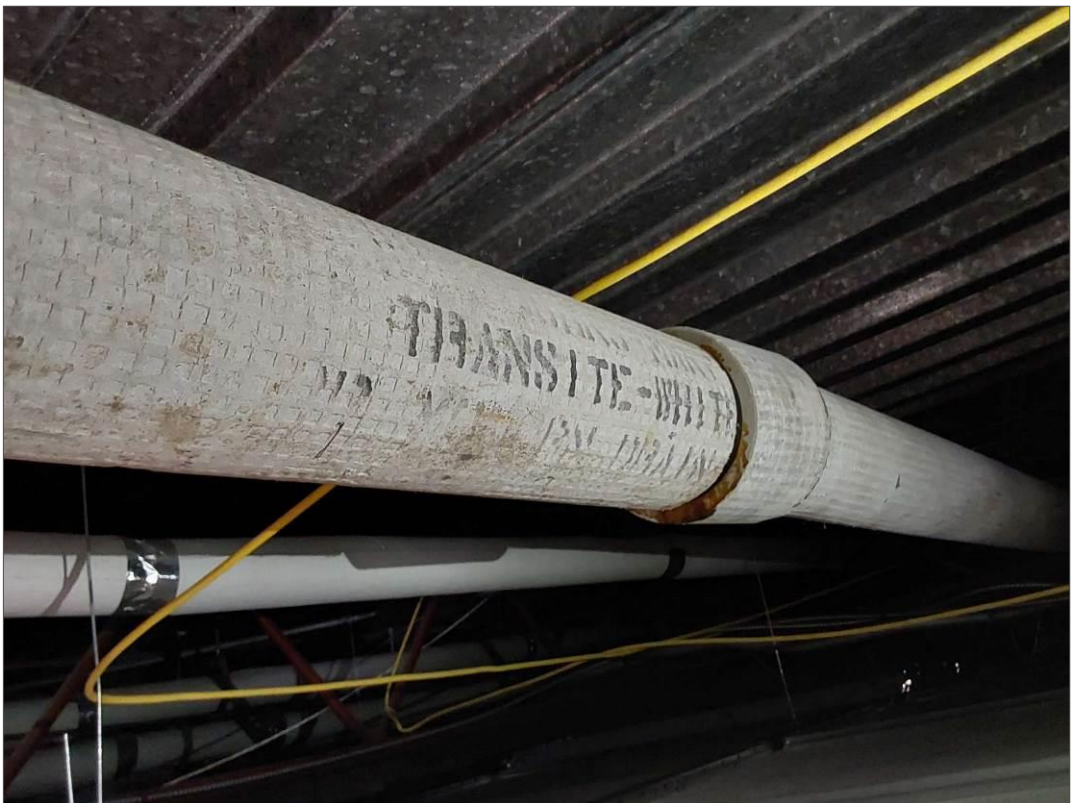
V9000 (Confirmed Asbestos), Piping, Cement Product, Kindergarten (Location #: 52) Transite pipe
