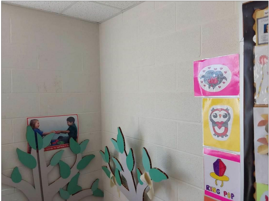
S0066E (None), Off-white paint on masonry wall, Other, Paint, 2014 Phase Construction (Location #: 77) Paint on masonry block
