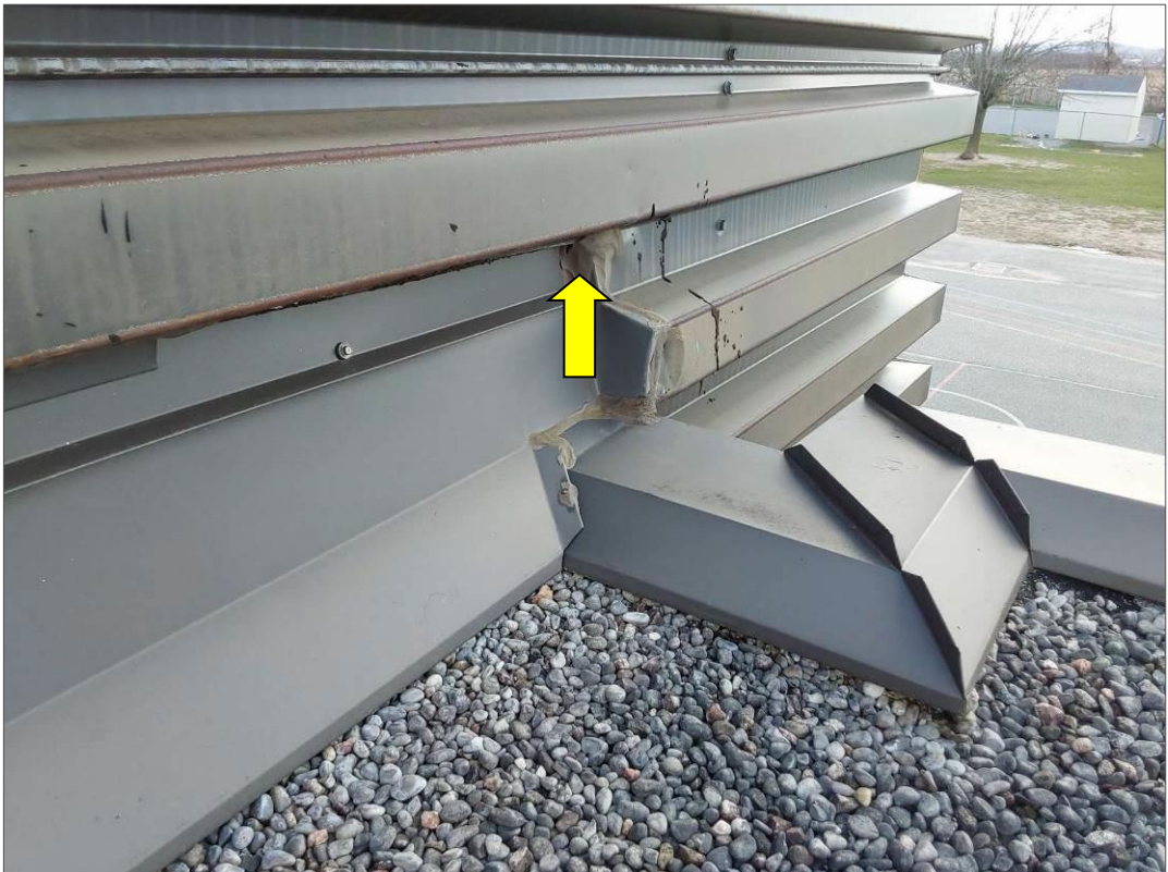
S0077A (None), Brown caulking on flashing, Other, Caulking, Roof F2 (Location #: 88)
