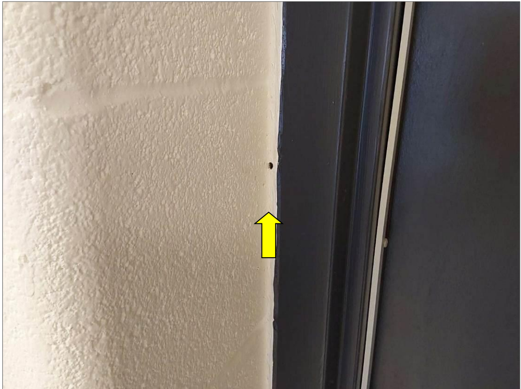
S0068A (None), White caulking around door frames, Other, Caulking, 2014 Phase Construction (Location #: 77)
