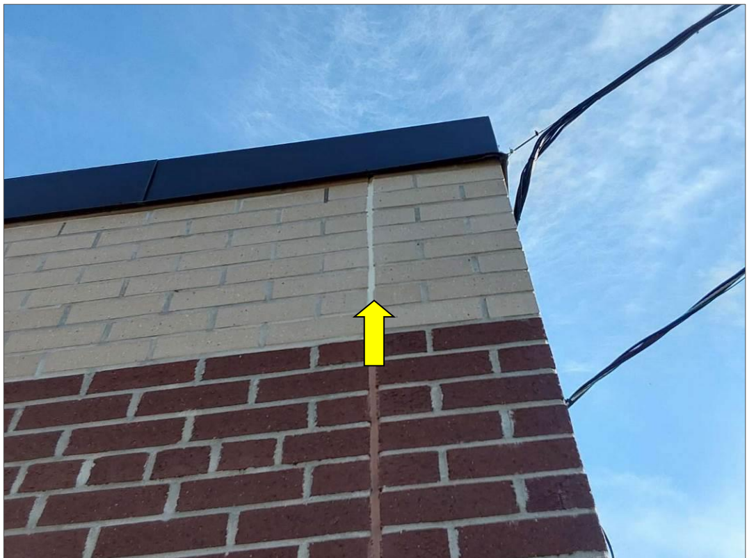
S0071C (None), White caulking on exterior brick, Other, Caulking, Exterior Wall For Renovation (Location #: 81)
