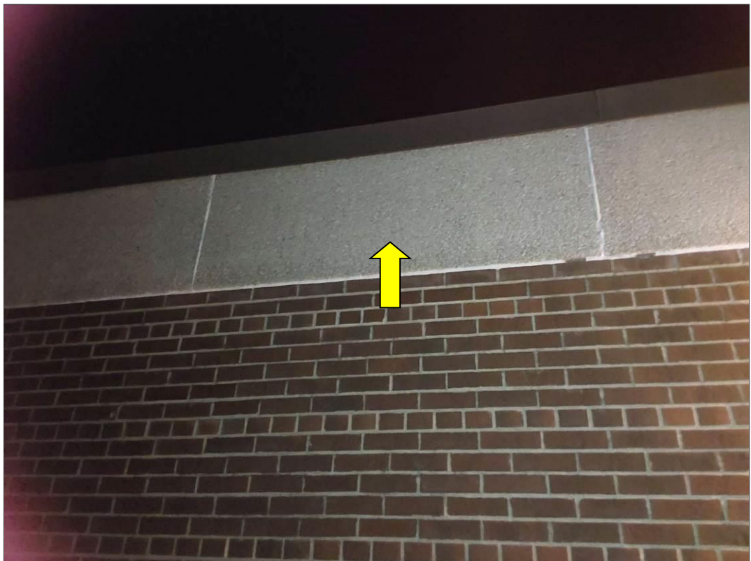
V9500 (Presumed Asbestos), Other, Fascia, Cement Product, Exterior Wall For Renovation (Location #: 81) Transite presumed present behind decorative panel
