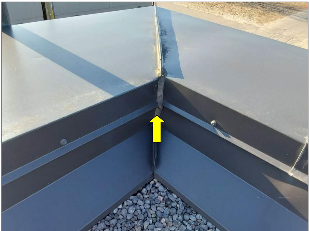
S0075C (None), Grey caulking on flashing, Other, Caulking, Roof H (Location #: 86)
