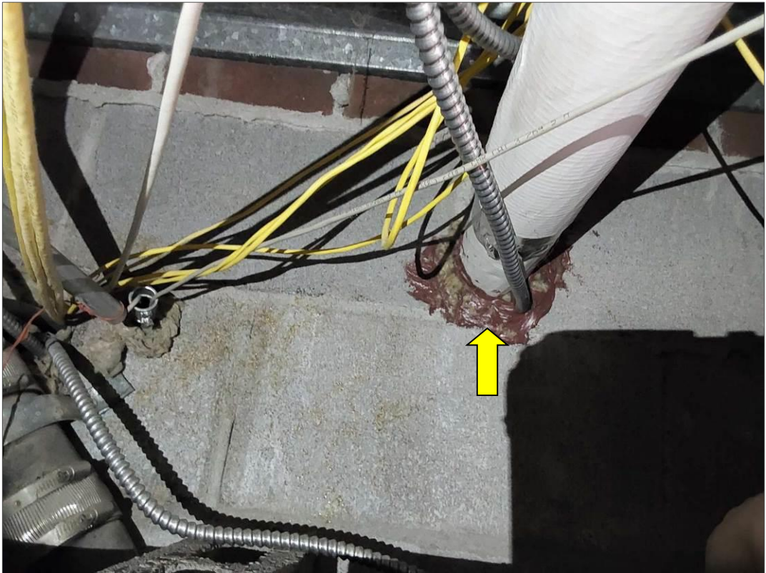
S0080C (None), Brown firestopping, Other, Firestopping (mastic), Corridor (Location #: 48)
