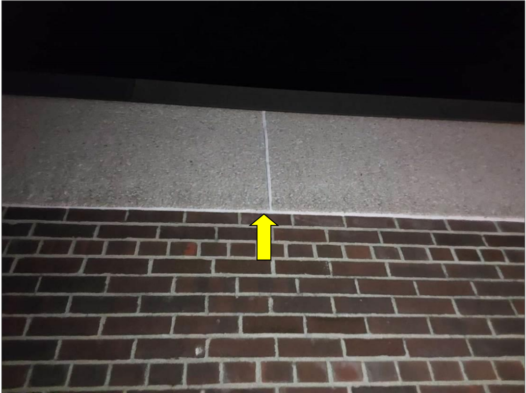
S0048C (Confirmed Asbestos), White caulking on fascia, Other, Fascia, Caulking, Exterior Wall For Renovation (Location #: 81)
