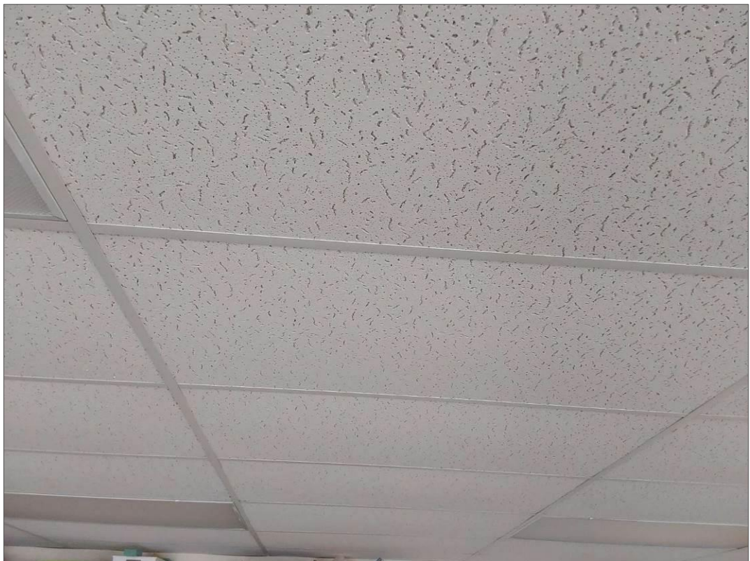
V0000 (None), 24"X48" large ridge with scattered pinhole, Ceiling, Ceiling Tiles (lay-in), 2014 Phase Construction (Location #: 77) Date stamped 08/14/13
