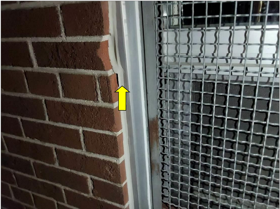
S0082C (None), Light grey caulking along window cages, Wall, Caulking, Exterior Wall For Renovation (Location #: 81)
