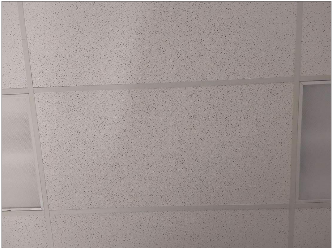
V0000 (None), 24x48 lay-in, fleck and pinhole, Ceiling, ACOUSTIC TILE, Ceiling Tiles (lay-in), Kindergarten (Location #: 52) Date stamp 08/09/18
