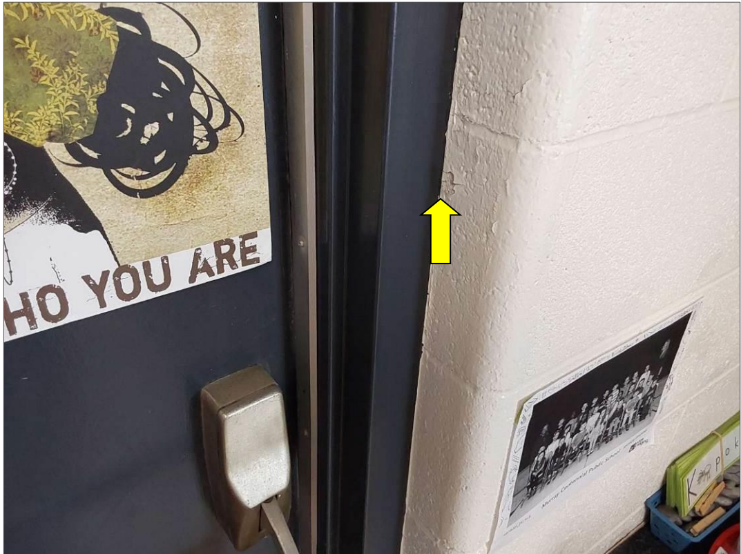
S0044A (None), White caulking on door frame interior side of exterior door, Other, Door, Caulking, Kindergarten (Location #: 52)
