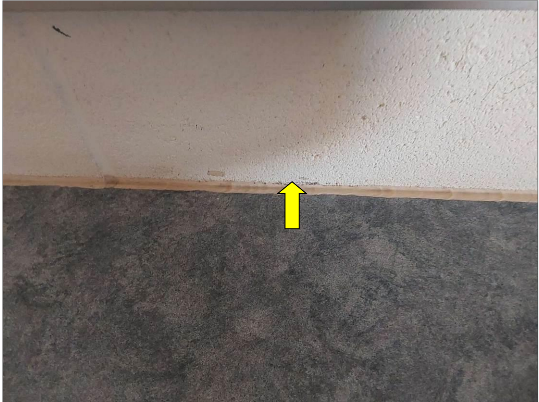
S0031 (None), Other, Caulking, Classroom (Location #: 50)
