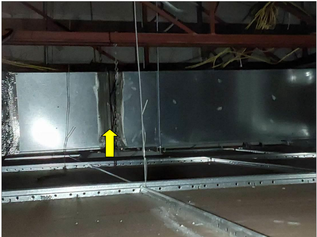
S0039A (None), Grey duct mastic, Duct, Mastic, Grey, Classroom (Location #: 40)
