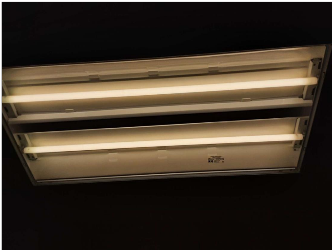
Mercury, V9000(Yes), LIGHT FIXTURE, Electrical Room (Location #: 8)
