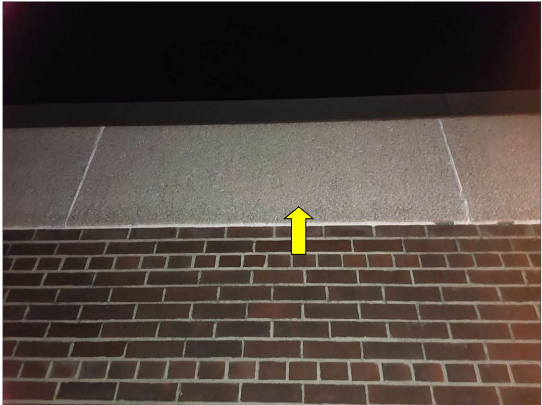
S0050C (None), clear pebbled rock fascia panels, Other, Fascia, Unidentified Material, Exterior Wall For Renovation (Location #: 81)
