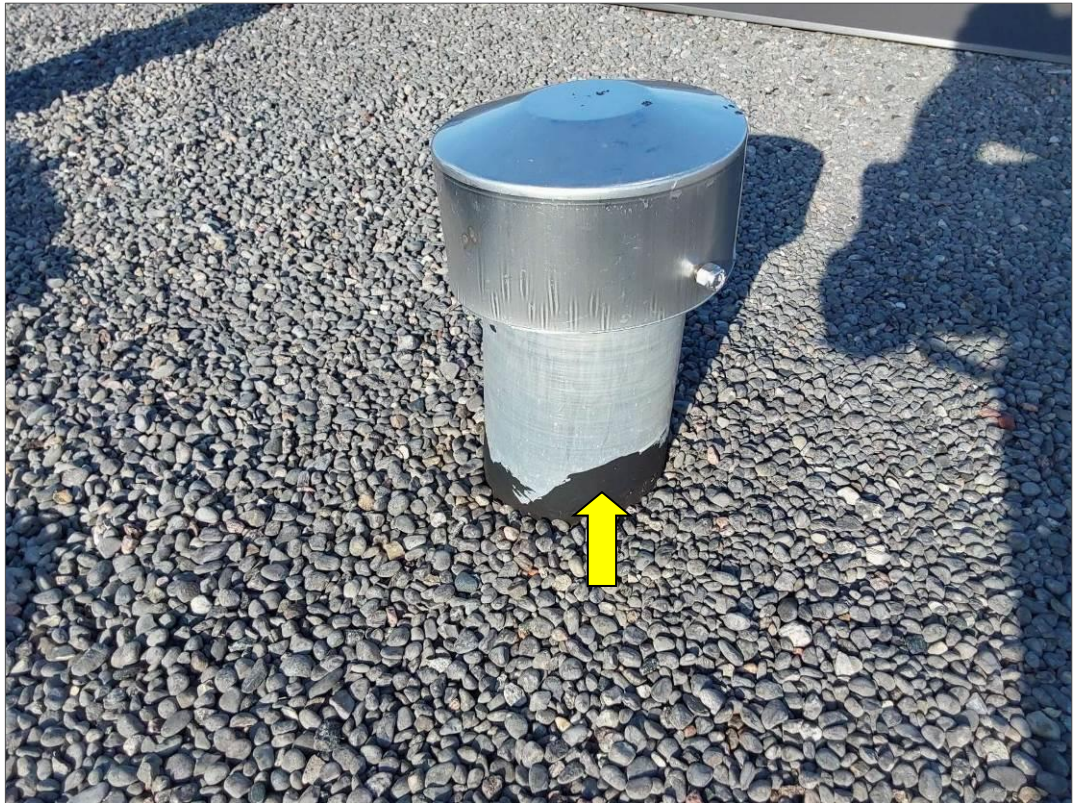
S0074C (None), Tar on vents, Other, Tar, Roof H (Location #: 86)
