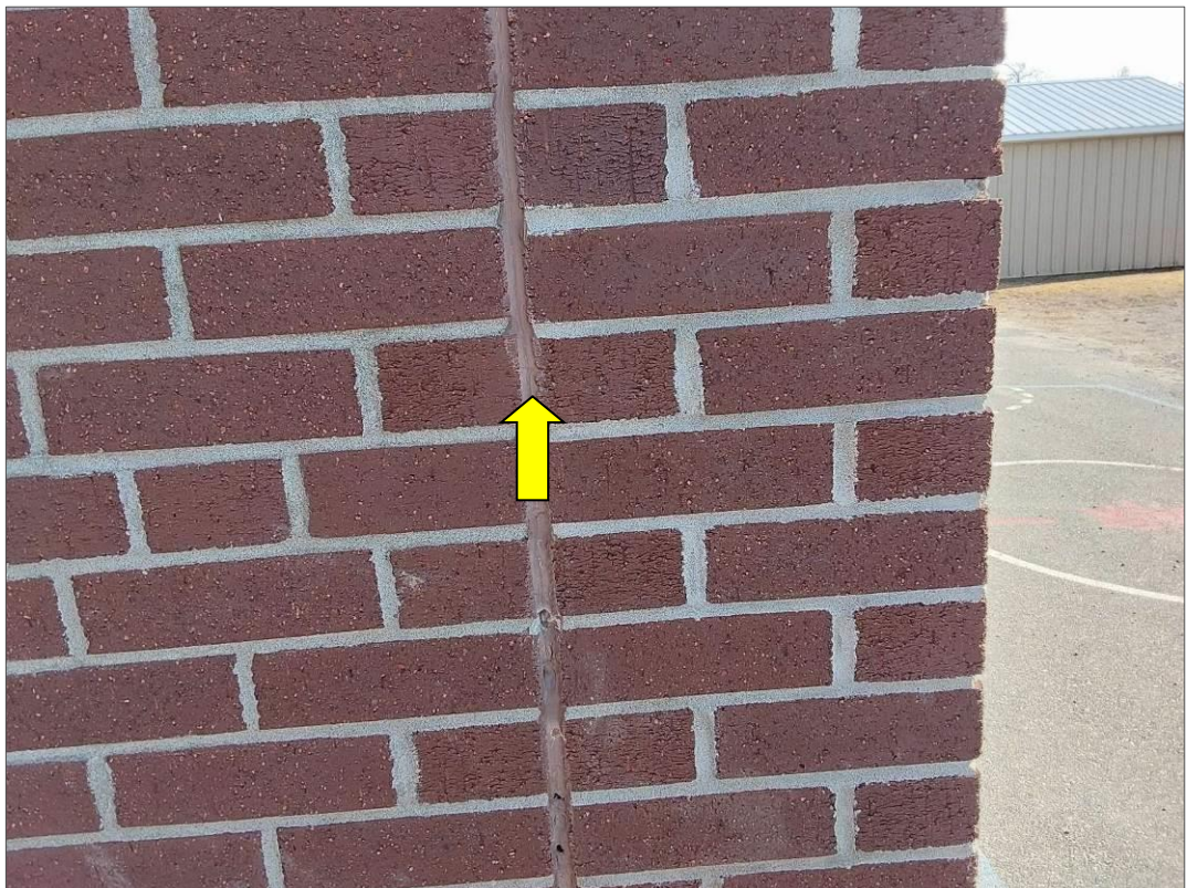
S0069C (None), Brown caulking on expansion joints and exterior door frame, Other, Caulking, Exterior Wall For Renovation (Location #: 81)
