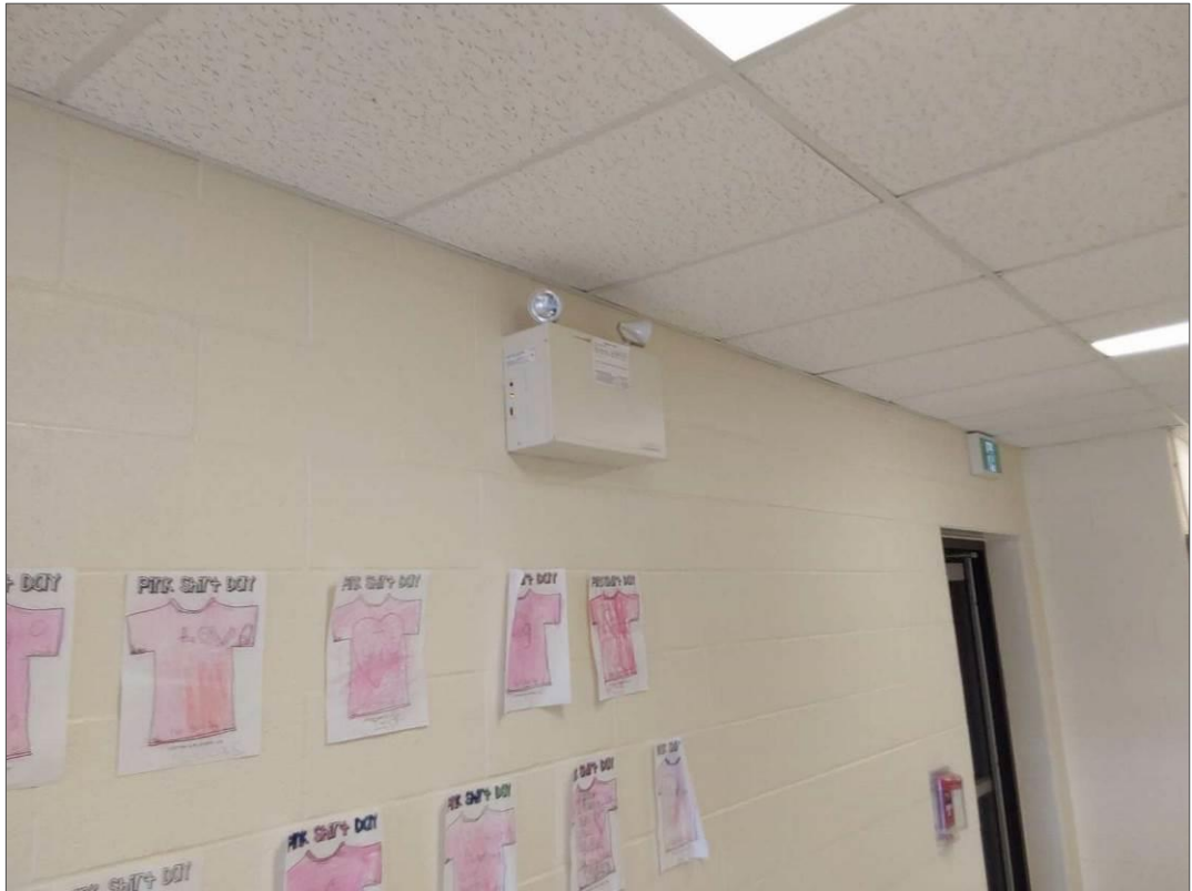
Pb Products, V9000(Yes), BATTERIES IN EMER. LIGHTS, 2014 Phase Construction (Location #: 77)
