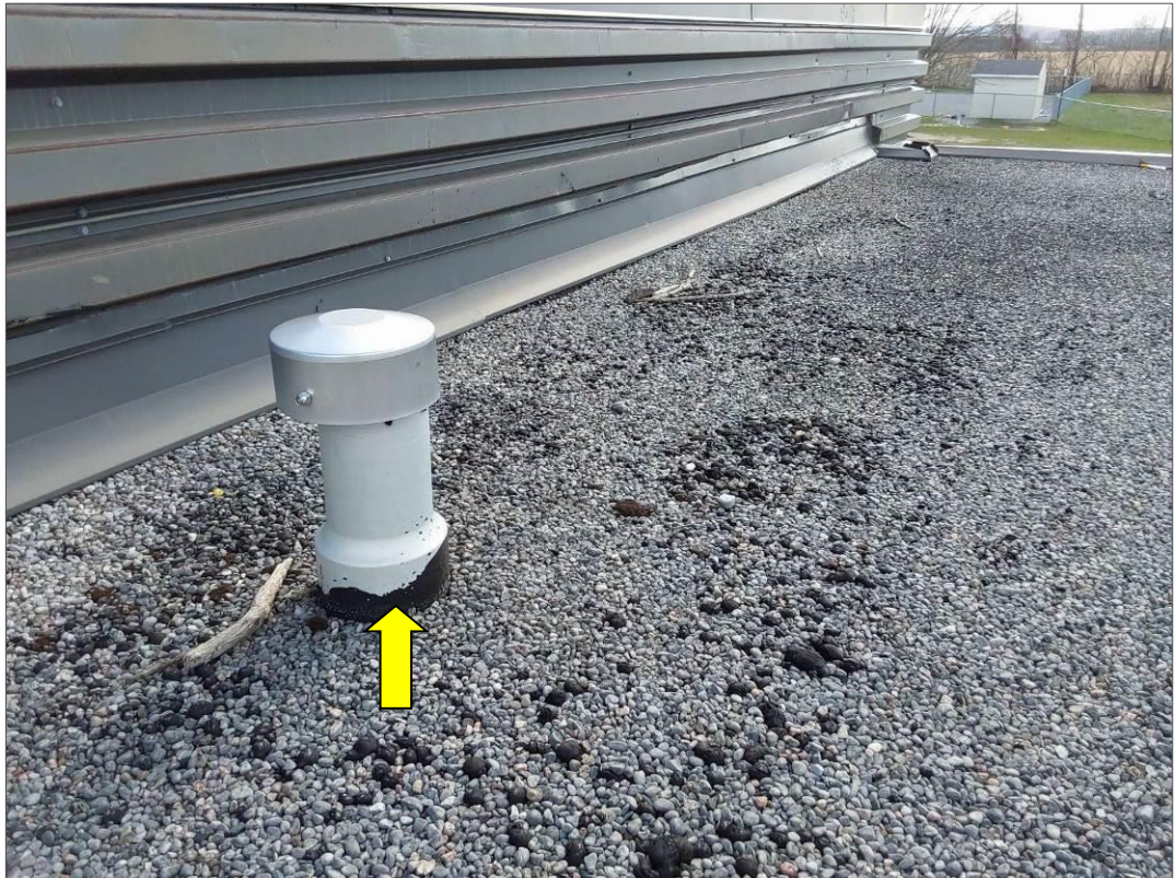
S0078A (None), Tar on vents, Other, Tar, Roof F2 (Location #: 88)
