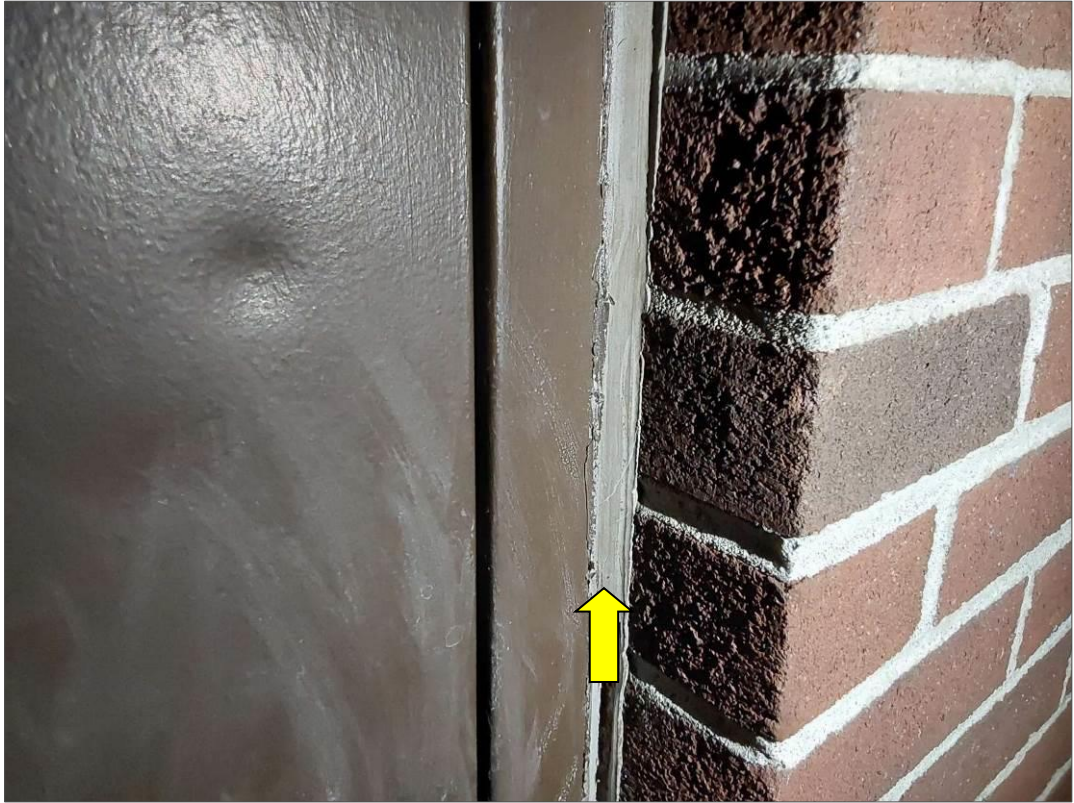
PCB, P0001(No), CAULKING, Grey caulking on exterior door, Exterior Wall For Renovation (Location #: 81)
