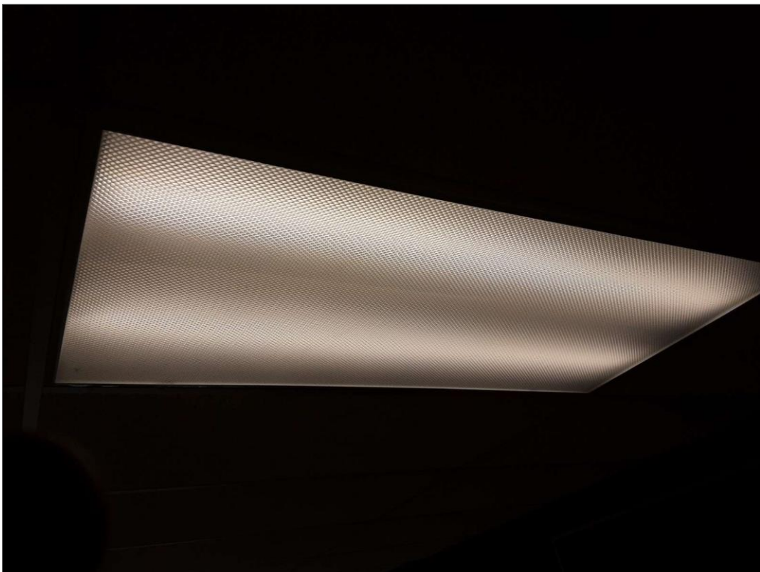
Mercury, V9000(Yes), LIGHT FIXTURE, Corridor (Location #: 47)
