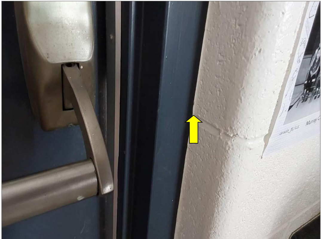
PCB, P0002(No), CAULKING, White caulking on interior side of door to exterior, Kindergarten (Location #: 52)
