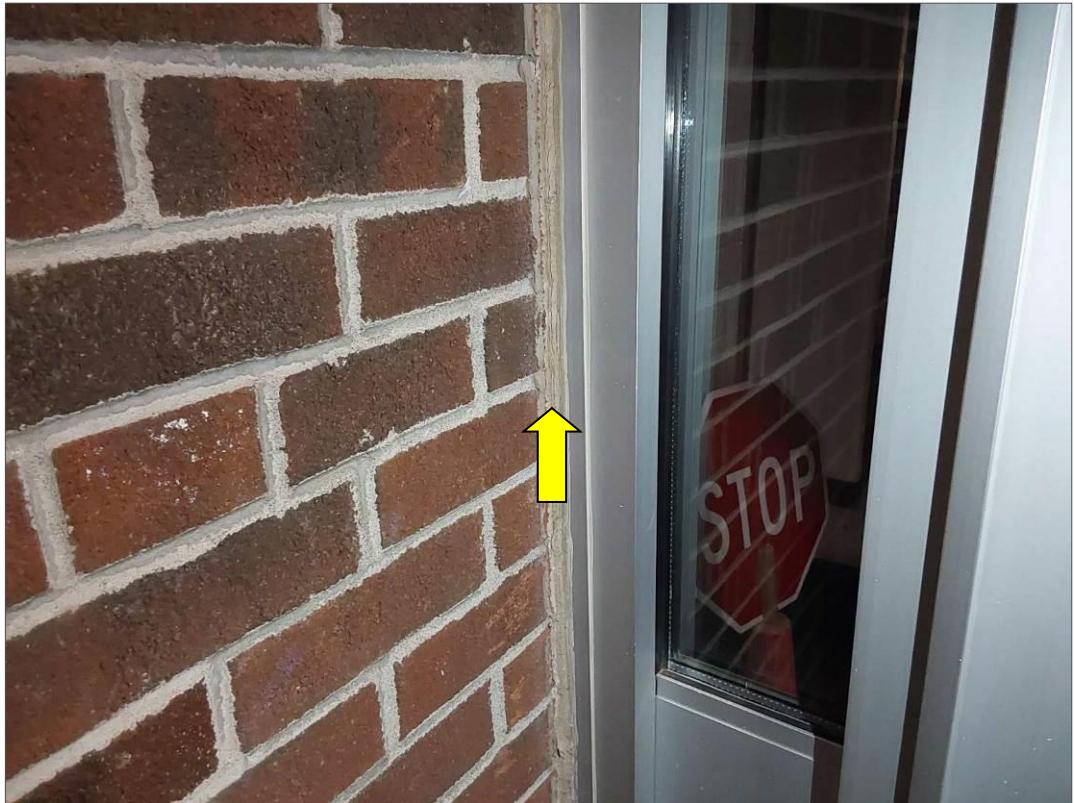
PCB, P0003(No), CAULKING, Dark grey caulking on exterior door, Exterior Wall For Renovation (Location #: 81)
