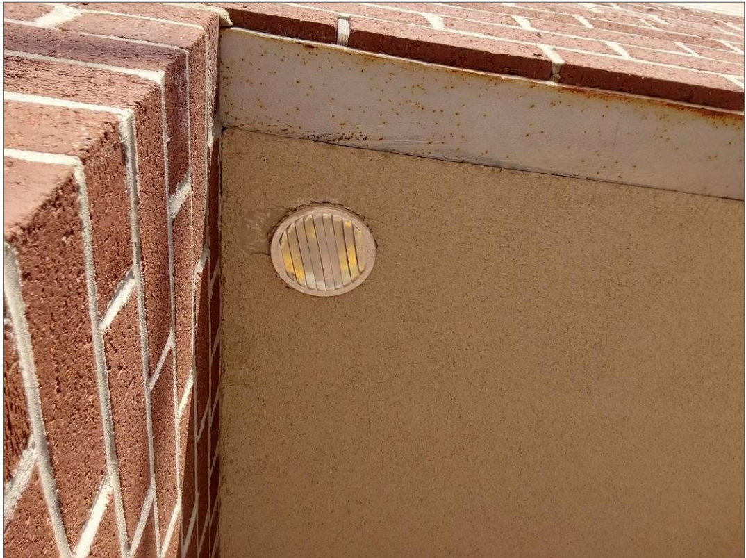
V9500 (Presumed Asbestos), Other, Soffit, Cement Product, Exterior Wall For Renovation (Location #: 81) Transite presumed present behind texture coat and decorative panel
