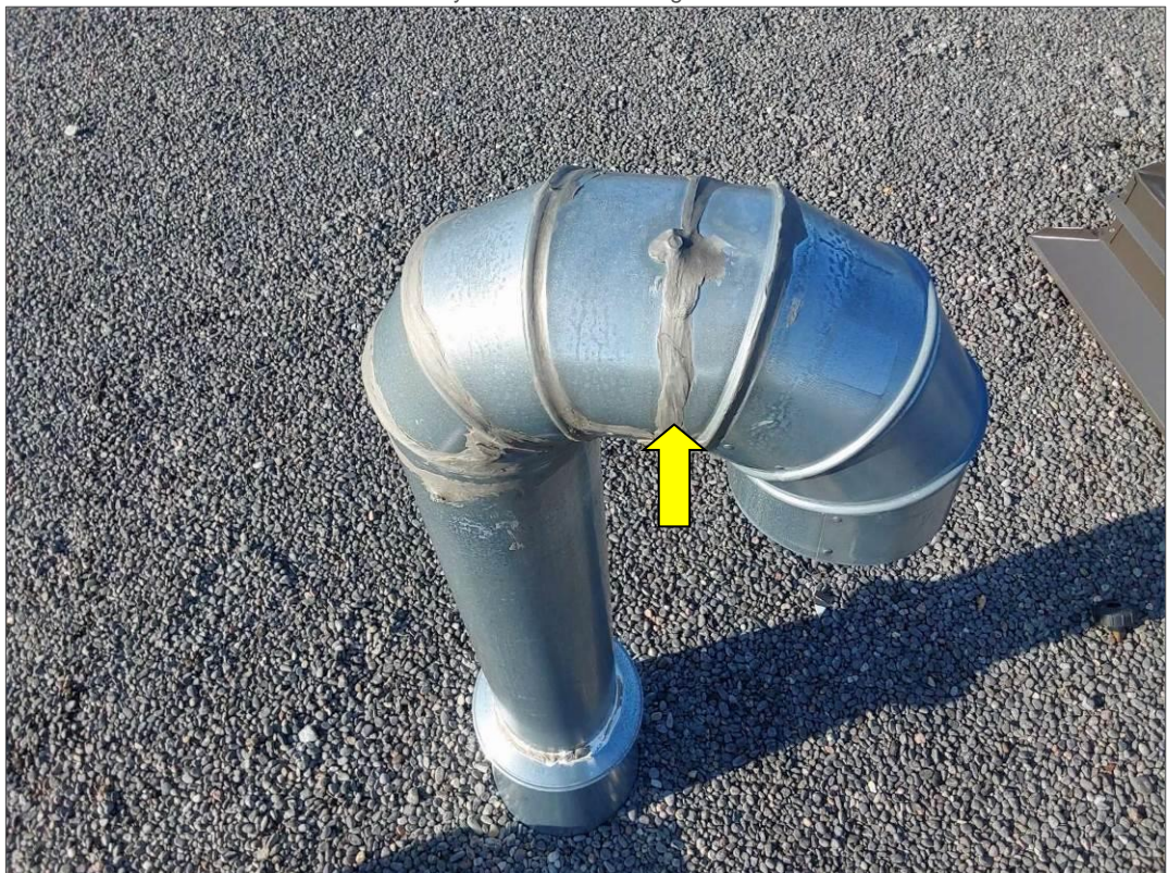
S0073C (None), Grey duct mastic, Duct, Mastic, Roof H (Location #: 86)
