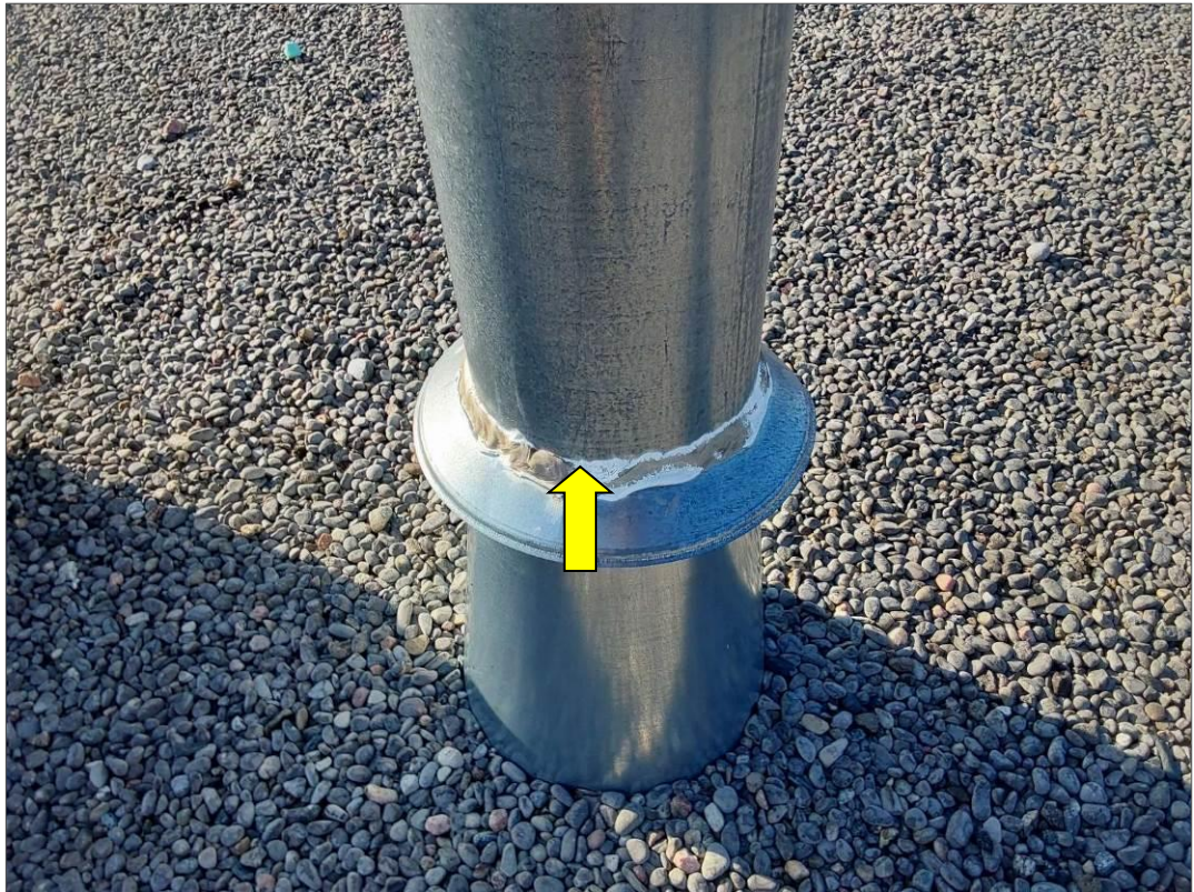
S0072C (None), White caulking on duct, Duct, Caulking, Roof H (Location #: 86) Grey duct mastic covering s0073
