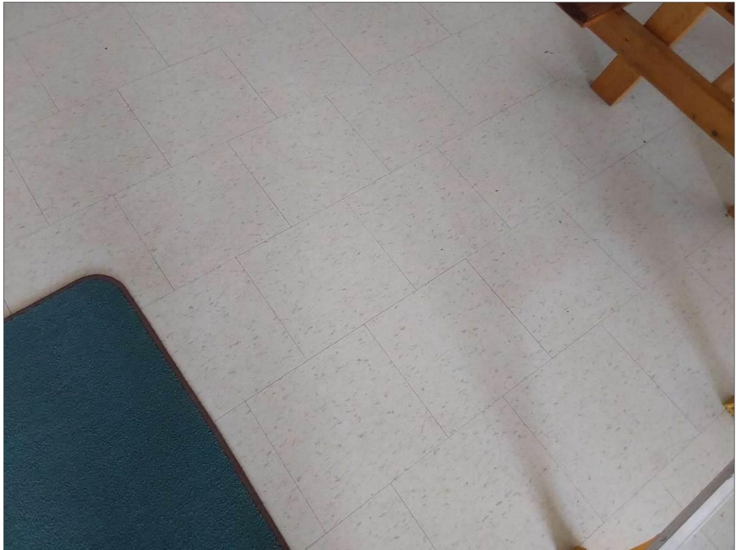
V0000 (None), 12" x 12" white with grey flecks, Floor, Vinyl Floor Tile and Mastic, 2014 Phase Construction (Location #: 77) Installed in 2014
