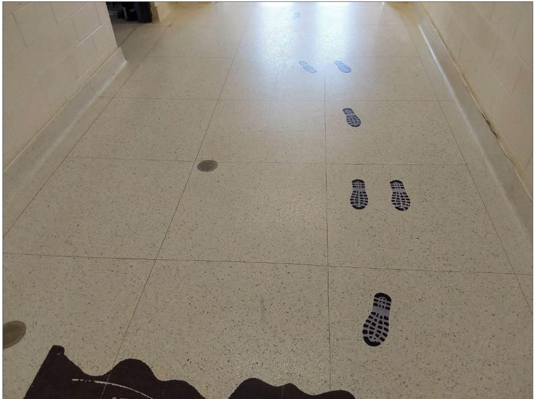
V9500 (Presumed Asbestos), Floor, Terrazzo, 2014 Phase Construction (Location #: 77)
