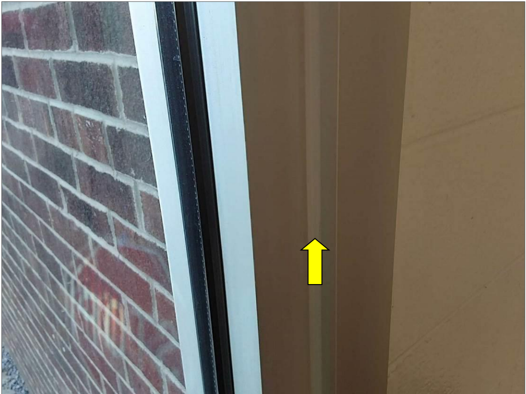
S0040A (None), Grey caulking on 2006 date stamped door, Other, Door, Caulking, Corridor (Location #: 48)
