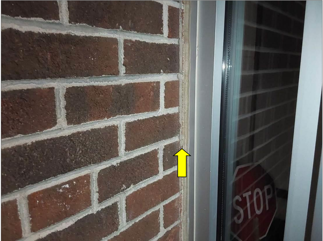
S0046C (None), Dark grey caulking on exterior door, Other, Door, Caulking, Exterior Wall For Renovation (Location #: 81)
