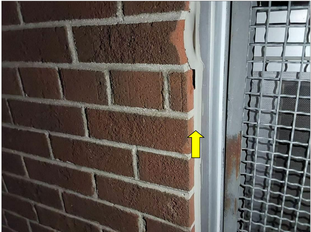
PCB, P0005(No), CAULKING, Light grey caulking along window cages, Exterior Wall For Renovation (Location #: 81)
