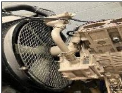
Generator, Generator Room (Location 1-02).
