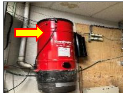
Superior Vacuum, Electrical Room (Location 1-10).
