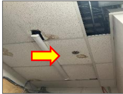
Water Staining on non-asbestos ceiling tiles, Electrical Room (Location 1-10).
