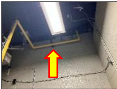
Uninsulated pipe, Generator Room (Location 1-02).
