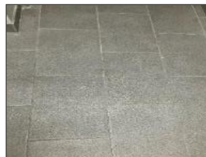
Presumed asbestos-containing thin-set present under 12"x24" grey ceramic tiles, Electrical Room (1-10).
