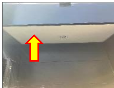
Non-asbestos stucco present on ceilings, Exterior (Location 0-00).
