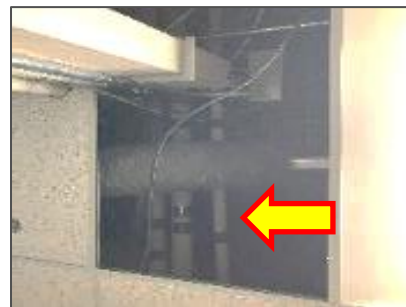
Pipe insulated with fibreglass and jacketed in canvas, Electrical Room (Location 1-10).
