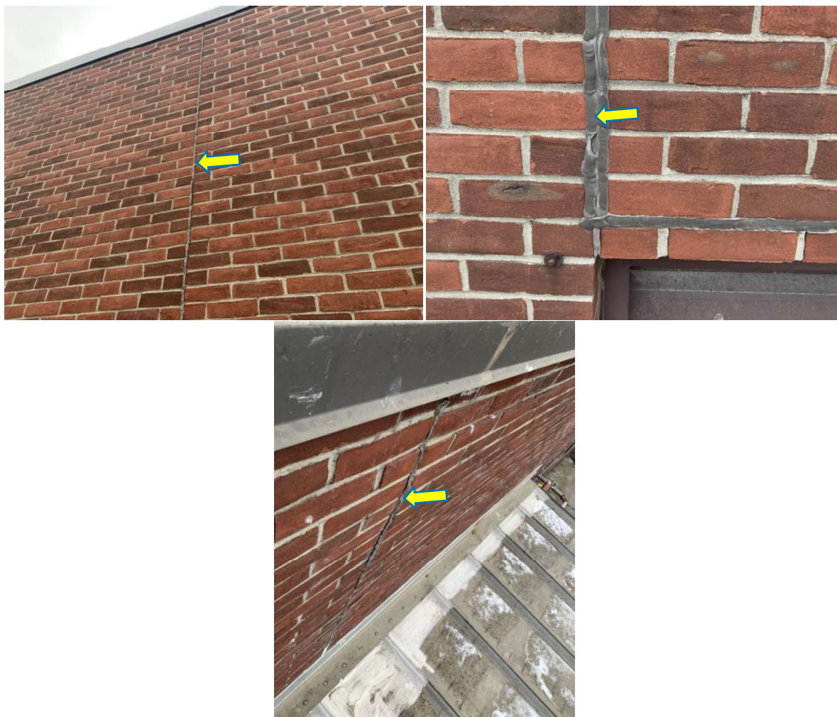
Photograph No. 3.1, 3.2 and 3.3: View of the non-asbestos brick wall joint caulking on the exterior of the subject building.
