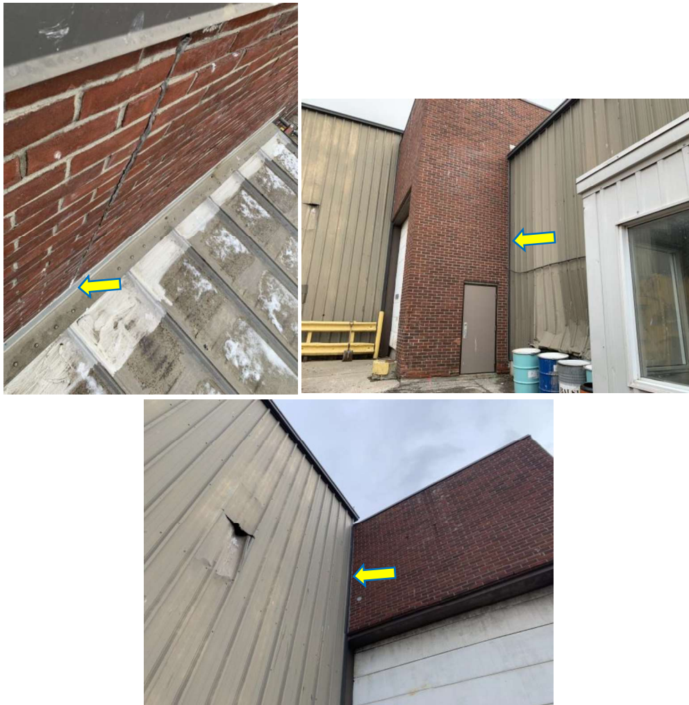
Photograph No. 4.1, 4.2, and 4.3: View of the asbestos containing caulking associated with metal frame of the loading dock and brick wall on the exterior of the subject building.
