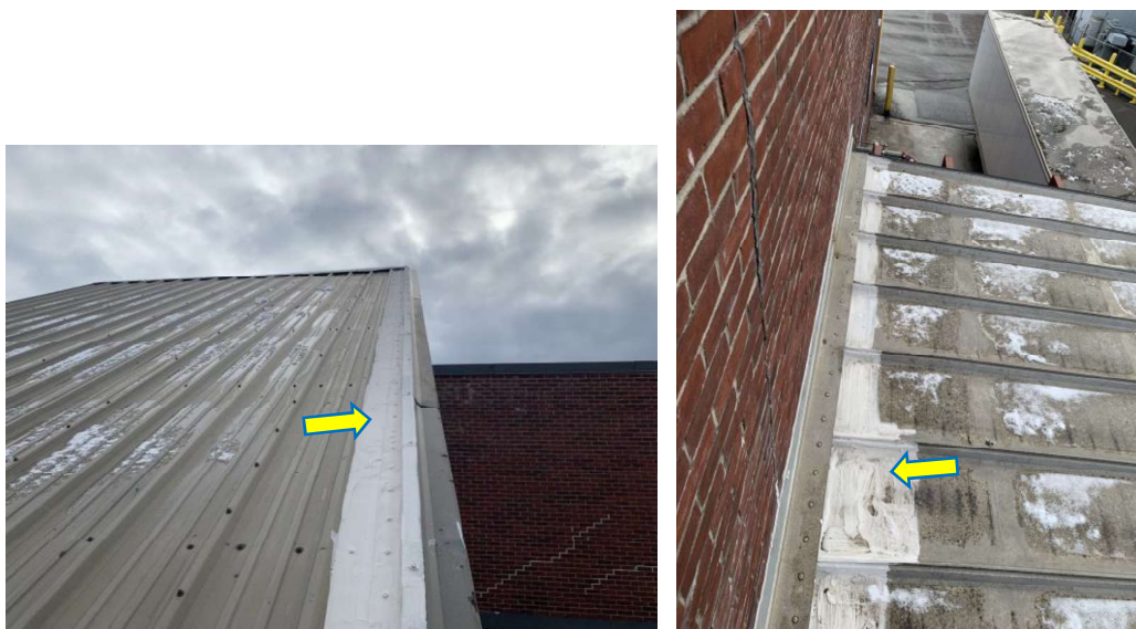
Photograph No. 2.1 and 2.2: View of the non-asbestos sealant (trowel-applied) on the main metal roof of the subject building. Similar sealant was observed on the loading dock metal roof.
