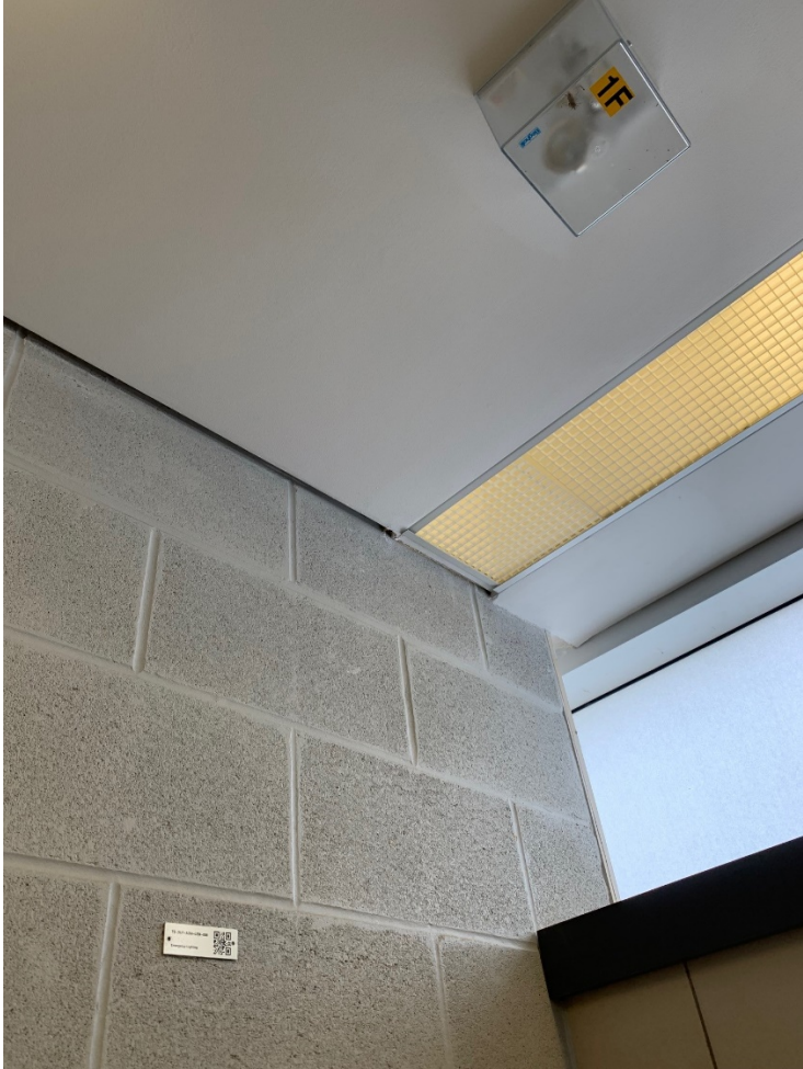
Figure 5: Tag Affixed on the Wall For Ceiling Asset
