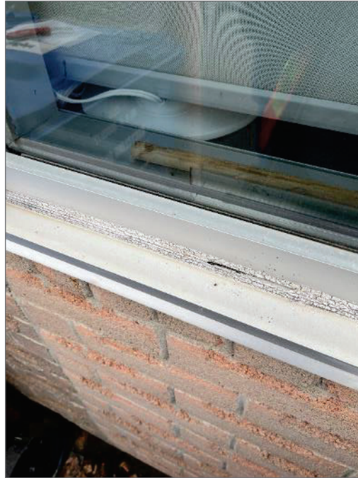
Photo 3 - Asbestos containing grey and off-white caulking on window frame.
