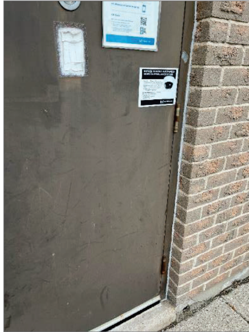
Photo 7 - Brown paint on doors.
