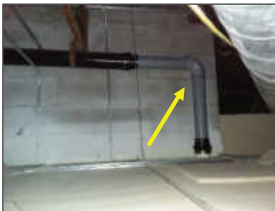
Photo 1: Non-asbestos PVC piping section which replaced the asbestos-containing Transite pipe that is no longer present in the Front Reception Area (Loc.8).
