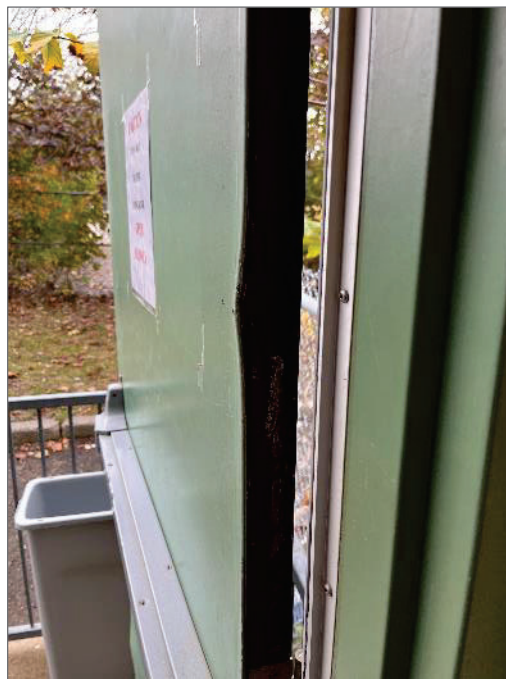
Photo 8 - Black paint on doors.
