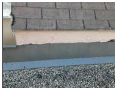
Paint, presumed to contain lead, present on metal attachment transition on roof section M (Loc. 5).
