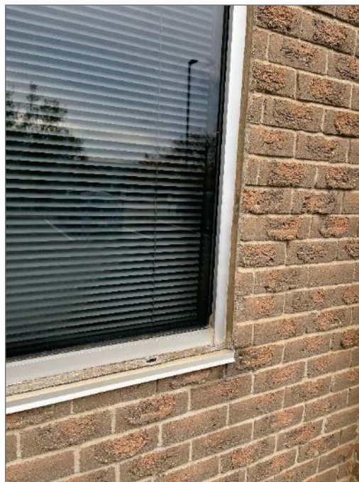
Photo 2 - Asbestos containing grey and off-white caulking on window frame.
