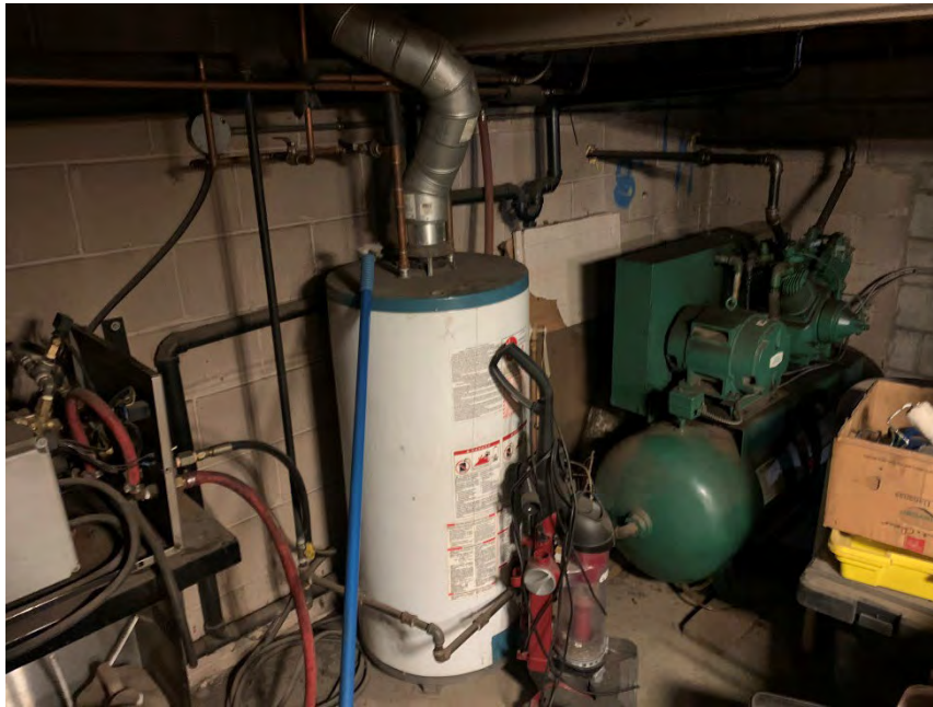
Photo 16 – Photo taken of the southern corner of the automotive garage facing south.
