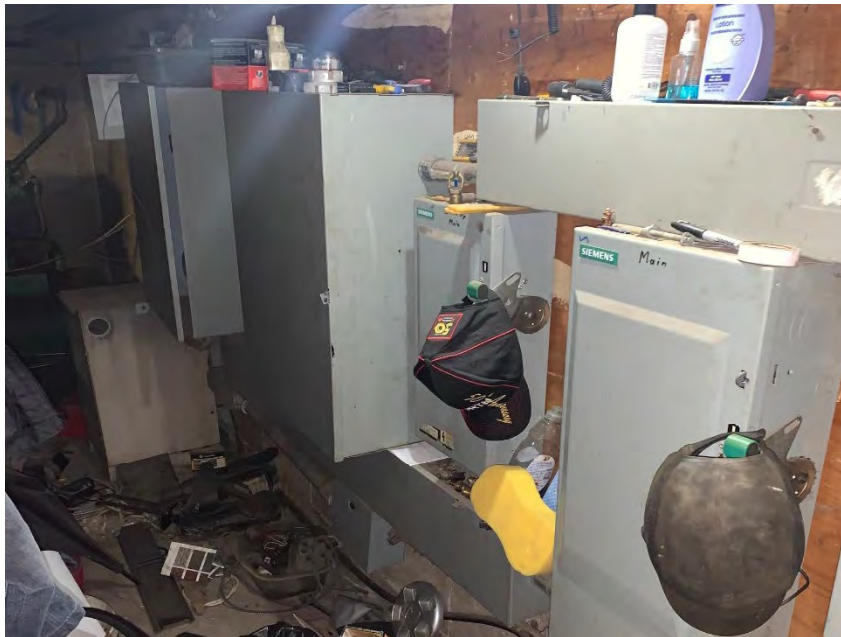
Photo 17 – Photo taken of the southern corner of the automotive garage facing south.
