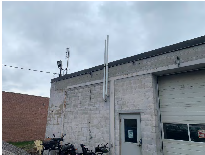
Photo 10 – Photo of the eastern corner of the garage, taken while facing south-east. An oil/water separator is in the eastern corner of the building and is connected to the residential side of the property in the north-east corner.
