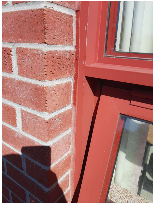
Photograph No. 2 – Red sealant on the exterior perimeter of the windows was sampled and found to be non-asbestos. Sampling also confirmed the sealants as non-PCB.
