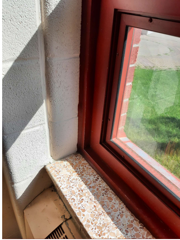
Photograph No. 1 – Red sealant on the interior perimeter of the windows was sampled and found to be non-asbestos. Sampling also confirmed the sealants as non-PCB.
