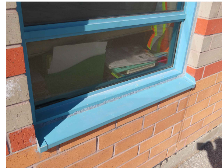
PHOTO 15: TYPICAL VIEW OF DETIORATING SEALANTS AT EXISTING WINDOWS TO BE REPLACED.
