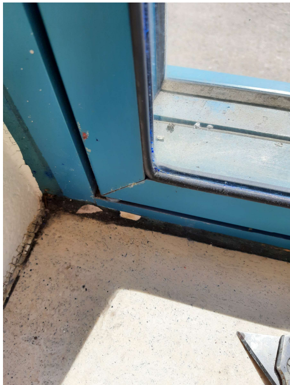
Photograph No. 2 – Black sealant on the interior side of the window was sampled and found to be non-asbestos and non-PCB.
