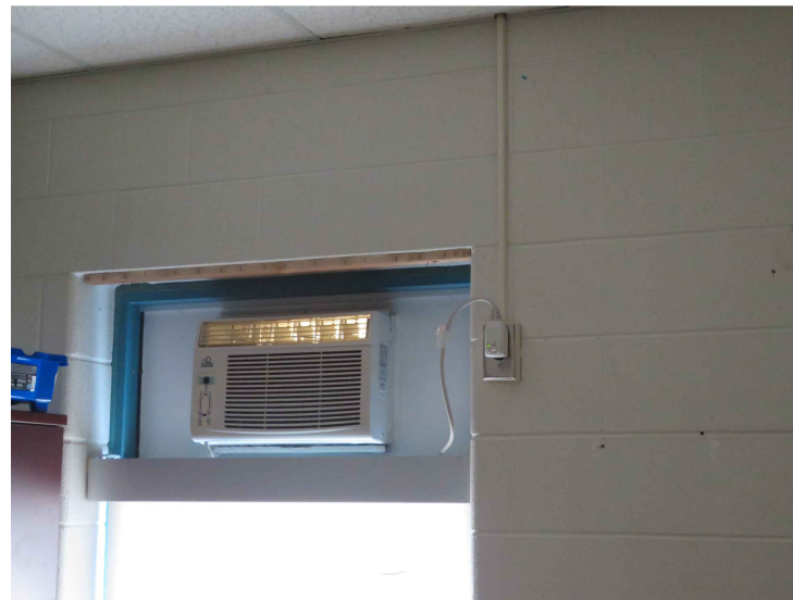
PHOTO 14: TYPICAL VIEW OF EXISTING A/C UNIT AND OUTLET.
