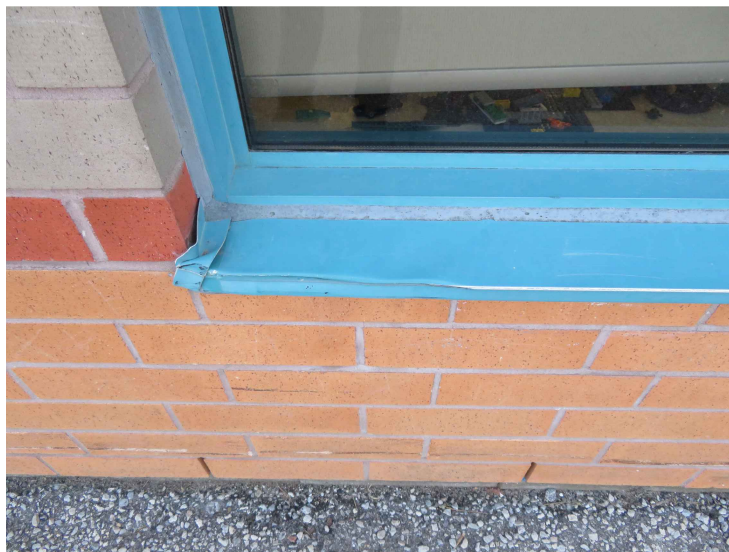
PHOTO 16: TYPICAL VIEW OF DAMAGED METAL FLASHINGS AT SILL.
