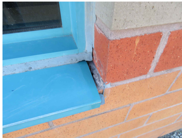
PHOTO 17: TYPICAL VIEW OF MISSING UPTURN FLASHING AT EXISTING WINDOW.
