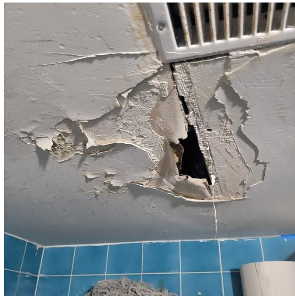
Photos 1, 2: View of water-damaged drywall ceiling.
