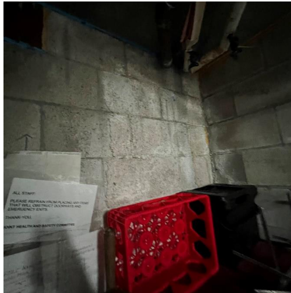
Photos 3, 4: View of water-damaged concrete block wall.
