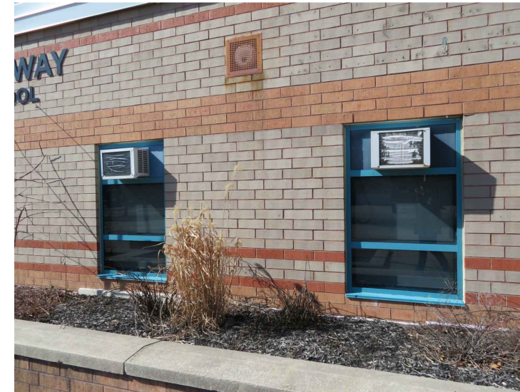
PHOTO 15: EXTERIOR VIEW OF EXISTING A/C UNITS TO BE REMOVED AND DISPOSED.
