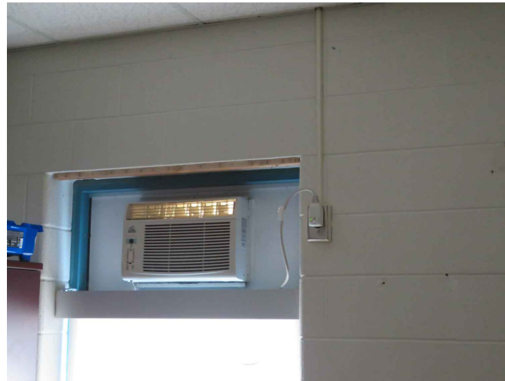
PHOTO 14: TYPICAL VIEW OF EXISTING A/C UNIT TO BE DISPOSED AND EXISTING OUTLET.
