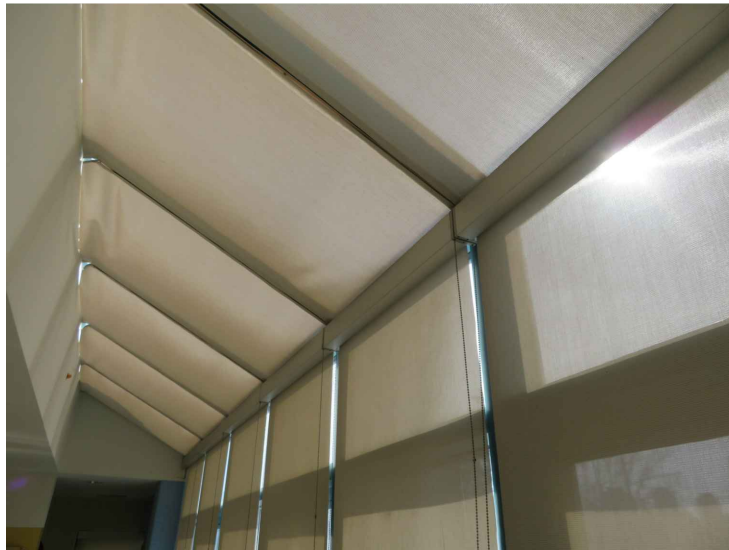
PHOTO 13: ADDITIONAL VIEW OF EXISTING SOLARIUM (W06) INTERIOR CONDITIONS.
