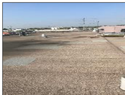
Roof top AC uninsulated, South roof section.
