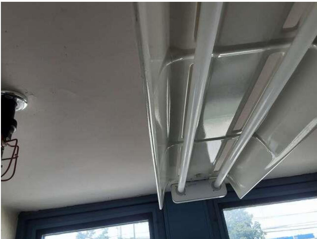
Mercury, V9000(Yes), LIGHT FIXTURE, T8, Sprinkler Room (Location #: 49).
