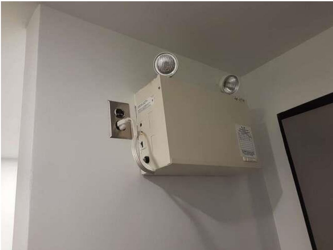
Pb Products, V9000(Yes), BATTERIES IN EMER. LIGHTS, Men's Washroom (Location #: 31).
