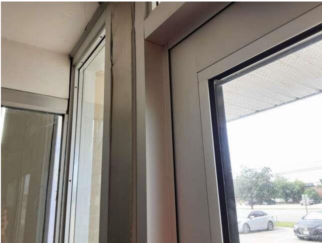
V0000 (None), Black butyl sealant, Other, Door, Caulking, Entrance Vestibule (Location #: 48).
