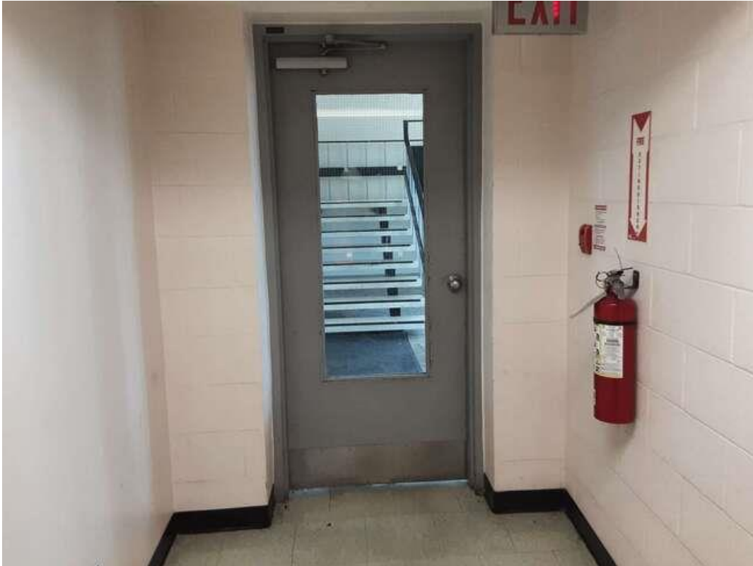
V0007(Lead, None), Light grey on door, Other, Corridor Men's (Location #: 47). 4 doors, including elevator door
