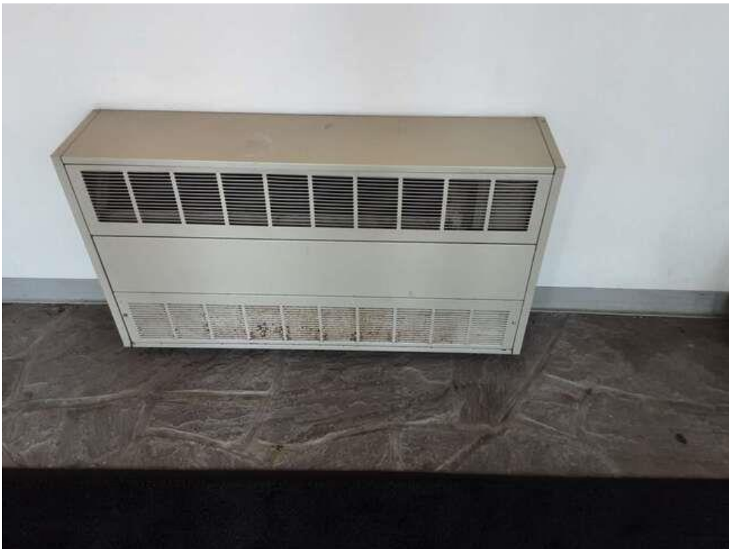
V0000 (None), Mechanical Equipment, Unit Heater, Not Insulated, Entrance Vestibule (Location #: 48).
