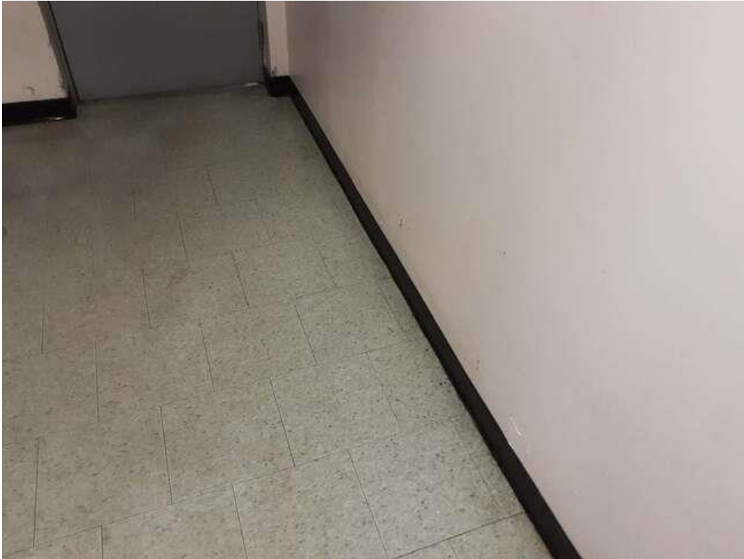
S0035A (None), Light yellow, Wall, Base, Mastic, Corridor Men's (Location #: 47). 4" black baseboard.
