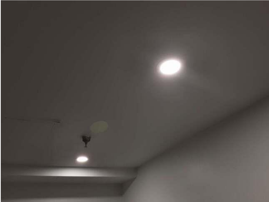
Mercury, V0000(No), LIGHT FIXTURE, LED, Men's Washroom (Location #: 31).
