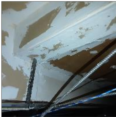
Non-asbestos drywall joint compound on the ceiling above acoustic ceiling tiles, Open Office Area (Loc. 27).
