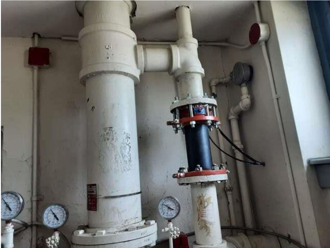
V0000 (None), Piping, Not Insulated, Sprinkler Room (Location #: 49).
