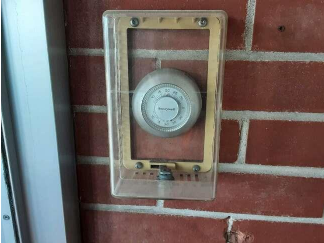
Mercury, V9000(Yes), THERMOSTAT, Entrance Vestibule (Location #: 48).
