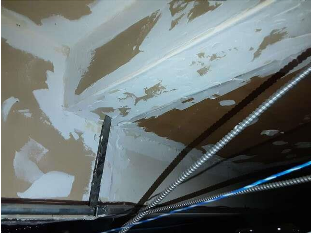
S0032D (None), Ceiling, Drywall and joint compound, Open Office Area (Location #: 27). Above ceiling tiles.
