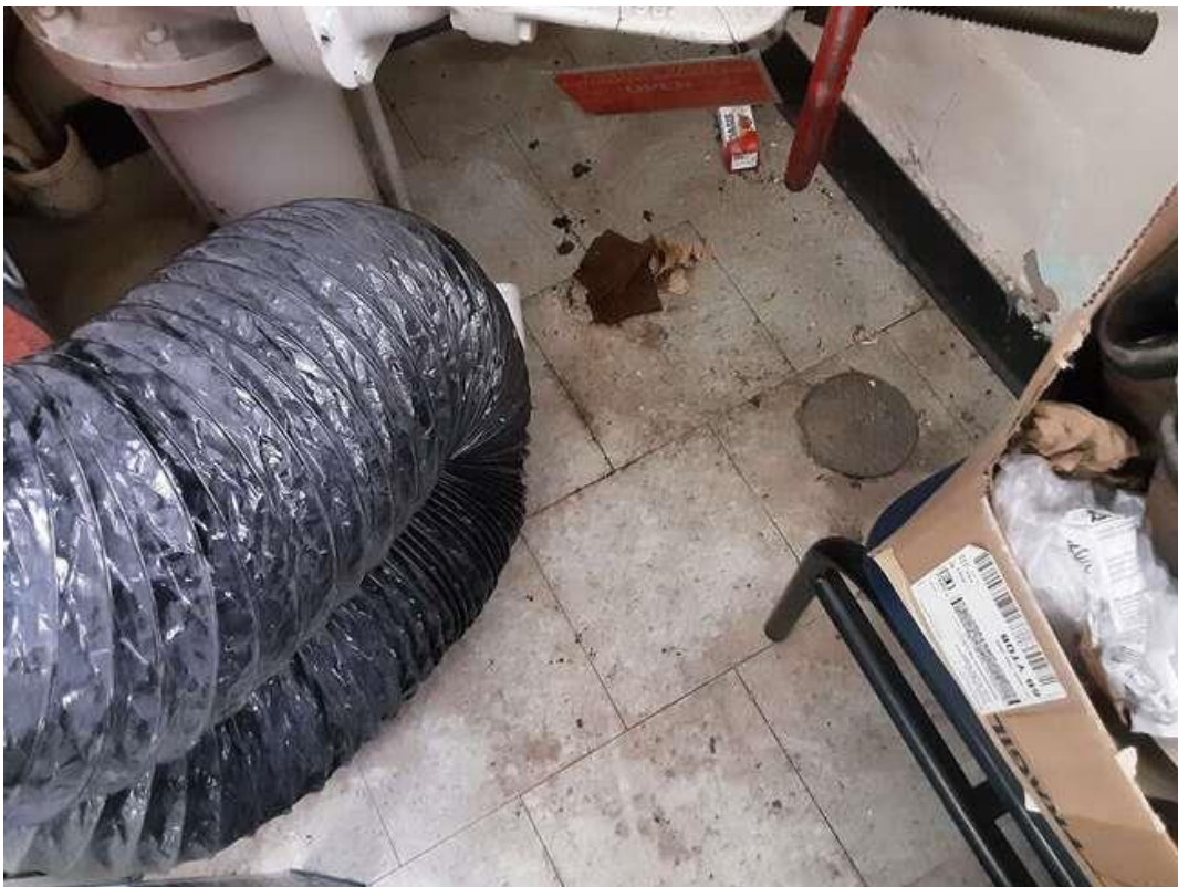
V0018 (None), 12 x 12 green with dark green flecks, Floor, All, Vinyl Floor Tile and Mastic, Sprinkler Room (Location #: 49).
