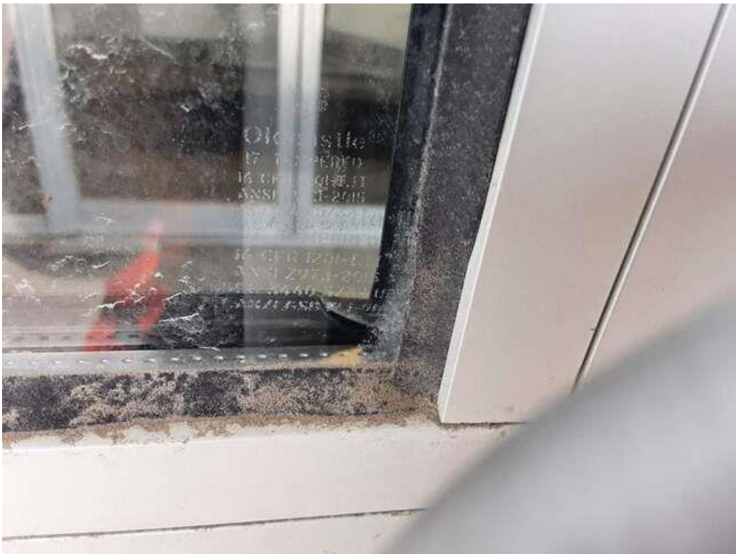
V0000 (None), Black butyl sealant, Other, Door, Caulking, Entrance Vestibule (Location #: 48). 2015 installed door
