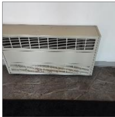
Uninsulated unit heater, Entrance Vestibule (Loc. 48).
