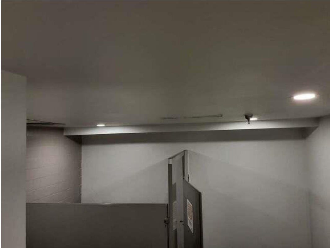
V0016 (None), Ceiling, Drywall and joint compound, Men's Washroom (Location #: 31).
