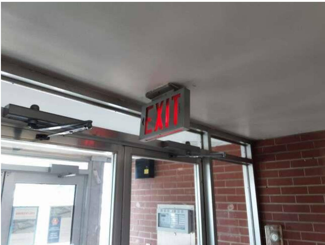
Pb Products, V9500(Presumed), BATTERIES IN EMER. LIGHTS, Entrance Vestibule (Location #: 48).
