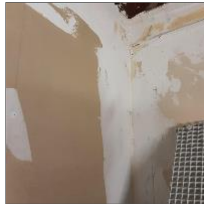
Non-asbestos drywall joint compound on wall finishes, Elevator Pit (Loc. 50).
