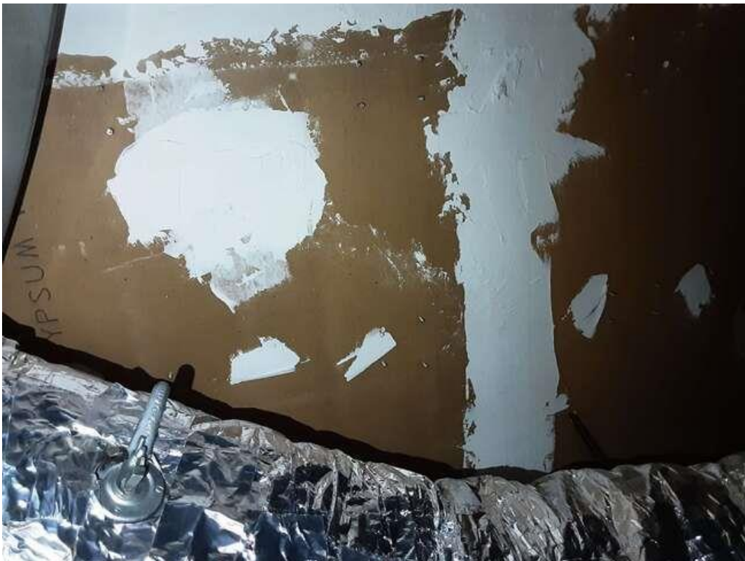
S0032C (None), Ceiling, Drywall and joint compound, Men's Washroom (Location #: 31). Above ceiling tiles.
