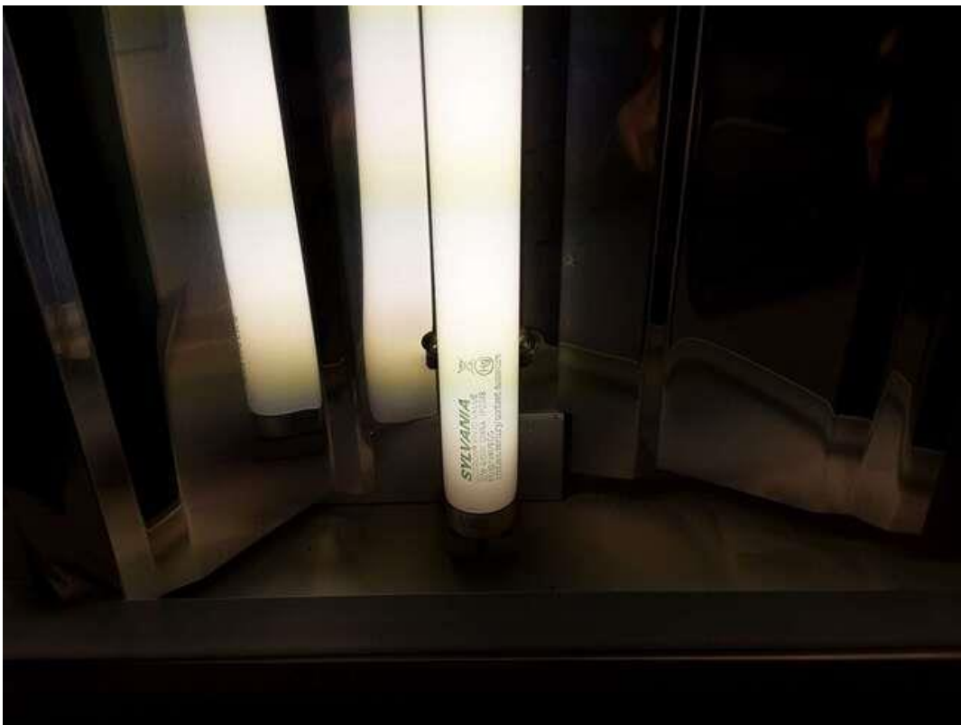
Mercury, V9000(Yes), LIGHT FIXTURE, T8, Corridor Men's (Location #: 47).
