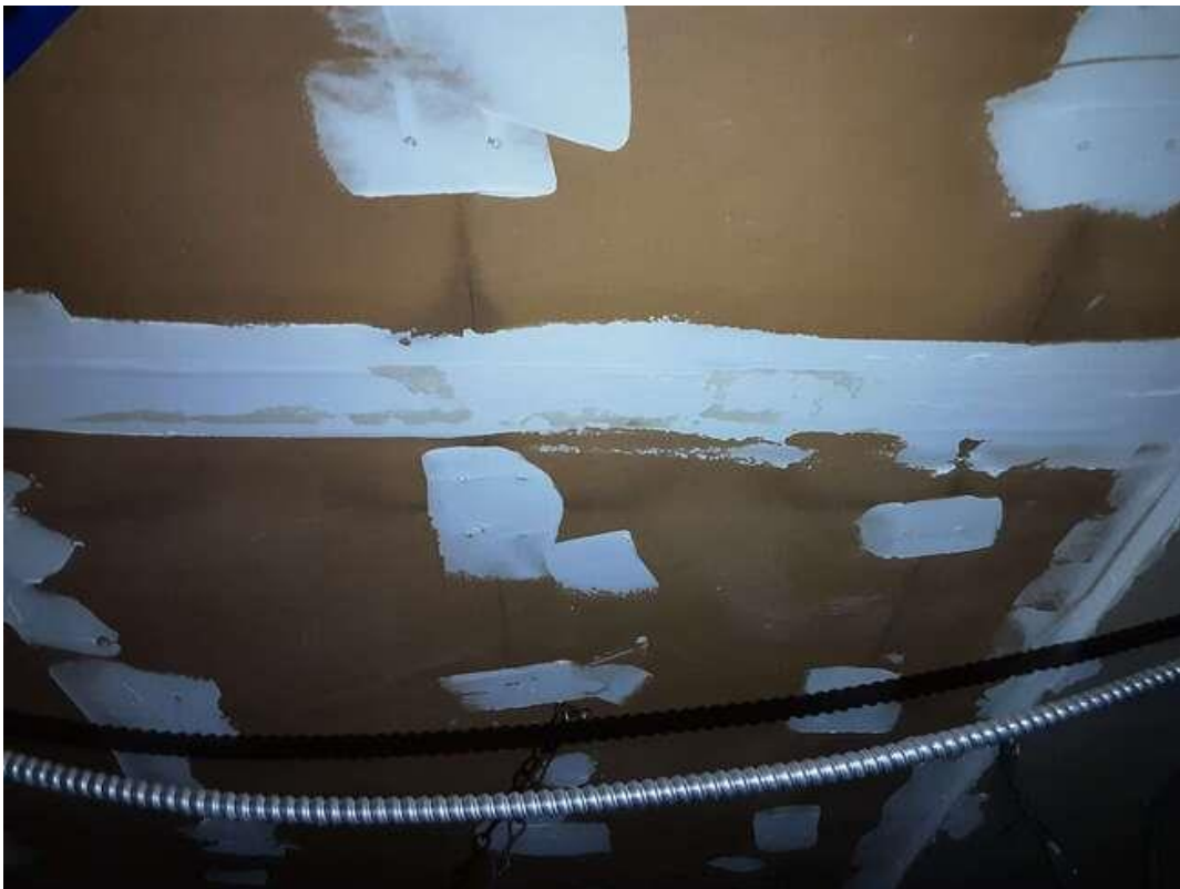
S0032A (None), Ceiling, Drywall and joint compound, Open Office Area (Location #: 27). Above ceiling tiles
