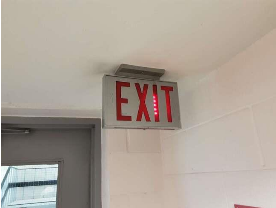
Pb Products, V9500(Presumed), BATTERIES IN EMER. LIGHTS, Corridor Men's (Location #: 47).
