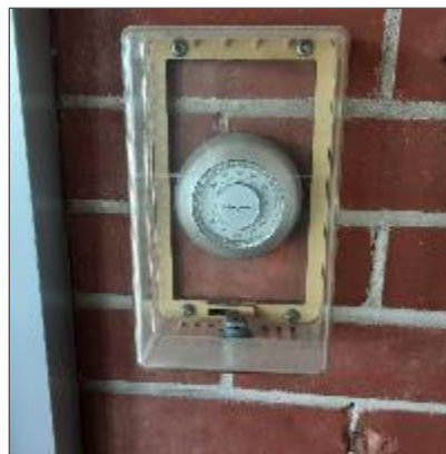
Thermostat with mercury-containing ampule, Entrance Vestibule (Loc. 48)
