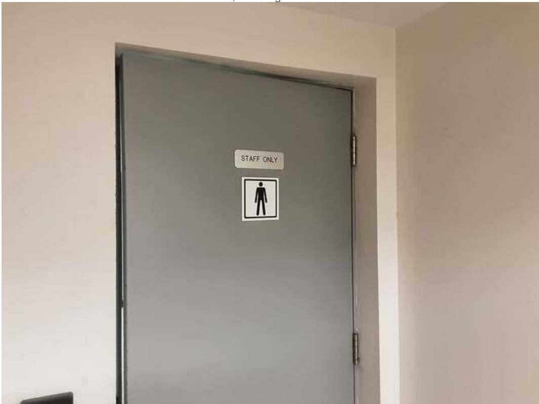
V0007(Lead, None), Light grey on door, Other, Corridor Men's (Location #: 47). 4 doors, including elevator door
