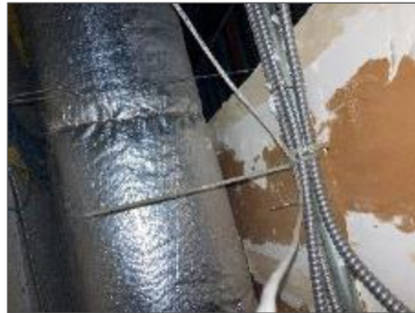
Non-asbestos fibreglass insulated duct, Open Office Area (Loc. 27).
