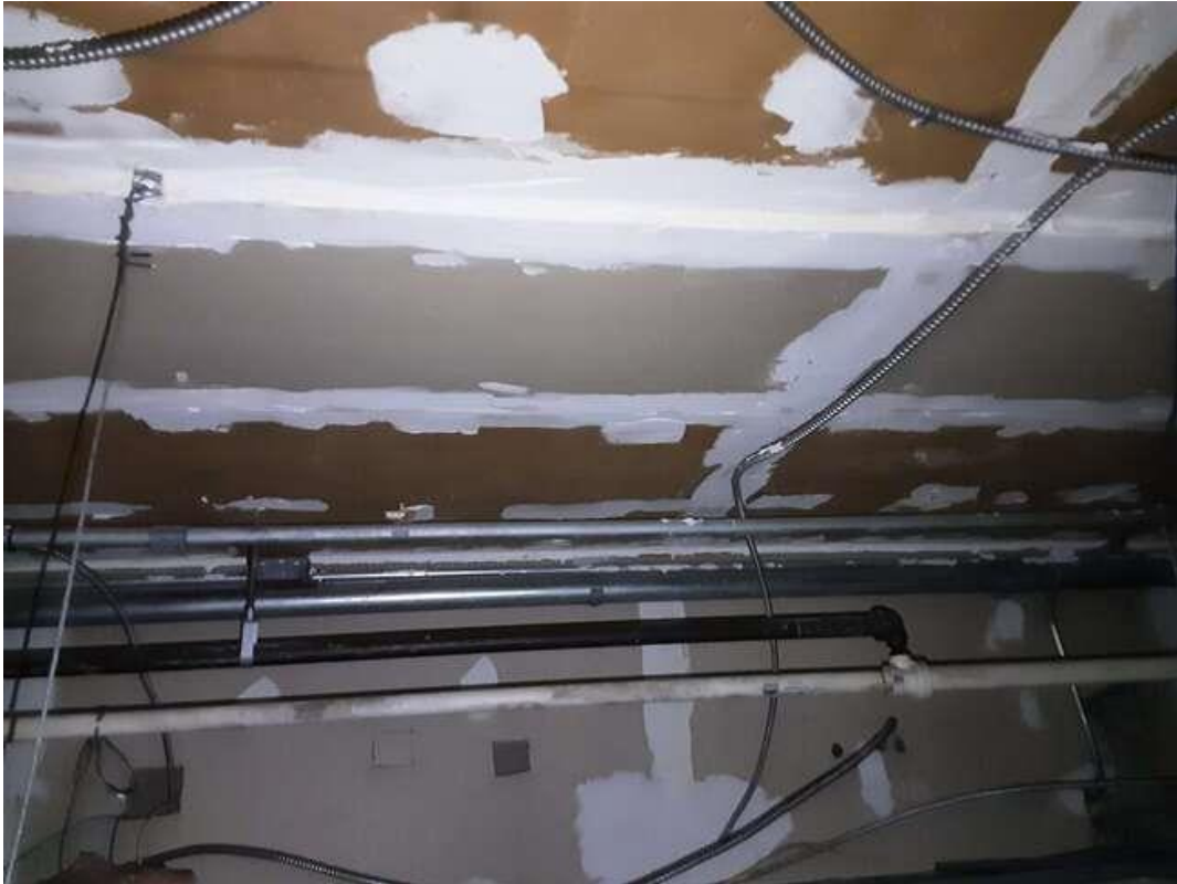
S0032A (None), Ceiling, Drywall and joint compound, Open Office Area (Location #: 27). Above ceiling tiles
