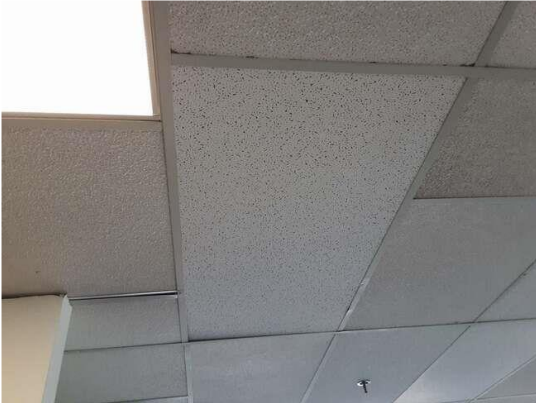
V0000 (None), 24x48 small fissures and pinholes, Ceiling, Ceiling Tiles (lay-in), Open Office Area (Location #: 27). Dated 01/03/14.
