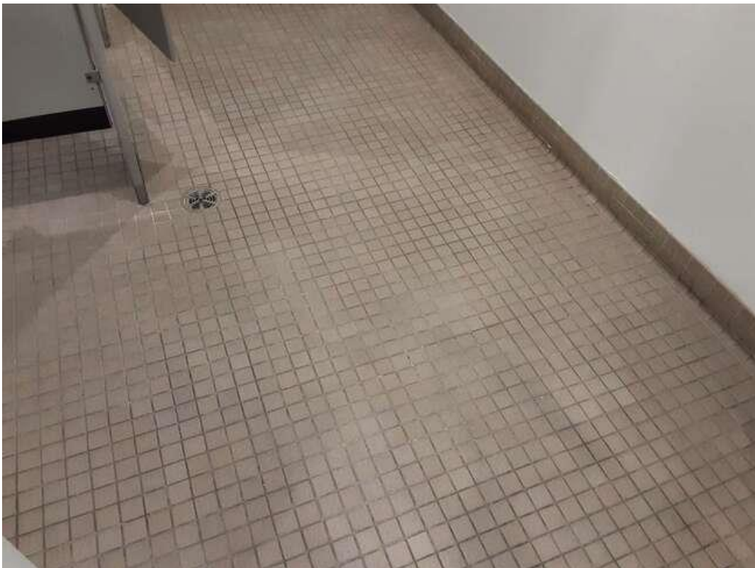
V0000 (None), 2x2 beige ceramic tile, Floor, Ceramic Tiles, Men's Washroom (Location #: 31).
