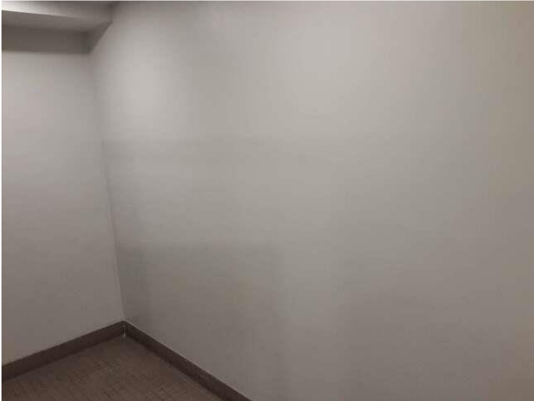
V0020 (None), Partition wall, Wall, Drywall and joint compound, Men's Washroom (Location #: 31).
