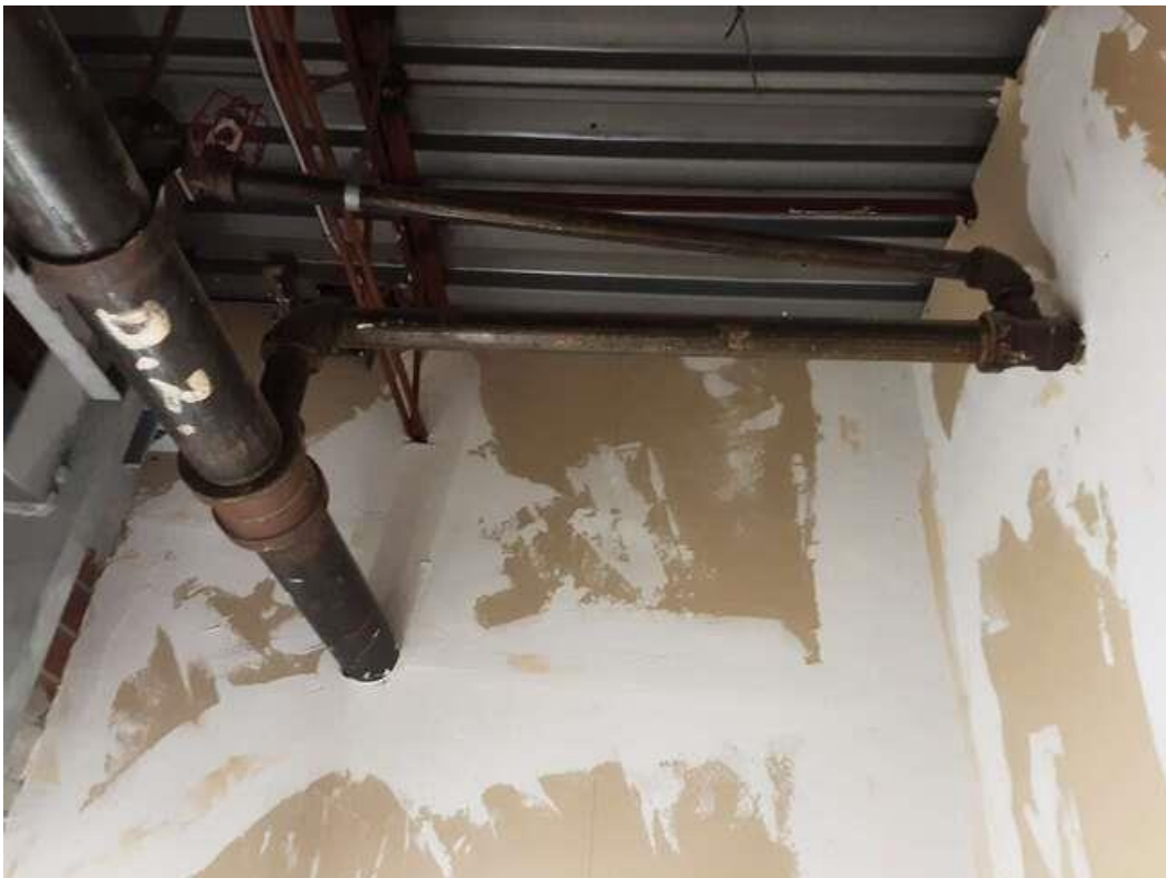
V0000 (None), Piping, All, Not Insulated, Elevator Pit (Location #: 50).
