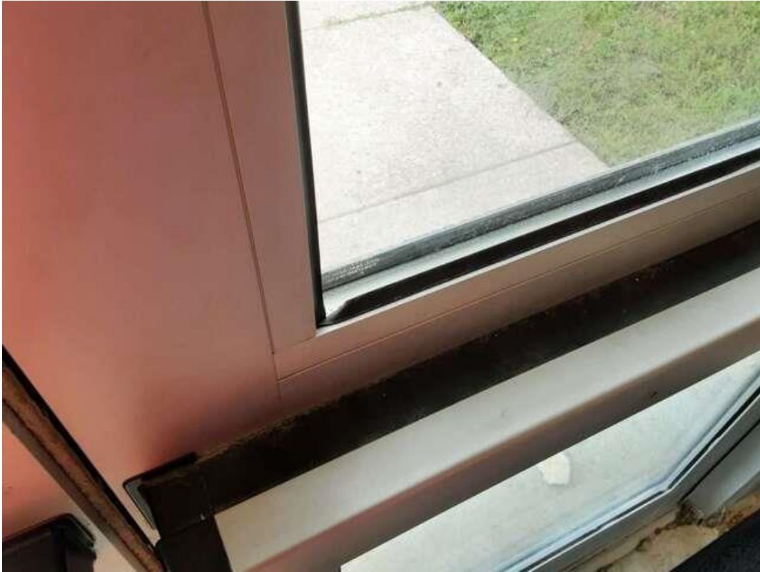
V0000 (None), Black butyl sealant, Other, Door, Caulking, Entrance Vestibule (Location #: 48). 2015 installed door
