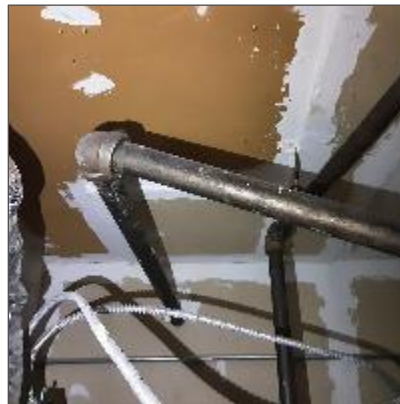
Non-insulated piping, Open Office Area (Loc. 27).
